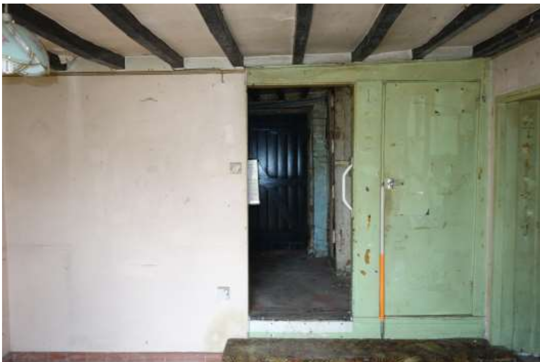
Plate 19: View looking W showing interior of dining room with exposed ceiling joists
