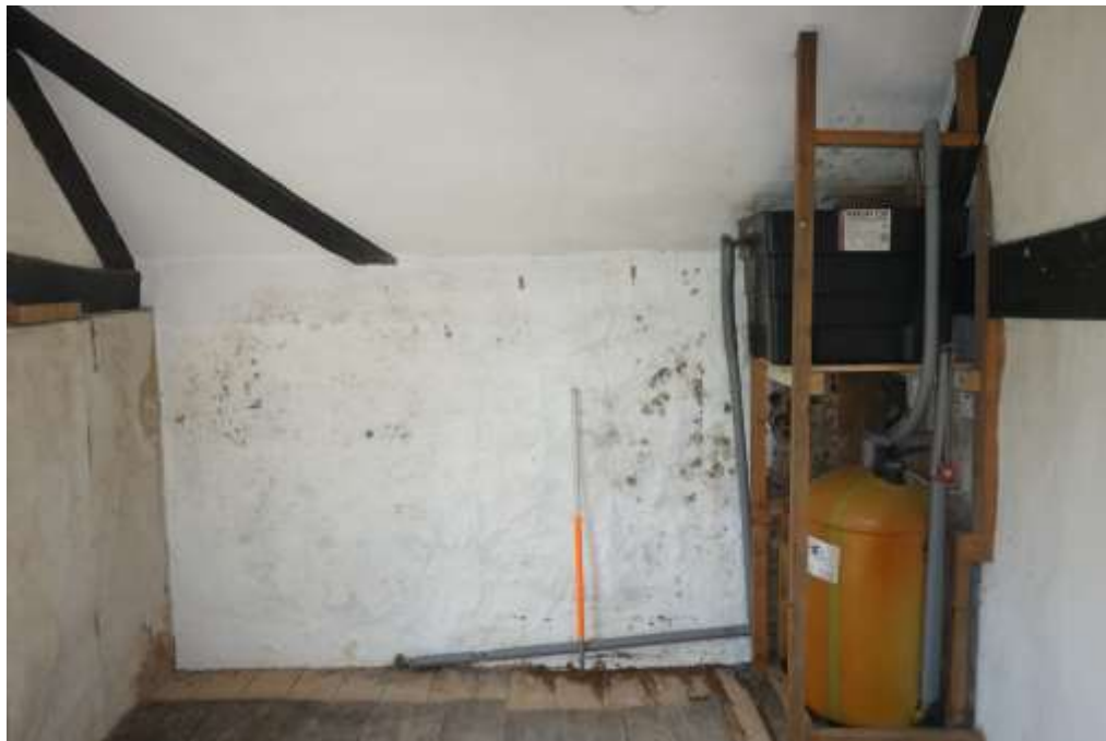
Plate 39: View S showing interior of first floor SE bedroom with planked floor and modern boiler in SW corner of room
