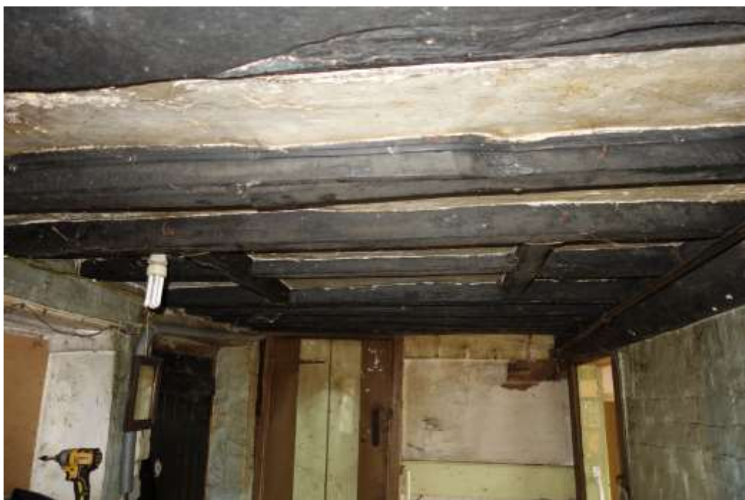
Plate 13: Internal view looking N showing detail of exposed ceiling joists and hatch in ceiling of entrance lobby
