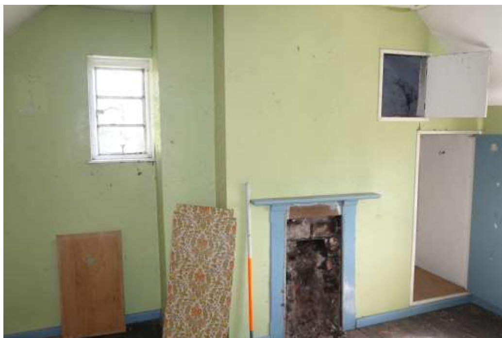
Plate 41: View looking N showing interior of master (NE) bedroom on first floor, with central fireplace flanked by cupboard to right and modern casement window to left
