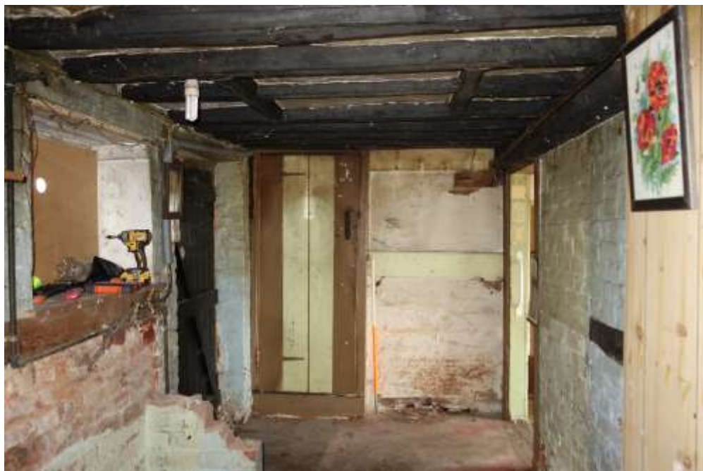
Plate 12: Internal view looking N towards staircase in ground floor lobby with exposed ceiling joists and blocked hatch in ceiling
