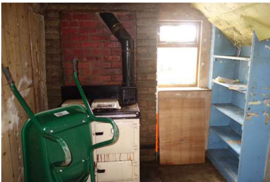
Plate 15: Internal view of kitchen looking E showing renewed brickwork in E wall to left of window
