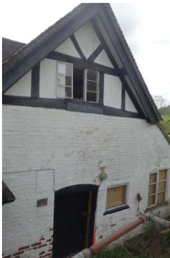
Plate 3: View looking ESE showing W gable of crosswing with segmental arched door and exposed timber framing in the apex of the gable
