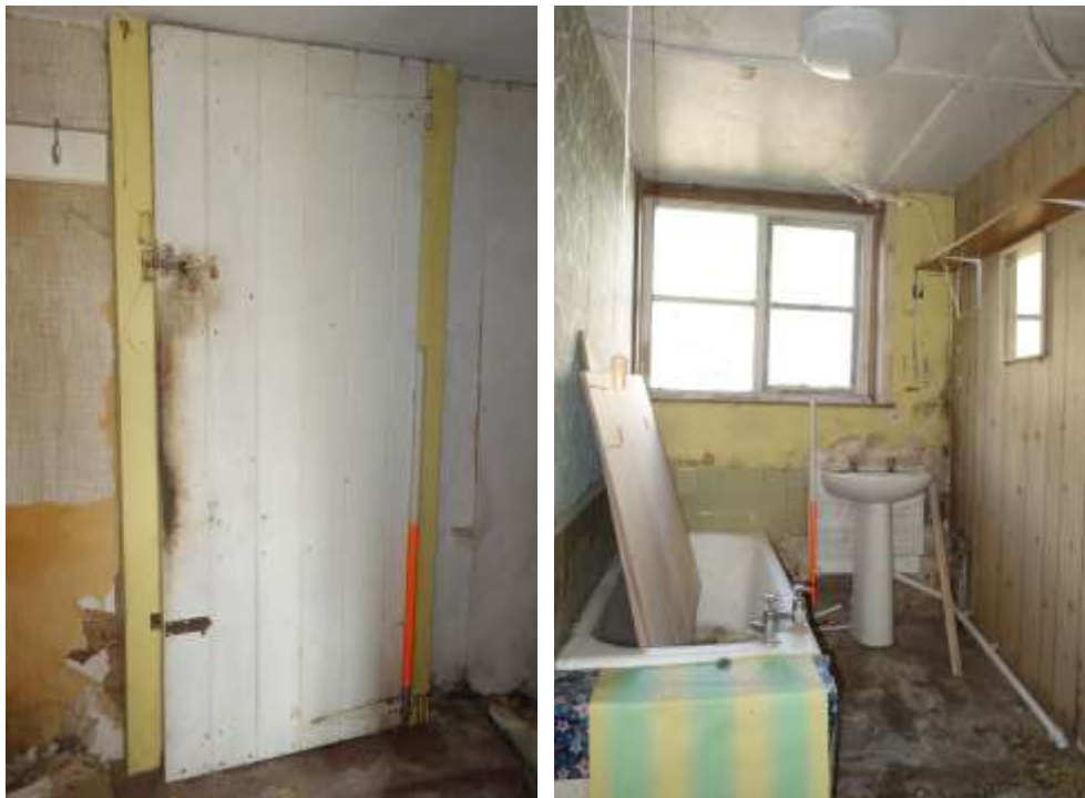
Plate 27: View looking W showing plank and batten door leading to bathroom extension Plate 28: View looking W showing interior of bathroom lit by casement window
