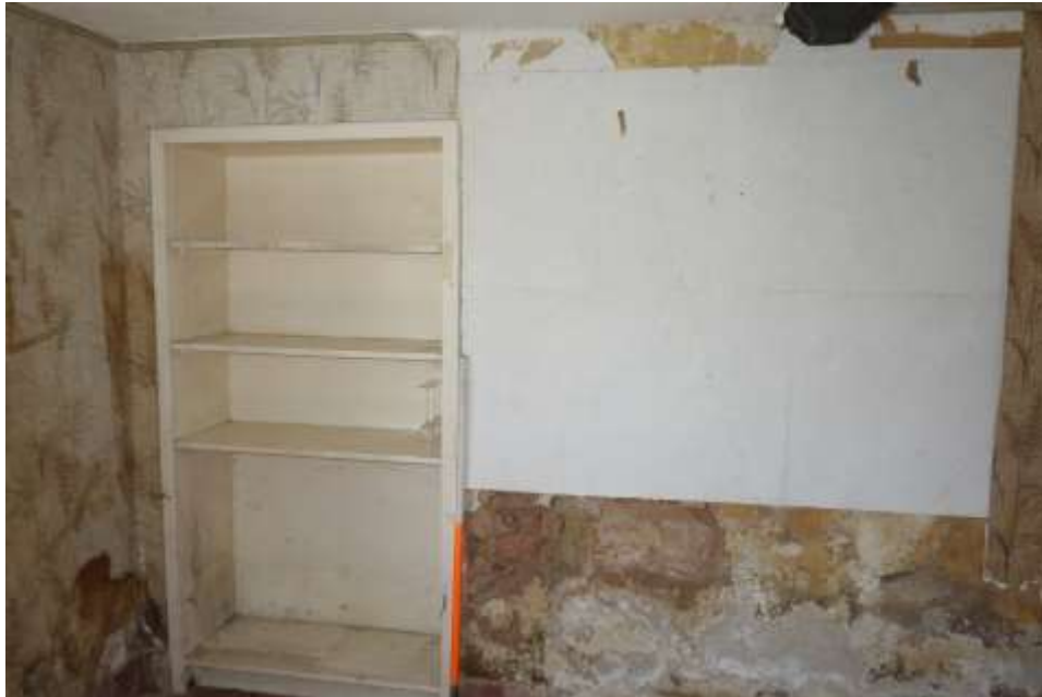
Plate 26: Internal view S showing S wall of living room with cupboard situated in recess to left of picture
