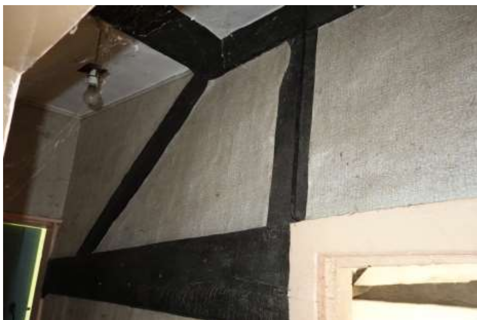
Plate 36: Internal view looking NNE showing detail of timber-framing in E wall of first floor landing
