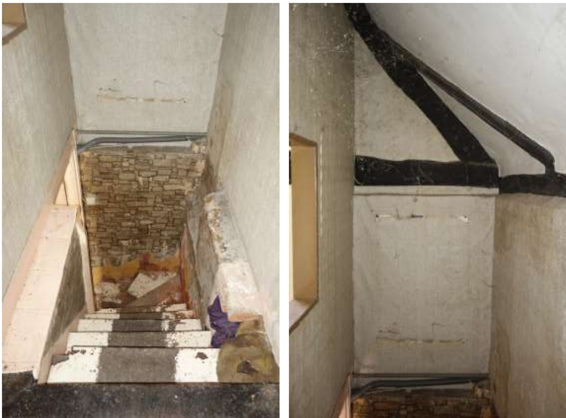
Plate 29: Internal view looking W showing detail of staircase viewed from first floor landing
