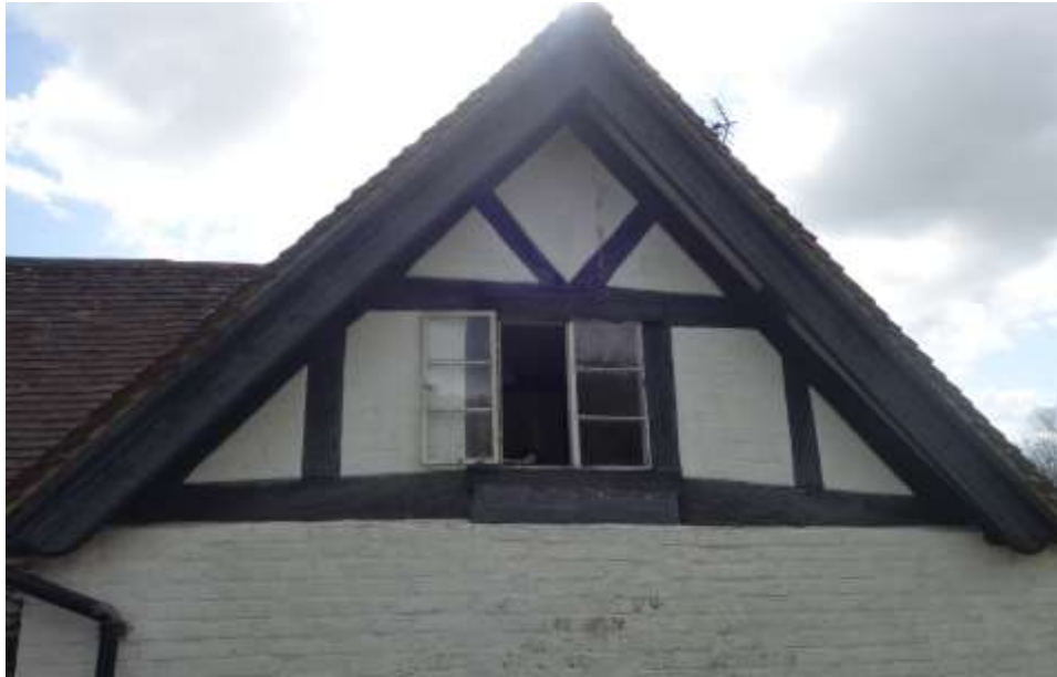
Plate 4: View looking E showing detail of exposed timber framing with brick nogging in W gable of crossing
