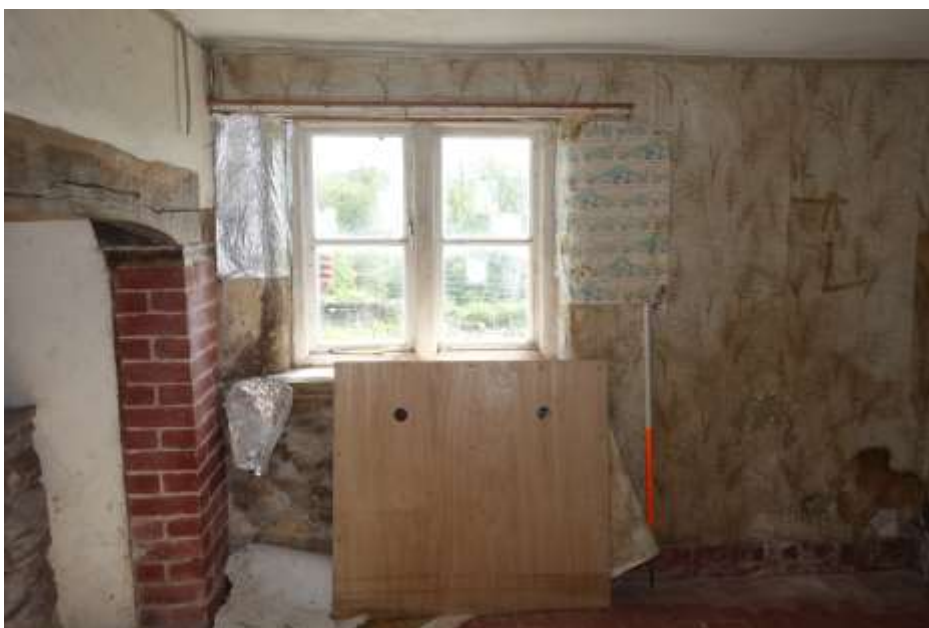
Plate 24: View looking E showing interior of living room lit by 4-pane casement window
