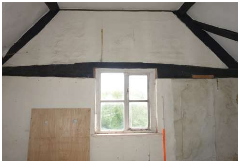
Plate 38: View E showing E wall of first floor SE bedroom with casement window inserted in exposed timber framing
