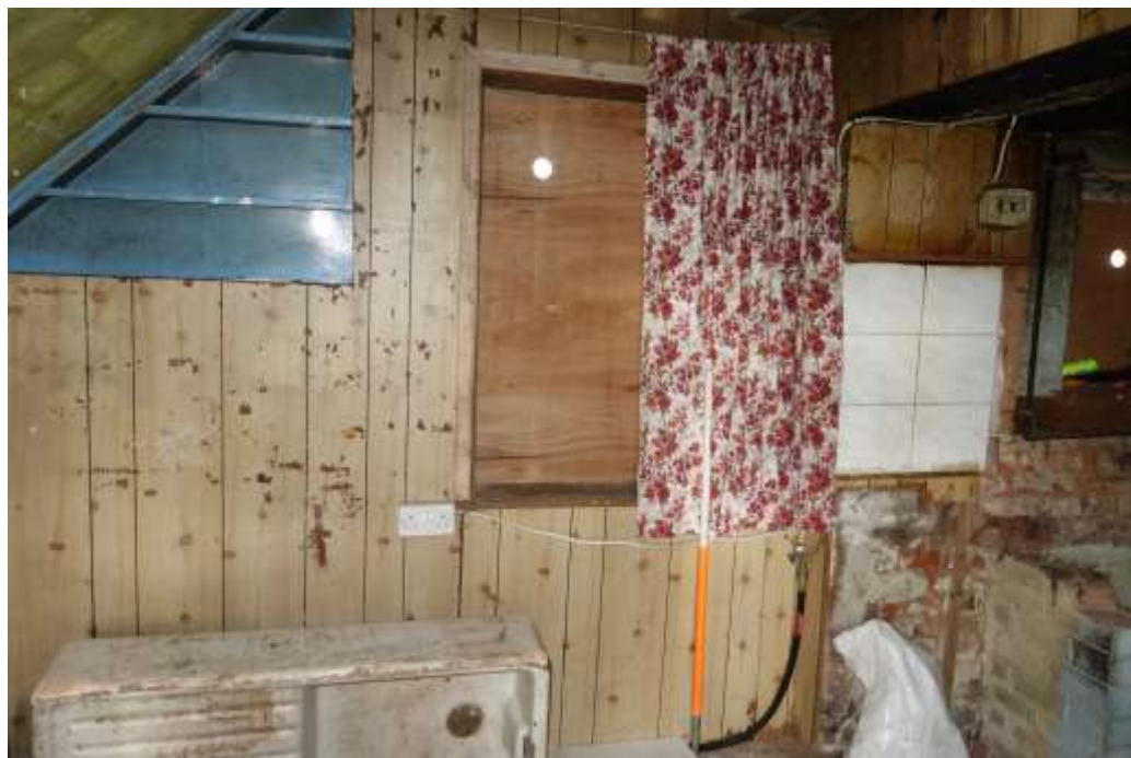
Plate 14: Internal view looking W showing W wall of kitchen extension with wooden panelling
