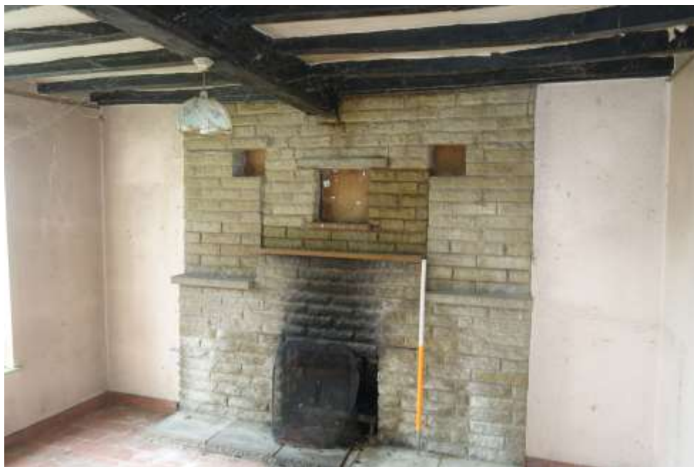
Plate 21: Internal view looking S showing fireplace in S wall of dining room with modern stone surround and exposed chamfered ceiling beam
