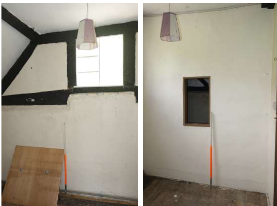
Plate 32: Internal view showing detail of timber-framing in W wall of first floor room Plate 33: Internal view looking S showing hatch in partition wall of first floor room overlooking staircase
