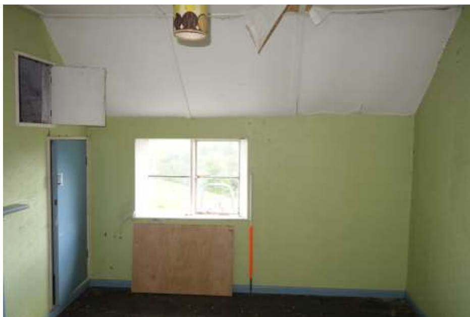
Plate 40: View E showing interior of master (NE) bedroom on first floor, lit by casement window in E wall
