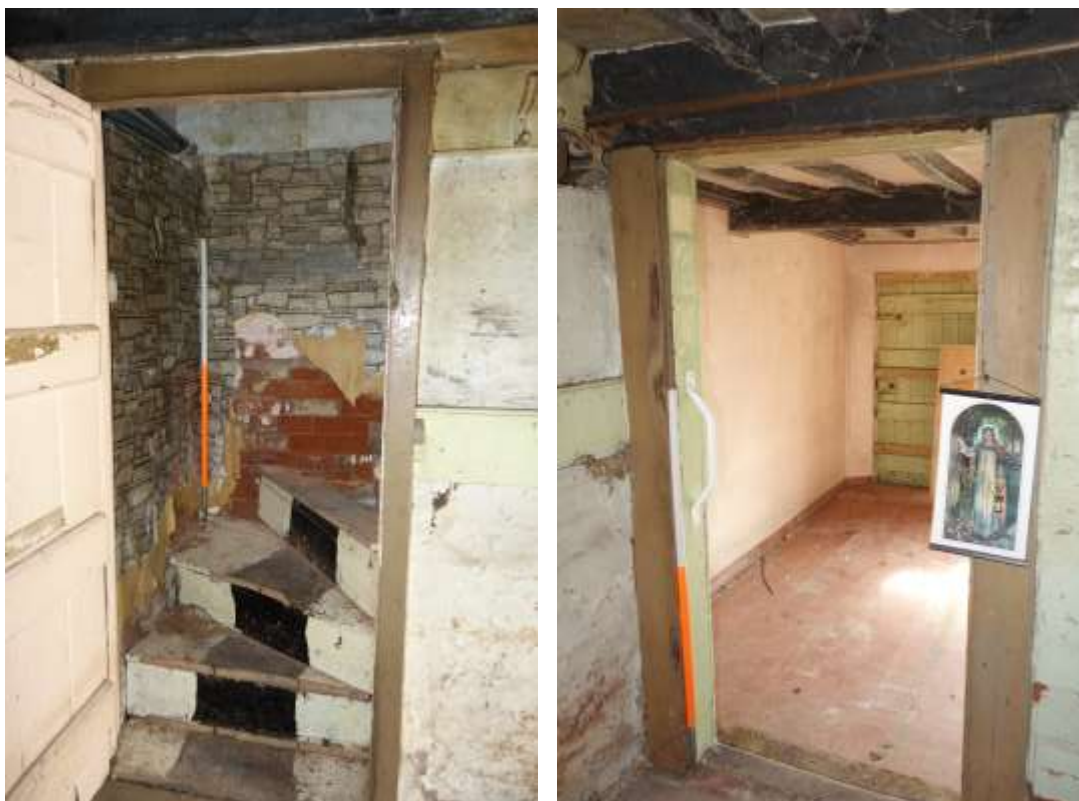
Plate 17: Internal view showing detail of wooden dog-leg staircase leading up to first floor with brickwork concealed by stone-patterned wallpaper
