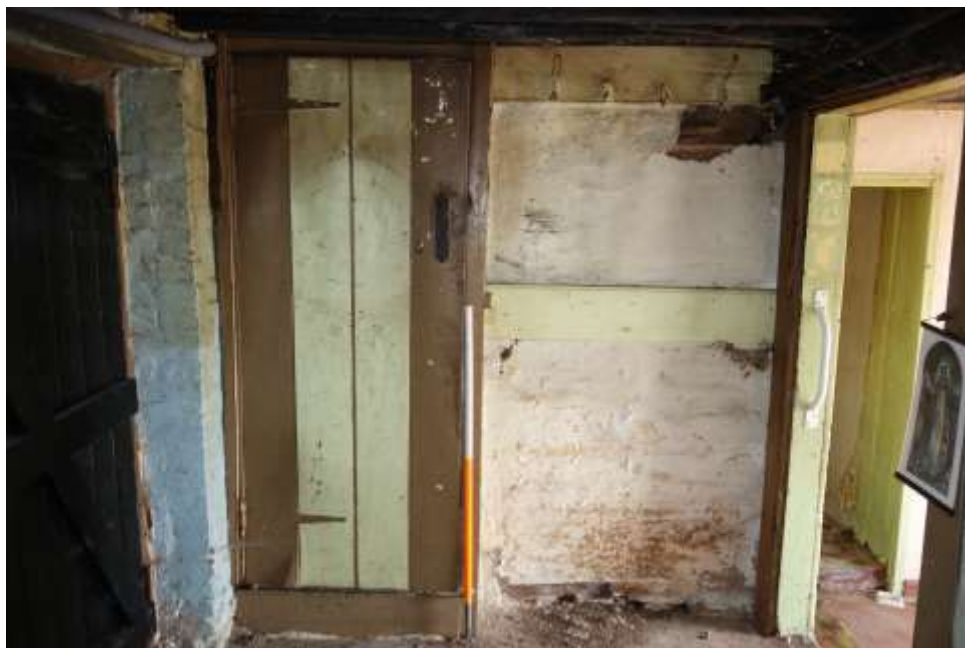
Plate 16: View looking N showing detail of narrow planked door at N end of lobby leading to stairs to first floor
