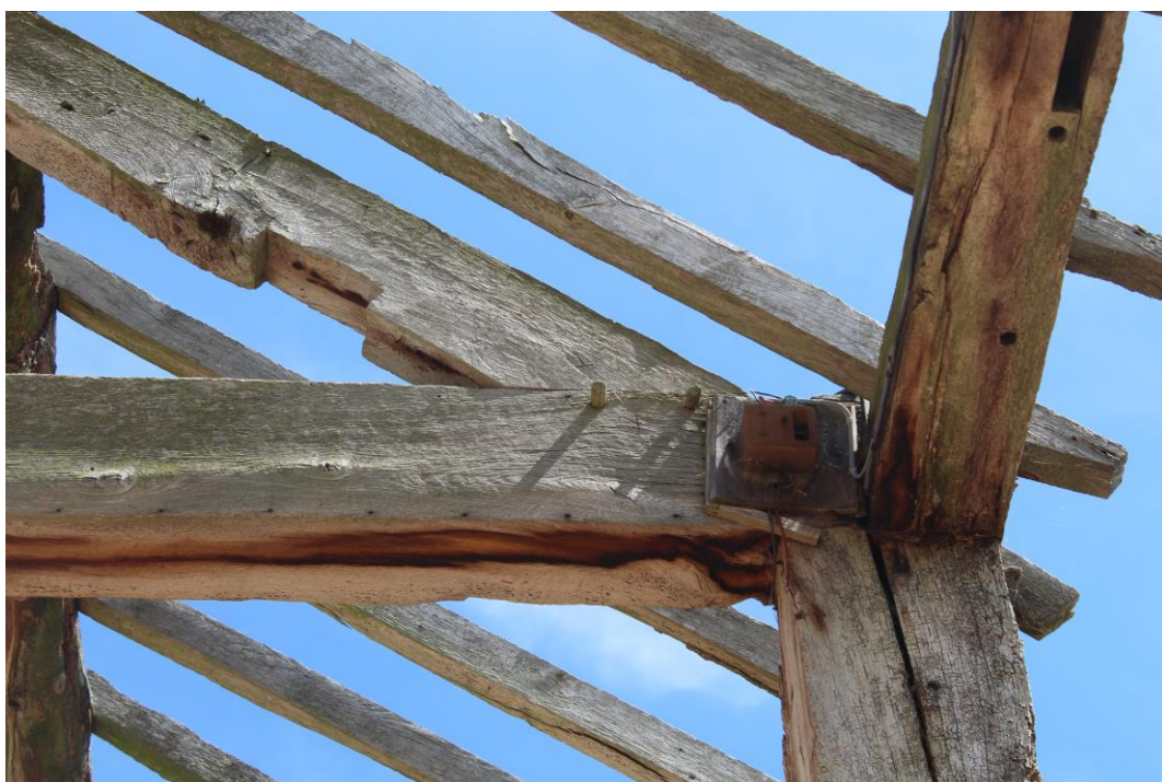
Plate 18: Internal view ESE showing the carpenters' marks on the S end of the central roof-truss
