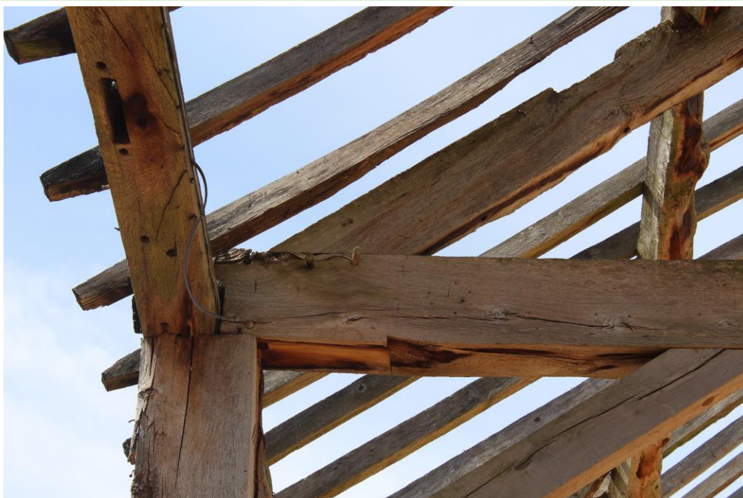
Plate 13: Internal view NE showing the carpenters' marks on the N end of the W roof-truss
