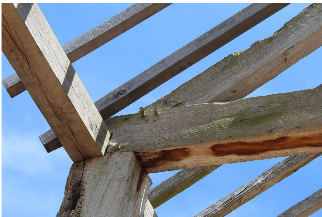
Plate 16: Internal view NE showing the carpenters' marks on the N end of the central roof-truss
