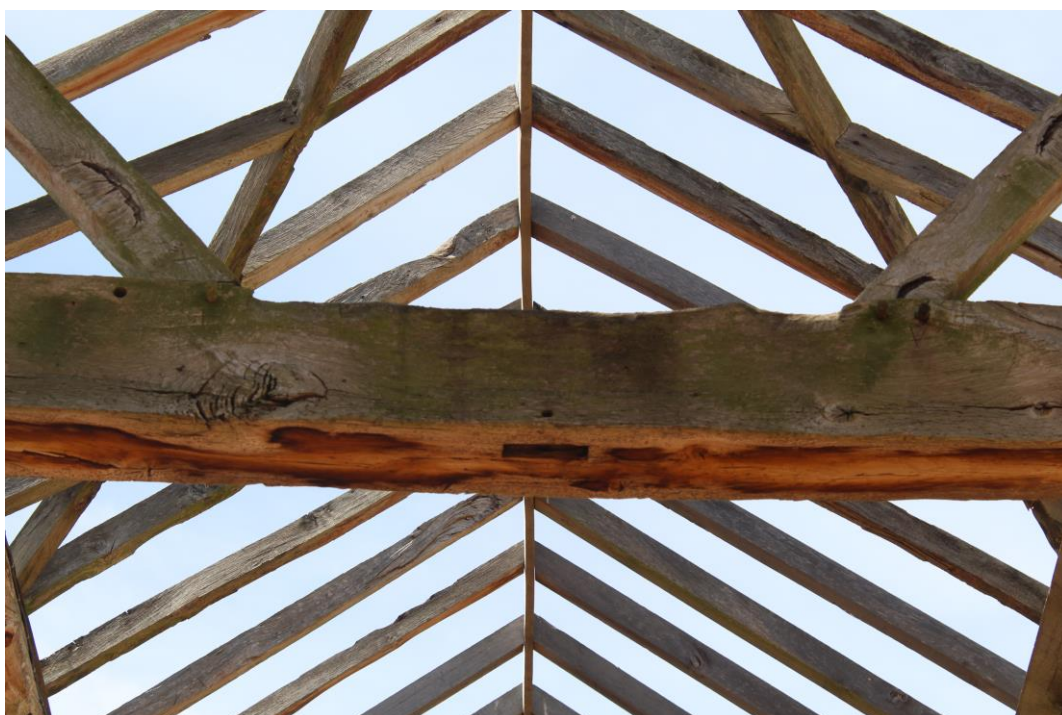
Plate 14: Internal view E showing the carpenters' marks on the central portion end of the W roof-truss
