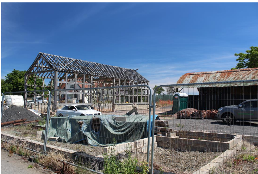
Plate 4: External view NE looking across the former courtyard towards the threshing barn
