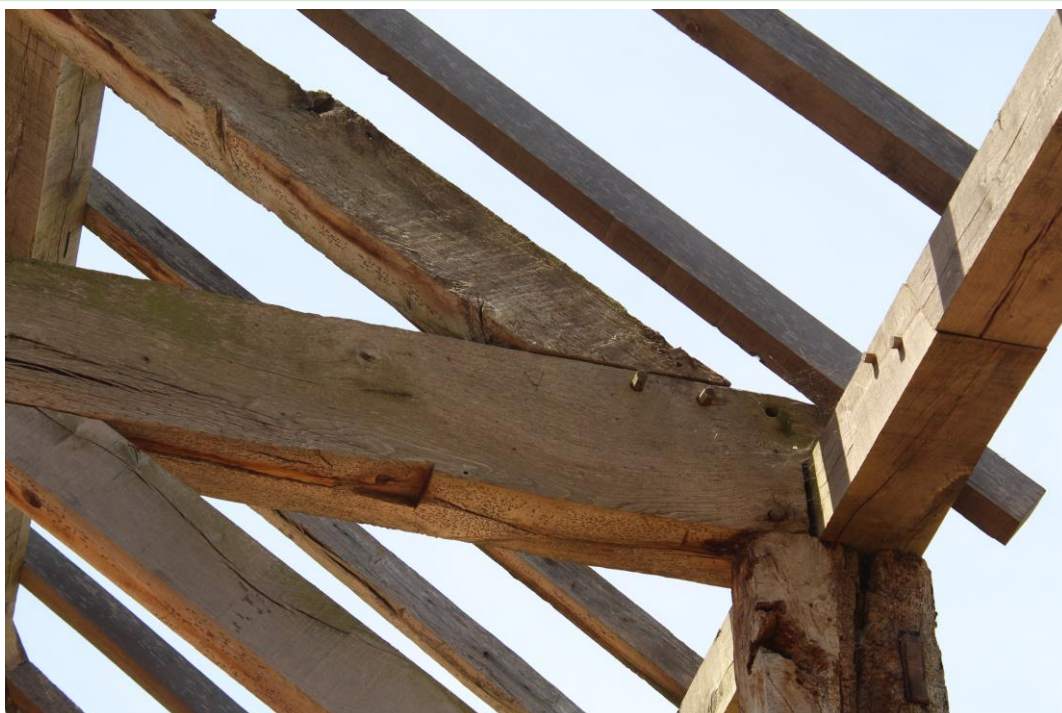
Plate 15: Internal view ESE showing the carpenters' marks on the S end of the central roof-truss
