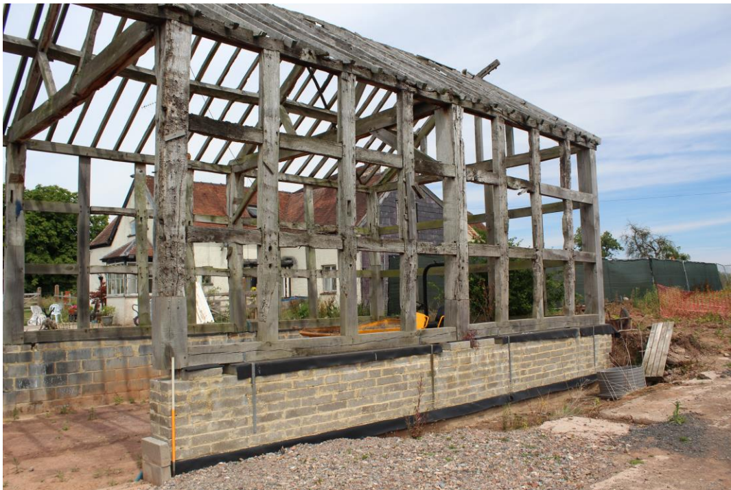
Plate 5: External view NE of the easternmost bays within the S facing section – showing low breeze block walls replacing the former masonry plinth, replacement sill plate, and butt and scarf joints within the spliced timber frames
