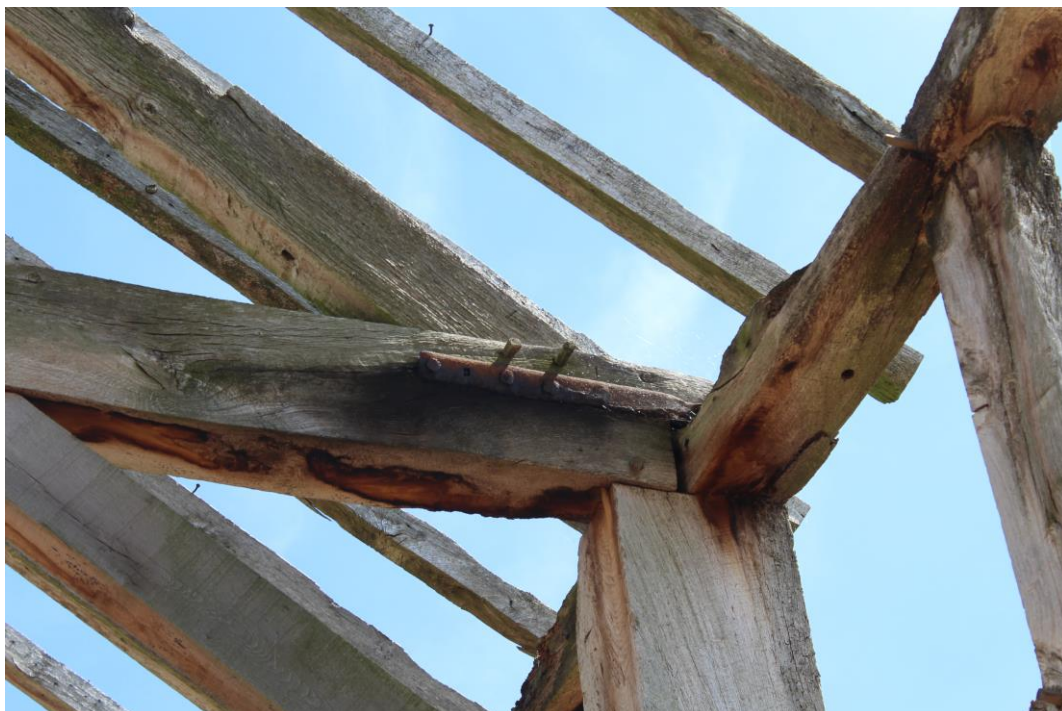
Plate 21: Internal view ESE showing the carpenters' marks on the S end of the E roof-truss
