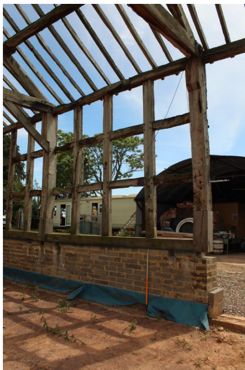
Plate 10: Representative internal view SSE showing stave-holes and slots within the historic timbers for internal subdivisions
