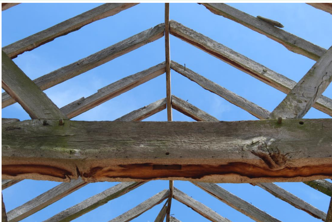
Plate 17: Internal view E showing the carpenters' marks on the central portion end of the central roof-truss
