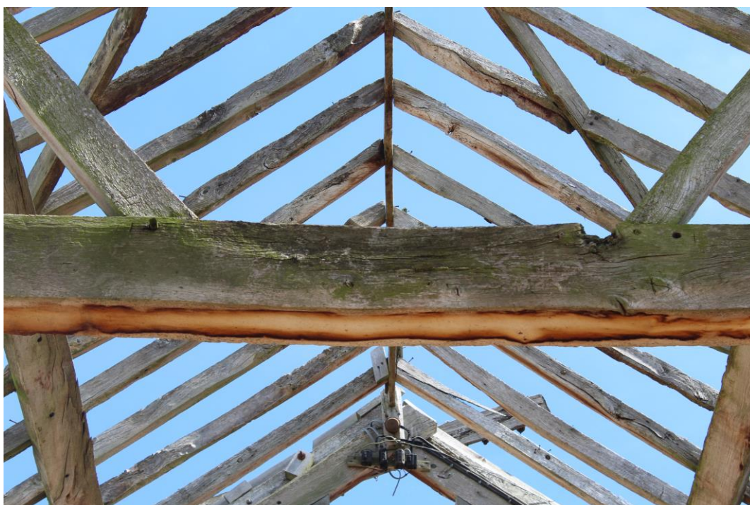
Plate 20: Internal view E showing the carpenters' marks on the central portion end of the E roof-truss
