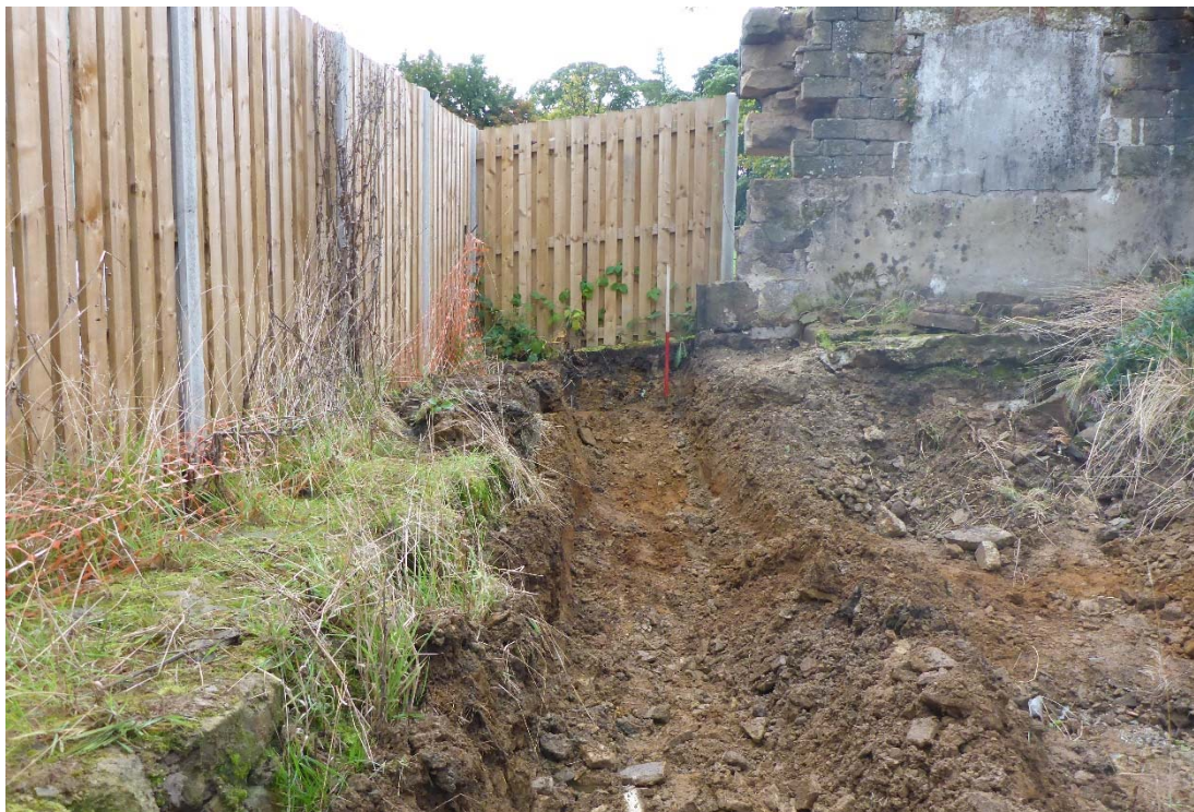
Plate 1: Monitored foundation trench adjacent to property boundary and former stone foundations, viewed facing south
