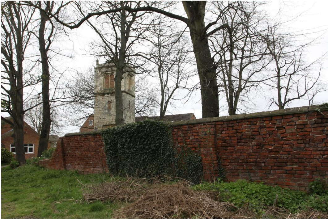
Plate 4 Interior view of wall showing lean and condition
