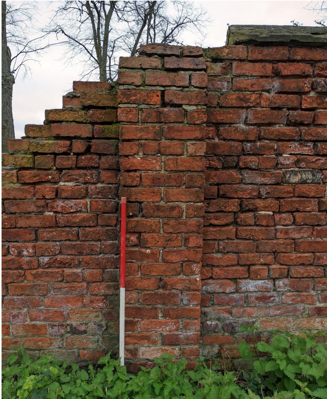
Plate 2 interior face of wall showing buttress and condition
