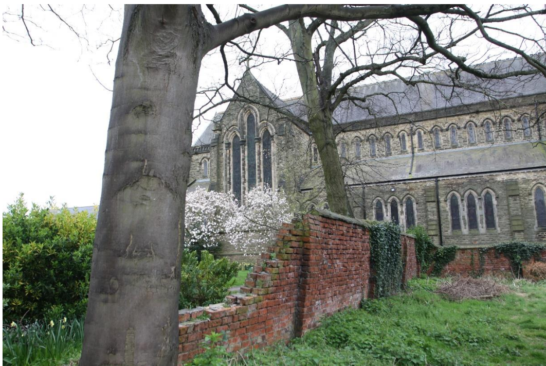
Plate 1 Interior view of wall showing condition and lean; St. Lawrence Church in background
