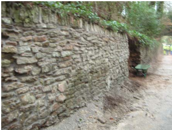
Chewton Mendip West Wall: Section of grouted and 'repointed' wall in foreground. Collapsing section (beside wheelbarrow) had to be removed and is awaiting rebuilding once the sewer trench work was clear
