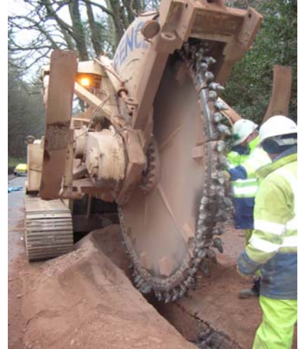
Wessex Water's trench cutting machine being checked over prior to recommencing excavation through the rock underlying the road surface
