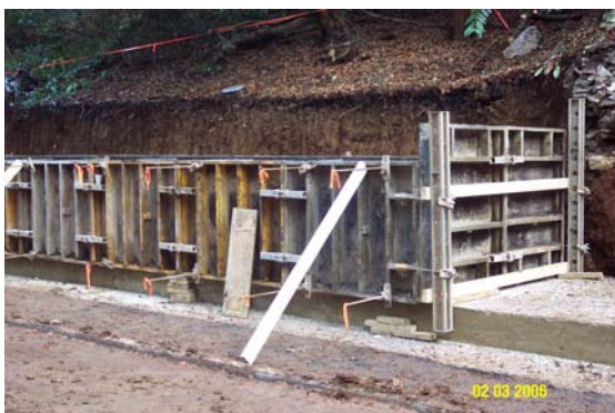
'Formwork' fixed in before concrete pour on one of the north east wall sections
