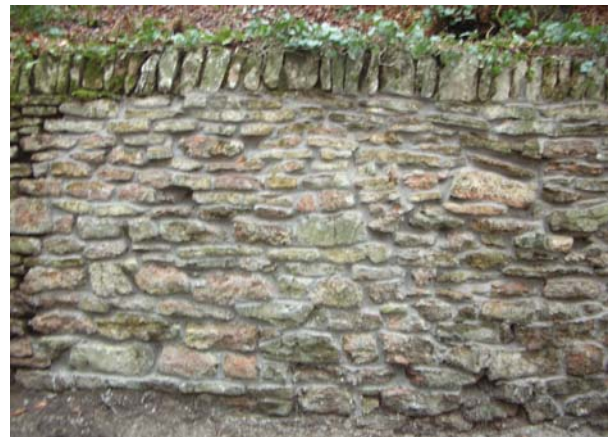
Detailed view of a section of wall after completion of grouting and 'repointing' work
