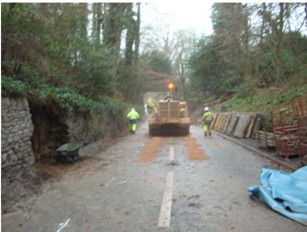
View north towards footbridge showing Wessex Water's trench cutting machine progressing south towards Bathway
