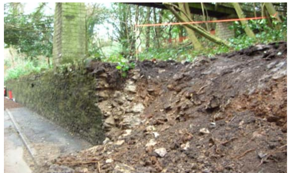
Chewton Mendip N.E. Wall. Demolition of wall, stone recovery and tree removal
