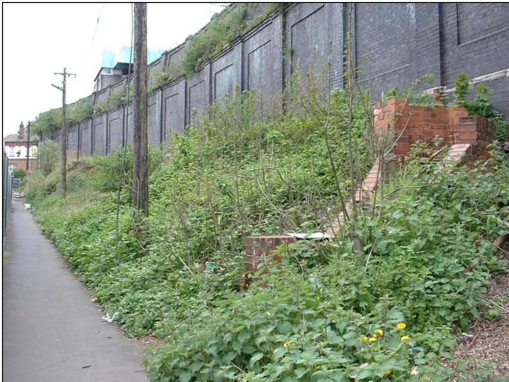
Plate 1 Retaining Wall for the High Level Station with the shelters at its base
