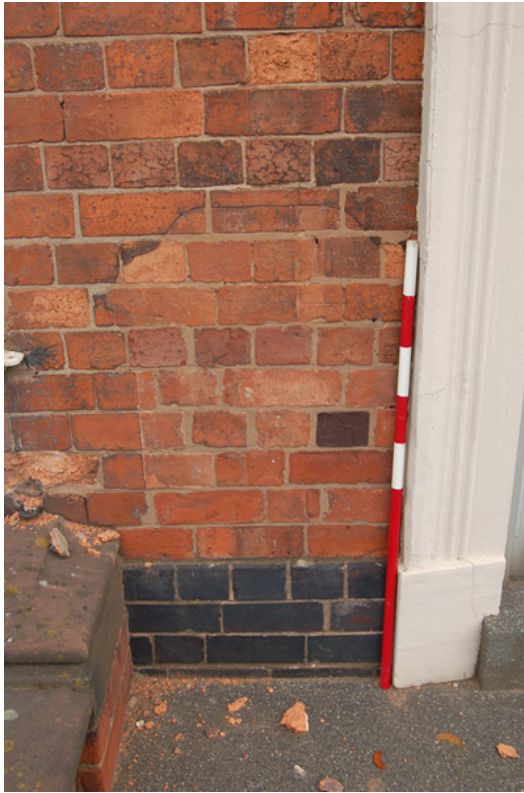
Plate 3: 'Ghost' of former porch pedestal.
