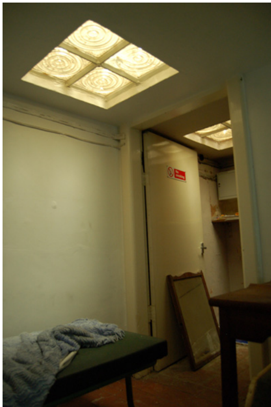
Plate 12: Glass tiles lighting G14 and basement stair.
