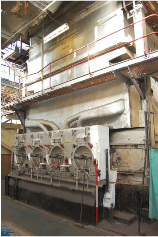
Plate 40: Building 21F; Boiler 7.
