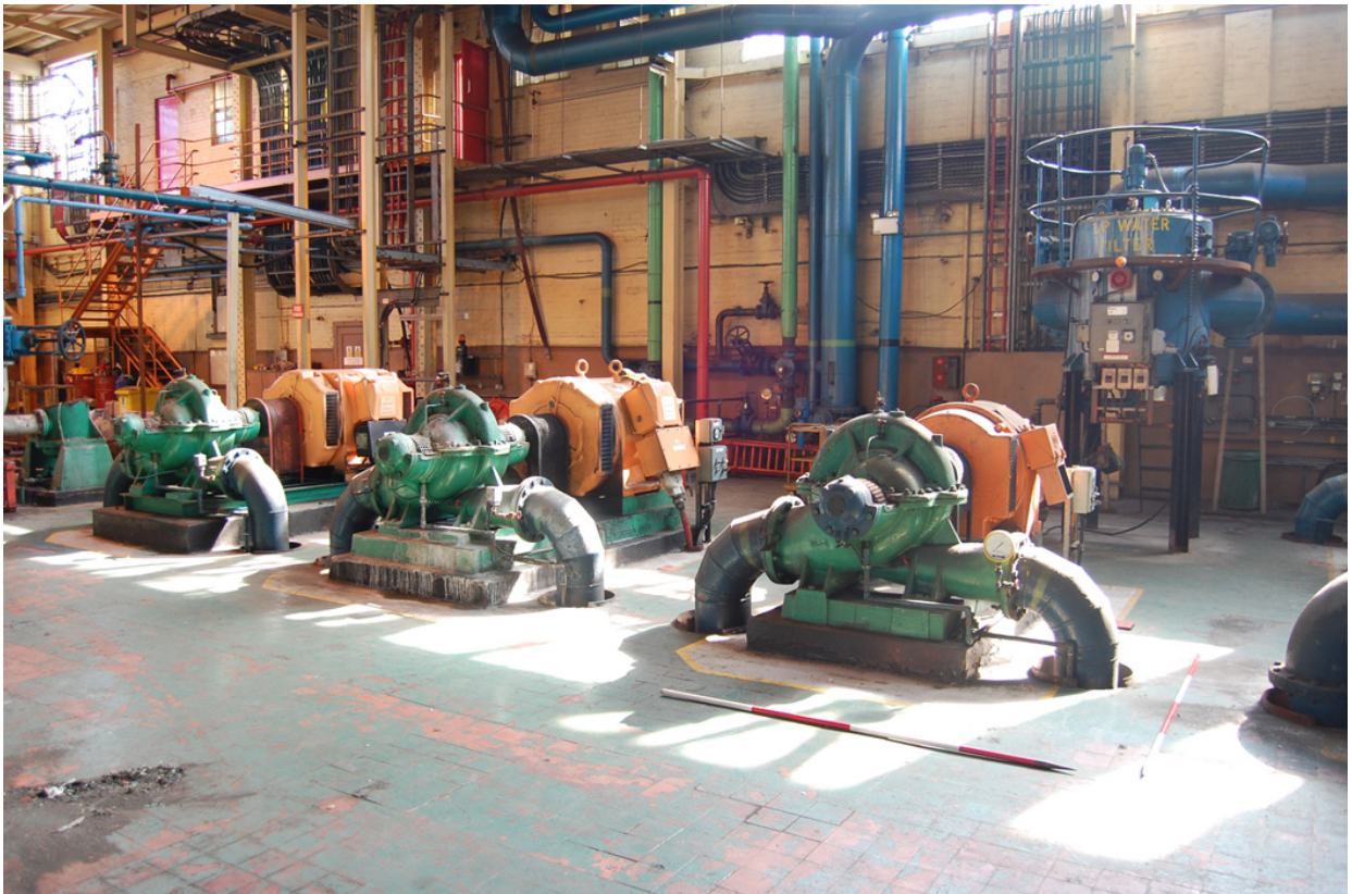
Plate 70: Low pressure water pumps (foreground) and filter (blue) within Building 22.
