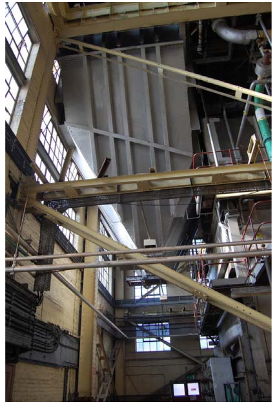
Plate 41: Building 21F; hopper feeding Boiler 7.
