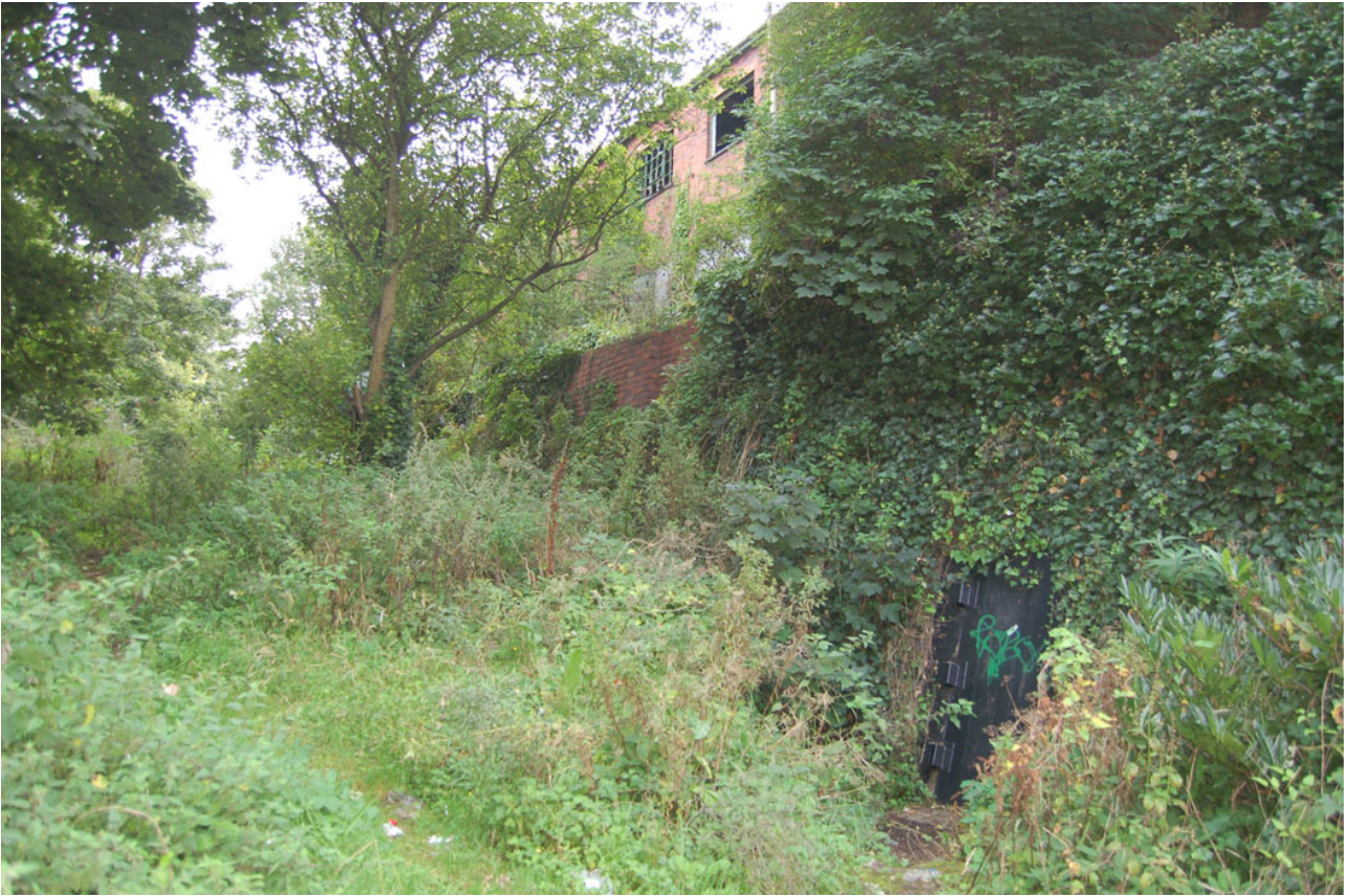
Plate 5: Blocked doorway to cavern complex (right) within retaining wall to west side of car park.
