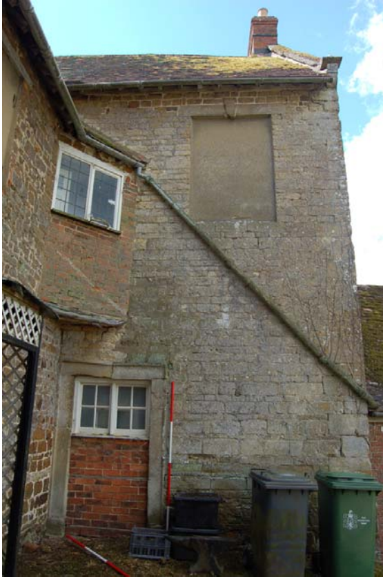
Plate 17: Blocked openings in north wall of south extension, note angled passage to left 1F level above blocked door.
