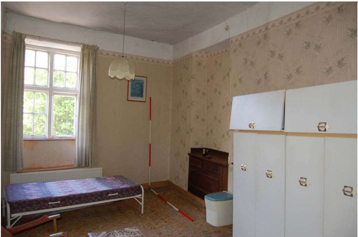
Plate 51: Room [1F07] looking south-west; note cupboard within blocked window of west wall.
