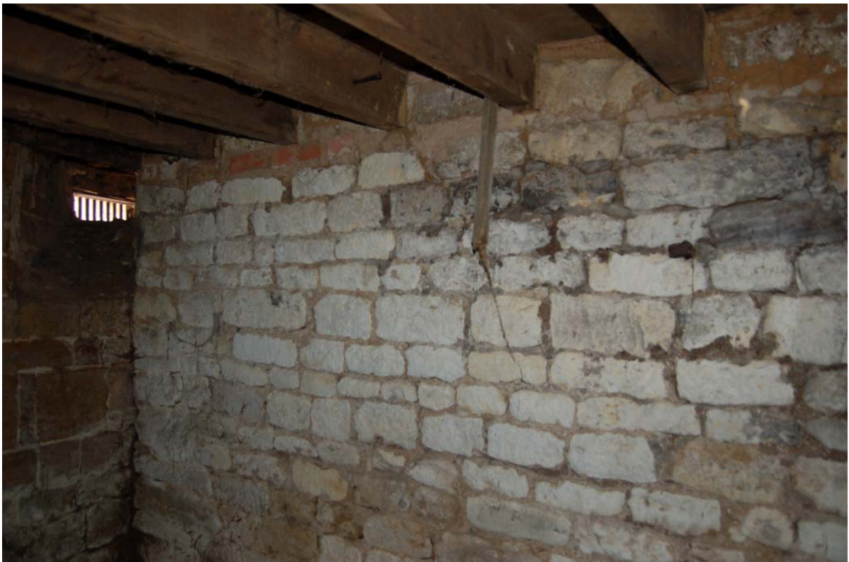
Plate 39: Basement [B01]; widened west wall abutting south wall adjacent to vent (left).
