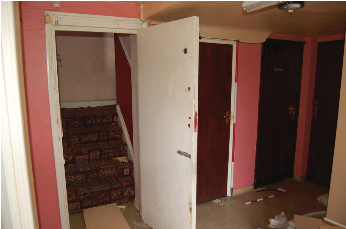
Plate 23: Rear lobby [G5]; doors to 1F (left), basement (middle) and Bar (right).
