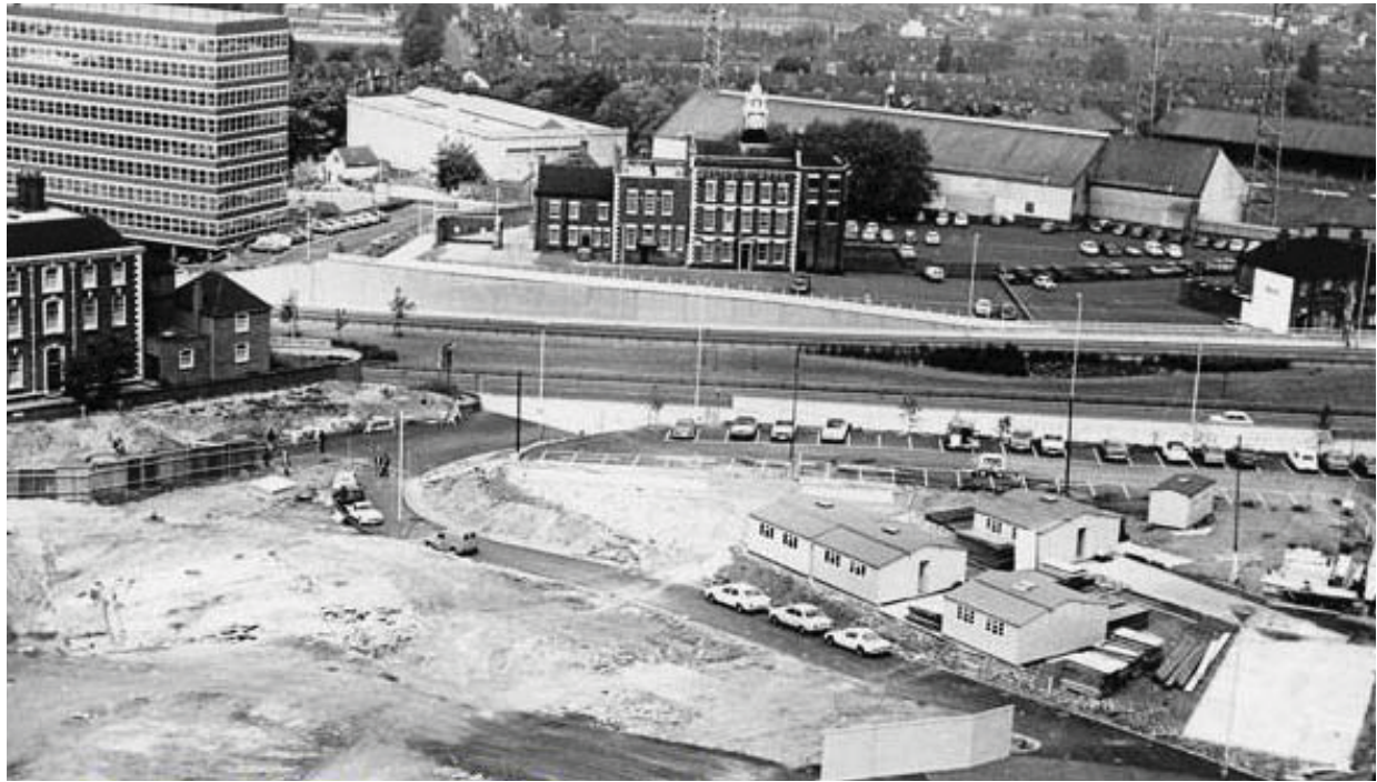
(a) General view looking north during construction of Wolverhampton Civic Centre, 1975 (WALS P/6353); Molineux Hotel to centre, Giffard House to left.
