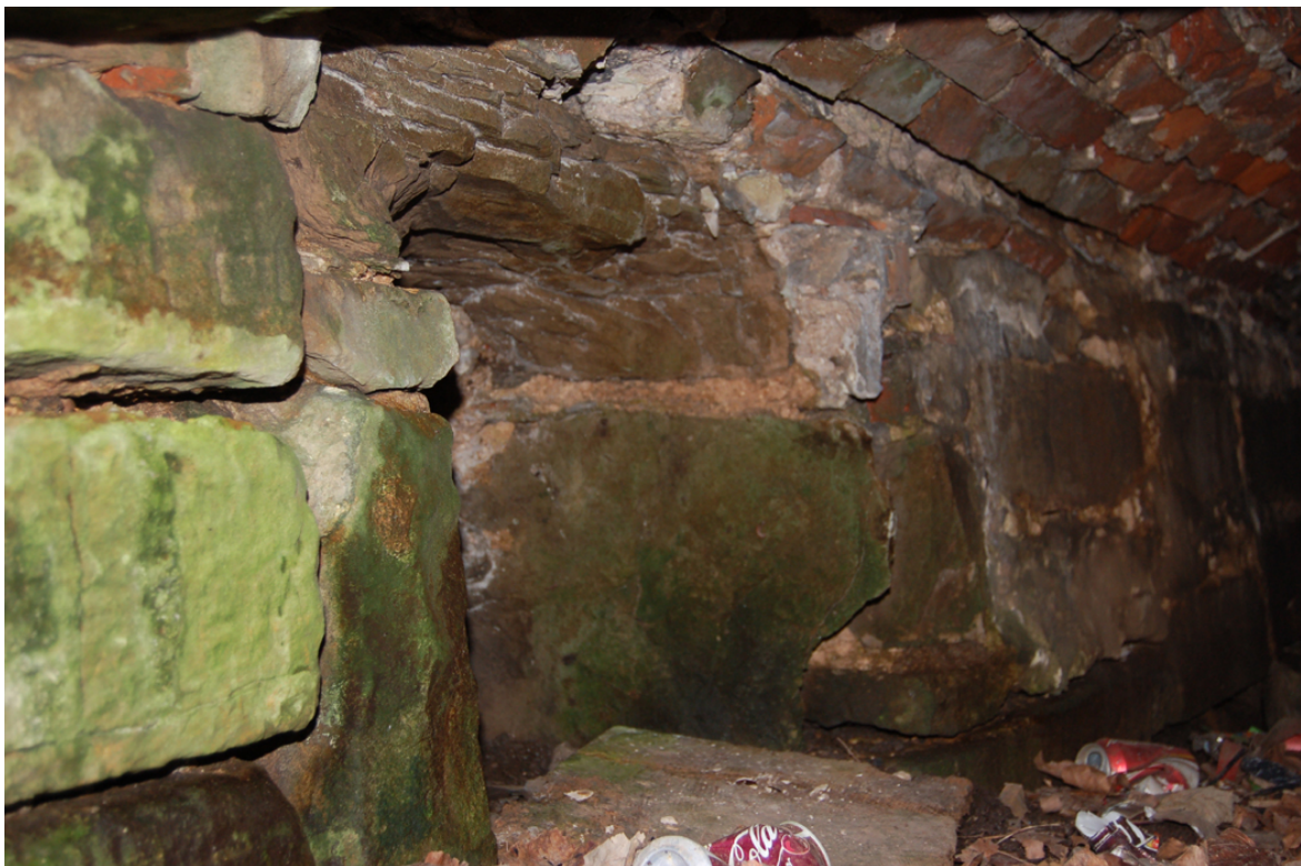
Plate 14: Culvert [C]; perpendicular channel [B2] opening off north end of east side, reflecting culvert [B] to south.
