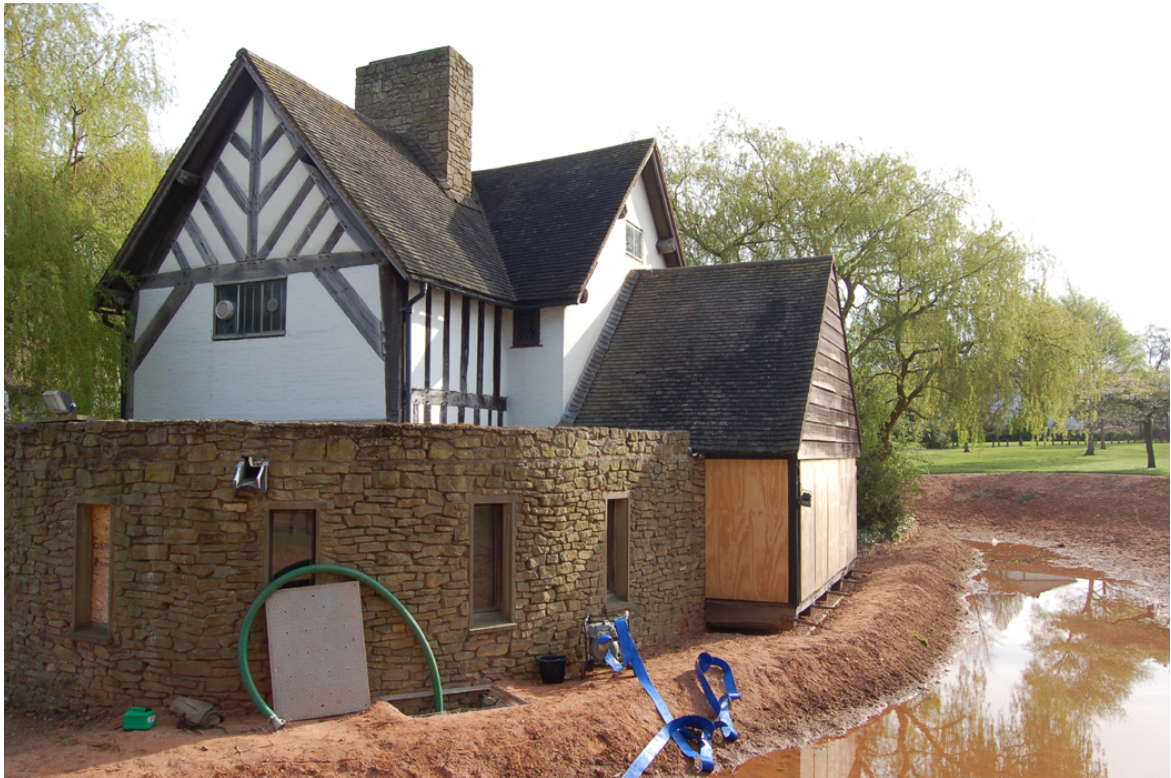
Plate 1: Culvert [A]; context shot looking north-east within C16 th /17 th kitchen range in background.
