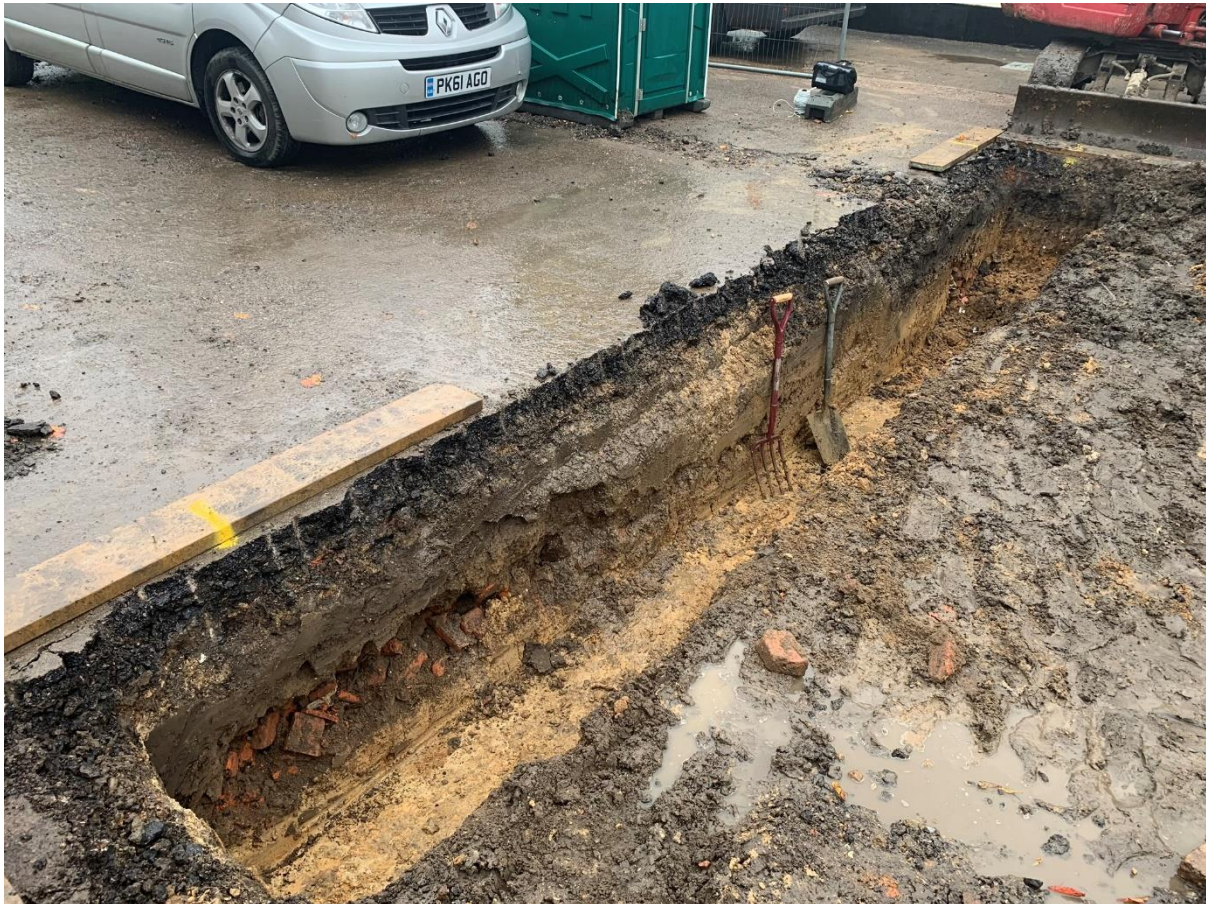
Figure 4: The foundation trench across the front of the building was the first one to be excavated. The sequence of tarmac (on a hoggin sub-base), made ground, subsoil and natural clay is clearly apparent in section, along with the modern soakaway at the near end of the trench. The modern pit was at the far end, but is mostly hidden in this view.
