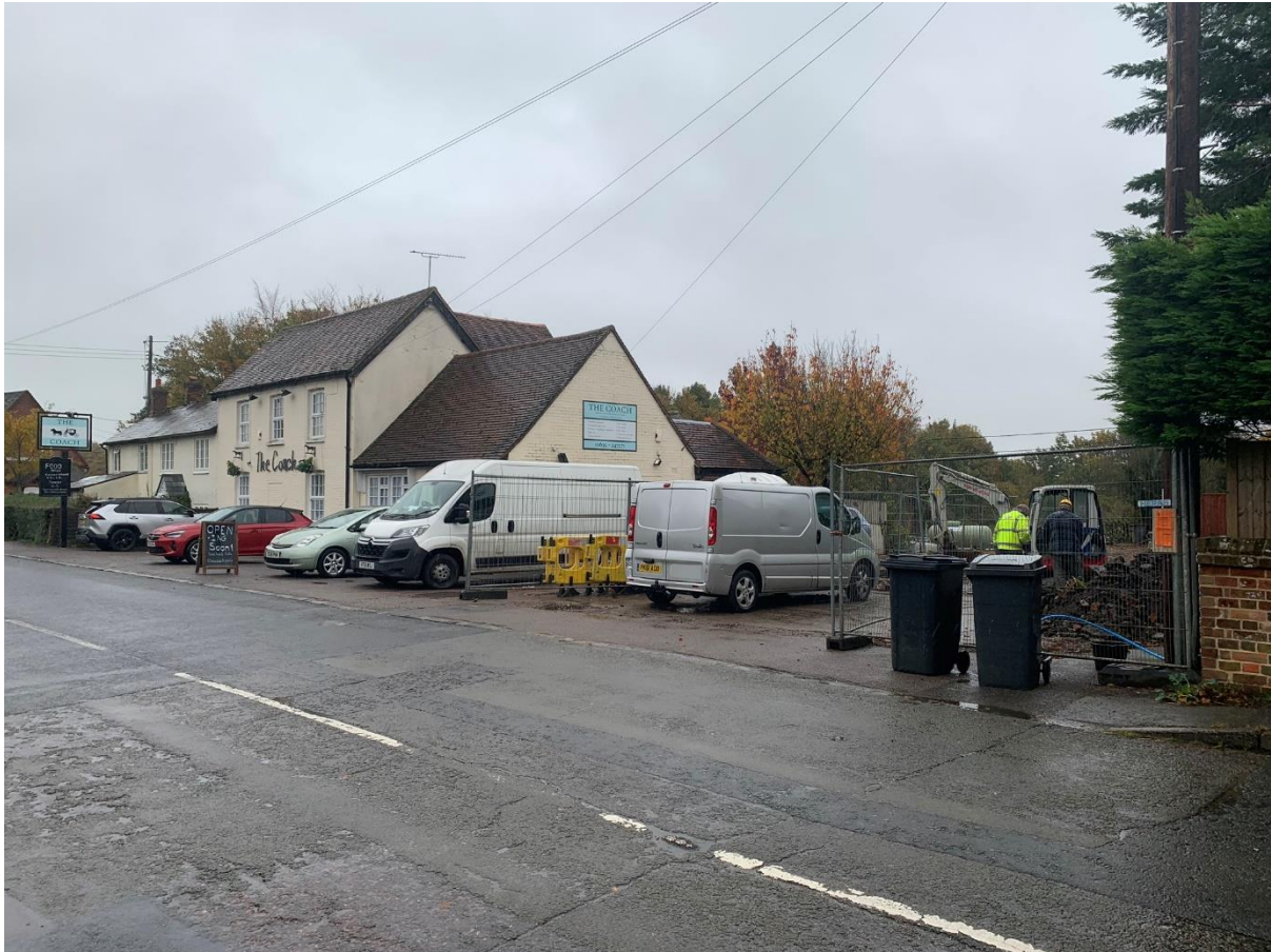
Figure 1: The Coach public house seen from the south-west, with excavation of the foundation trenches for a new house to its south under way on 29 October 2020.
