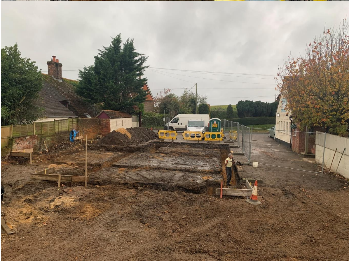
Figure 5: Views of the excavation nearing completion looking south-east (top), and finished looking north-west.
