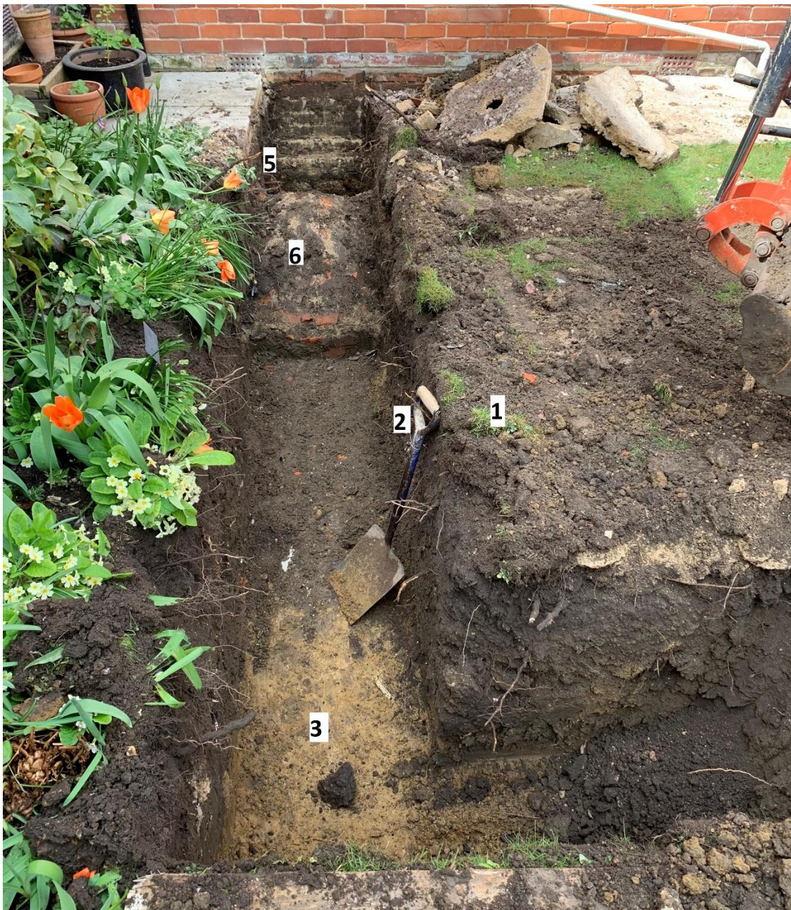
Figure 4: The south foundation trench looking west to the house, with context numbers shown. The 'soil' in front of drain 6 is trample at the base of the trench.
