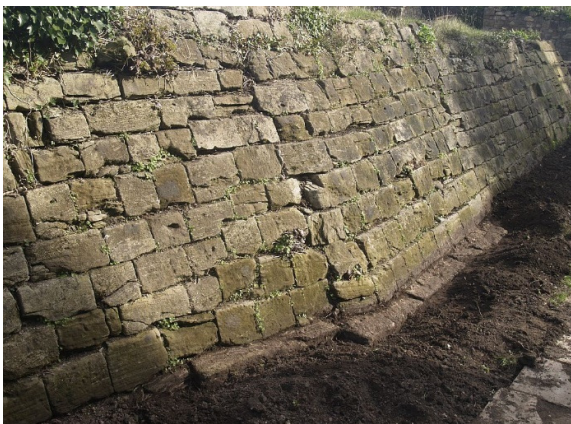
Figure 4: Wall B from the west showing the foundation course exposed by gardening at B2.
