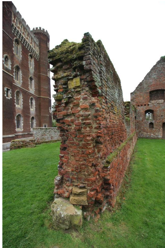
Figure 33 North end of the surviving east elevation wall, looking south-east. Note the stub of the projecting transverse wall and the base of the stone door jamb
