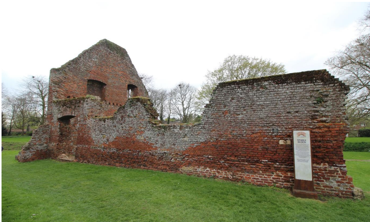
Figure 23 The east elevation of the building, looking south-west. Note the interpretation panel identifying the building as the "Stable Block". Image taken in February 2017.
