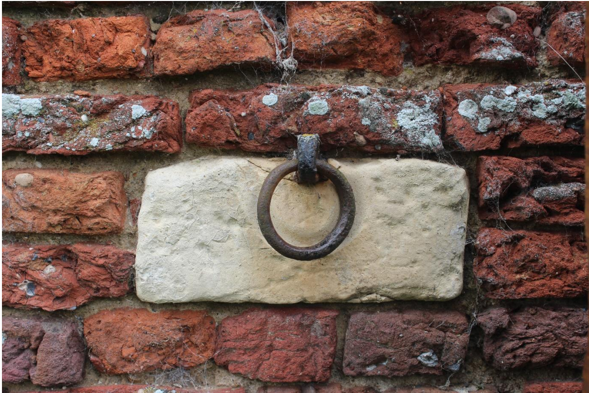
Figure 20 The northernmost of four stones originally associated with iron rings in the east elevation of the building, looking west
