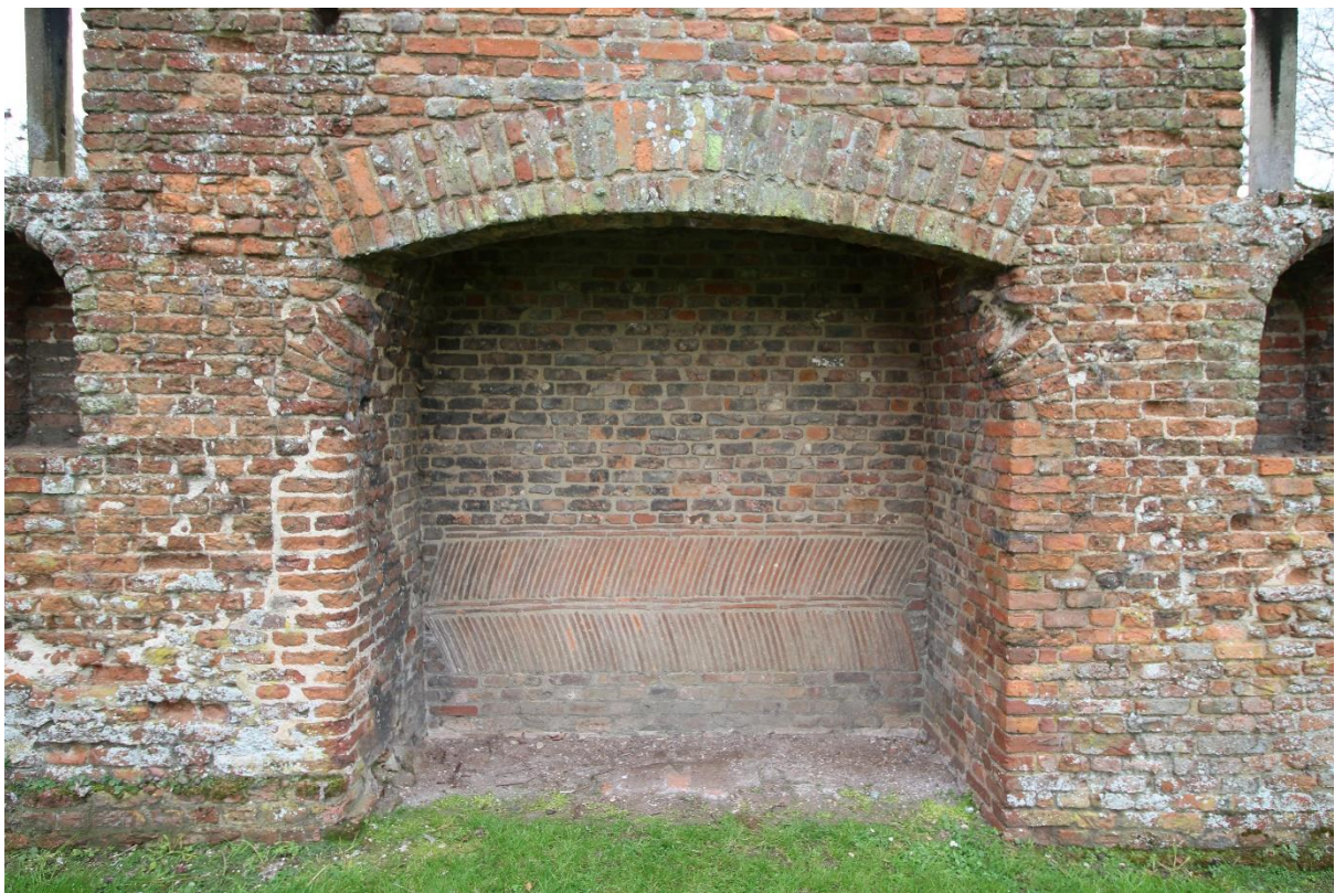
Figure 29 Detail of the rebuilt ground floor fireplace in the south elevation, looking south. Note the springers for the original arched head in the jambs below the current lintel.
