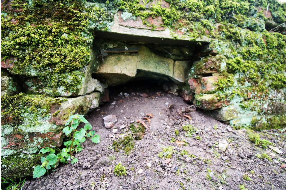
Figure 38 Blocked drain in the foundations of the west elevation of the north range, looking east
