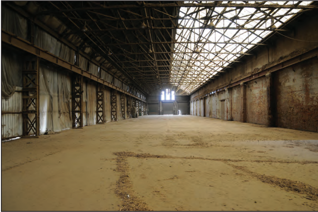
Photograph No. Washwood169 Description: Shed interior Site Location: A3 Direction From: E
