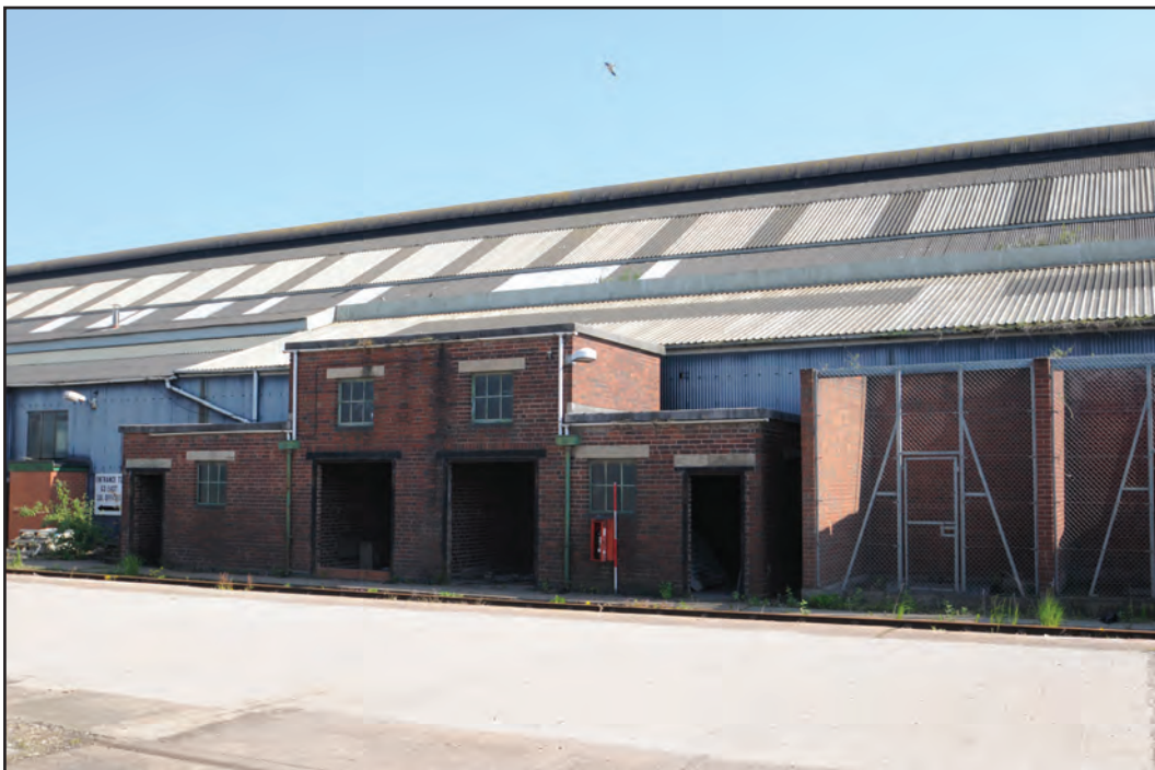
Photograph No. Washwood104 Description: Brick built storage units on exterior north of Building G Site Location: G7? Direction From: NW
