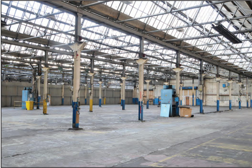
Photograph No. Washwood073 Description: View across sheds interior, taken from within D9 Site Location: D5-D9 Direction From: SW
