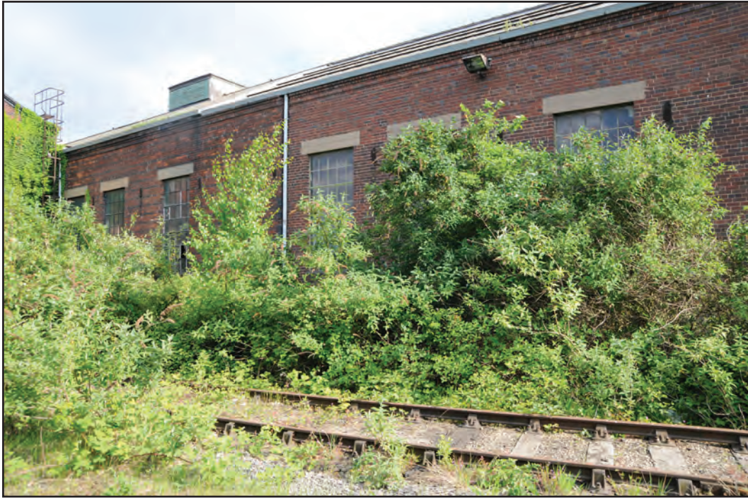
Photograph No. Washwood093 Description: Exterior north elevation Site Location: F4 Direction From: NW
