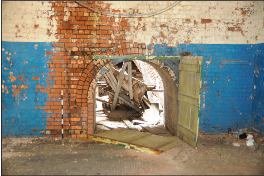
Photograph No. Washwood049 Description: Arched access to chimney at west end of south wall Site Location: C6a Direction From: N
