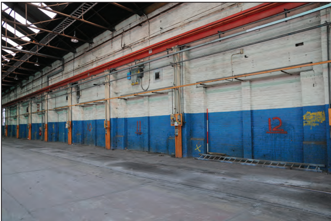
Photograph No. Washwoodo10 Description: Brick wall on north side of G3 with blocked openings, stanchions and steel rail Site Location: G3 Direction From: SE
