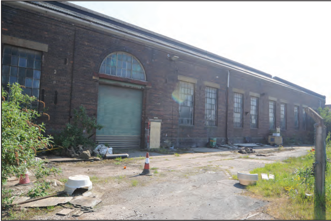
Photograph No. Washwood099 Description: west end of exterior north elevation Site Location: G3 Direction From: NE
