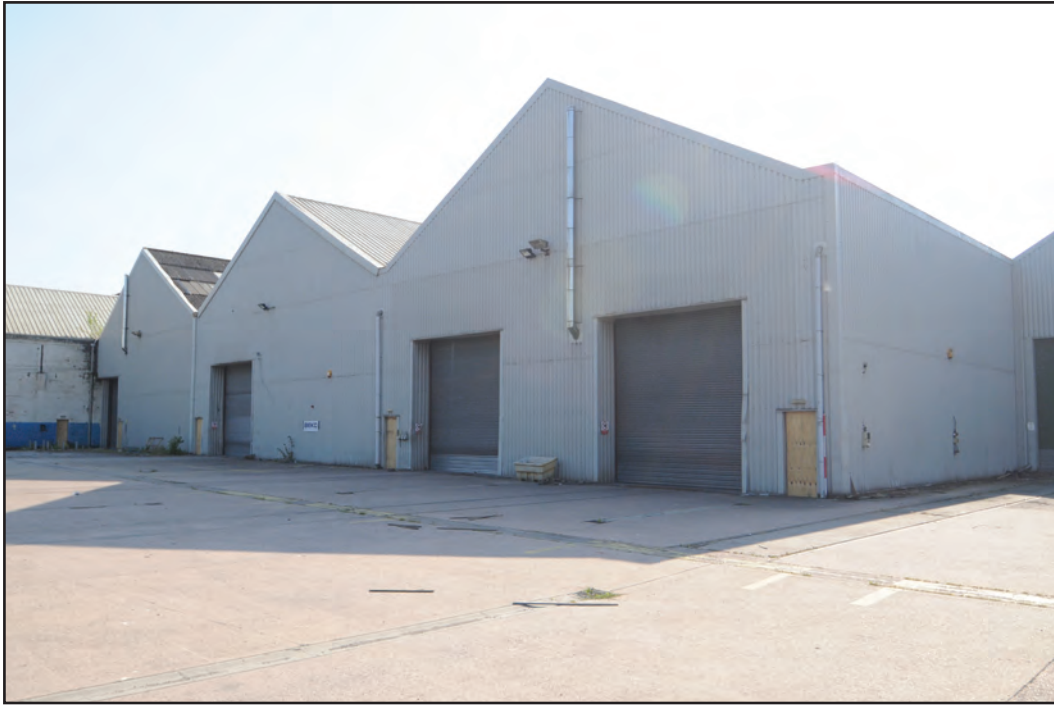
Photograph No. Washwood107 Description: Exterior east gable ends of C1-C3 and exterior north elevation of C1 Site Location: C1-C3 Direction From: NE
