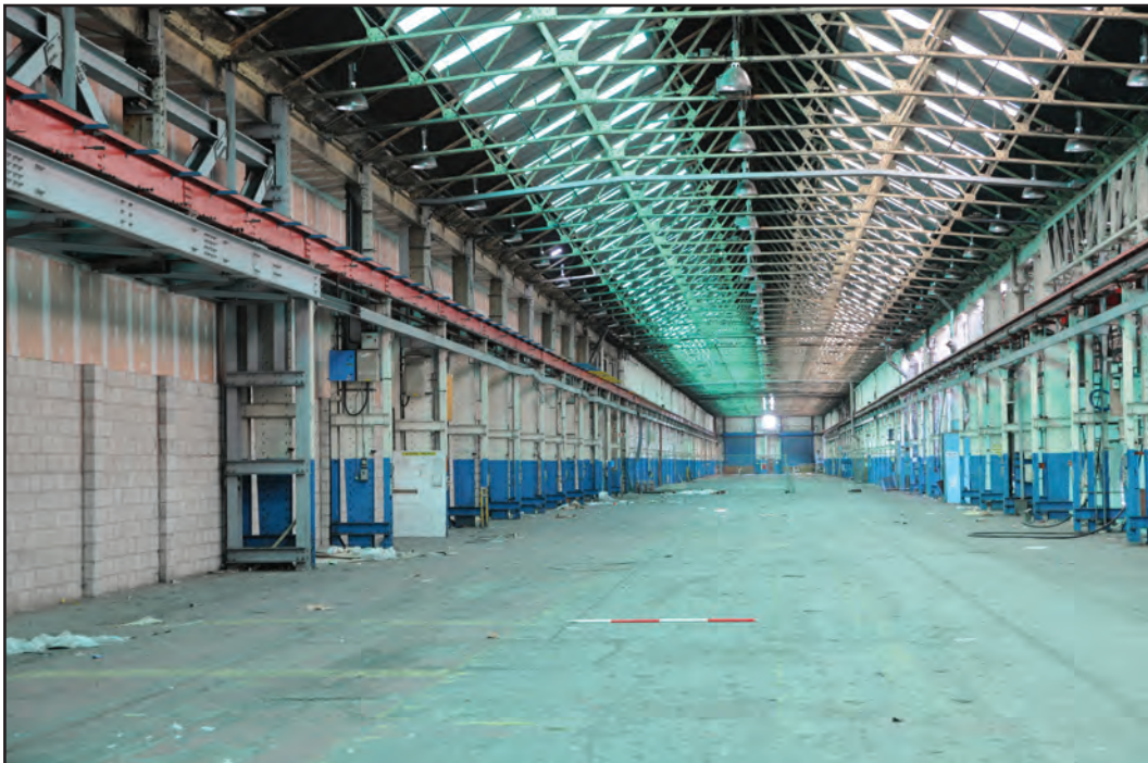
Photograph No. Washwood028 Description: Shed interior with missing pilaster on south side to allow for sideways movement of machinery in C1, now breeze-blocked up Site Location: G4 Direction From: NE
