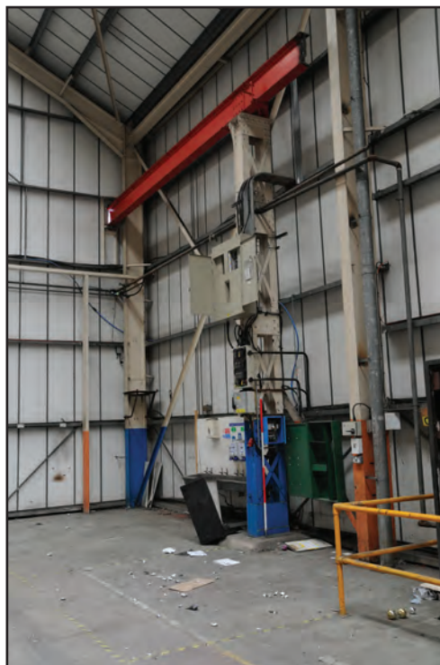
Photograph No. Washwood210 Description: Original stanchion and cut-off rail above in west corner of shed Site Location: HX Direction From: NW
