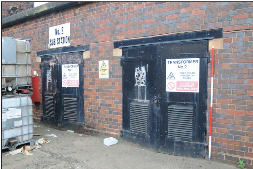
Photograph No. Washwood126 Description: Detail of metal doors Site Location: No. 2 sub-station Direction From: NW
