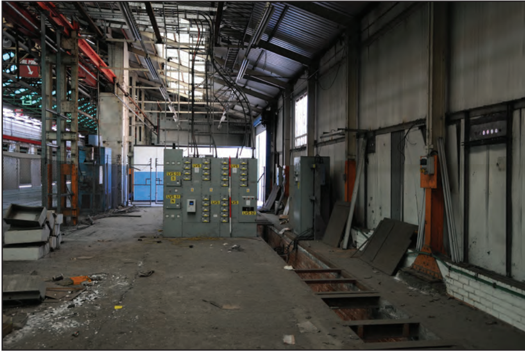
Photograph No. Washwood005 Description: Shed interior with inspection trench and electrical boxes Site Location: G2 Direction From: E
