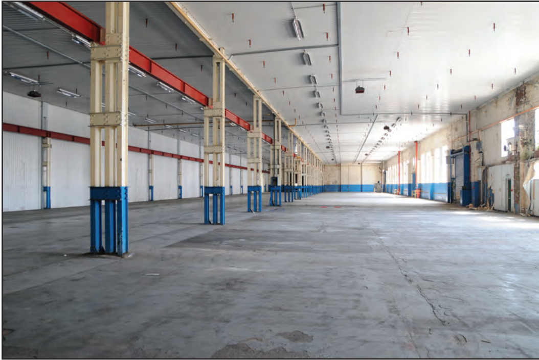
Photograph No. Washwood045 Description: View across shed interiors, taken from within C5 Site Location: C4/C5a Direction From: WSW
