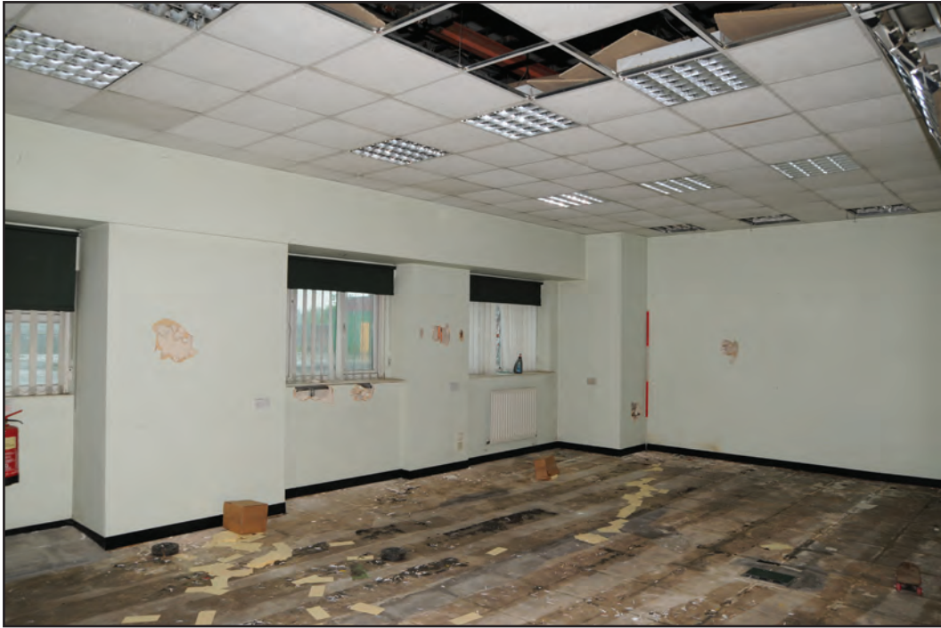
Photograph No. Washwood189 Description: Typical office area Site Location: A7 Direction From: NW
