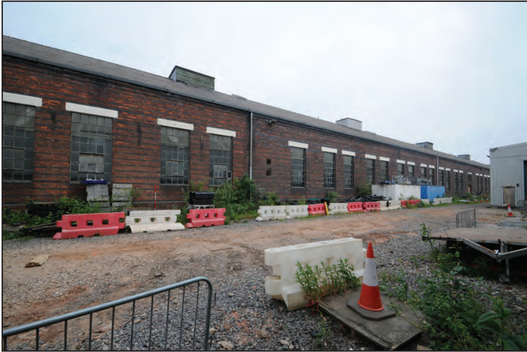
Photograph No. Washwood137 Description: Central area of exterior south elevation Site Location: F5 Direction From: SW
