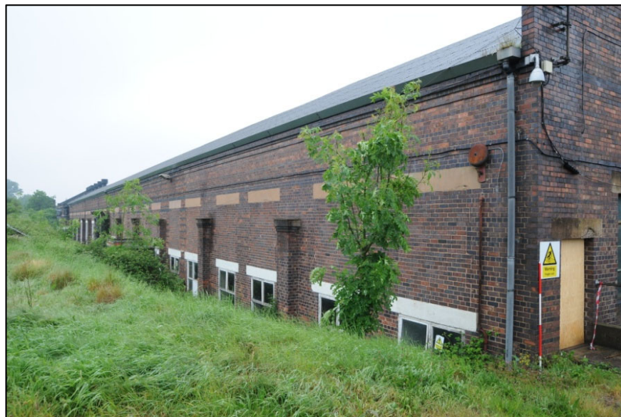
Plate 15: View from the elevated road at the southern end of the site
