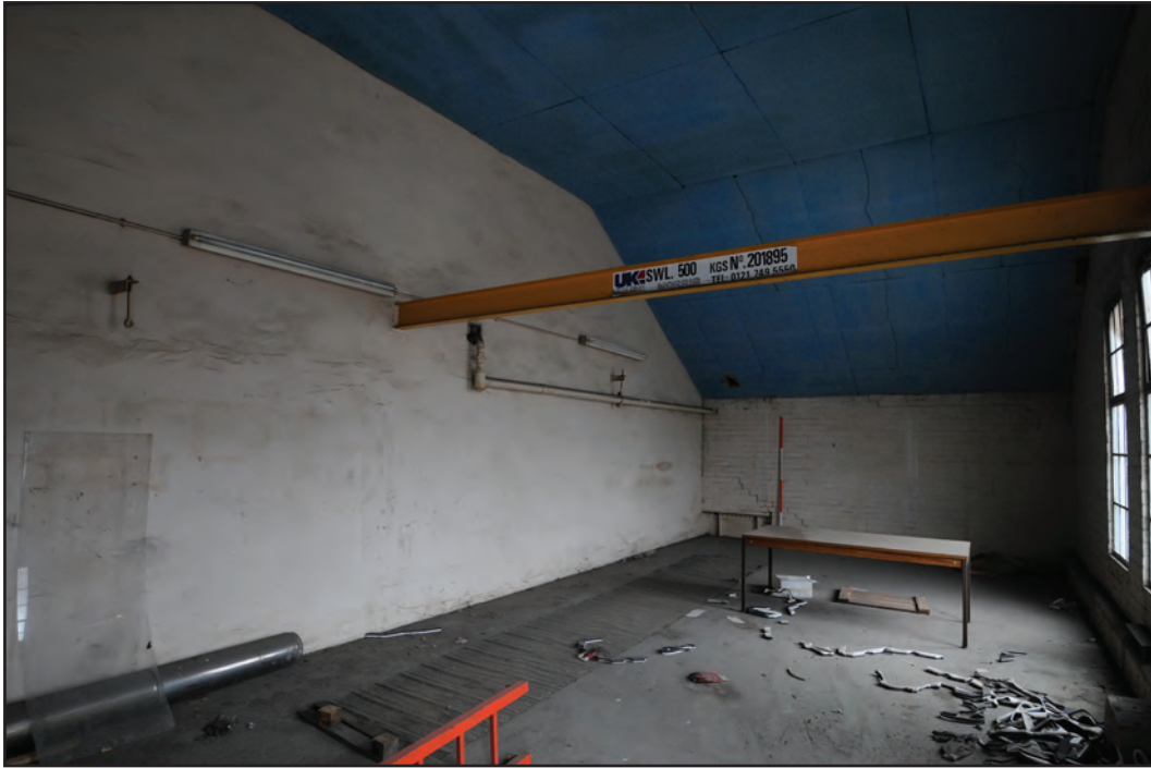
Photograph No. Washwood141 Description: Interior of first floor winch room Site Location: E3 Direction From: SW
