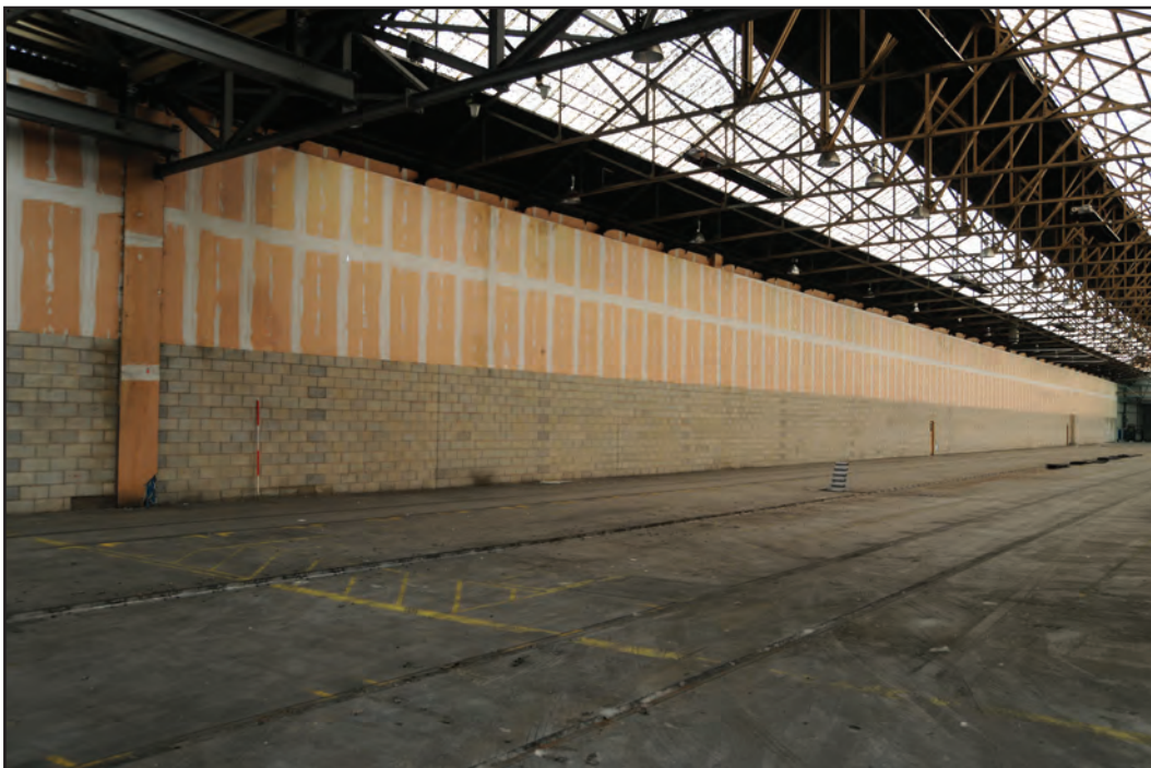
Photograph No. Washwood040 Description: Breeze block north interior elevation Site Location: C1 Direction From: SW
