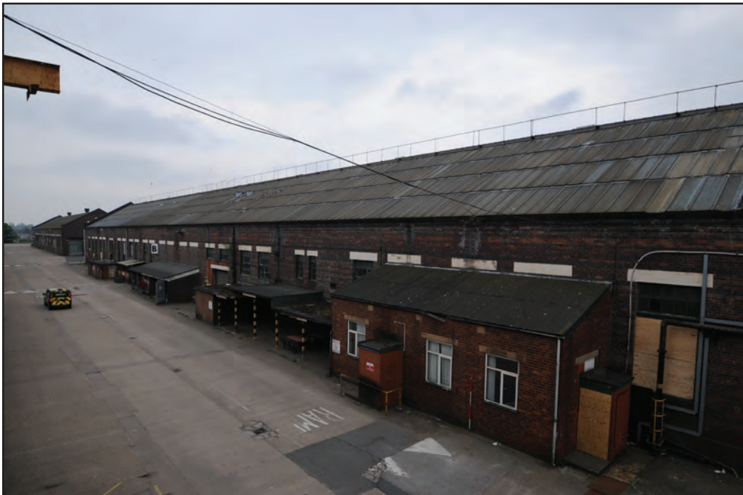
Photograph No. Washwood144 Description: Exterior north elevation Site Location: B1 Direction From: above NW
