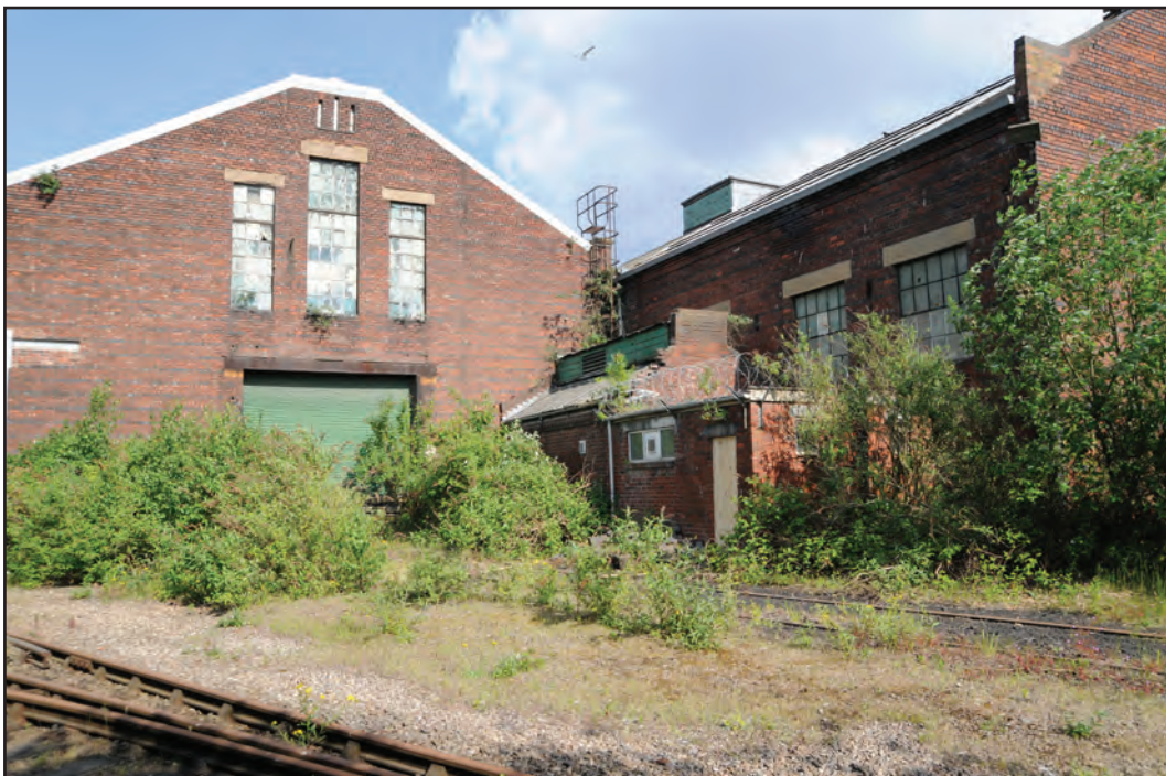
Photograph No. Washwood094 Description: F3 exterior west gable end and F4 exterior north elevation with small brick shed on exterior Site Location: F2/F3 Direction From: NW
