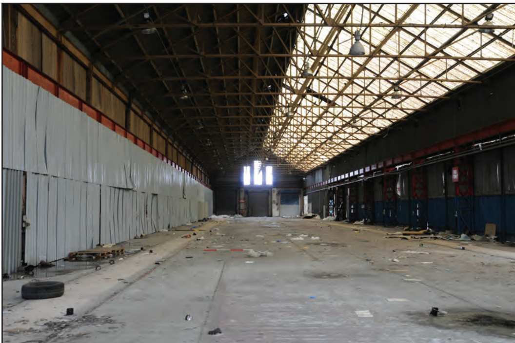
Photograph No. Washwood198 Description: General view of shed interior Site Location: B2 Direction From: E
