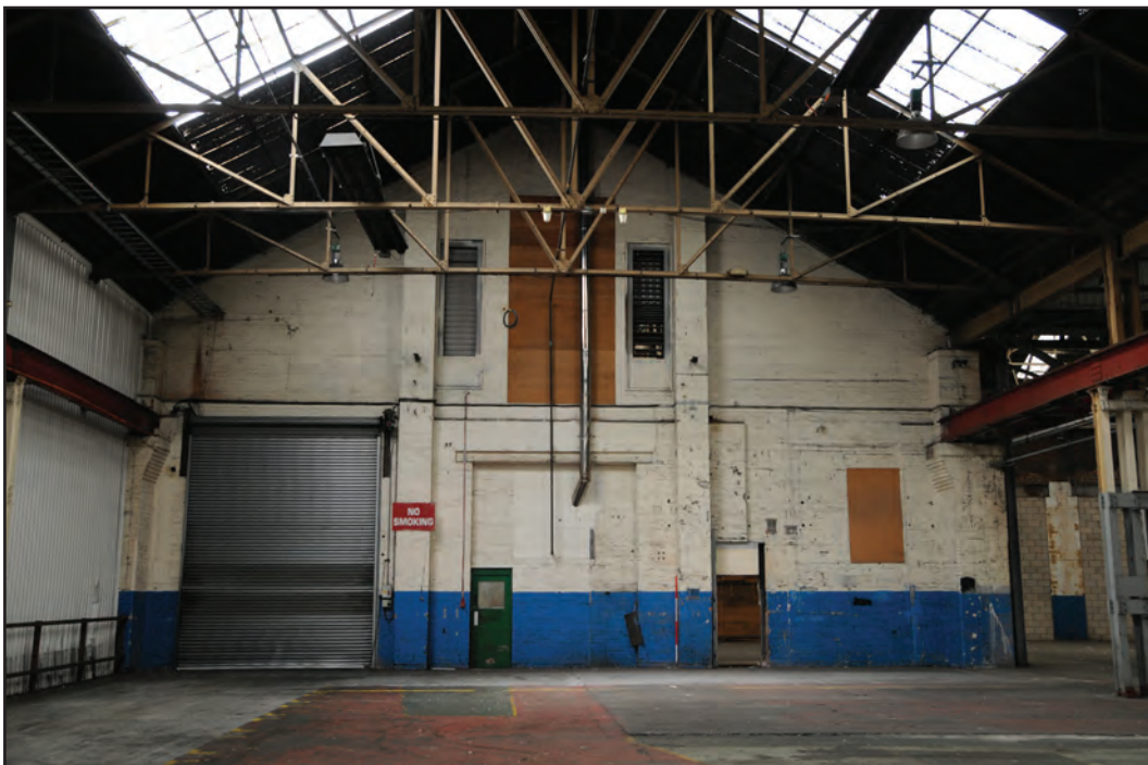
Photograph No. Washwood036 Description: West gable end of C3 shed and open end of shed C2 (on right of photo), both allowing access into shed D10 Site Location: C3/C2/D10 Direction From: ESE
