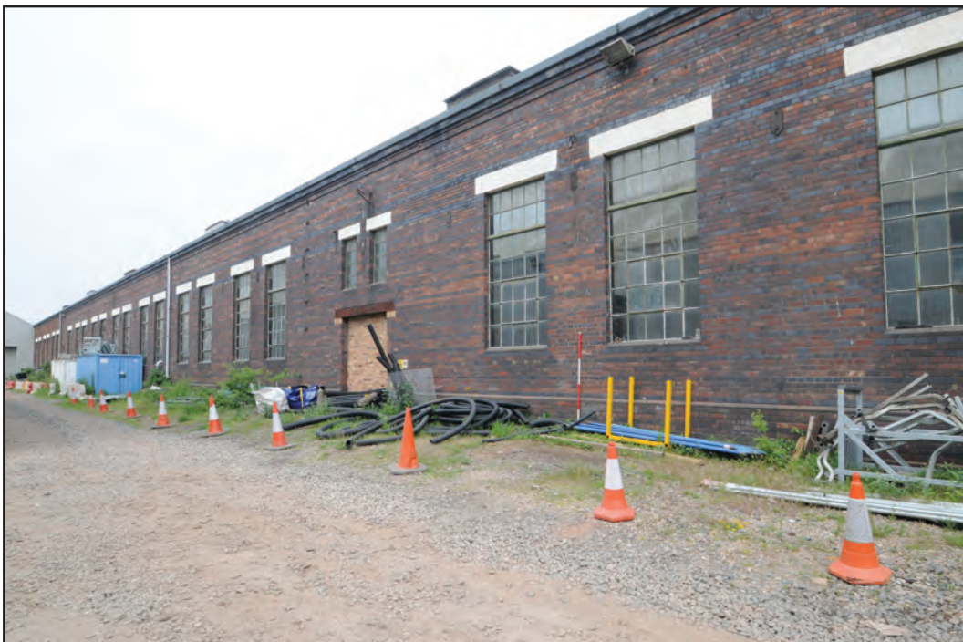
Photograph No. Washwood138 Description: Blocked doorway in central section of exterior south elevation Site Location: F5 Direction From: SE
