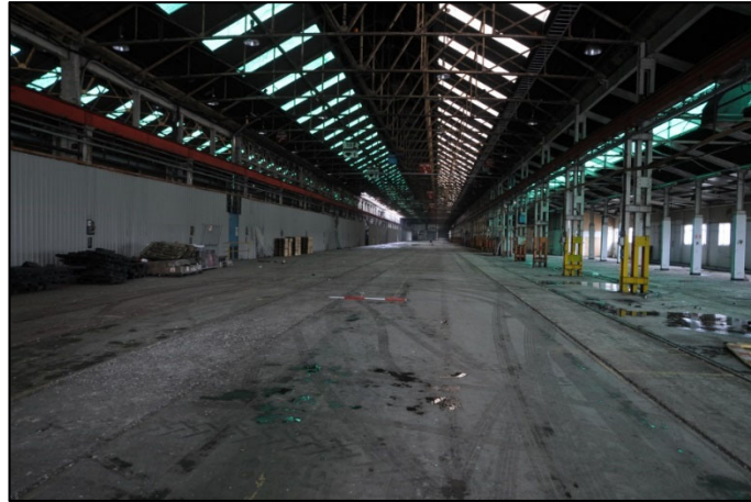
Plate 2: Internal view of Block G showing G3 with G2 and G1 to the right of the photograph
