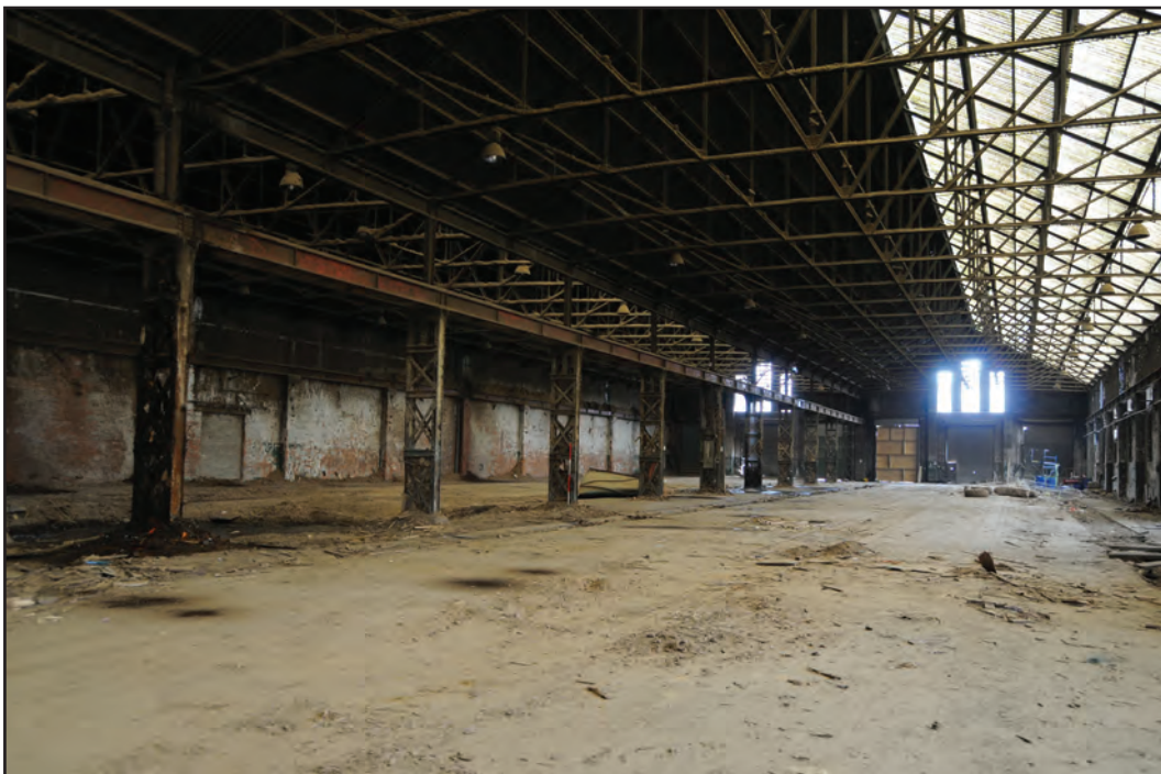
Photograph No. Washwood182 Description: View across shed interiors Site Location: A1/A2 Direction From: NE
