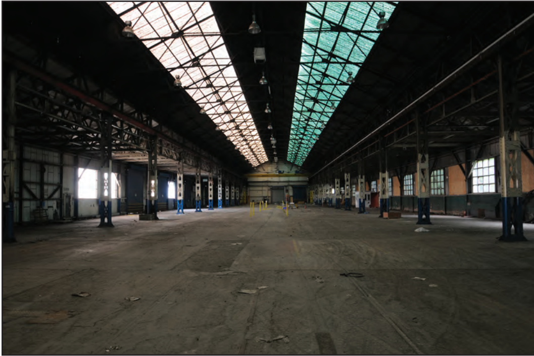
Photograph No. Washwood133 Description: Shed interior Site Location: H1 Direction From: W
