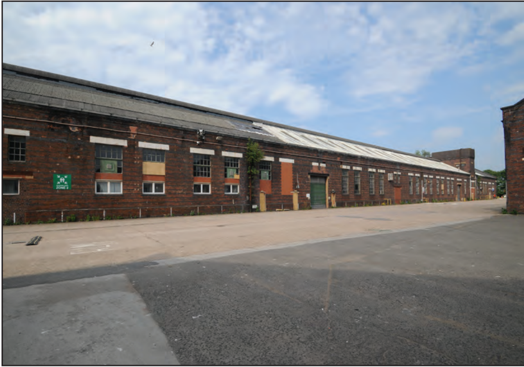
Photograph No. Washwood149 Description: Exterior south elevation, central area Site Location: C5 Direction From: SW
