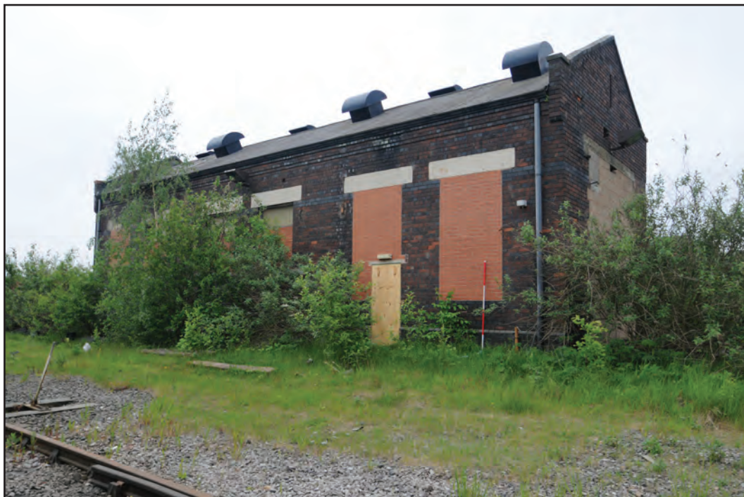
Photograph No. Washwood120 Description: Exterior north and west elevations with blocked openings and ventilation equipment on the roof Site Location: Loco shed Direction From: NW
