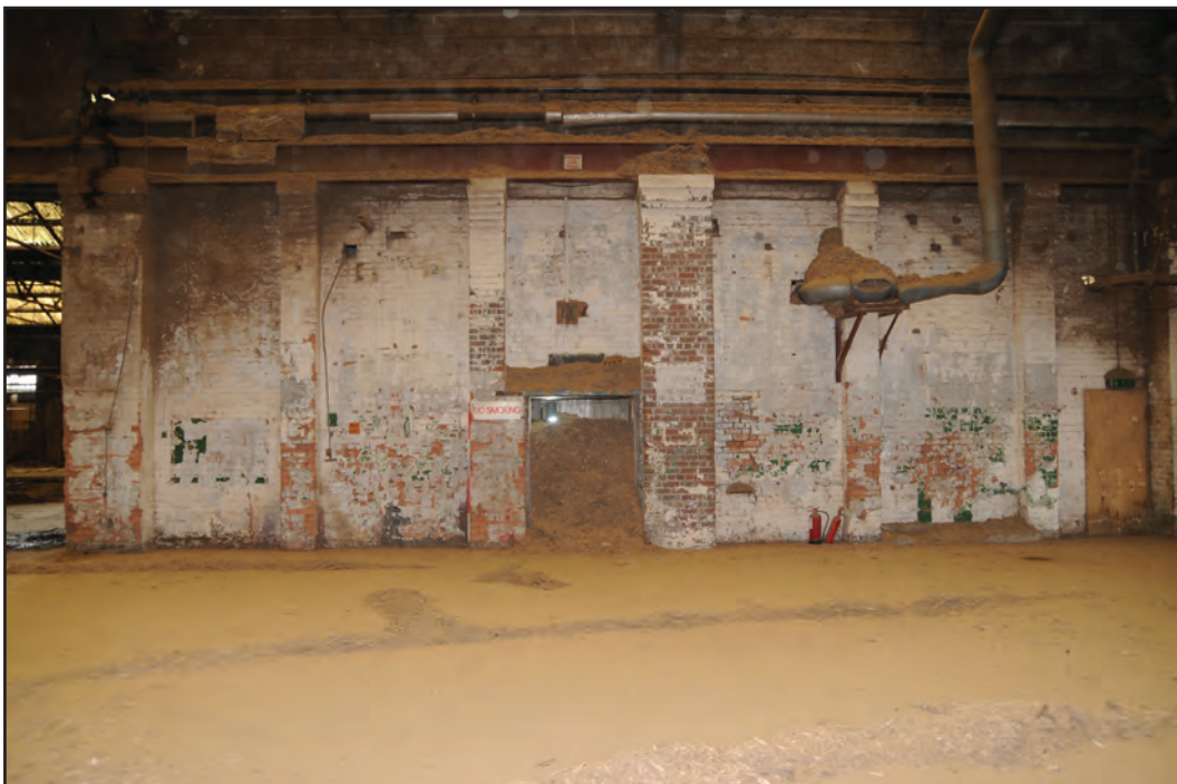
Photograph No. Washwood170 Description: Blocked opening at east end of north interior elevation, with additional small pilasters Site Location: A3 Direction From: S
