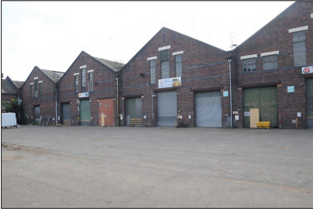
Photograph No. Washwood163 Description: Exterior east gable ends Site Location: B3-B5 Direction From: NE
