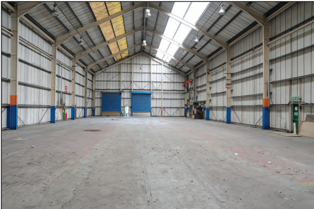
Photograph No. Washwood208 Description: Shed interior Site Location: HX Direction From: W
