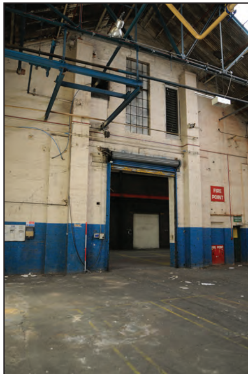
Photograph No. Washwood044 Description: Interior west gable end with steel rails in southwest corner of room Site Location: C5b Direction From: ESE
