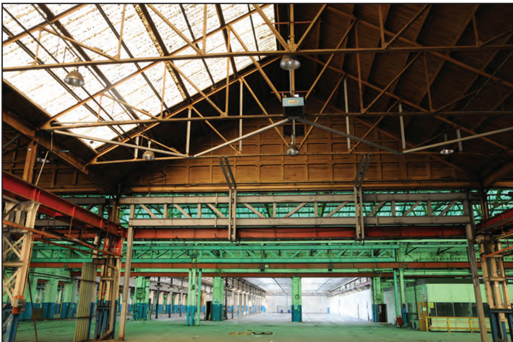
Photograph No. Washwood084 Description: Interior east end timber gable Site Location: F2-F5 Direction From: W
