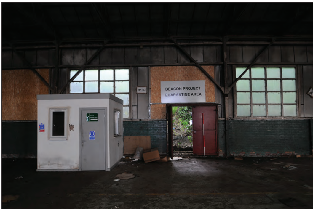
Photograph No. Washwood132 Description: Detail of door and cabin office at centre of south wall Site Location: H1 Direction From: N
