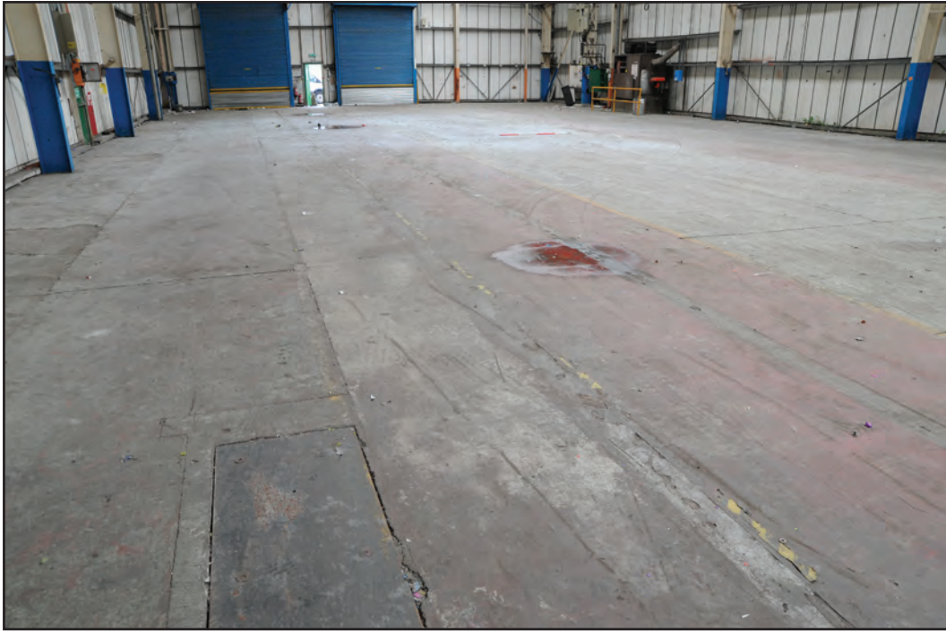
Photograph No. Washwood209 Description: Detail of train rail on cast concrete floor Site Location: HX Direction From: WNW
