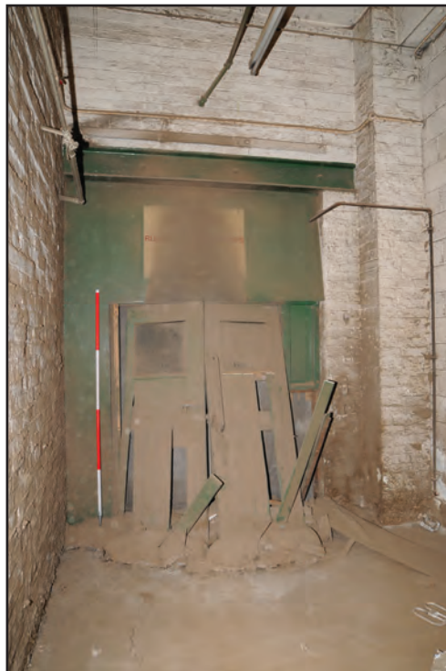
Photograph No. Washwood192 Description: Blocked access from offices into A2 ground floor Site Location: A7 Direction From: E
