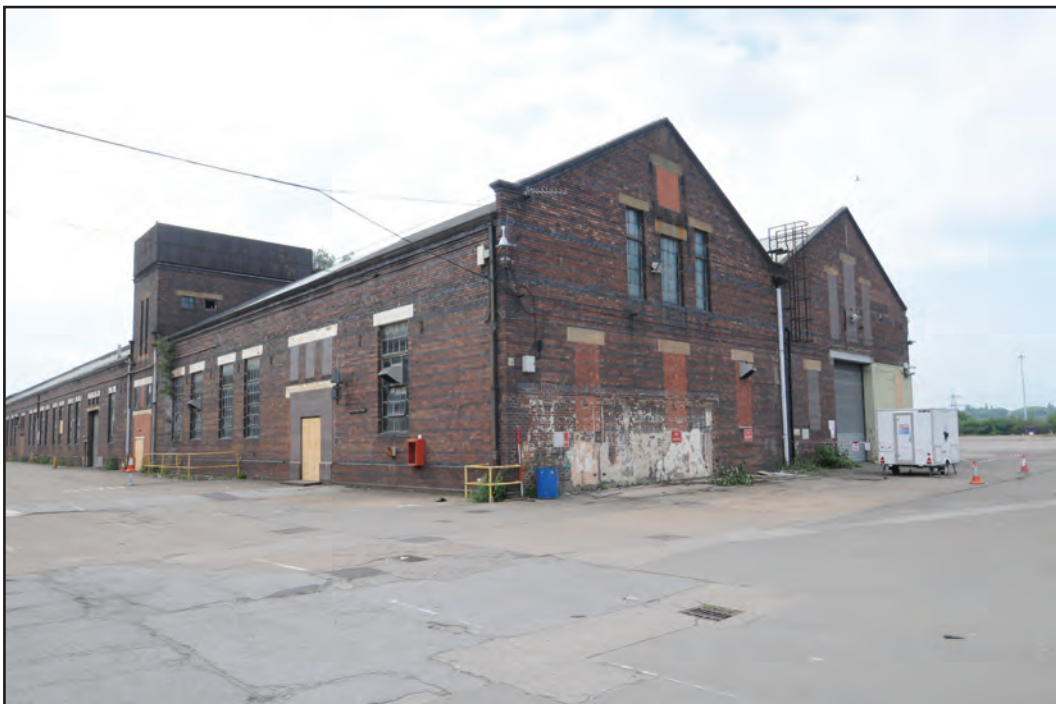
Photograph No. Washwood146 Description: Exterior east gable ends of C6a and C6c, exterior south elevation of C6b and C6c Site Location: C6a-C6c Direction From: SE
