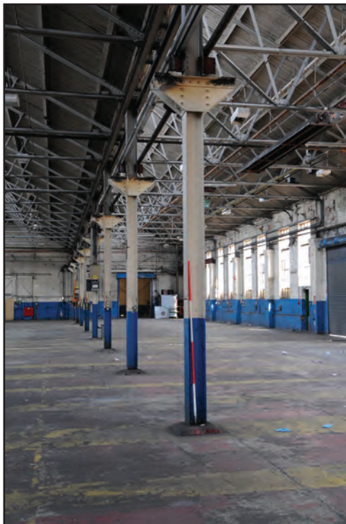
Photograph No. Washwood074 Description: Detail of stanchion separating D8 and D9 sheds Site Location: D8/D9 Direction From: WNW
