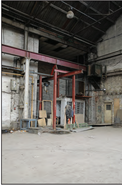
Photograph No. Washwood187 Description: Detail of southwest corner of shed interior with hoist equipment Site Location: A4 Direction From: NE
