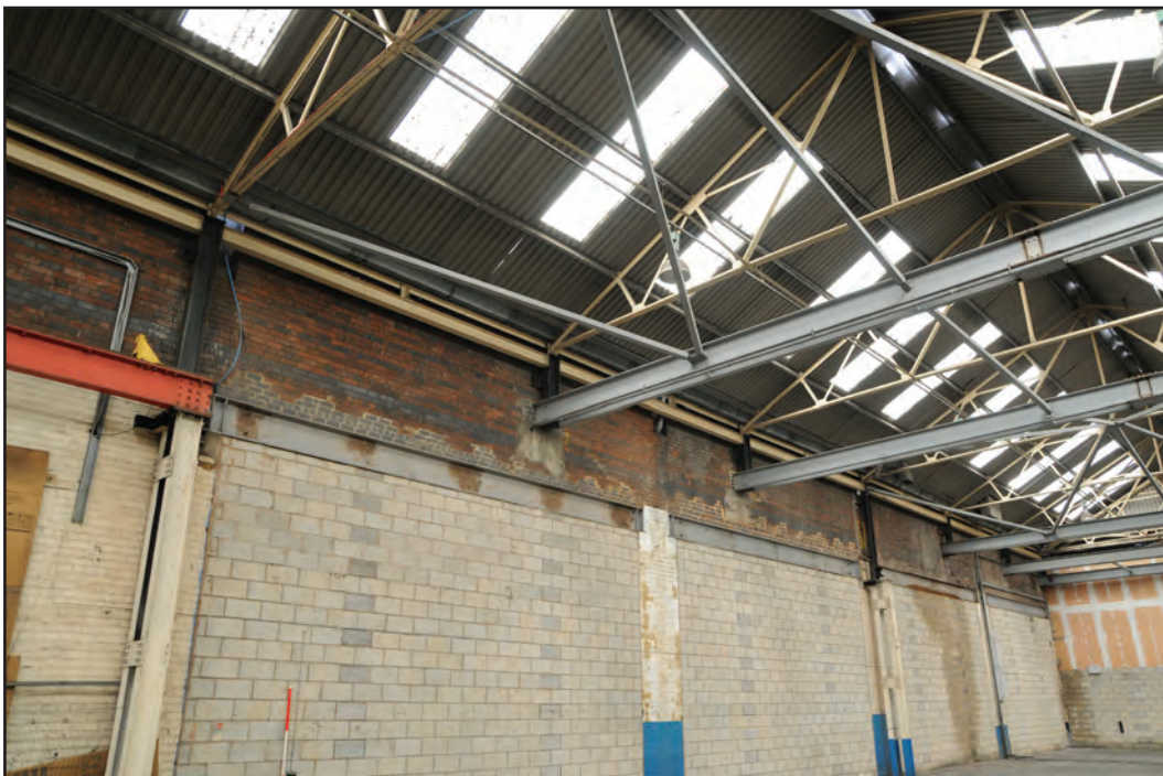
Photograph No. Washwood042 Description: north end of west interior elevation, breeze-blocks stopping access to sheds D1-D4 with detail of varying wall types and change in steel superstructure Site Location: D10 Direction From: NW
