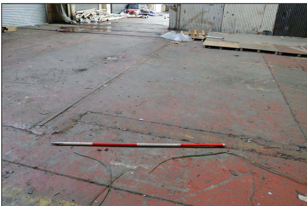
Photograph No. Washwood200 Description: Cast concrete floor with rails and drains at west end of interior Site Location: B2 Direction From: SE
