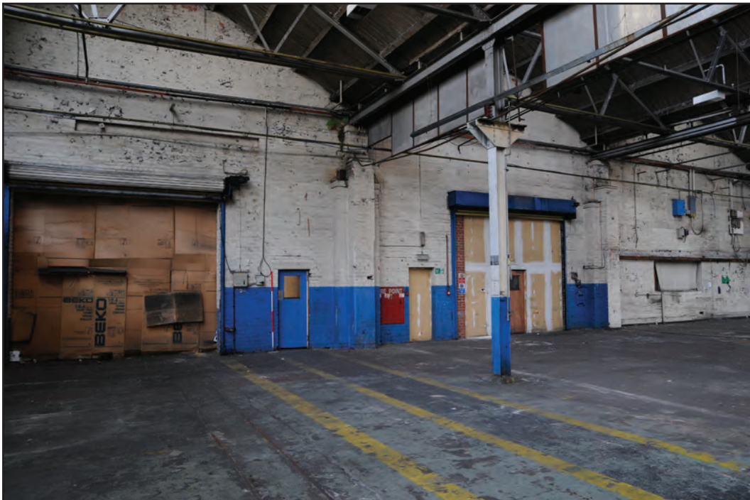
Photograph No. Washwood070 Description: Internal east gable ends Site Location: D5-D7 Direction From: NW
