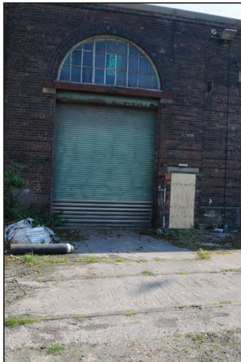
Photograph No. Washwood100 Description: Detail of roller door at west end of exterior north elevation Site Location: G3 Direction From: N
