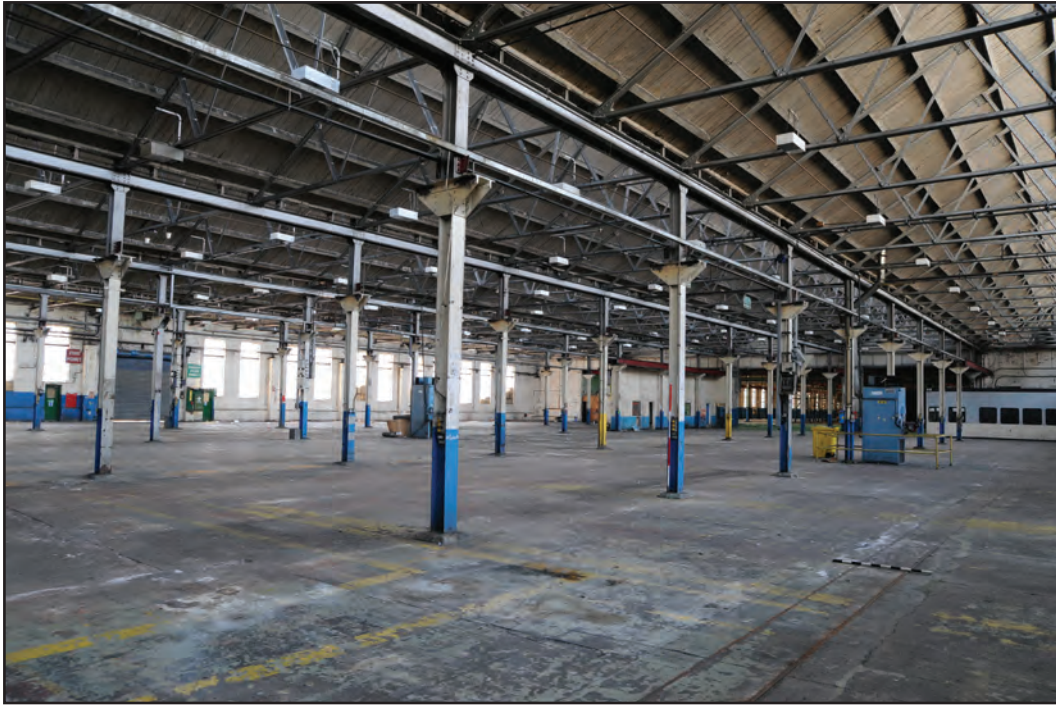
Photograph No. Washwood069 Description: View across sheds interior, taken from within D5 Site Location: D5-D9 Direction From: NE
