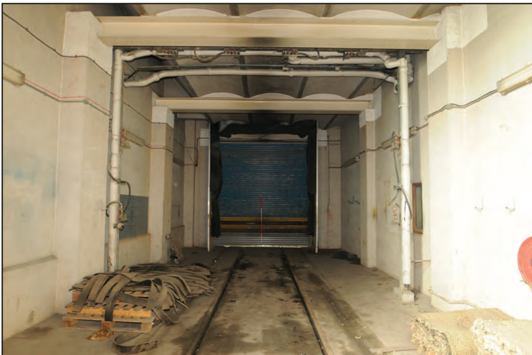
Photograph No. Washwood114 Description: Interior of train washing room, east end with roller door leading through to west gable end of G3 Site Location: G6c Direction From: W
