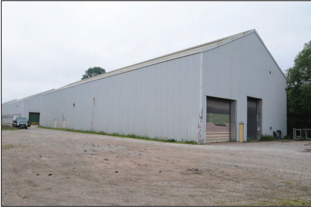
Photograph No. Washwood121 Description: Exterior north and west elevations Site Location: HX Direction From: NW
