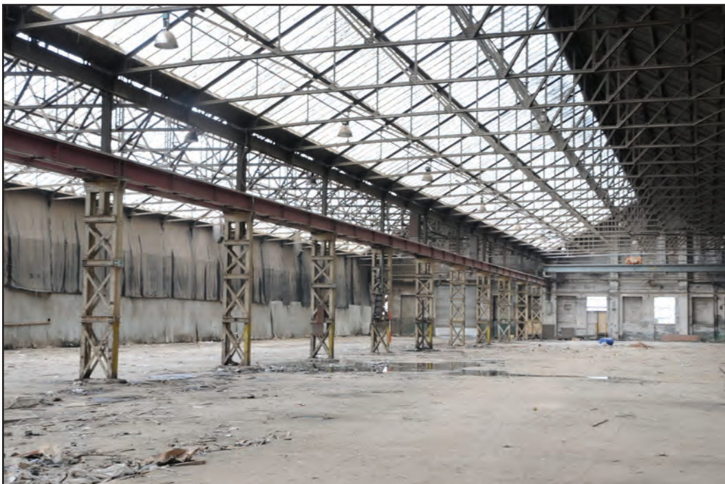
Photograph No. Washwood186 Description: View across sheds interior, taken from within A5 Site Location: A5/A4 Direction From: SW
