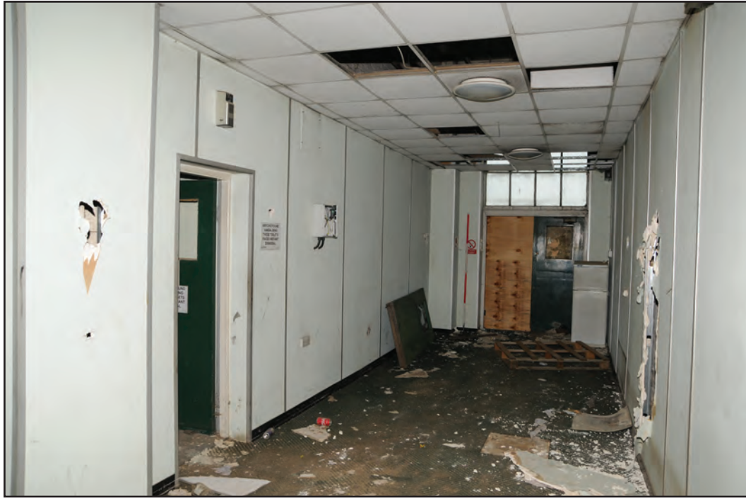
Photograph No. Washwood191 Description: Office entry and lobby area Site Location: A7 Direction From: SW
