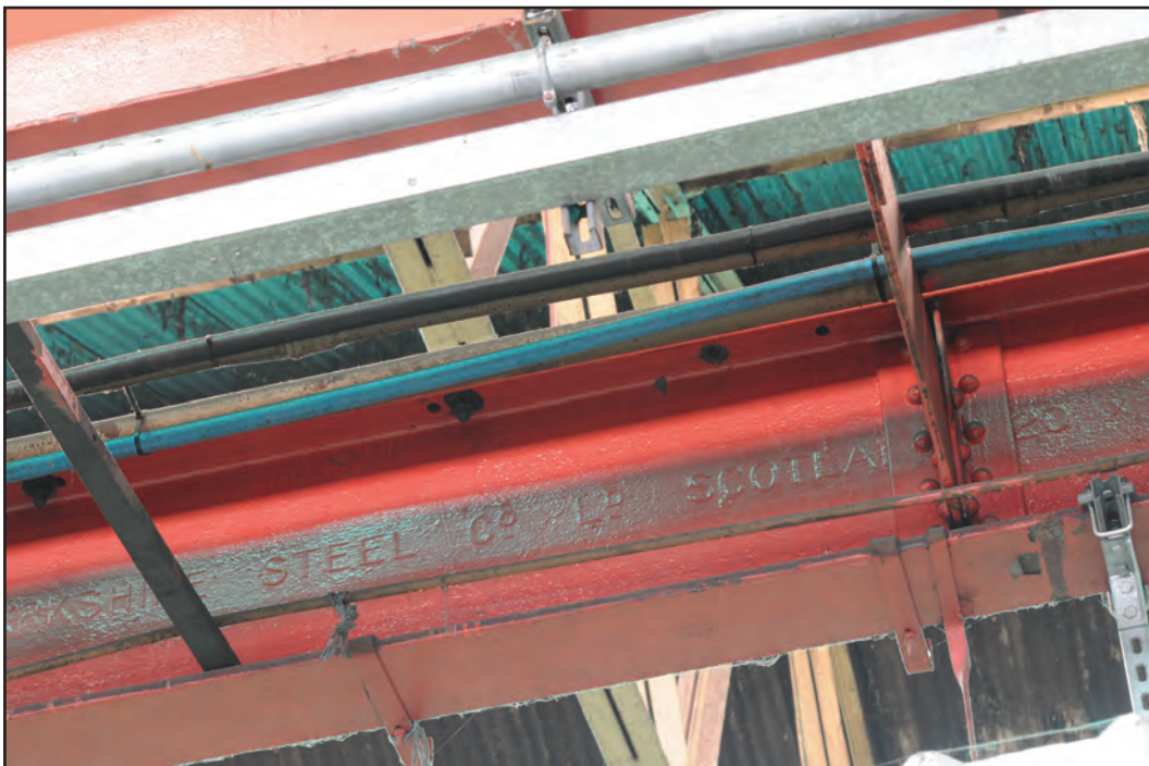
Photograph No. Washwood014 Description: LANARKSHIRE STEEL CO LD SCOTLAND 20 X 7 1/2 Foundry mark on steel rail Site Location: G4 Direction From: N
