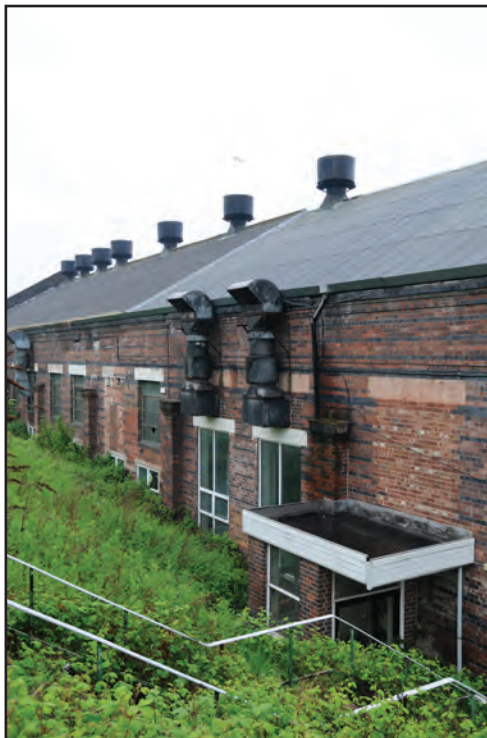
Photograph No. Washwood234 Description: Ventilators in the centre of south exterior elevation Site Location: A6 Direction From: SE
