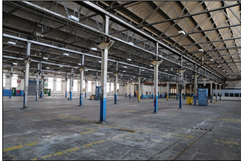
Plate 5: showing the steel stanchions and the saw-tooth roof structure of Block D
