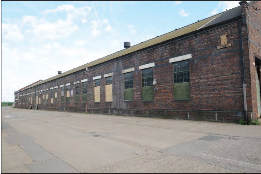
Photograph No. Washwood167 Description: Exterior north elevation of offices at east end of A1 Site Location: A1 Direction From: NNE
