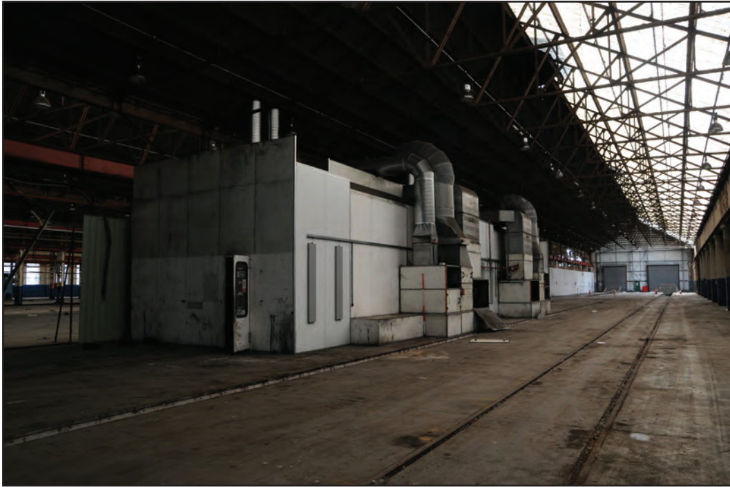
Photograph No. Washwood079 Description: Shed interior with spraying room Site Location: F1 Direction From: NE
