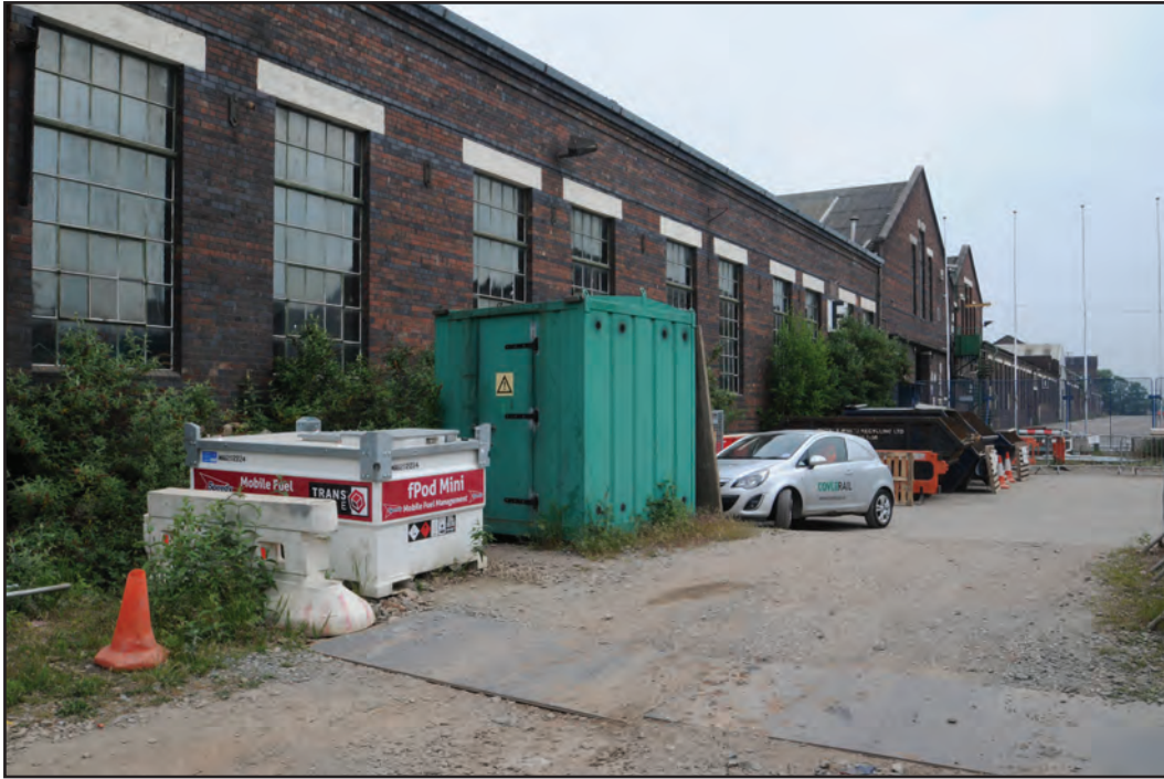
Photograph No. Washwood139 Description: east end of exterior south elevation Site Location: F5 Direction From: SW
