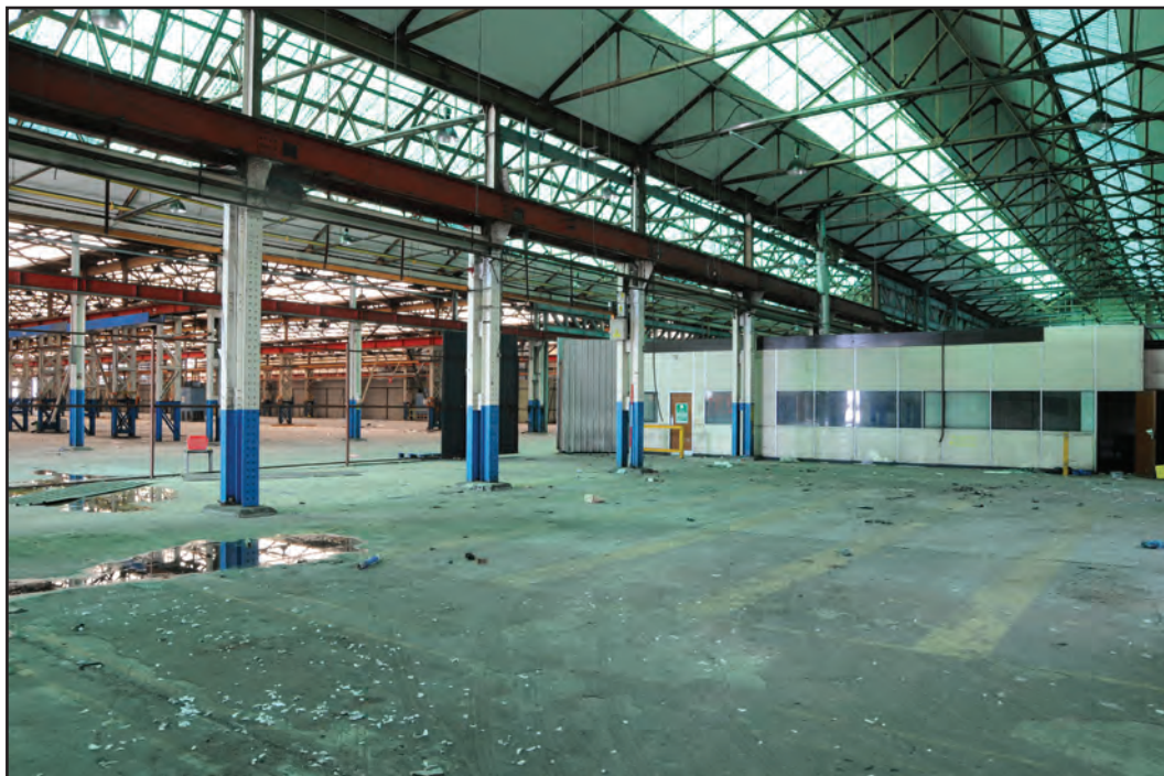
Photograph No. Washwood076 Description: View across sheds interior with office space separating the north and south shed ends Site Location: E1/E2 Direction From: SE
