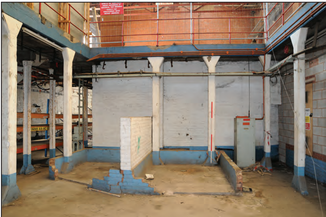
Photograph No. Washwood062 Description: Ground floor concrete supports and low brick internal divisions Site Location: C6d Direction From: E
