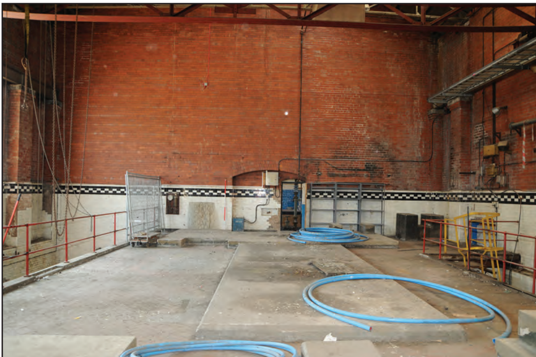
Photograph No. Washwood058 Description: Engine house interior west elevation with blocked arched opening, tiling and water control Site Location: C6c Direction From: E
