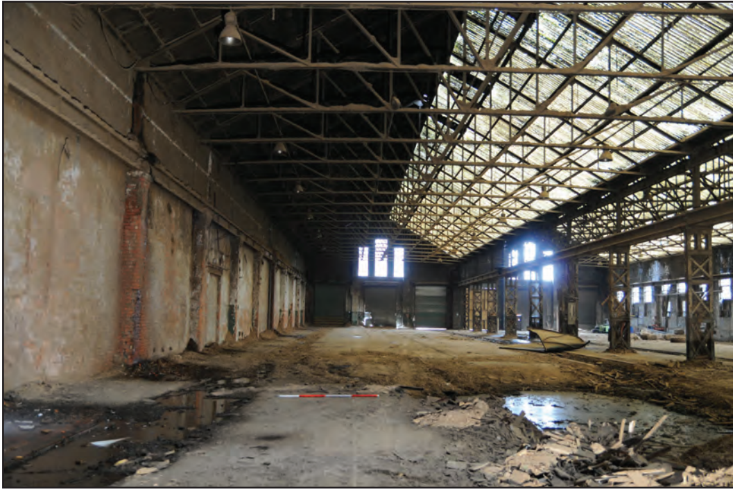
Photograph No. Washwood175 Description: Shed interior Site Location: A2 Direction From: E
