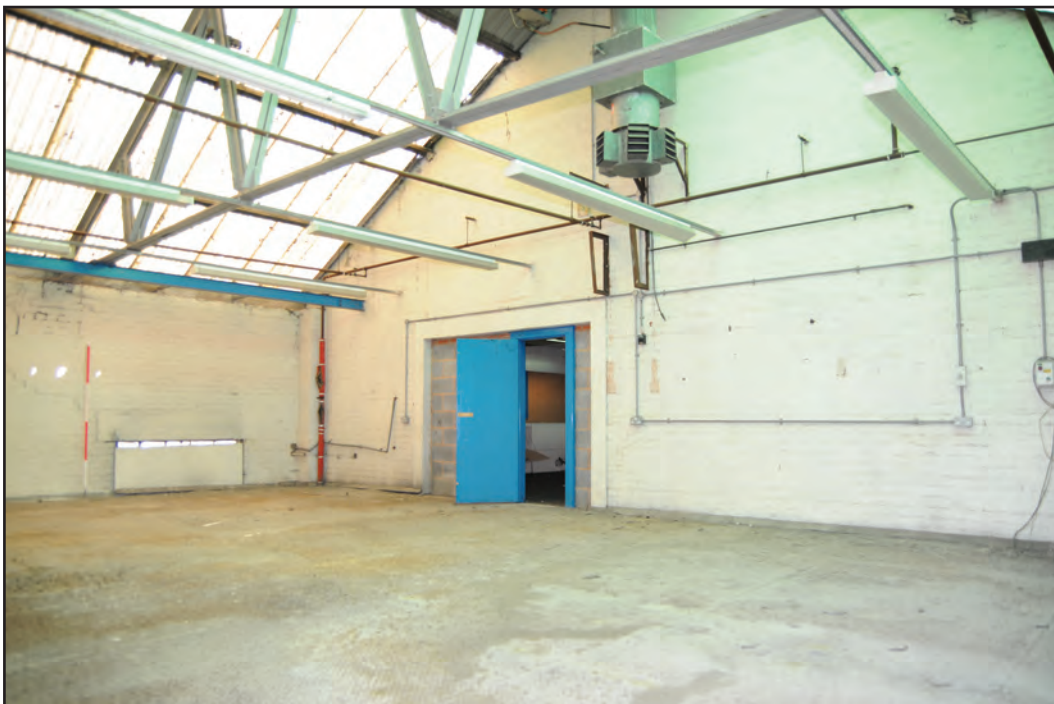
Photograph No. Washwood020 Description: Metal-floored room at west end of C6 Site Location: G9 Direction From: SW
