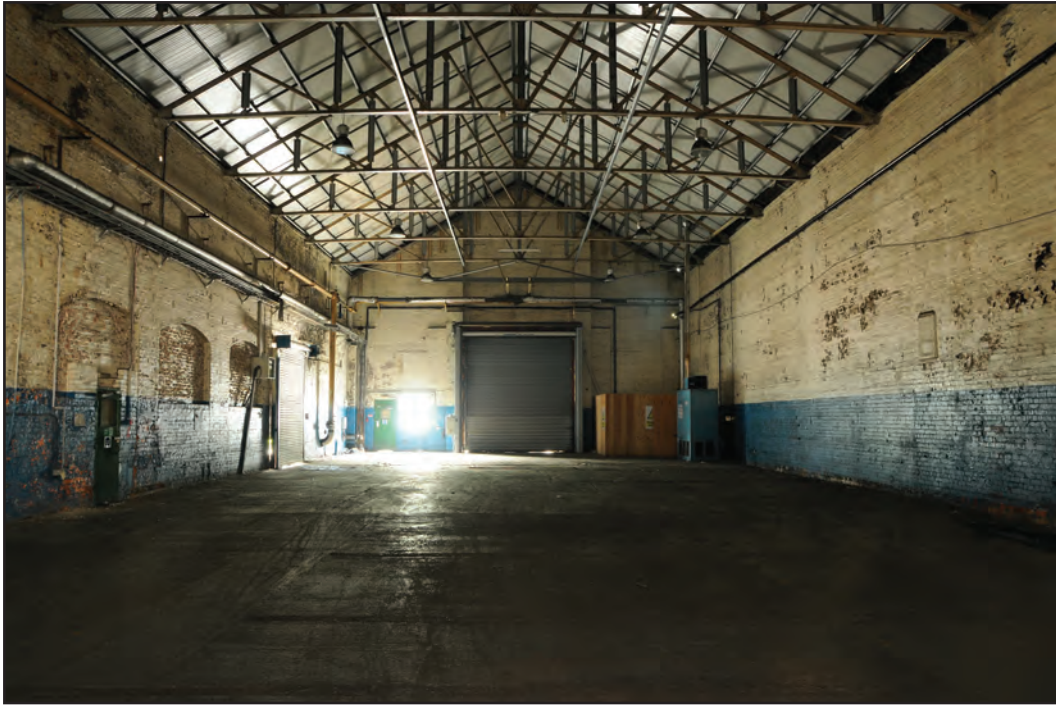
Photograph No. Washwood047 Description: Internal view of the shed Site Location: C6a Direction From: W
