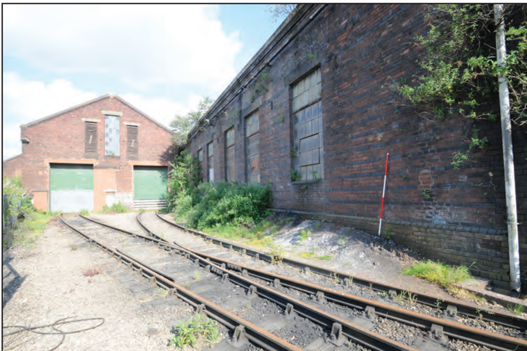
Photograph No. Washwood098 Description: F1 exterior north elevation and G4 exterior west gable end Site Location: F1/G4 Direction From: WNW
