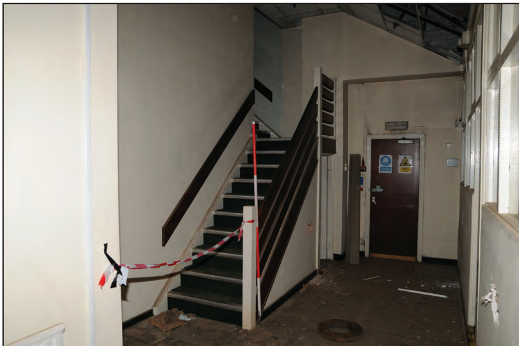
Photograph No. Washwood188 Description: Stairs within office area Site Location: A7 Direction From: ENE
