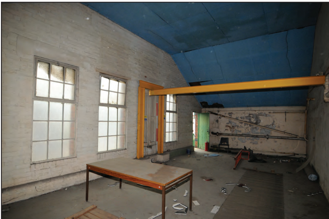
Photograph No. Washwood142 Description: Interior of first floor winch room Site Location: E3 Direction From: NE
