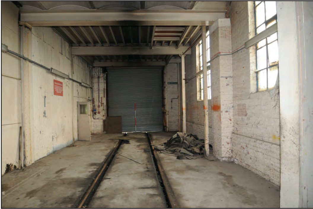
Photograph No. Washwood113 Description: Interior of train washing room, west end Site Location: G6c Direction From: E
