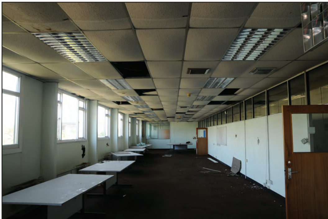
Photograph No. Washwood008 Description: Interior of largest office space Site Location: G5 Direction From: W
