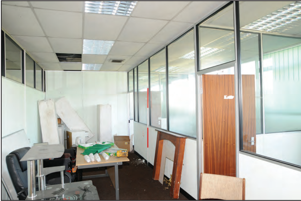
Photograph No. Washwoodo09 Description: Interior of offices with internal glass divisions Site Location: G5 Direction From: ESE
