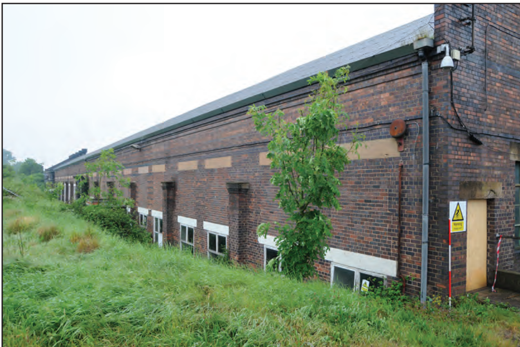
Photograph No. Washwood232 Description: Exterior south elevation at east end Site Location: A6 Direction From: ESE
