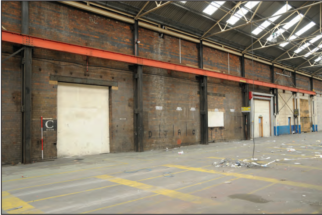
Photograph No. Washwood043 Description: Centre of west interior elevation, with wall signs Site Location: D10 Direction From: SE
