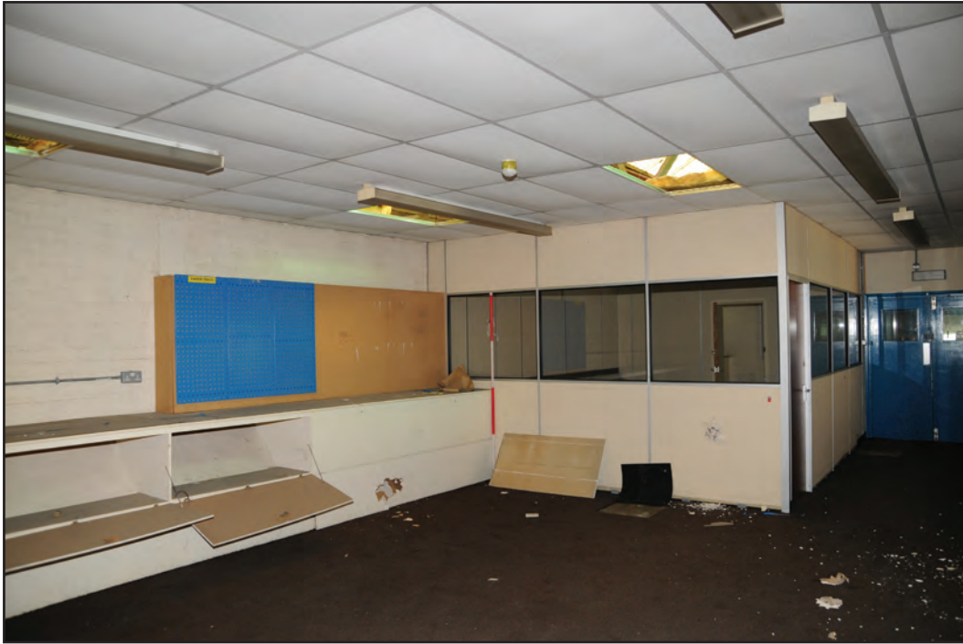
Photograph No. Washwood019 Description: Interior office divisions Site Location: G8 Direction From: SW
