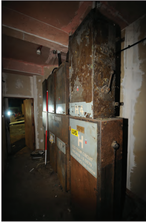
Photograph No. Washwood129 Description: Switch board/circuit breaker Site Location: H1 Direction From: SW
