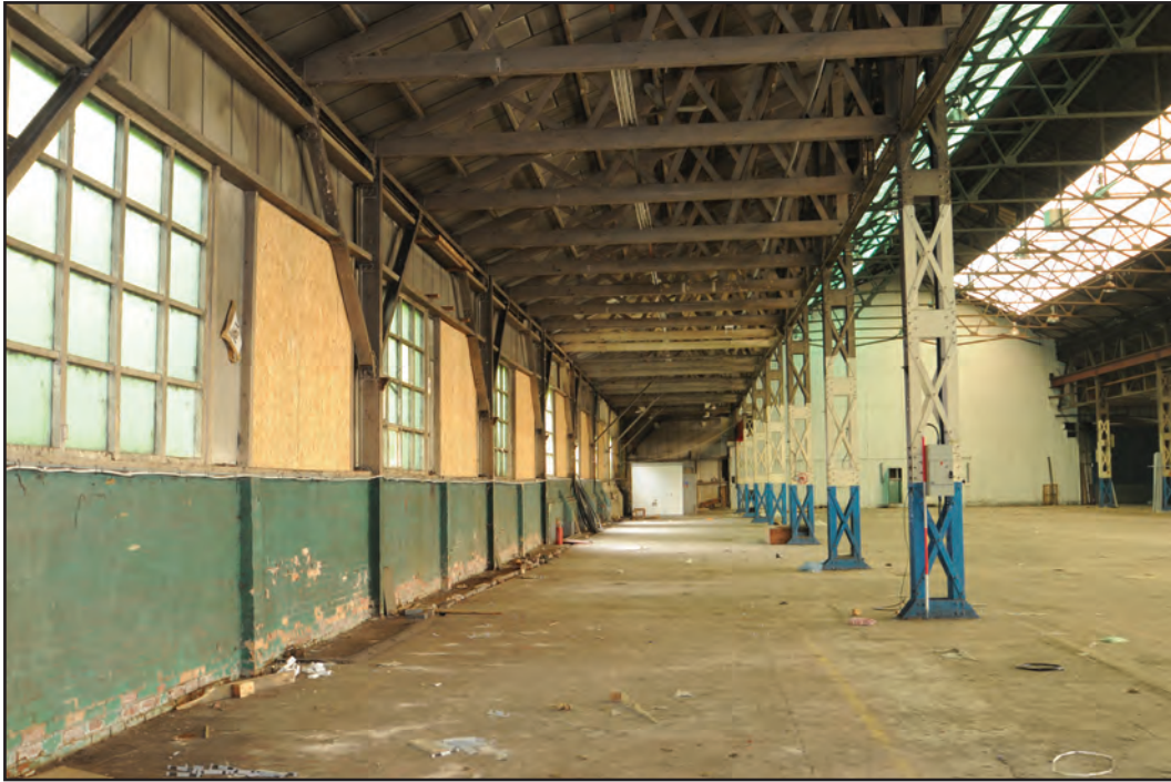
Photograph No. Washwood131 Description: View across south aisle Site Location: H1 Direction From: E
