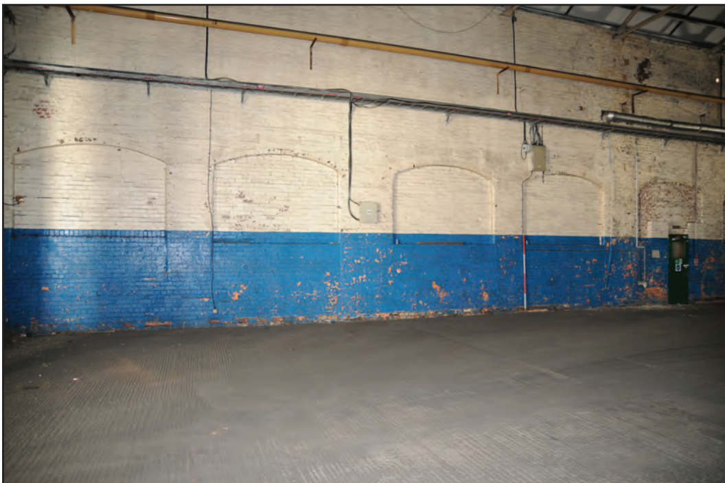
Photograph No. Washwood048 Description: Blocked openings at west end of north interior elevation Site Location: C6a Direction From: SW
