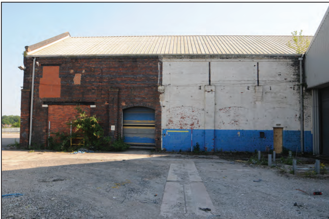
Photograph No. Washwood108 Description: Exterior north elevation with blocked openings (small, door and arched), brick pilasters and brick corbels Site Location: C6a Direction From: N
