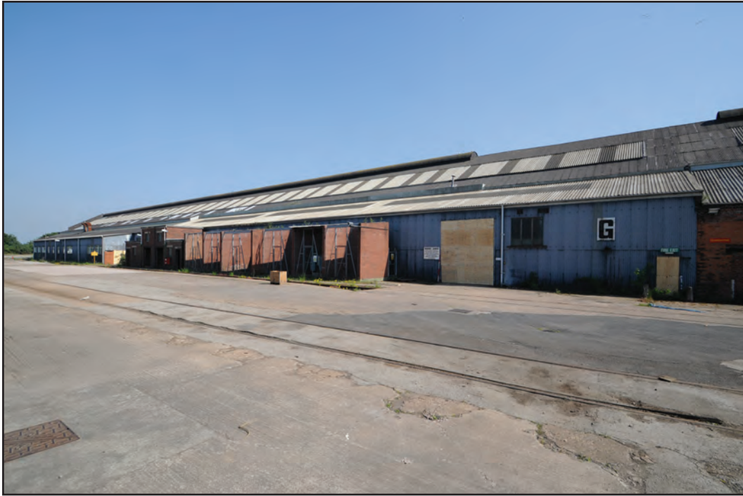
Photograph No. Washwood103 Description: Exterior north elevation of corrugated lean-to aisle Site Location: G2 Direction From: NW
