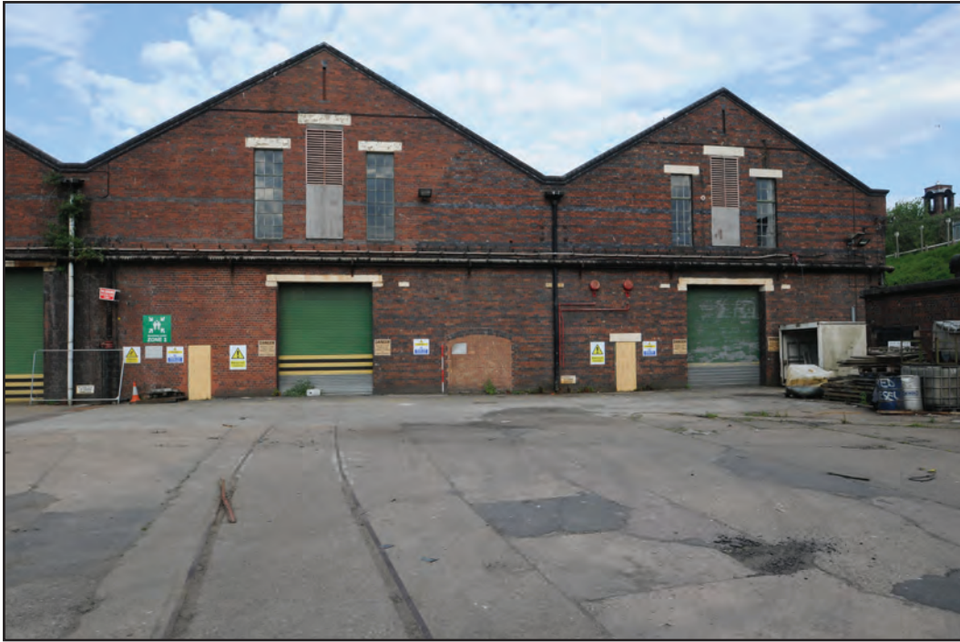
Photograph No. Washwood155 Description: Exterior west gable ends Site Location: B5/B6 Direction From: W
