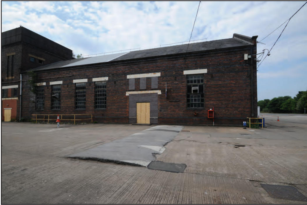
Photograph No. Washwood147 Description: Exterior south elevation Site Location: C6c Direction From: SSE
