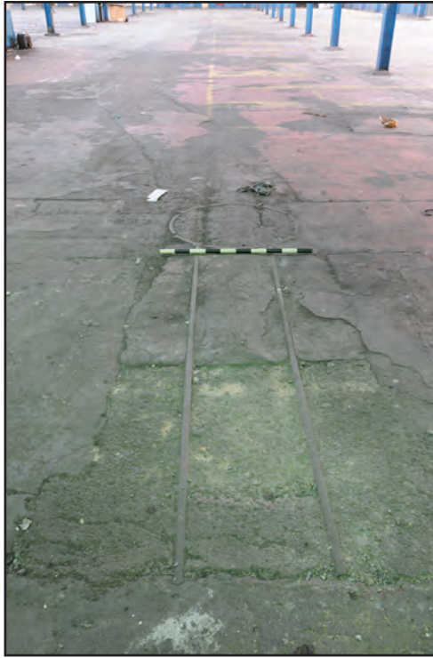
Photograph No. Washwood075 Description: Cart rail with turning circle at interior west end of shed Site Location: D8 Direction From: W
