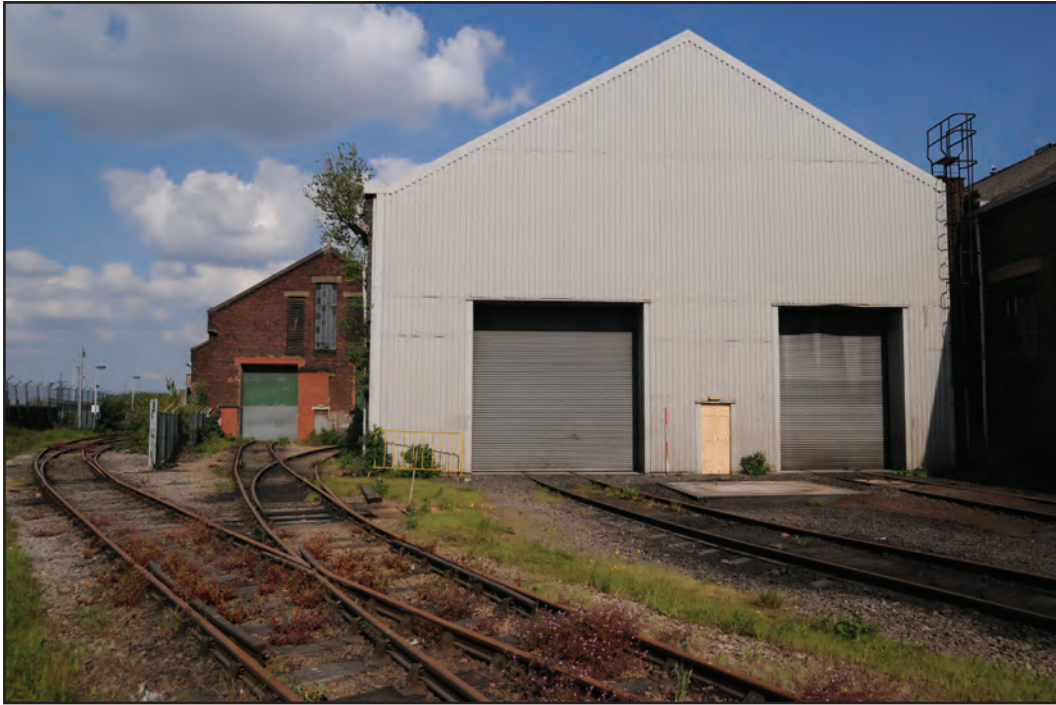
Photograph No. Washwood097 Description: Exterior west metal paneled gable end Site Location: F1 Direction From: W
