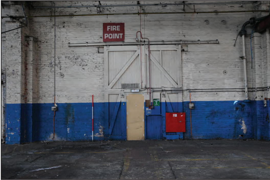
Photograph No. Washwood071 Description: Sliding door on internal east gable end Site Location: D8 Direction From: W
