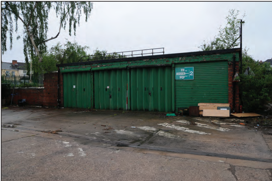
Photograph No. Washwood236 Description: Exterior north elevation Site Location: Firehouse? Direction From: NW
