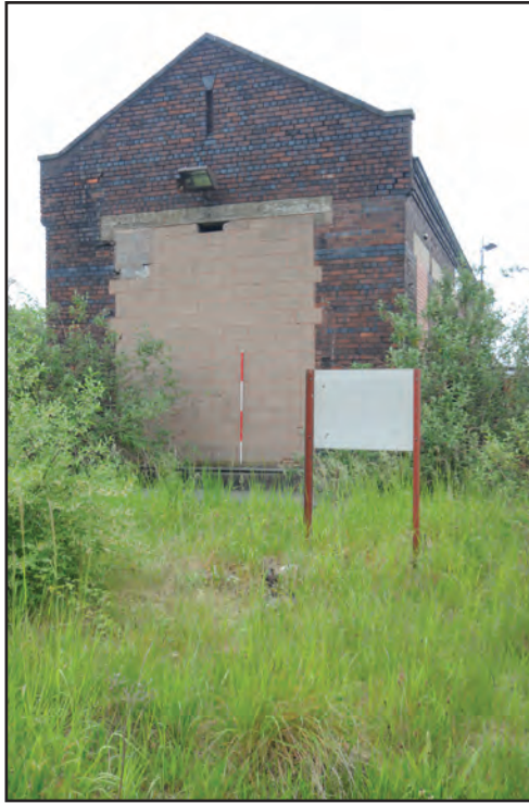
Photograph No. Washwood119 Description: Exterior west elevation with blocked roller door Site Location: Loco shed Direction From: WSW
