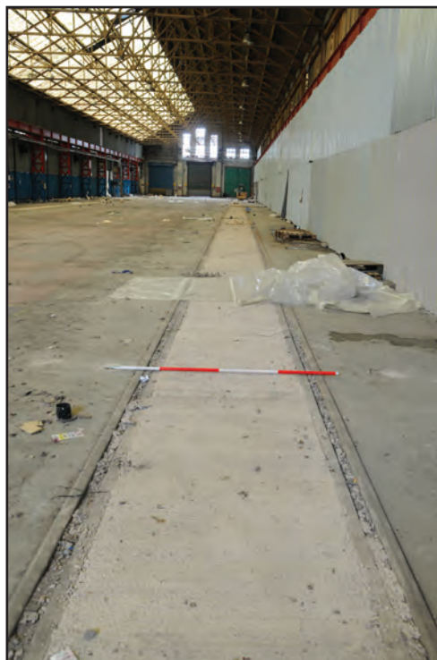
Photograph No. Washwood202 Description: Train rails oriented east-west at south side of shed interior with modern concrete infill of inspection trench Site Location: B2 Direction From: W
