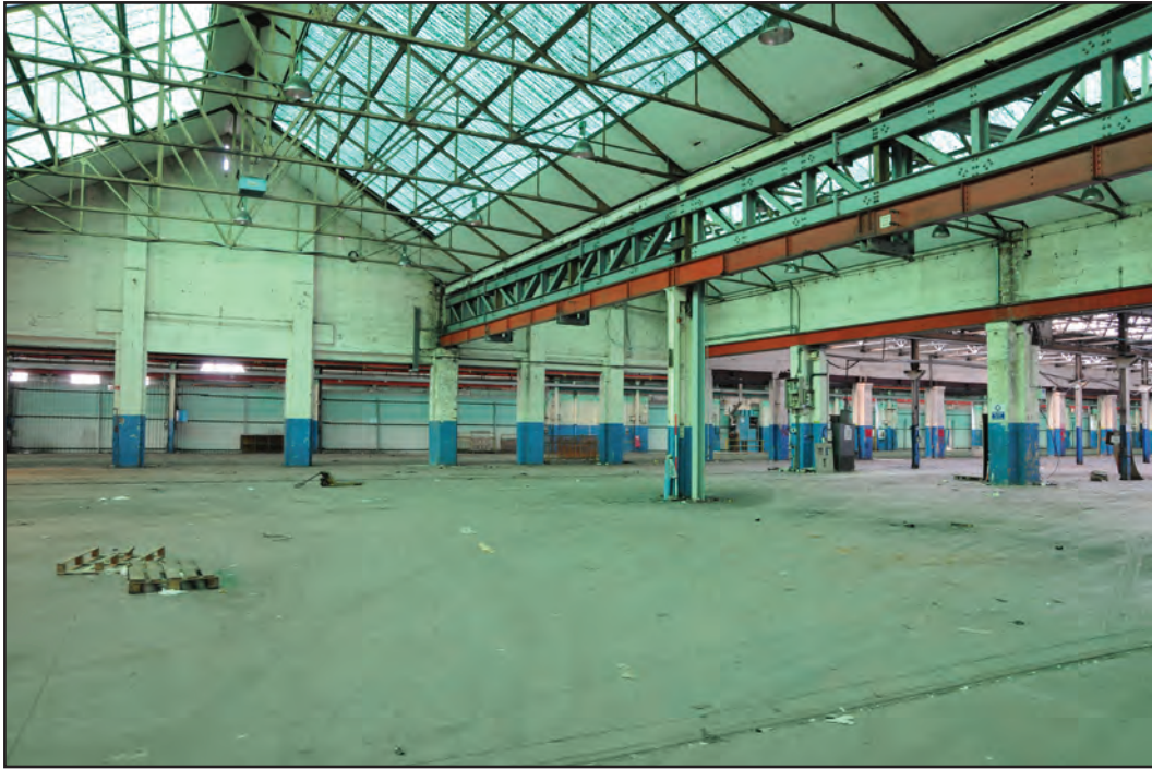
Photograph No. Washwood077 Description: Interior north gable ends of sheds Site Location: E1/E2 Direction From: SSW
