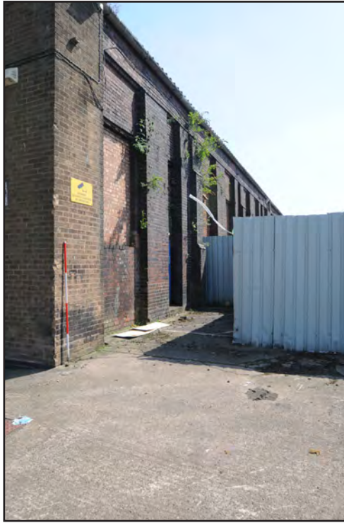
Photograph No. Saltley065 Description: Exterior west elevation, north end Site Location: Anixter Direction From: NNW
