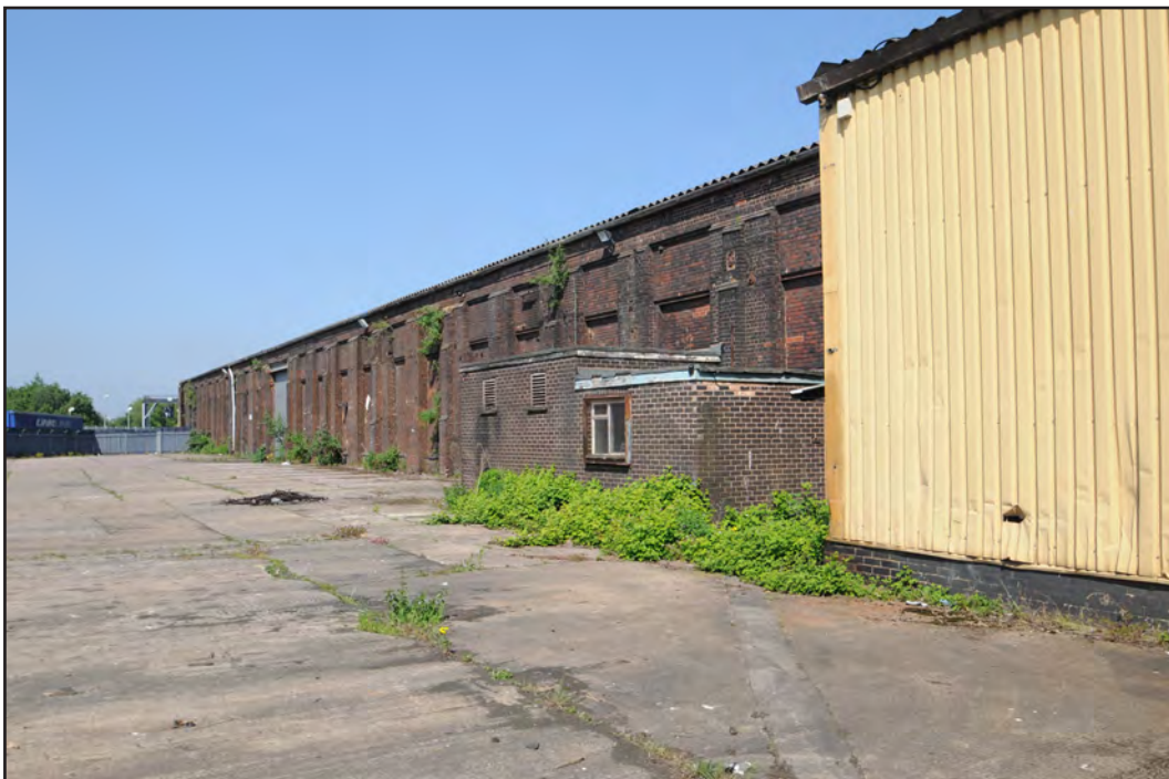
Photograph No. Saltleyo68 Description: Exterior west elevation, central area Site Location: Anixter Direction From: SW
