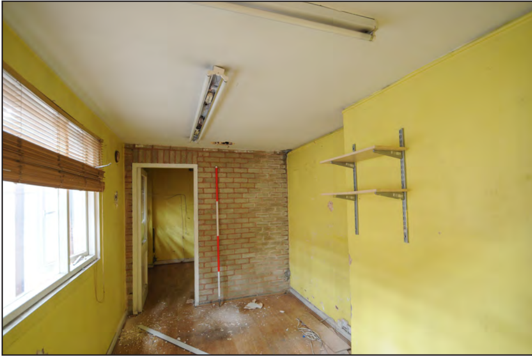
Photograph No. Saltley005 Description: General view of office space interior Site Location: Unit 3 Direction From: E
