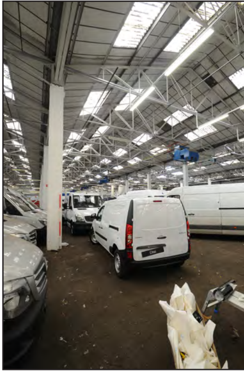
Photograph No. Saltley021 Description: Detail view of stanchion and roof trusses Site Location: Mercedes-Benz Direction From: NNE
