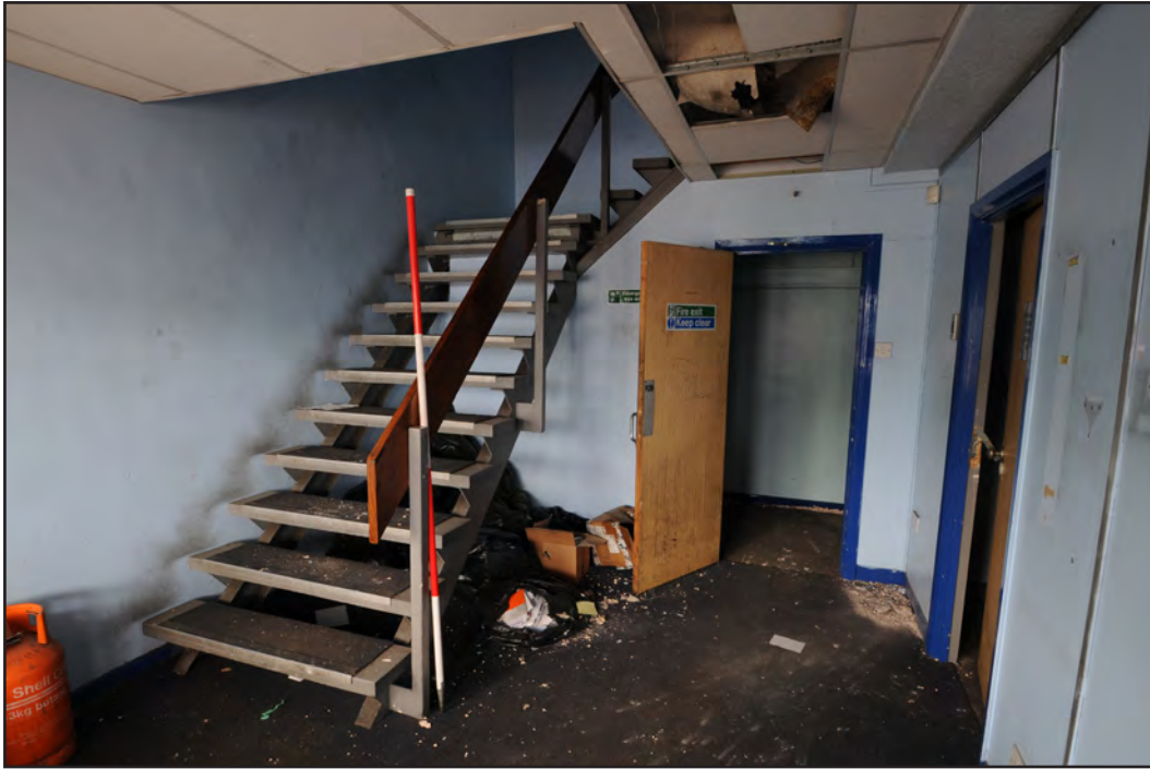
Photograph No. Saltley073 Description: Stairway at northwest corner of building Site Location: Unit 5 Direction From: SW
