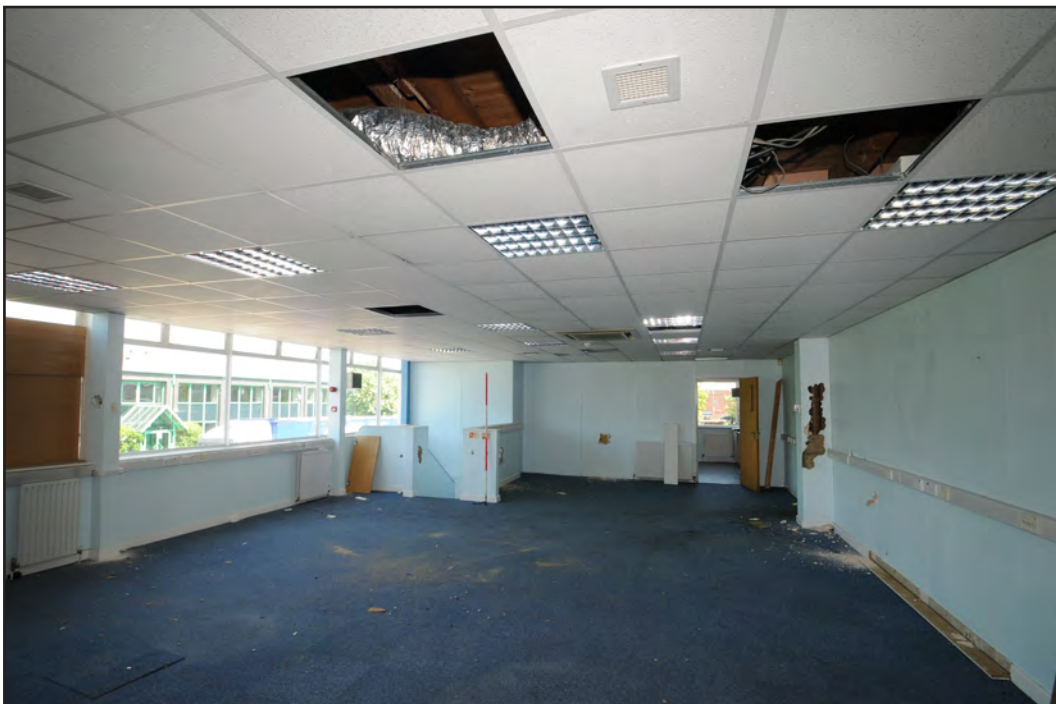
Photograph No. Saltley050 Description: General view of 1st floor office space Site Location: Anixter Direction From: SW
