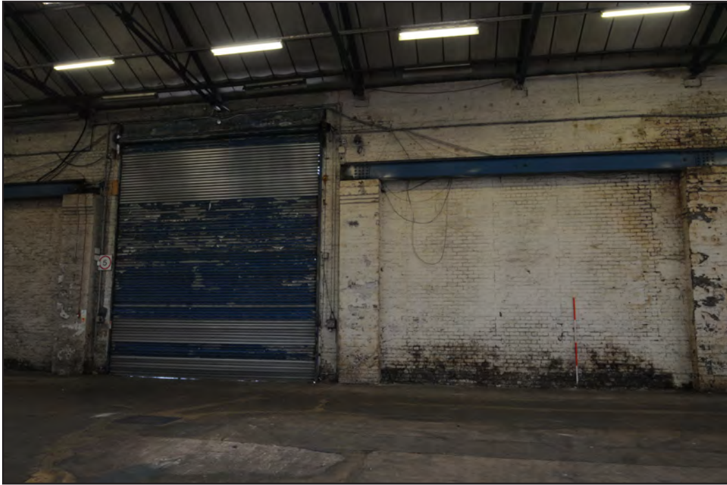
Photograph No. Saltley053 Description: Internal west wall, south end Site Location: Anixter Direction From: NE
