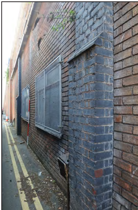
Photograph No. Saltley058 Description: Windows of office space at south end of exterior east elevation Site Location: Anixter Direction From: NNE
