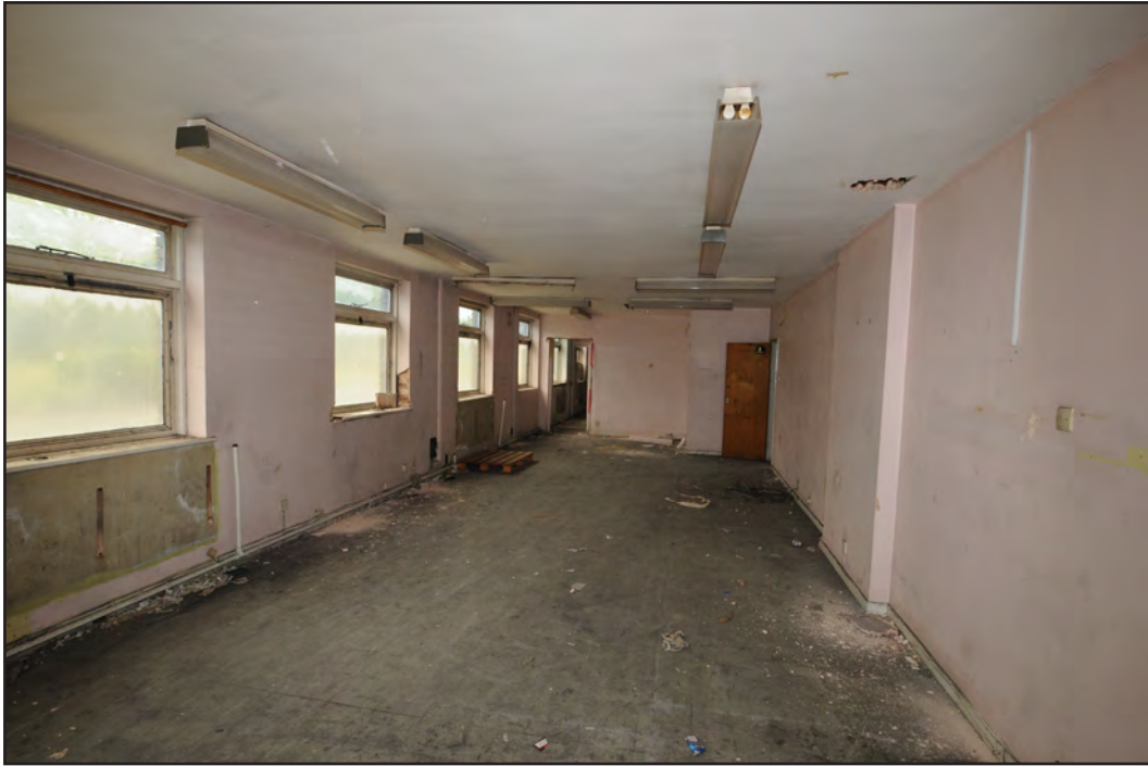
Photograph No. Saltley071 Description: Ground floor office space Site Location: Unit 5 Direction From: SSE
