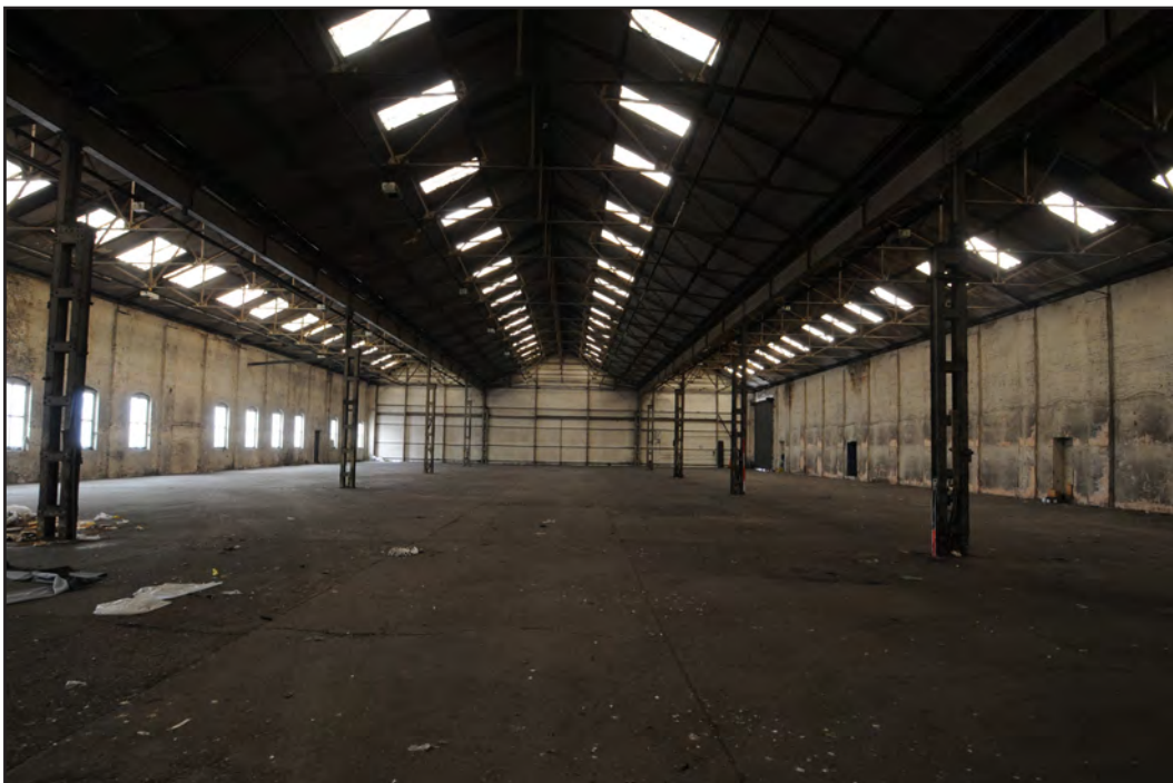
Photograph No. Saltley074 Description: General view of shed interior Site Location: Unit 5 Direction From: N
