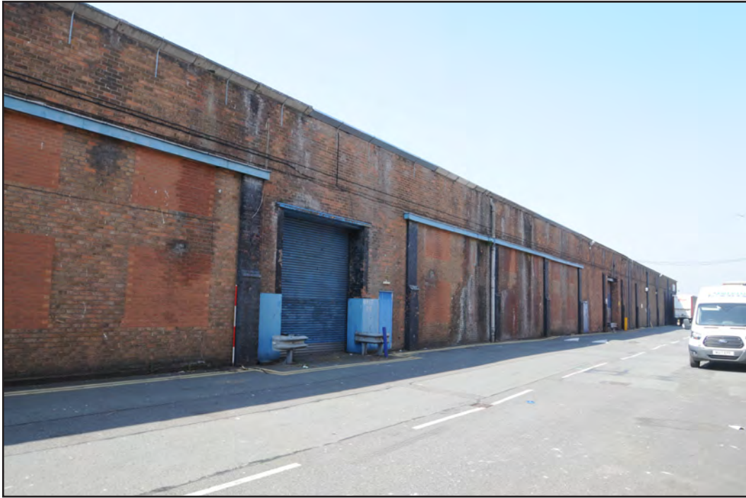
Photograph No. Saltley059 Description: Exterior east elevation, central area Site Location: Anixter Direction From: SE
