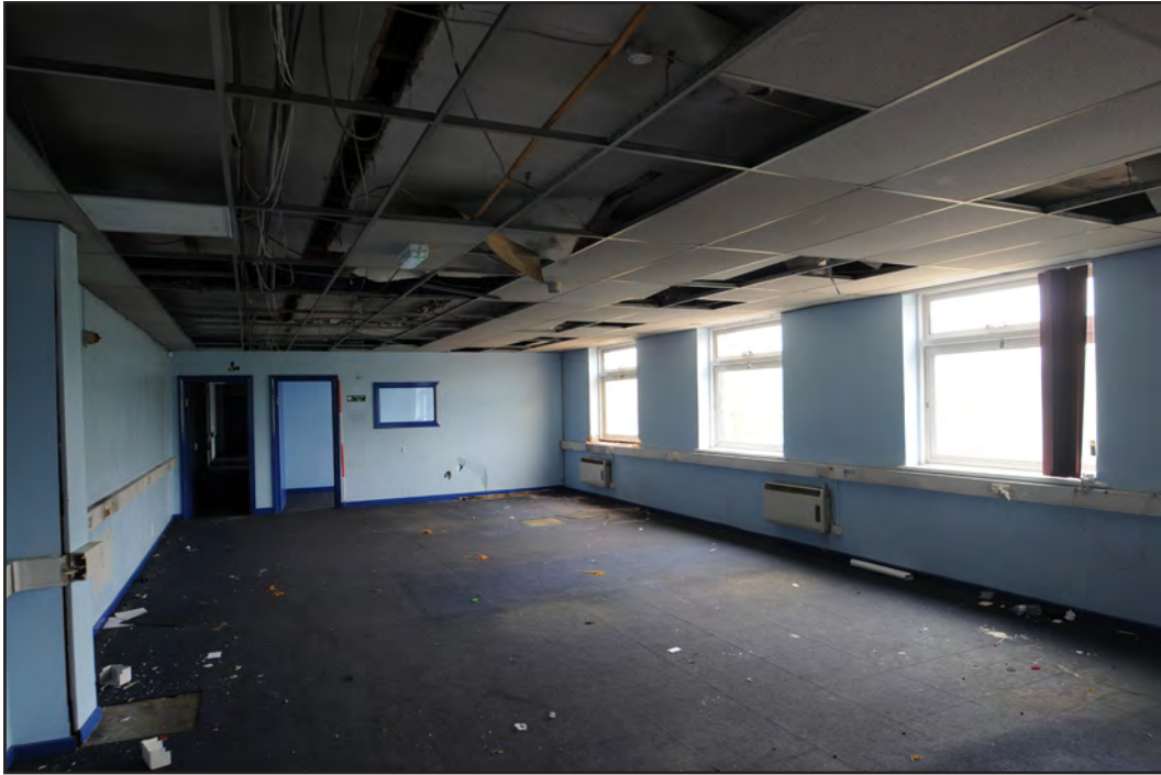
Photograph No. Saltley069 Description: 1st floor office space Site Location: Unit 5 Direction From: NNE
