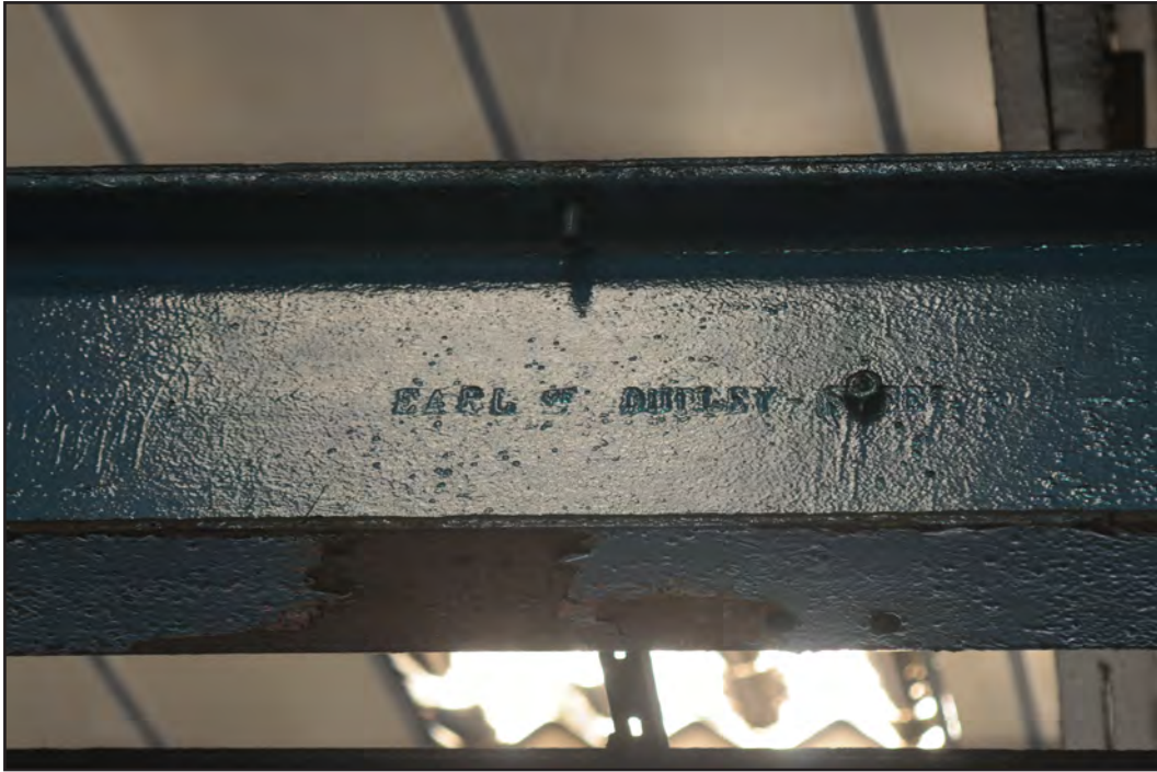
Photograph No. Saltley045 Description: EARL OF DUDLEY STEEL foundry mark on rail above stanchions at northeast interior corner of buildings Site Location: Anixter Direction From: E
