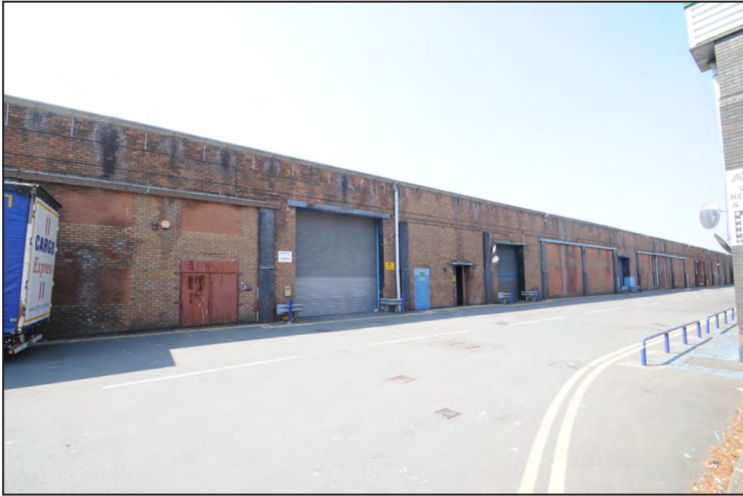
Photograph No. Saltley057 Description: Exterior east elevation, south end Site Location: Anixter Direction From: SE
