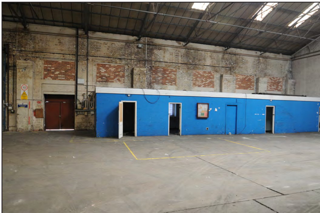
Photograph No. Saltley040 Description: southeast interior corner of sheds with brick offices and blocked openings Site Location: Anixter Direction From: WNW
