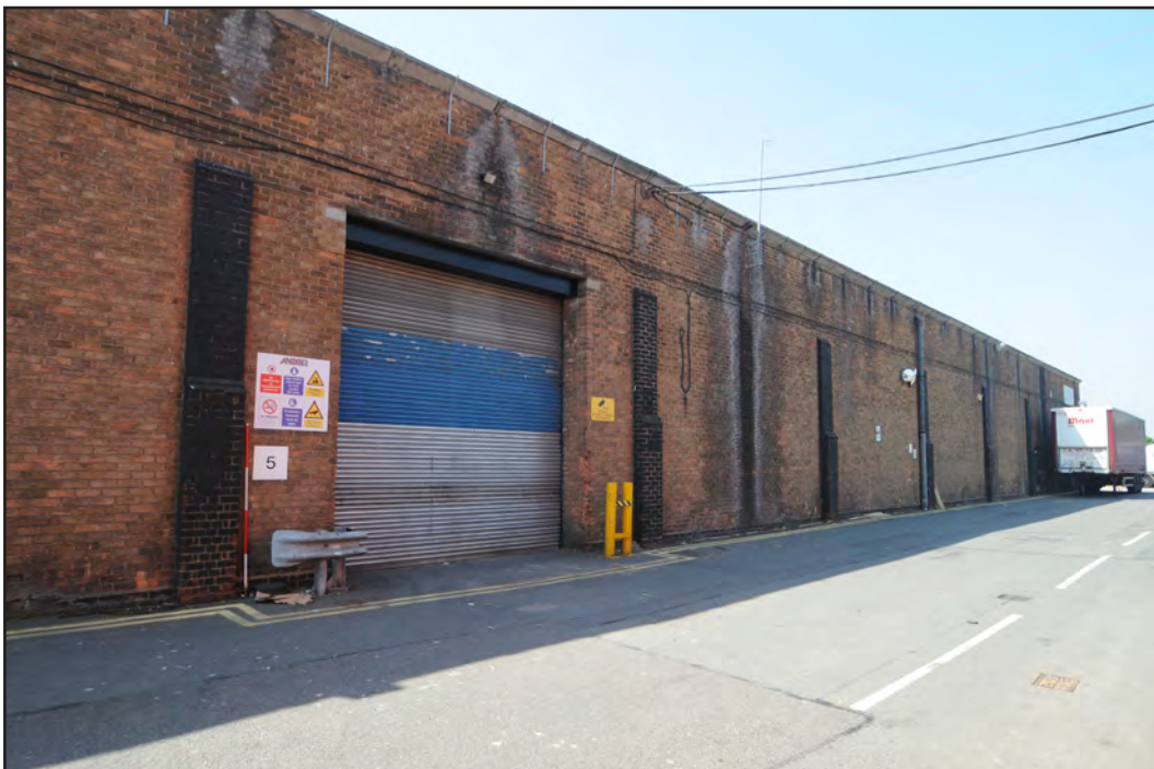
Photograph No. Saltley060 Description: Exterior east elevation, north end of shed Site Location: Anixter Direction From: SE
