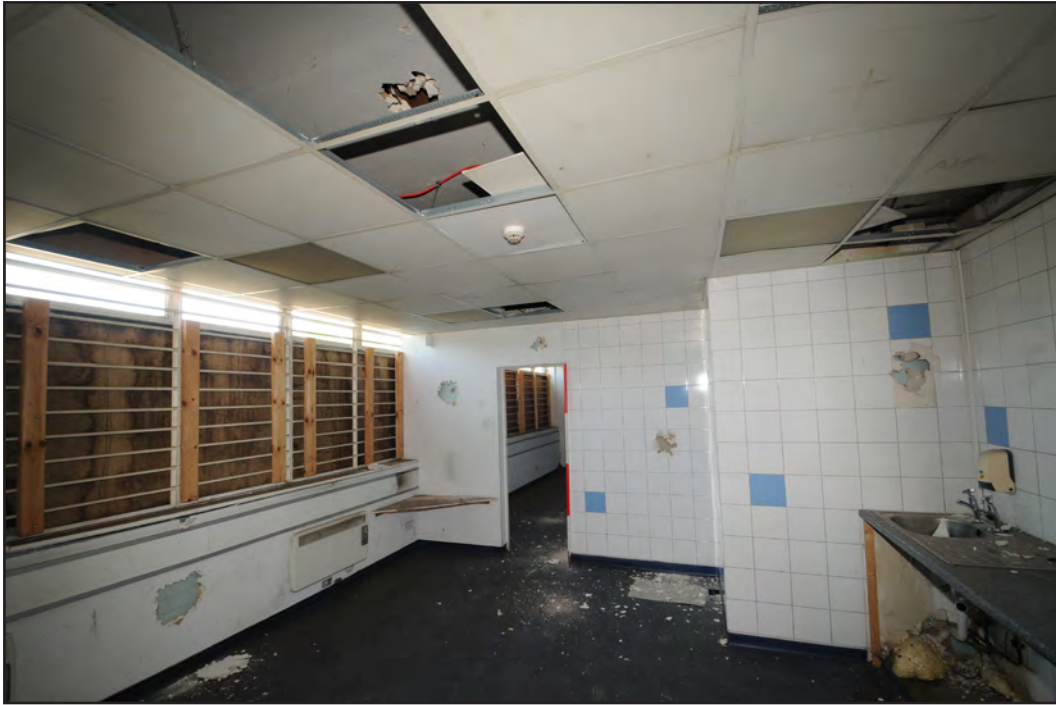
Photograph No. Saltley051 Description: Kitchen as part of office space at northwest of building Site Location: Anixter Direction From: WSW
