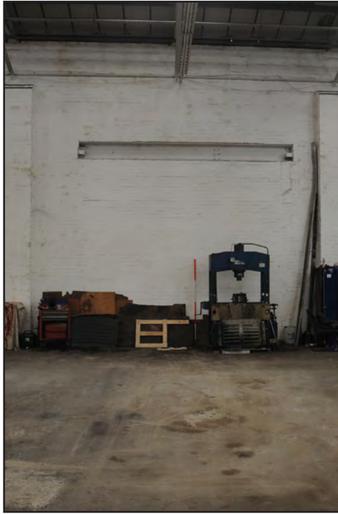
Photograph No. Saltley023 Description: Detail of blocked entrance at north end of east wall Site Location: Mercedes-Benz Direction From: W
