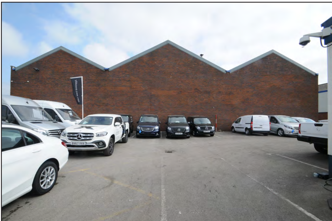
Photograph No. Saltley008 Description: General view of exterior south gable wall Site Location: Unit 3 Direction From: S
