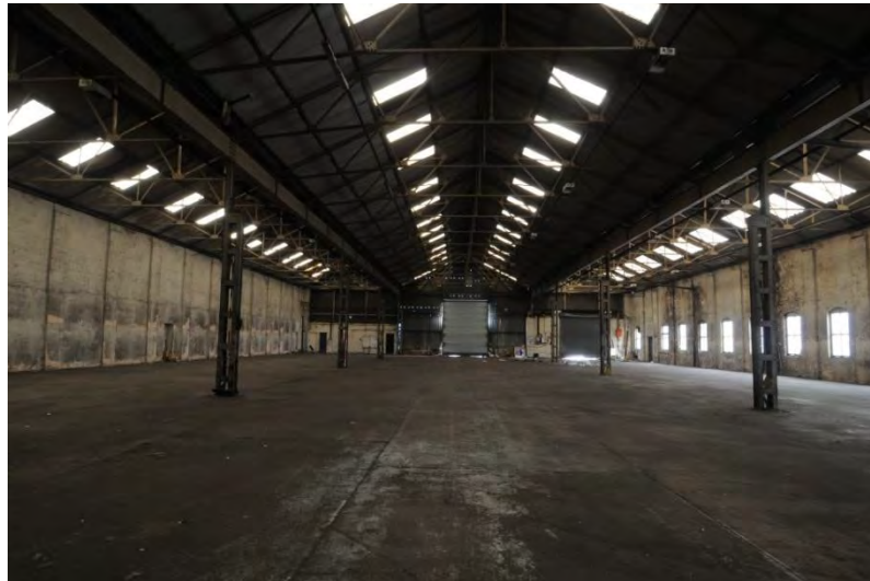
Plate 7 Interior of Unit 5 (Shed C) with the blocked window openings to the left of the picture
