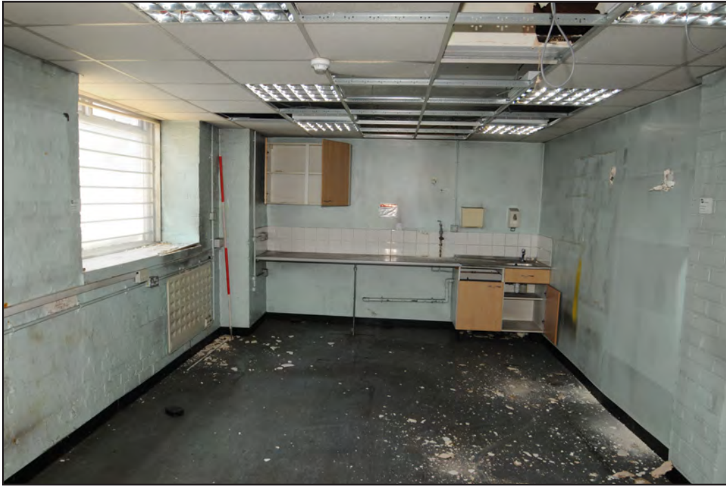
Photograph No. Saltley037 Description: Interior view of brick office kitchen space Site Location: Anixter Direction From: N
