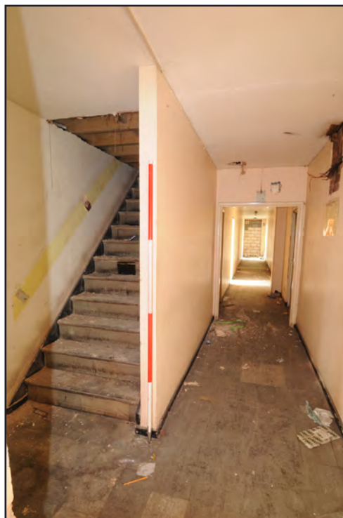
Photograph No. Saltley072 Description: Corridor and truncated stairway Site Location: Unit 5 Direction From: SSE
