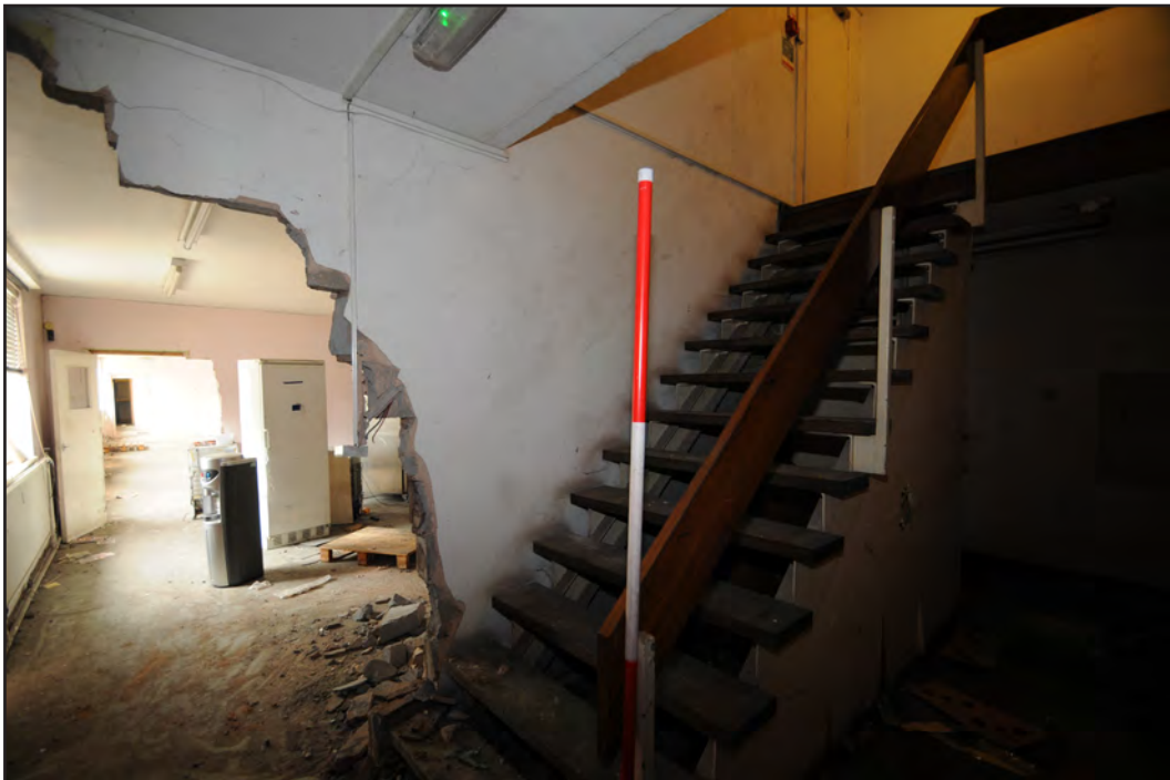
Photograph No. Saltley070 Description: Stairway at southwest corner of building Site Location: Unit 5 Direction From: SW
