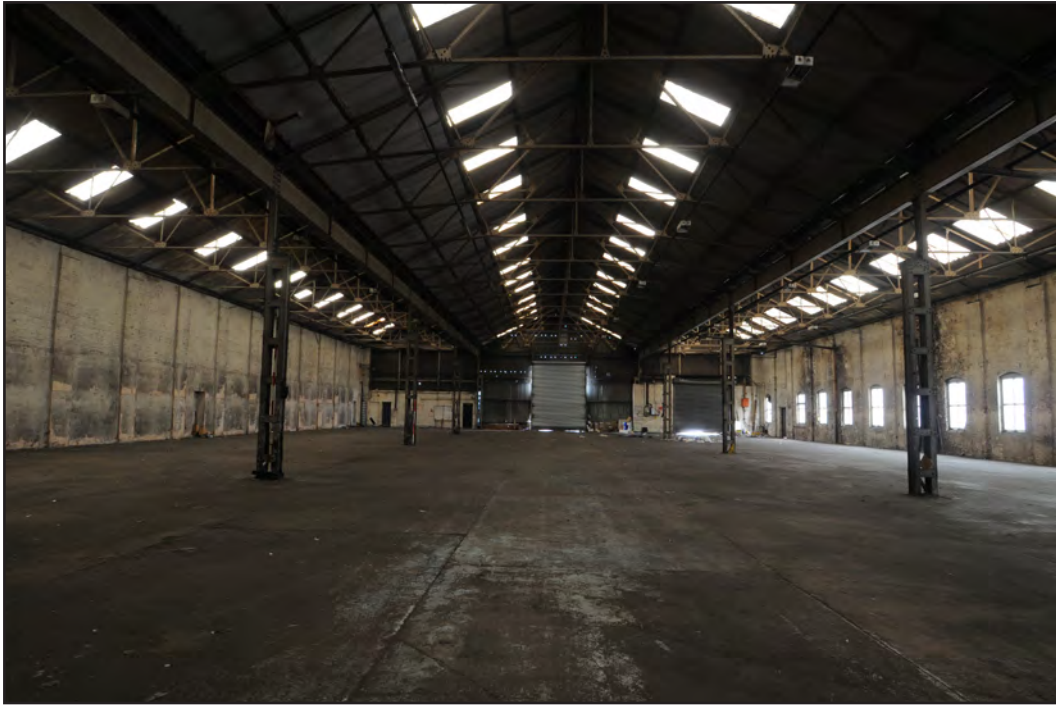
Photograph No. Saltley075 Description: General view of shed interior Site Location: Unit 5 Direction From: S
