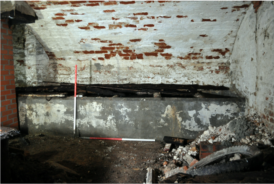
Plate 7: Cell 1 looking north showing row of vats along north wall. 1m scales.
