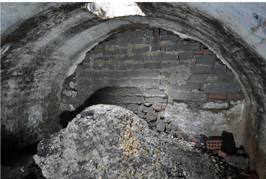
Plate 12: Cell 2 looking west showing rebuilt west wall and access through opening in vault.
