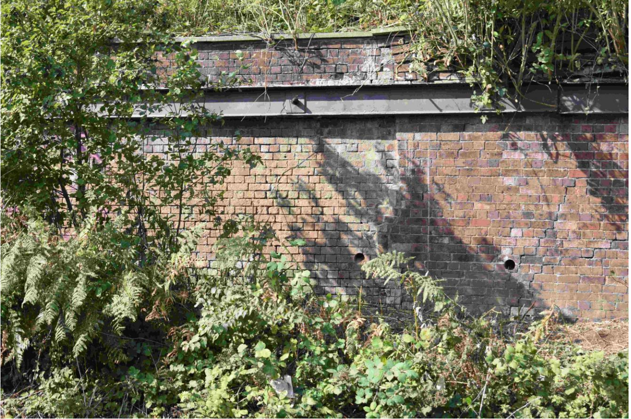
Plate 19: Structural break in Section C with earlier brickwork to left (c.1830s) and slightly later to right (taken 21 September 2020)
