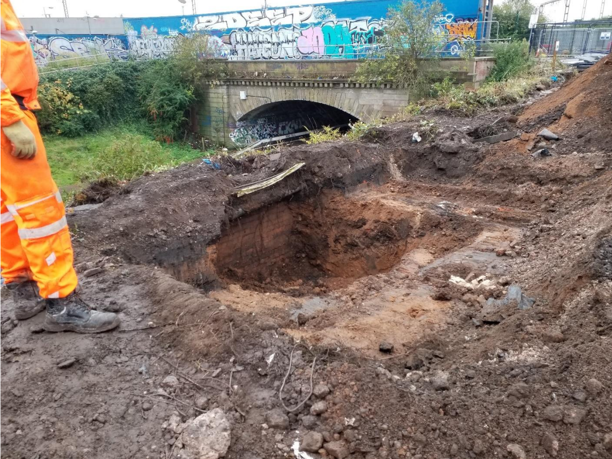
Plate 34: Wall exposed in excavation works to west of canal (photo taken 2 October 2020 by LM)
