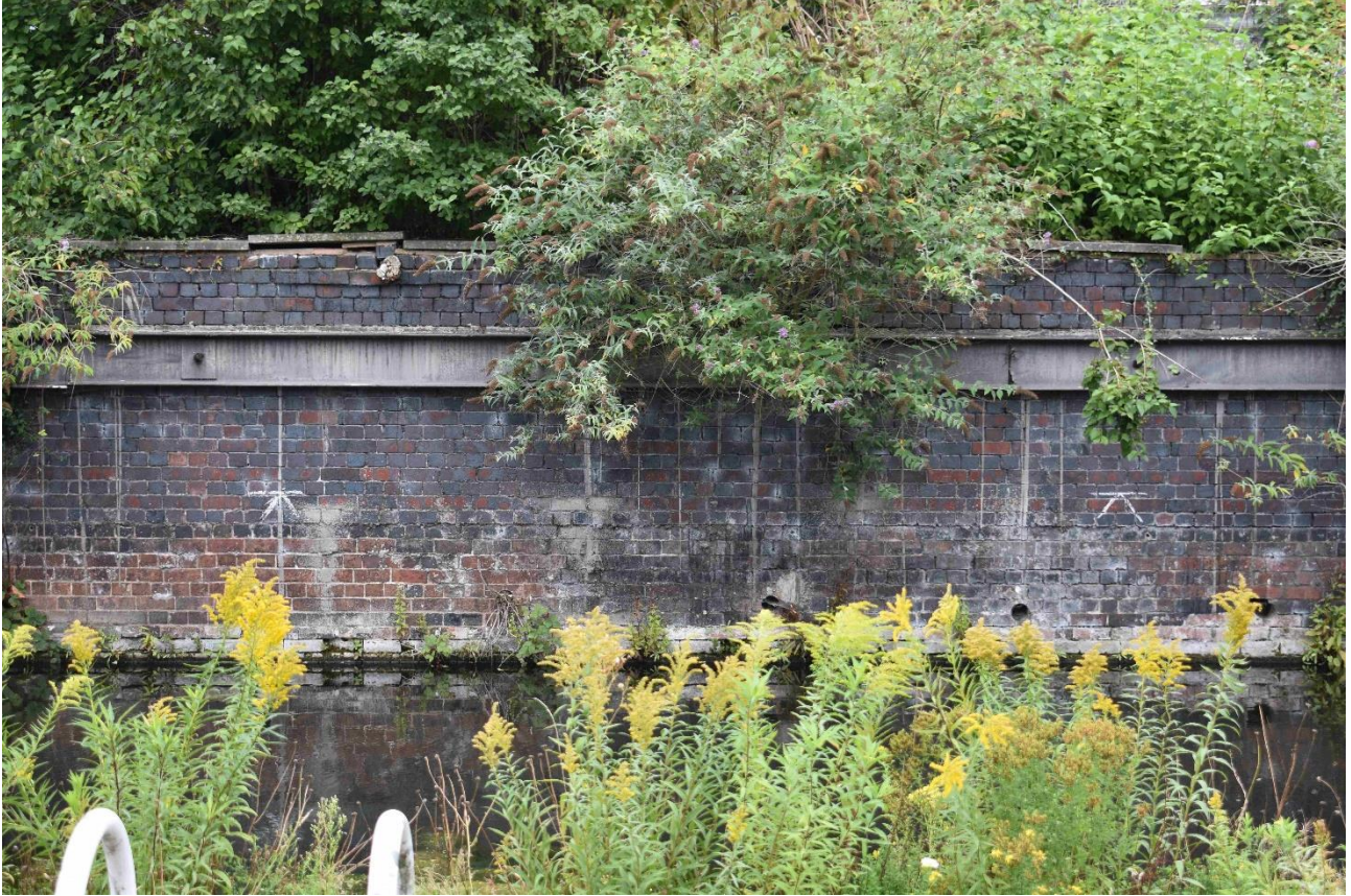
Plate 8: Section B (central part of the canal wall) taken 14 August 2020. Note the lower 10 courses older than courses above. Also note vegetation and poor condition of the canal wall
