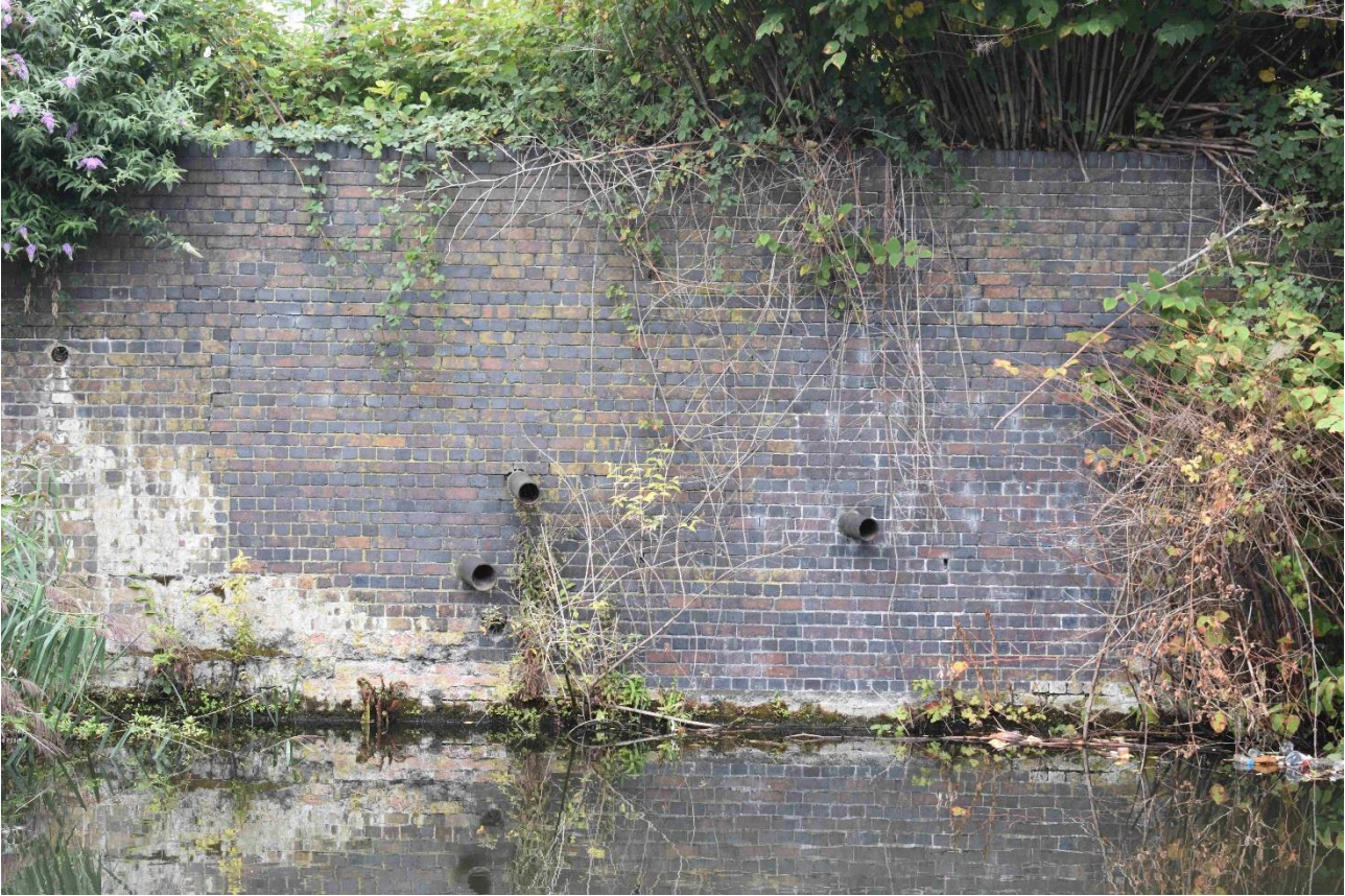
Plate 5: North section of the canal wall (Section A) taken 14 August 2020. Note vertical break towards left edge of image with yellow bricks to south (possibly late 19th or early 20th-century rebuild) and red/blue bands of brick to north (late 19th century) which was favoured by the LNWR. The upper 10 courses across both areas are from a later phase when the canal wall was raised.
