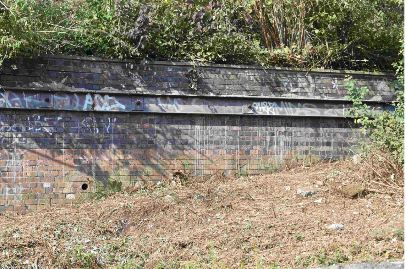
Plate 18: Northern part of Section C after vegetation removal (taken 21 September 2020). The lower part of the brickwork here may be mid-late 19th century while the darker upper part may be late 19th or early 20th century.
