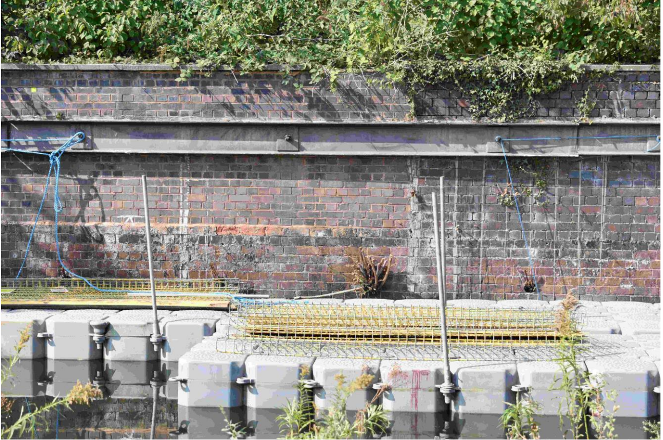
Plate 25: Structural break in Section B after vegetation removal (taken 21 September 2020)
