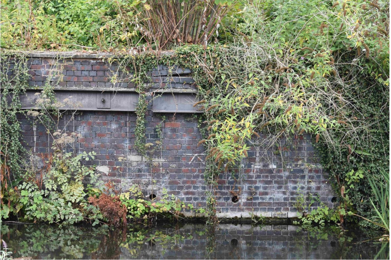
Plate 6: Section B (central part of the canal wall). Note extent of vegetation cover and bulging of brickwork towards top of the canal wall (taken 14 August 2020)
