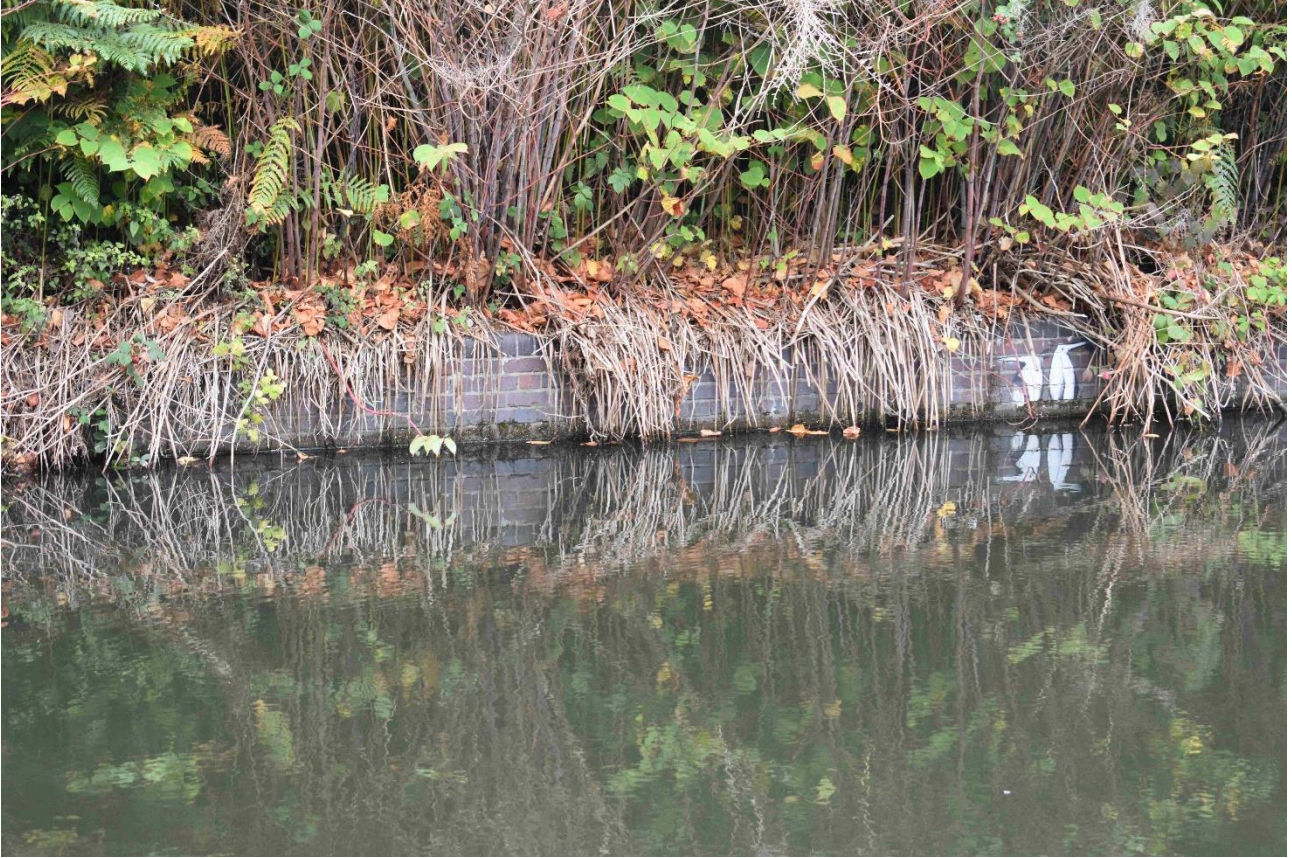
Plate 12: Low part of the southern section of the canal wall (Section C). Taken 14 August 2020
