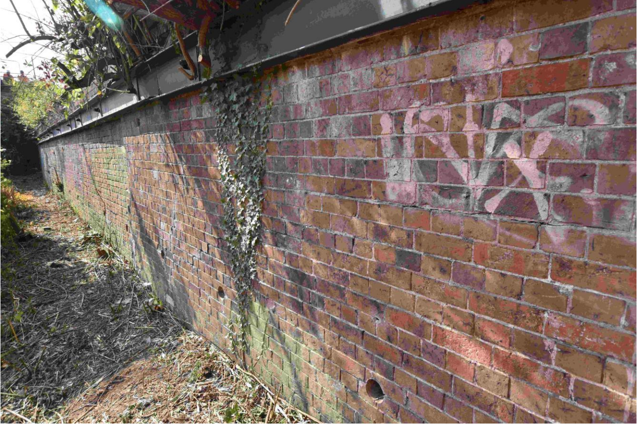
Plate 23: Section C looking southwards (taken 21 September 2020). The brickwork in the foreground is probably mid 19th-century in date and slightly later than the 1838 brickwork in the distance.
