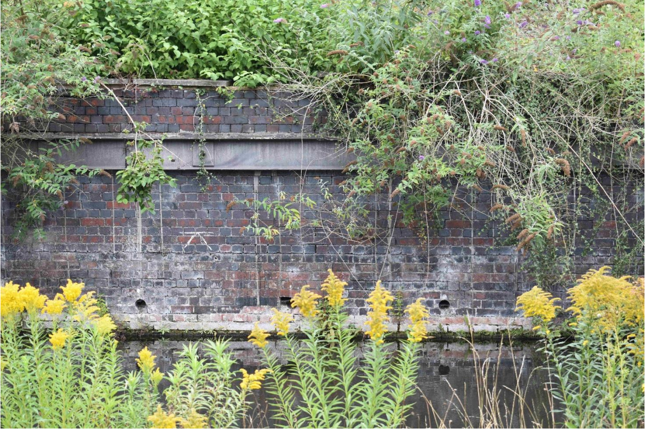
Plate 7: Section B (central part of the canal wall) taken 14 August 2020. Note the lower 10 courses (probably mid to late 19th century) older than courses above.
