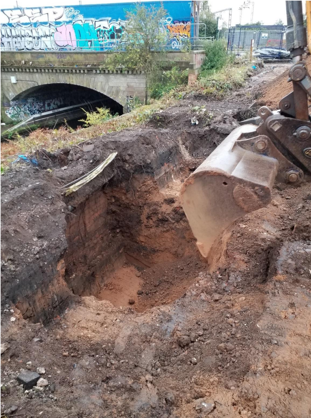
Plate 33: Wall exposed in excavation works to west of canal (photo taken 2 October 2020 by LM)
