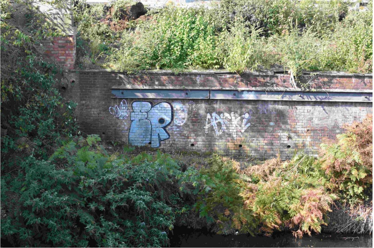
Plate 21: Southern end of Section C, adjacent to 1838 railway bridge, after vegetation removal (taken 21 September 2020). This brickwork is probably largely contemporary with the 1838 bridge.
