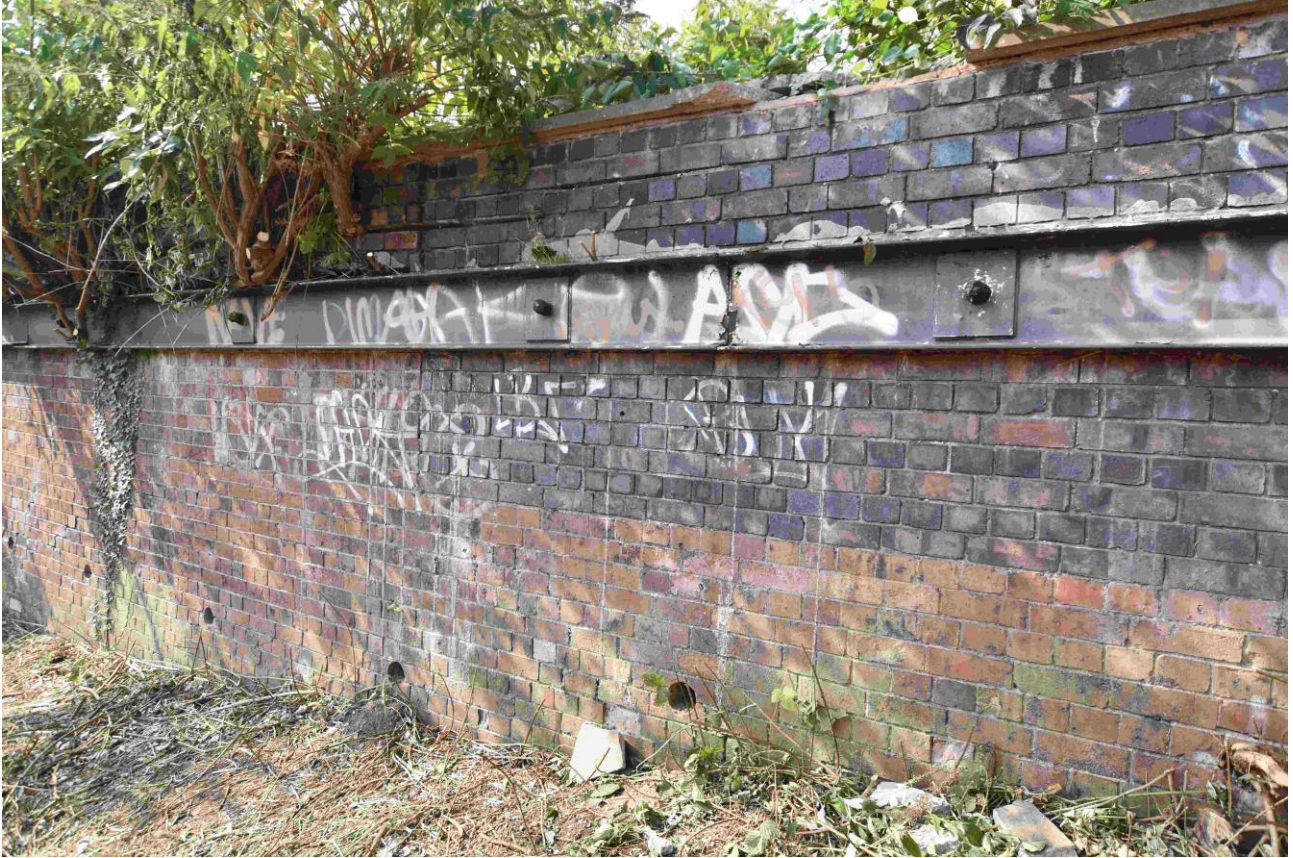
Plate 24: Northern part of Section C with later area of dark blue brick (taken 21 September 2020)
