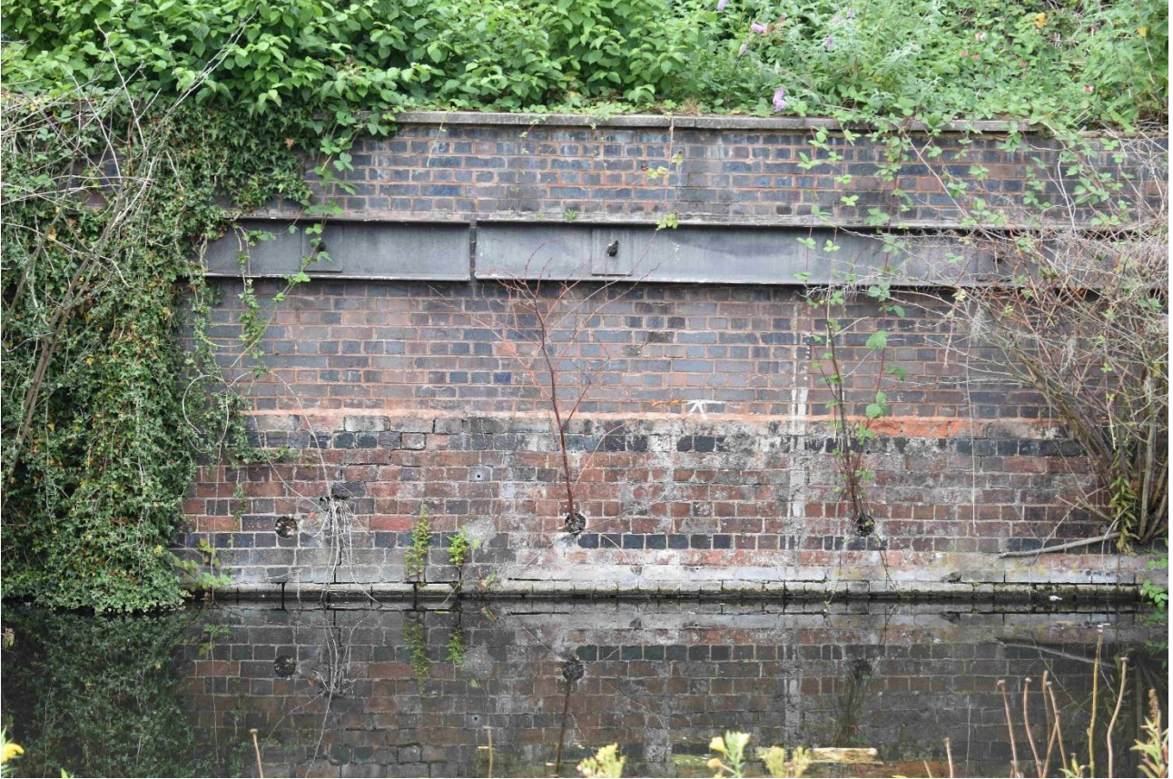
Plate 10: Southern end of Section B (central part of the canal wall) with lower 10 courses possibly mid 19th century in date and upper part of wall (c.19 courses) dating to a much later rebuild (late 20th or 21st century). Taken 14 August 2020
