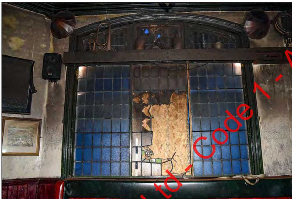
Plate 48: Damaged window facing Banbury Street
