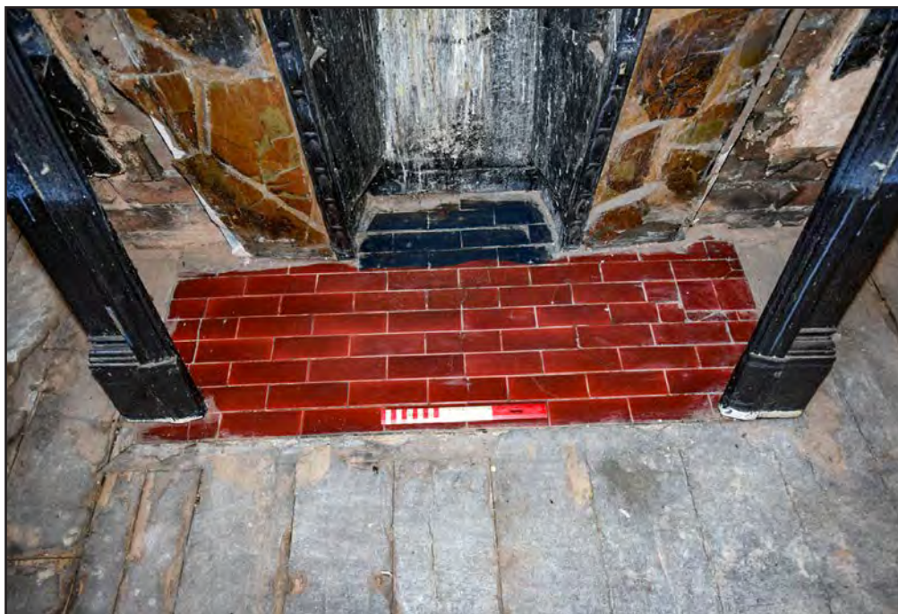
Plate 139: Fireplace at east end of Room F1 showing hearth exposed during works
