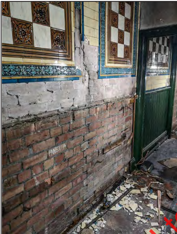
Plate 82: Former corridor after removal of mid-height boarding (photograph taken by Holland Contracting)
