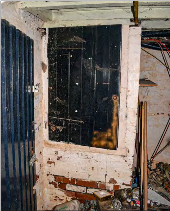
Plate 115: Enclosure for safe in room B3
