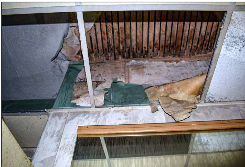
Plate 151: Lath and plaster visible in F6c above modern ceiling
