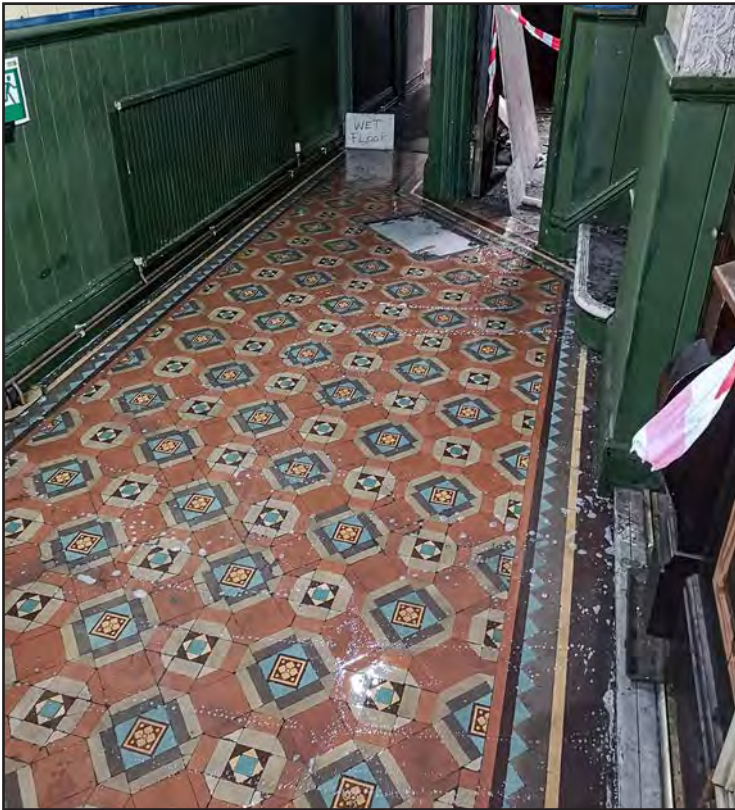
Plate 71: Decorative floor tiles in former corridor to east side of pub (photograph taken by Holland Contracting)
