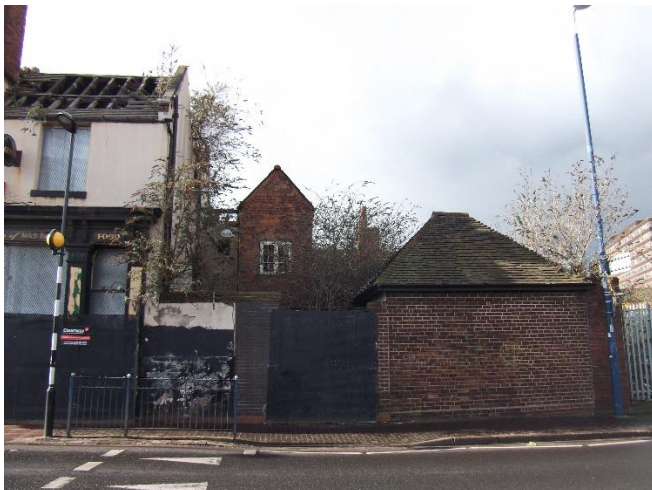
C: Additions to the rear of Freeman Street, accessed from Park Street, showing the toilet block and stair turret (east elevation)
