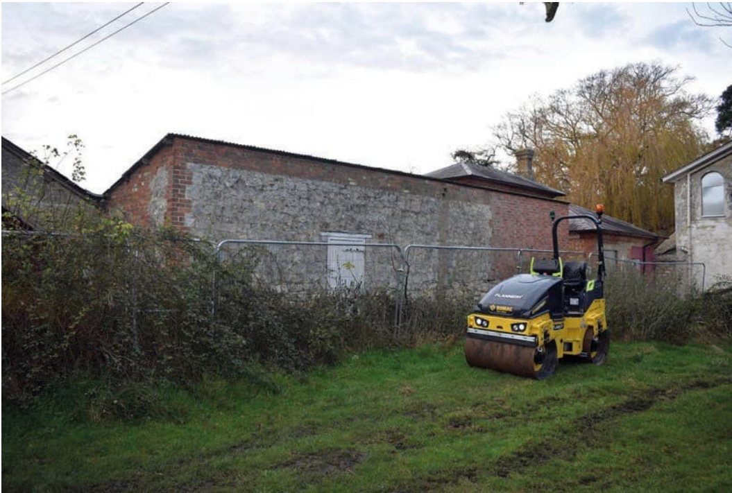
Photo B 93: General aspect towards the north west from within the rear garden area
