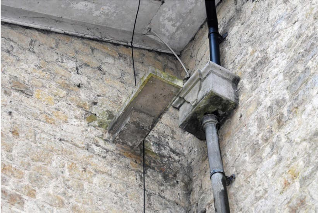
Photo B 20: Stone corbel in north east corner with decorative stone hopper adjacent
