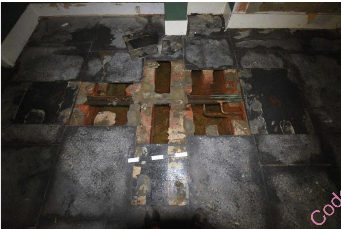
Photo B 35: Brick sub-floor structure beneath slate floor in rear room G1
