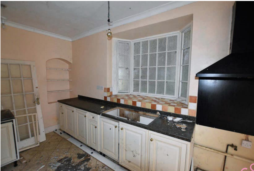
Photo B 82: East kitchen area G6 facing west with alcove in west wall
