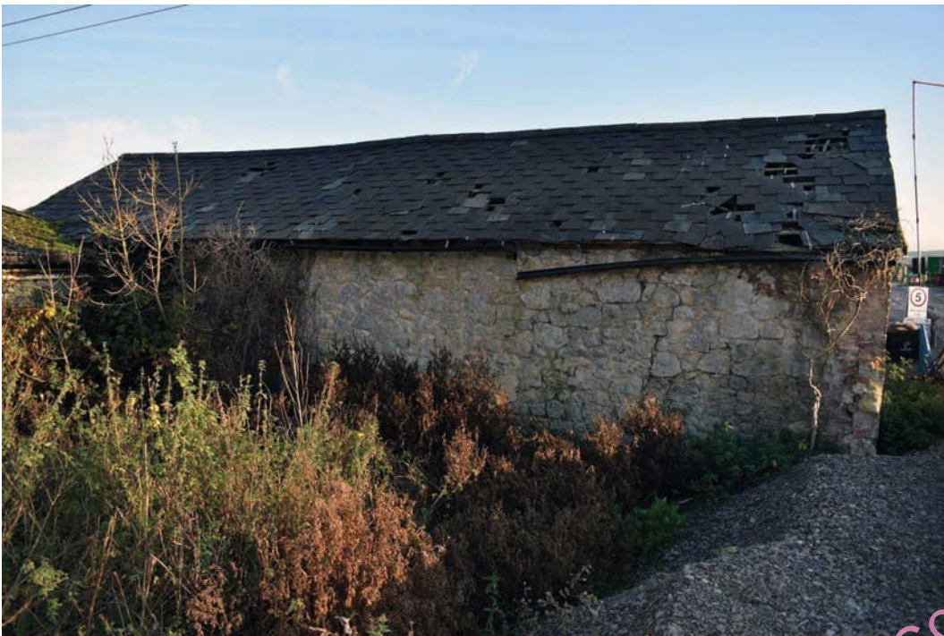
Photo B 110: North, rear elevation to the dairy-yard after removal of boundary wall
