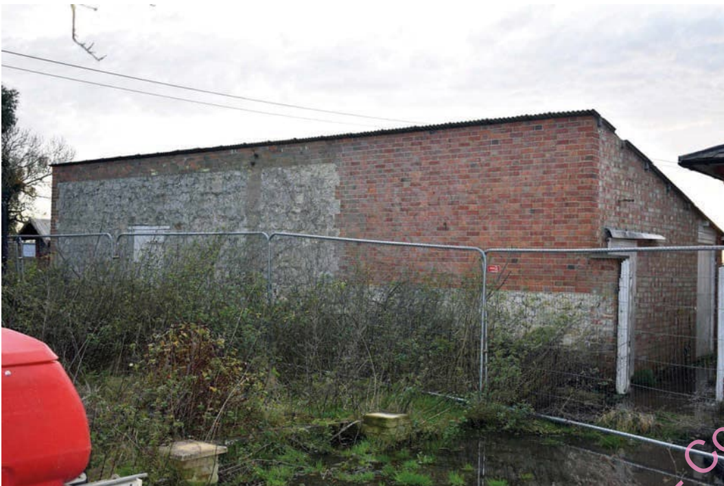
Photo B 94: East, rear wall showing brickwork distinct from that evident on the north wall
