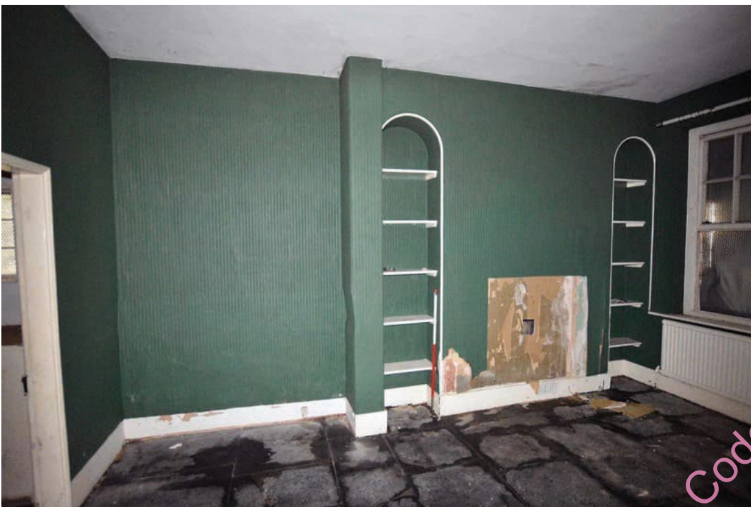
Photo B 33: Blocked fire place and arched alcoves within rear room G1
