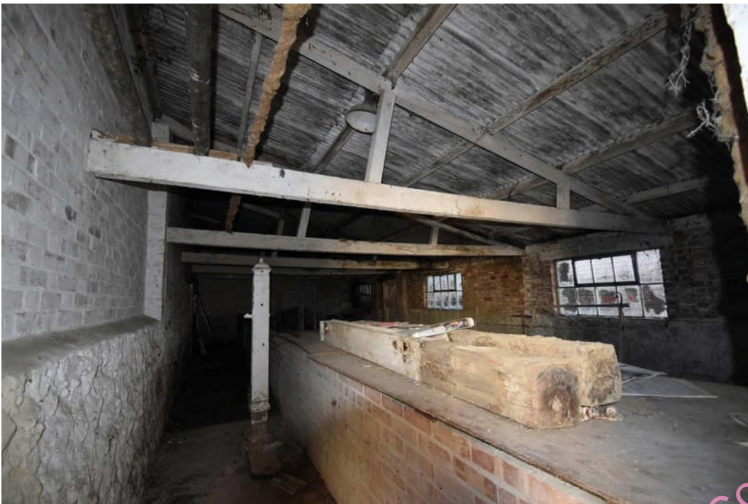
Photo B 96: General internal aspect looking south along the rear feeding passage
