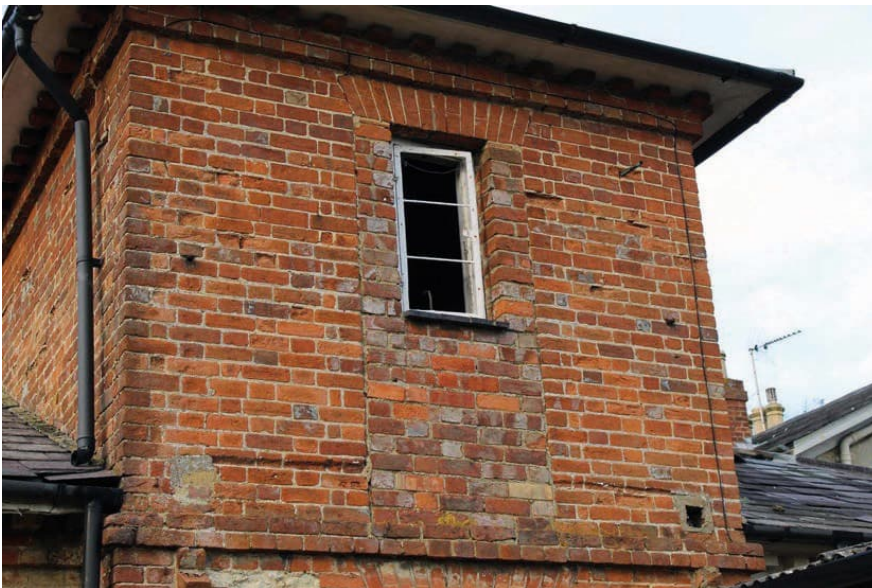
Photo B 72: Blocked loading door and window in upper storey
