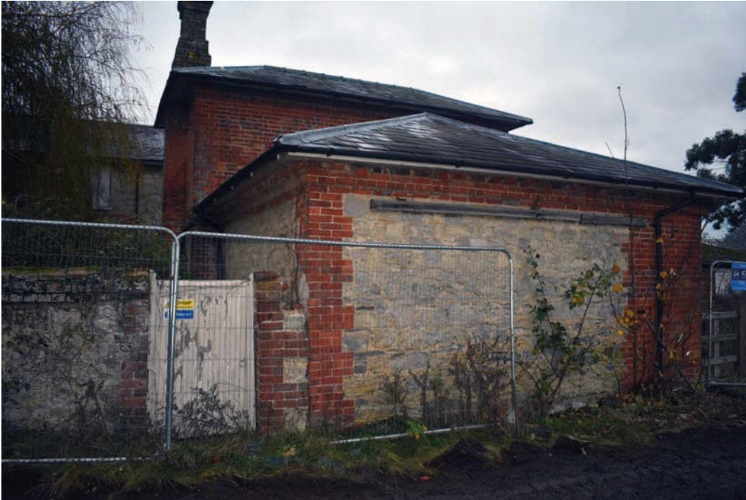
Photo B 69: West elevation showing possible truncation of front (west side) garden wall
