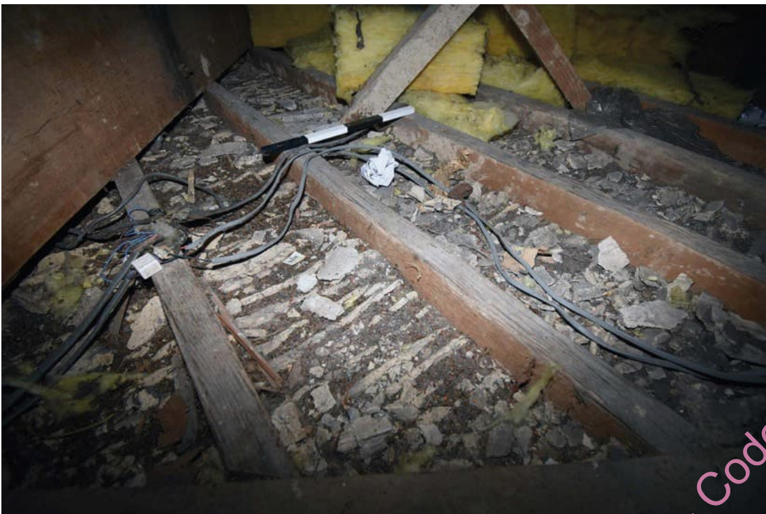
Photo B 64: Ceiling joists over first floor laid oblique to the building
