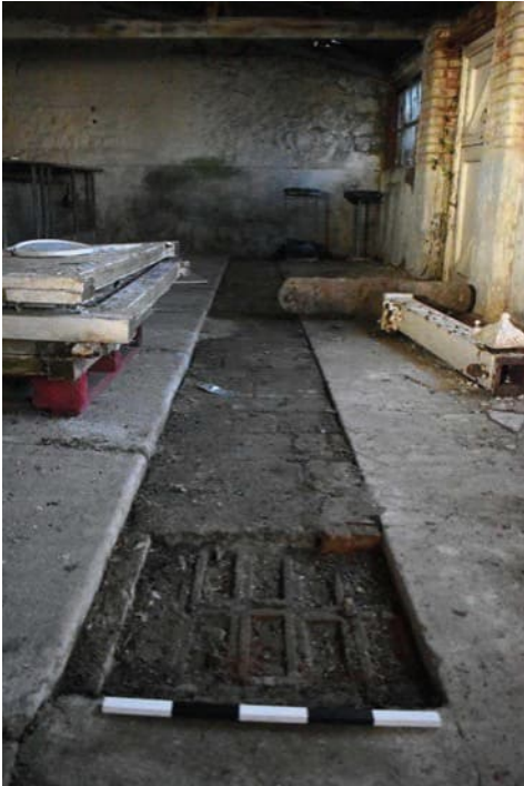
Photo B 105: Floor channel within western front parts of the building looking south
