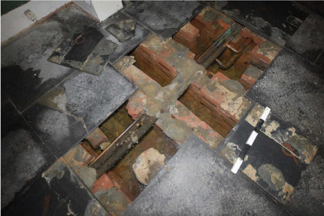
Photo B 36: Structural details of sub-floor support to slates in rear room G1
