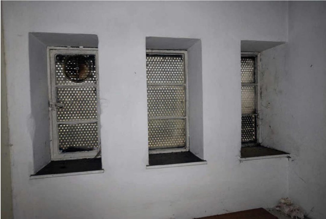
Photo B 40: Interior view of windows in east elevation to kitchen G5
