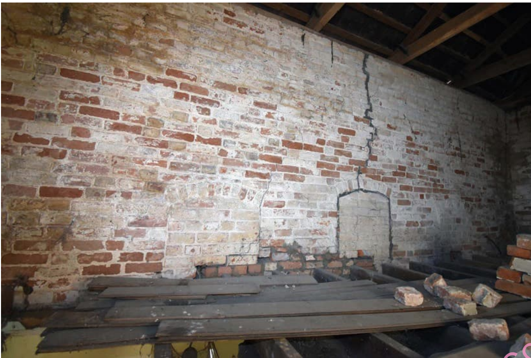
Photo B 86: Blocked openings in west wall within upper floor central space
