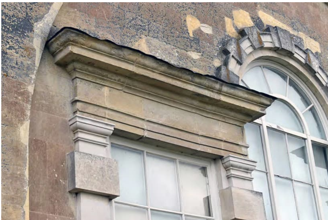
Photo B 19: Detail of the tripartite window in the west front of Claydon House
