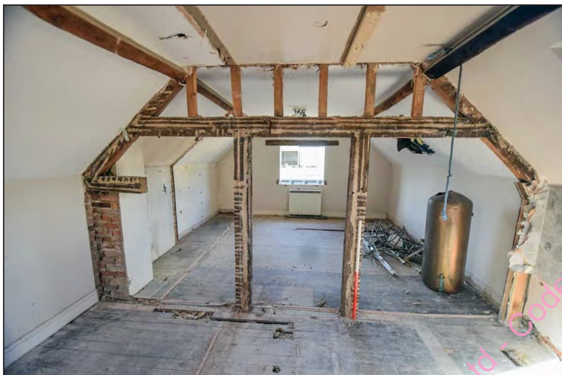
Photo A- 48: Structure dividing wall in rear extension
