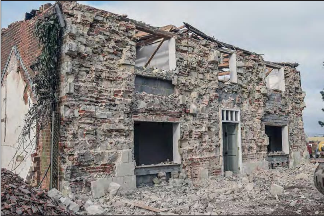
Photo B 1: The east front façade of the farmhouse after the ashlar facing has been stripped away
