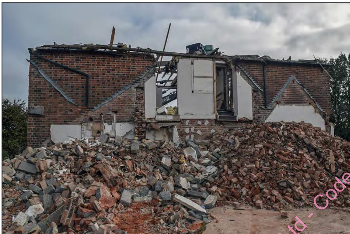
Photo A- 50: Rear, west elevation of farmhouse after removal of rear extensions
