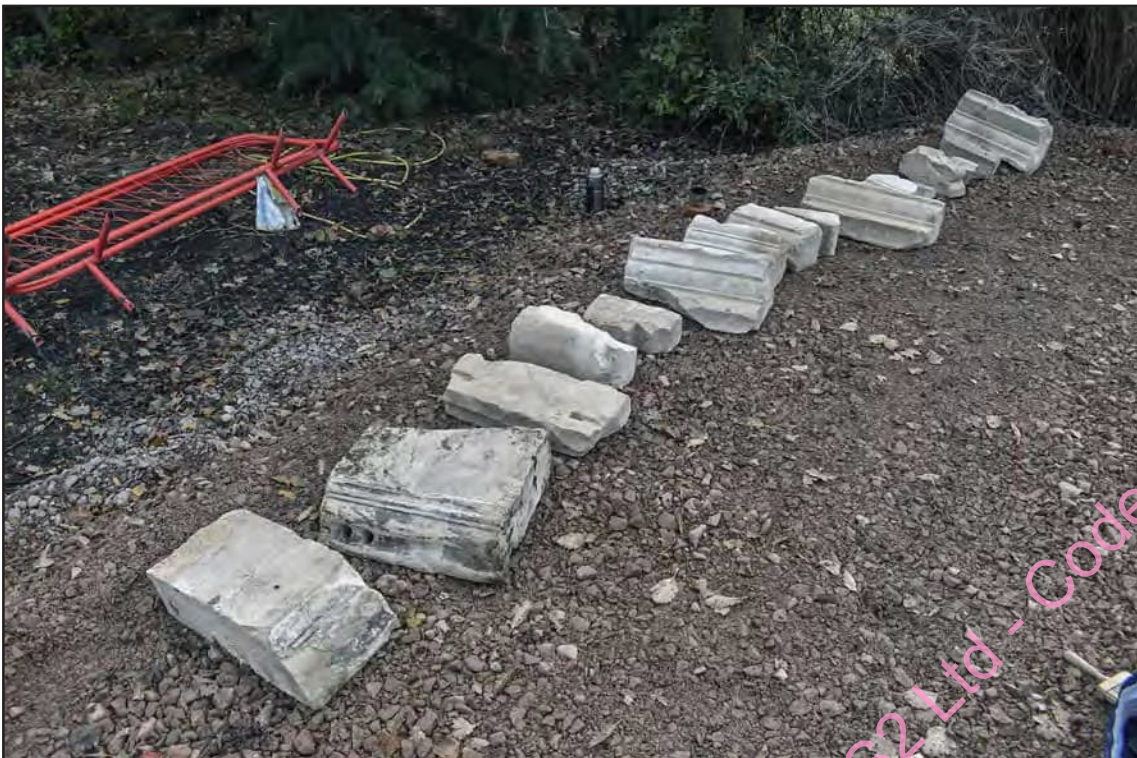
Photo B 2: Some of the masonry that was stripped from the east façade
