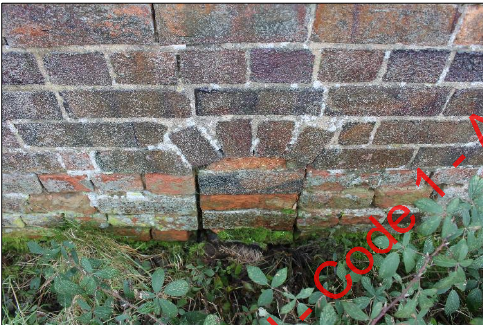
Plate 292: A blocked drainage chute in the western elevation of Building 11.
