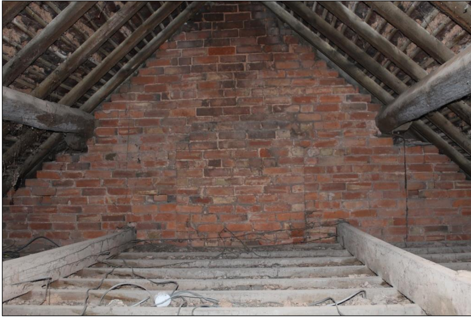
Plate 96: The roof construction above Rooms 26 and 27, viewed from the loft hatch within the northern wall of Room 33, Building 1.
