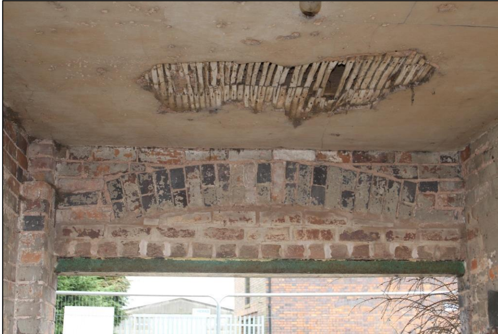
Plate 154: Detail of segmental brick lintel and exposed lath and plaster ceiling at the eastern extent of Room 5, Building 3.
