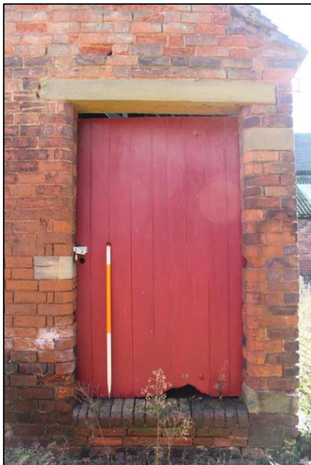
Plate 137: Detail of door opening with chamfered surrounds within the western gable of Building 4.
