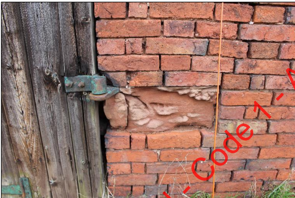
Plate 211: The sandstone blocks holding the pintels of the large threshing door in the southern elevation of Building 7.
