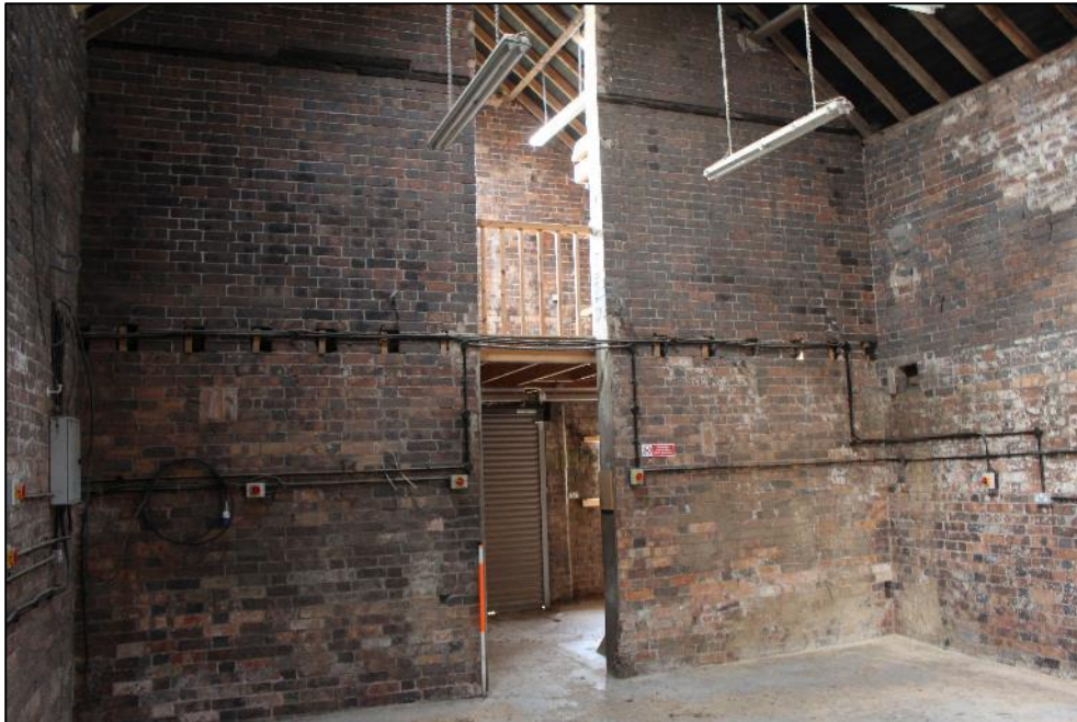
Plate 200: The dividing wall in the centre of Building 6, viewed from the northern half of the building.
