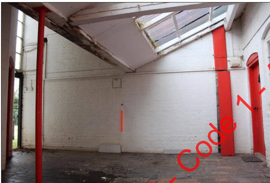
Plate 59: The external, western wall of Room 7, Building 1, viewed from within the covered courtyard.
