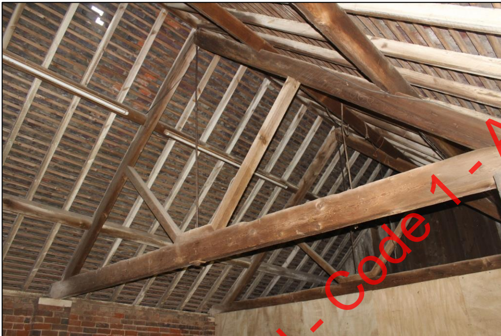
Plate 181: Overview of the King-bolt roof construction within Room 3, Building 5, viewed from the south-west.
