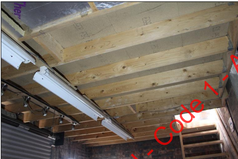
Plate 203: The floor of the inserted mezzanine in the southern half of Building 6.
