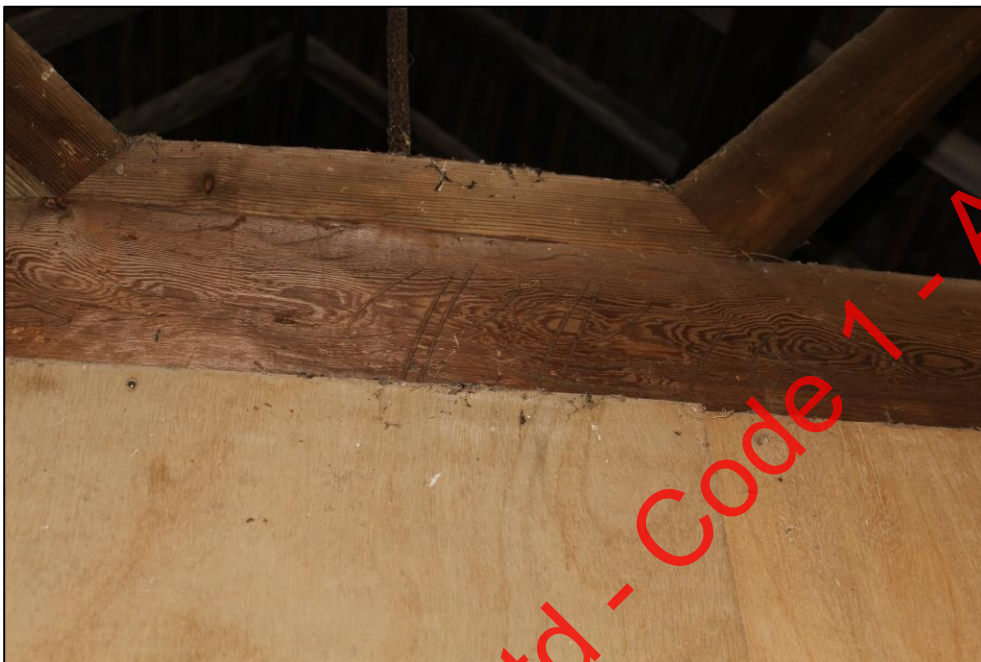
Plate 183: Detail of carvings and Baltic timber marks on the tie beam of the eastern truss between Room 3 and Room 2, Building 5.
