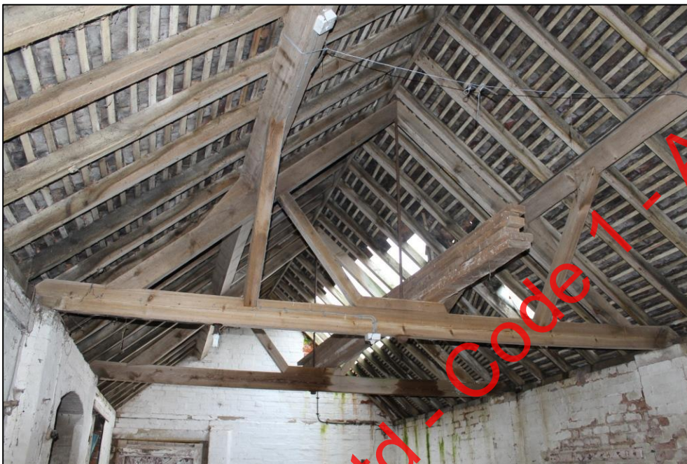
Plate 165: Detail of King-bolt roof construction within Room 8, Building 4, viewed from the east.
