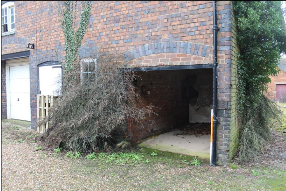
Plate 128: The northern extent of the eastern elevation of Building 3, viewed from the north-east.
