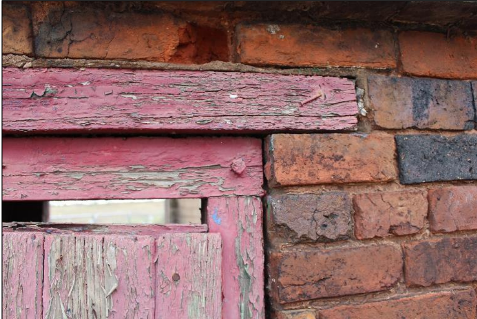
Plate 258: Detail of the pegged timber door frame on the southern elevation of Building 10a.
