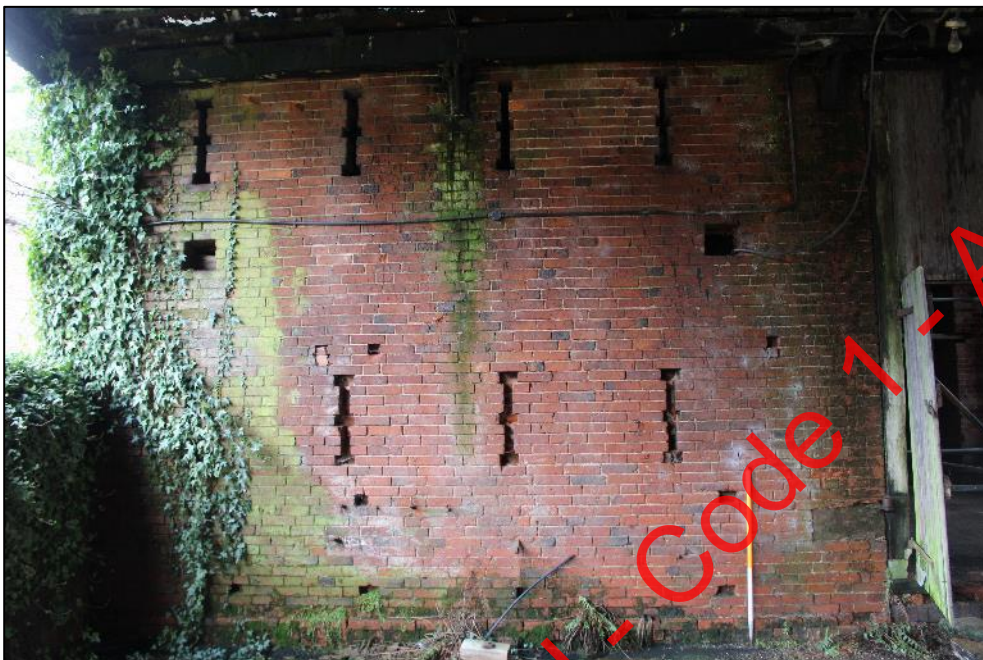
Plate 213: The eastern side of the northern elevation of Building 7, showing the ventilation holes and slits.
