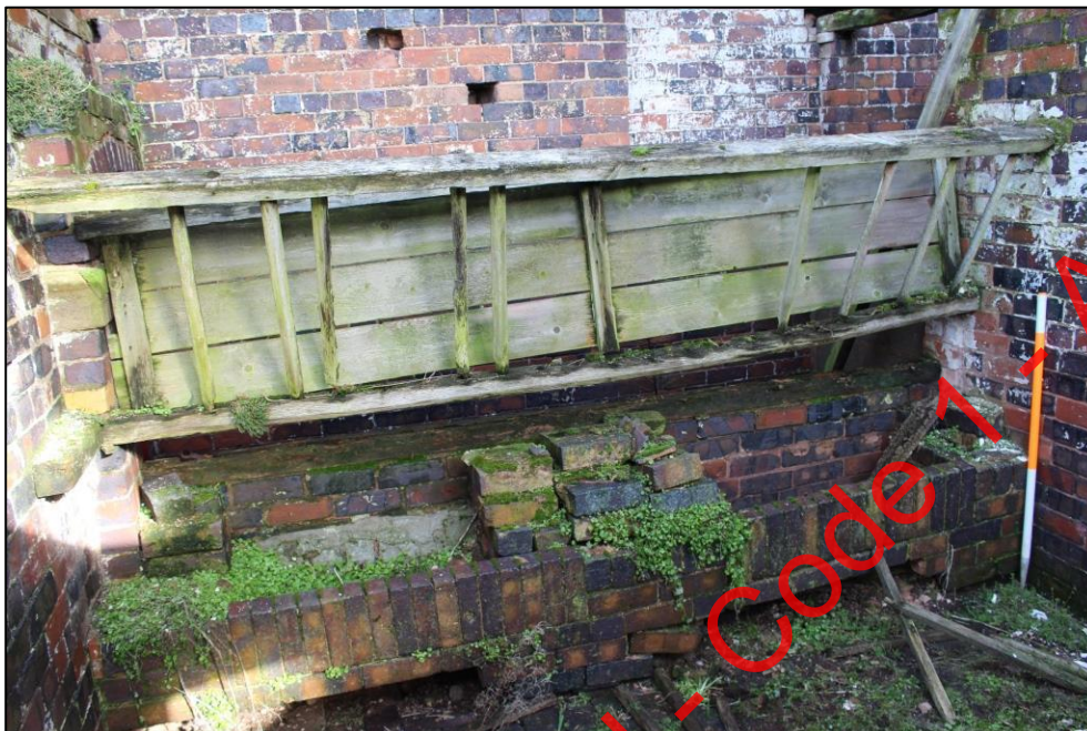
Plate 119: The northern wall of Room 14, Building 2 and the brick and timber built feeding trough.
