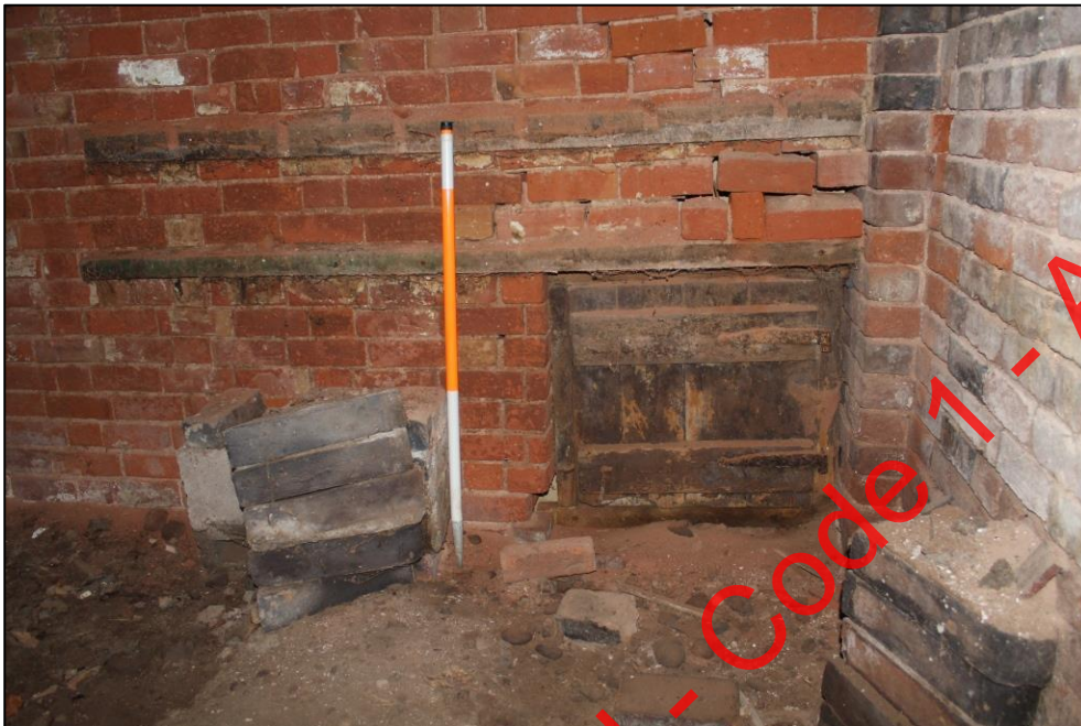
Plate 177: Timber door and hatch at ground level within the north-western corner of Room 1, Building 5.
