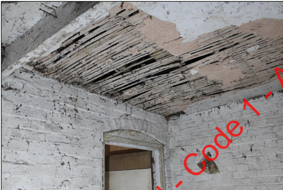
Plate 151: Exposed lath and plaster ceiling within the south-eastern corner of Room 4, Building 3.
