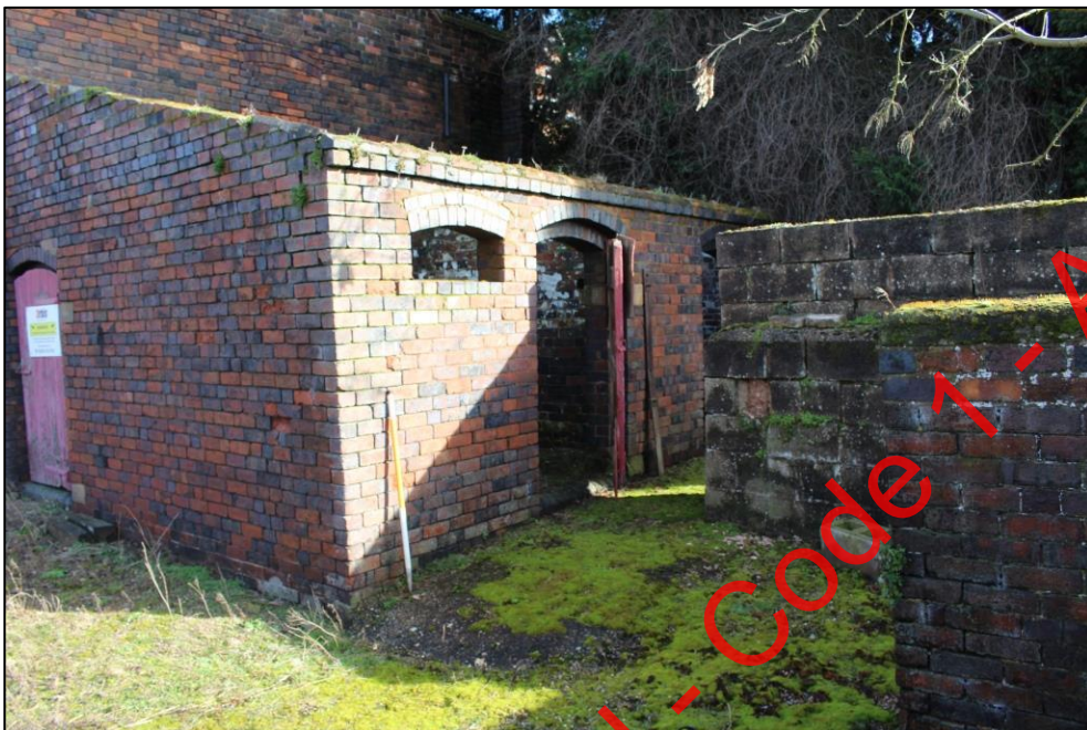
Plate 115: Lean to stables against the southern gable of Building 2, viewed from the south-west.
