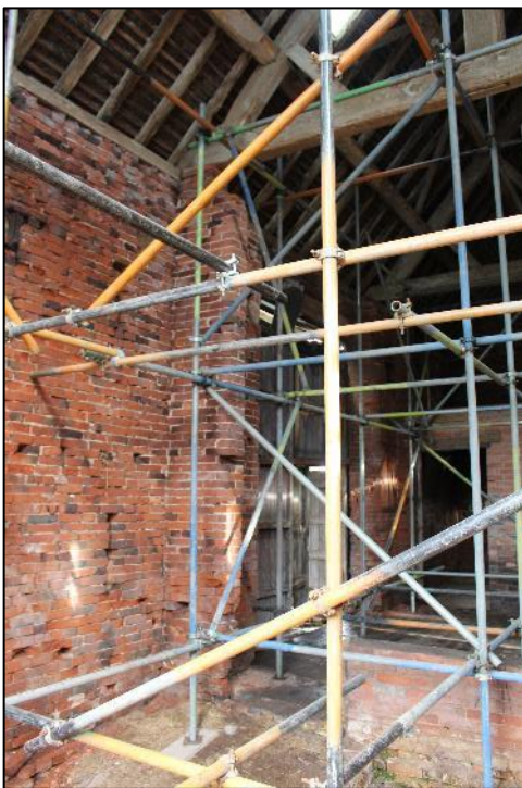
Plate 217: The northern wall within Building 7, taken from the western side of the barn.
