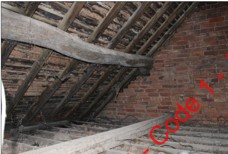
Plate 97: The roof construction above Rooms 26 and 27, viewed from the loft hatch within the northern wall of Room 33.
