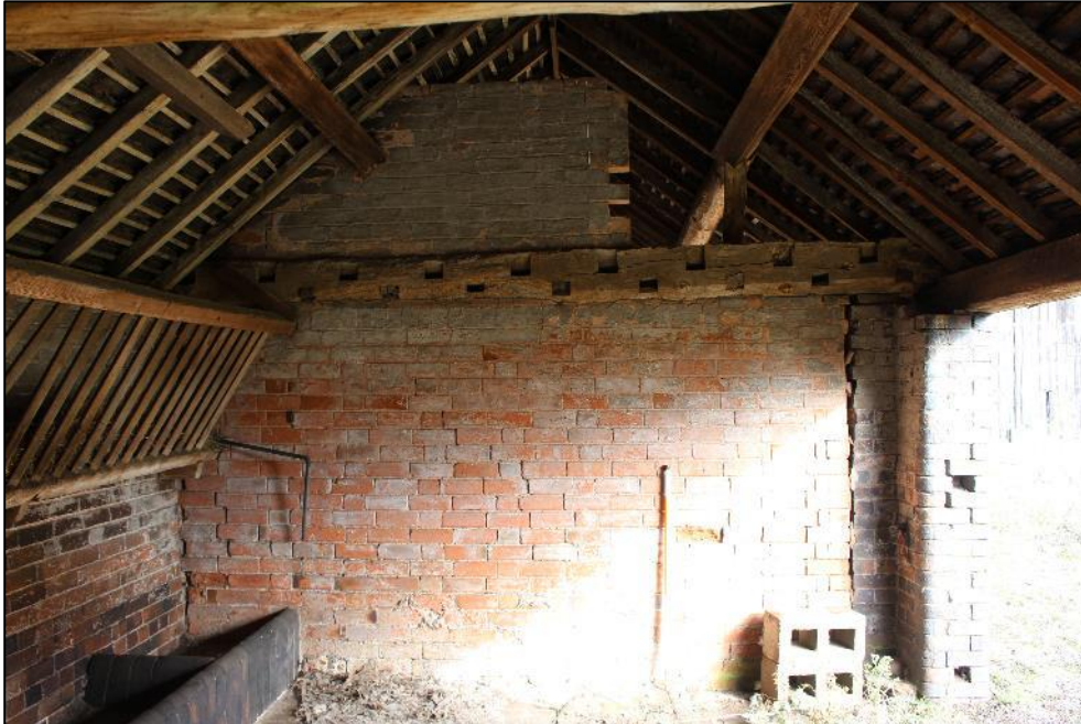
Plate 301: The dividing wall between the northern and southern rooms of Building 11, taken from within the southern room.
