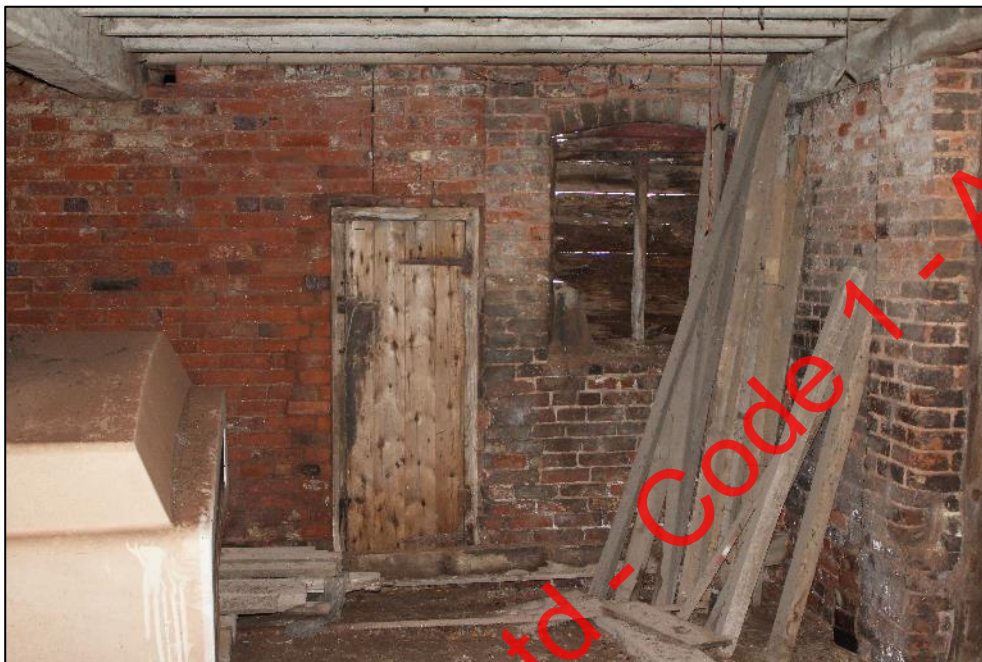
Plate 276: The northern end of the western wall of Building 10b. The break in brick coursing is visible to the right of the doorway.
