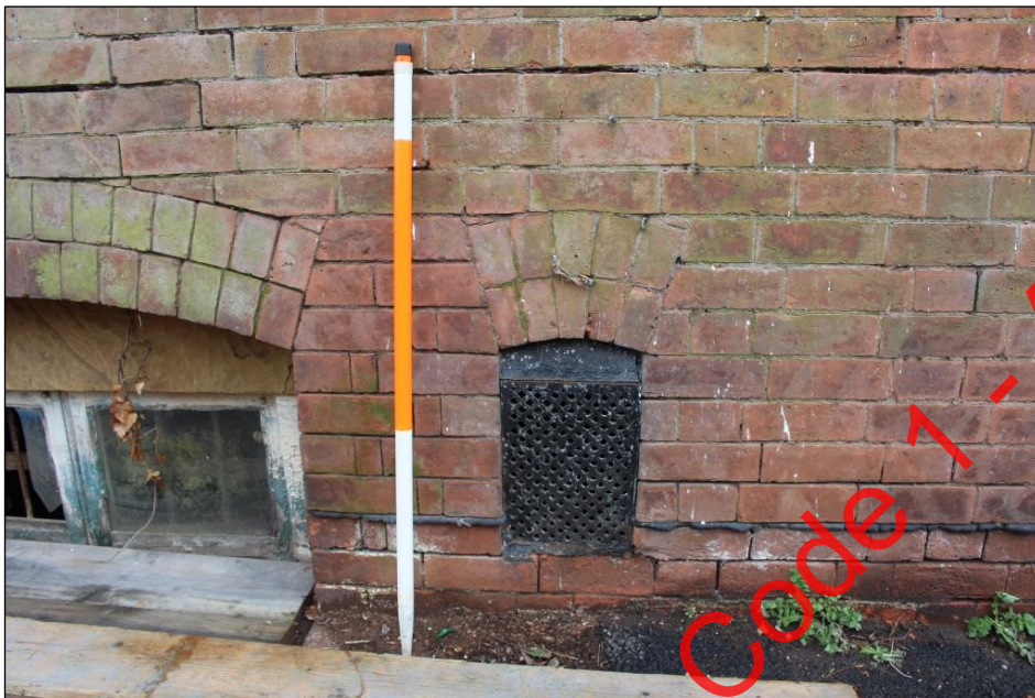
Plate 33: Vent to cellar situated beneath a segmental brick arch within the eastern elevation.
