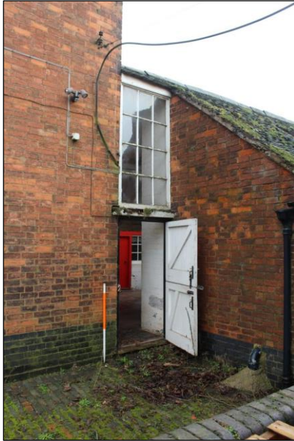
Plate 36: The joint between the northern elevation of Building 1 and the single storey wash house.
