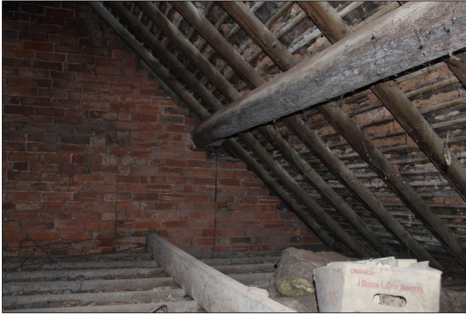
Plate 98: The roof construction above Rooms 26 and 27, viewed from the loft hatch within the northern wall of Room 33.
