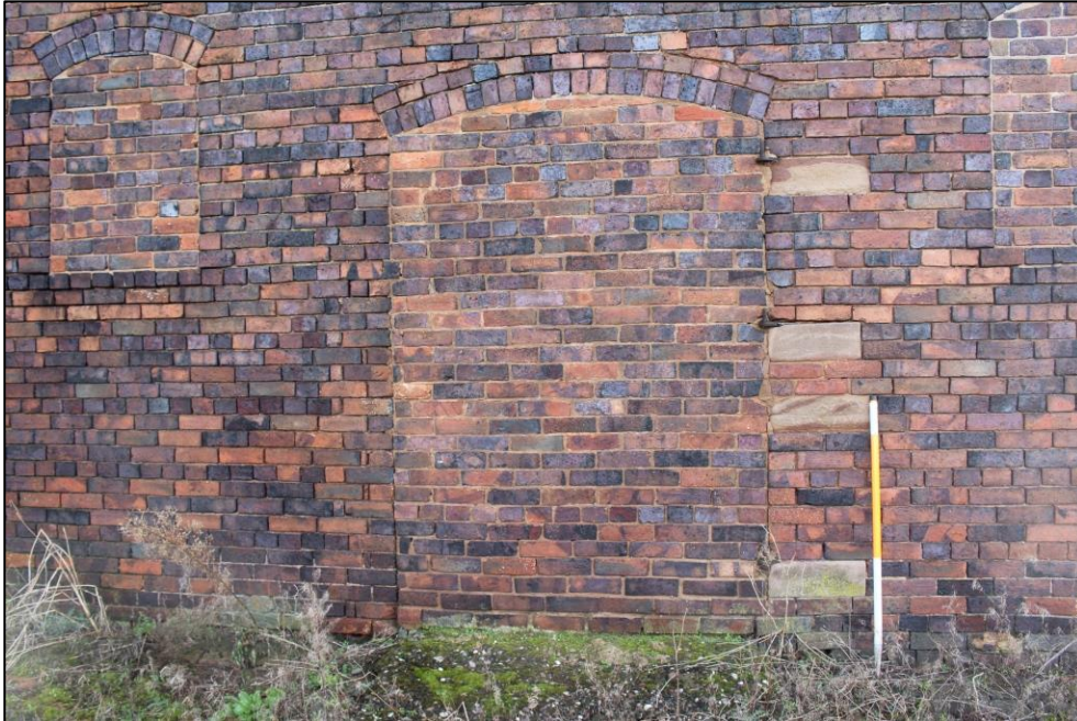
Plate 110: Detail of blocked window and door openings situated beneath segmental brick arches within the western elevation of Building 2.
