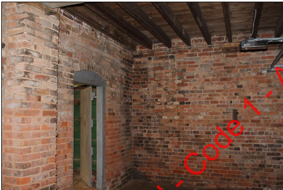
Plate 143: The western and northern walls of Room 1, Building 3, viewed from the south-east.
