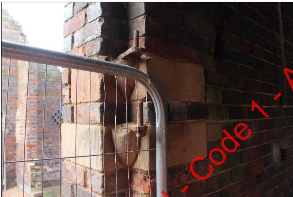
Plate 235: The large sandstone blocks and pincels attached to the large doorway in the eastern elevation of Building 8.
