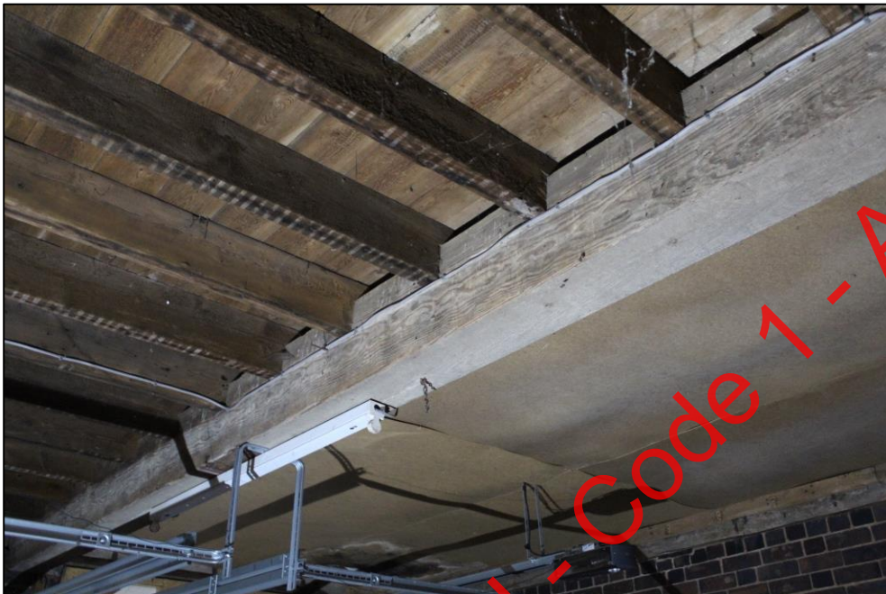
Plate 145: Detail of exposed ceiling construction in Room 1, Building 3, viewed from the north-west.
