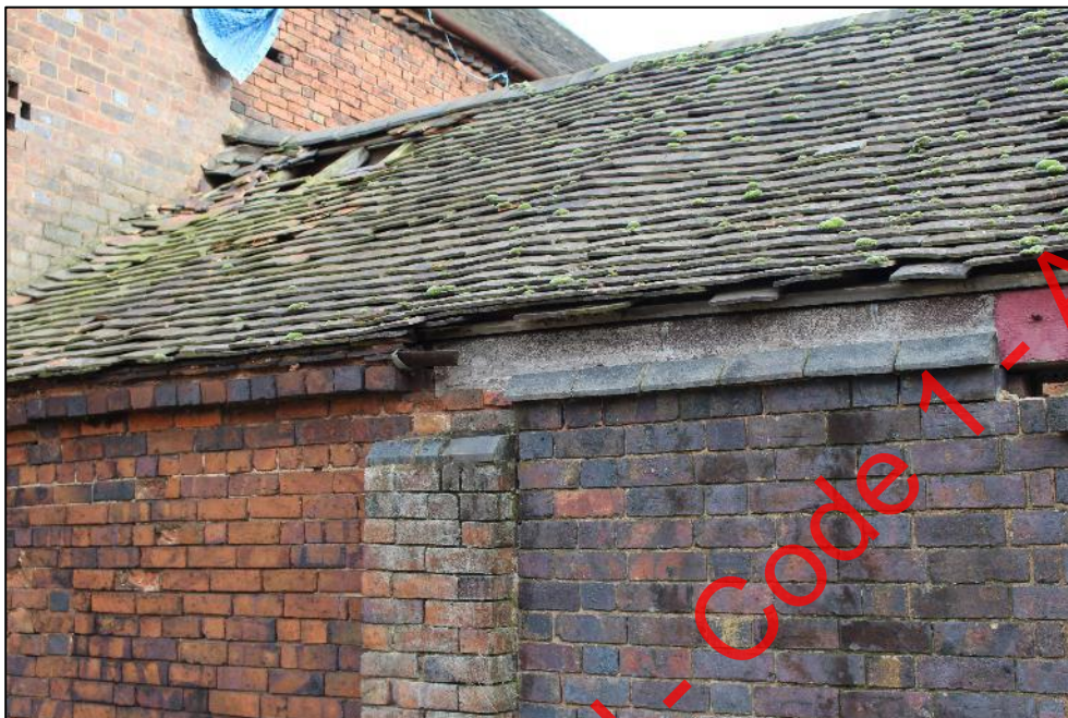
Plate 294: The change at eaves level on the northern side of the western elevation of Building 11, indicative of the blocking of an opening.
