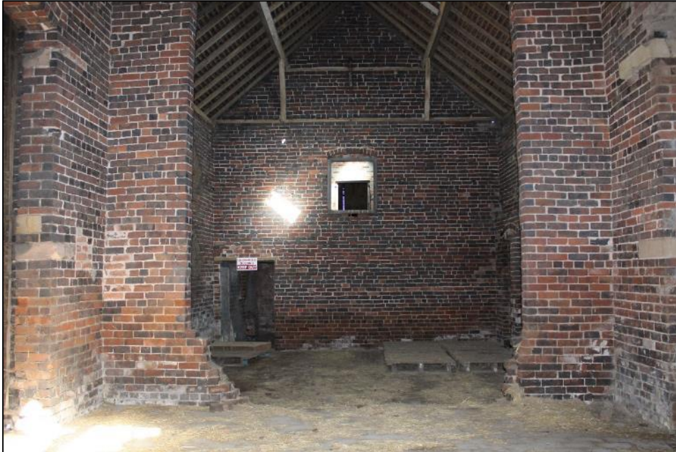
Plate 236: The interior of Building 8 prior to demolition, facing north towards Building 10. Photograph taken by DJV.
