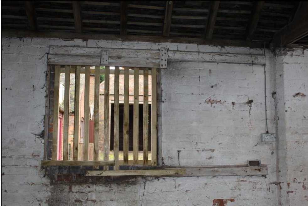
Plate 164: Detail of the remains of a sliding shutter to the southern wall of Room 8, Building 4.
