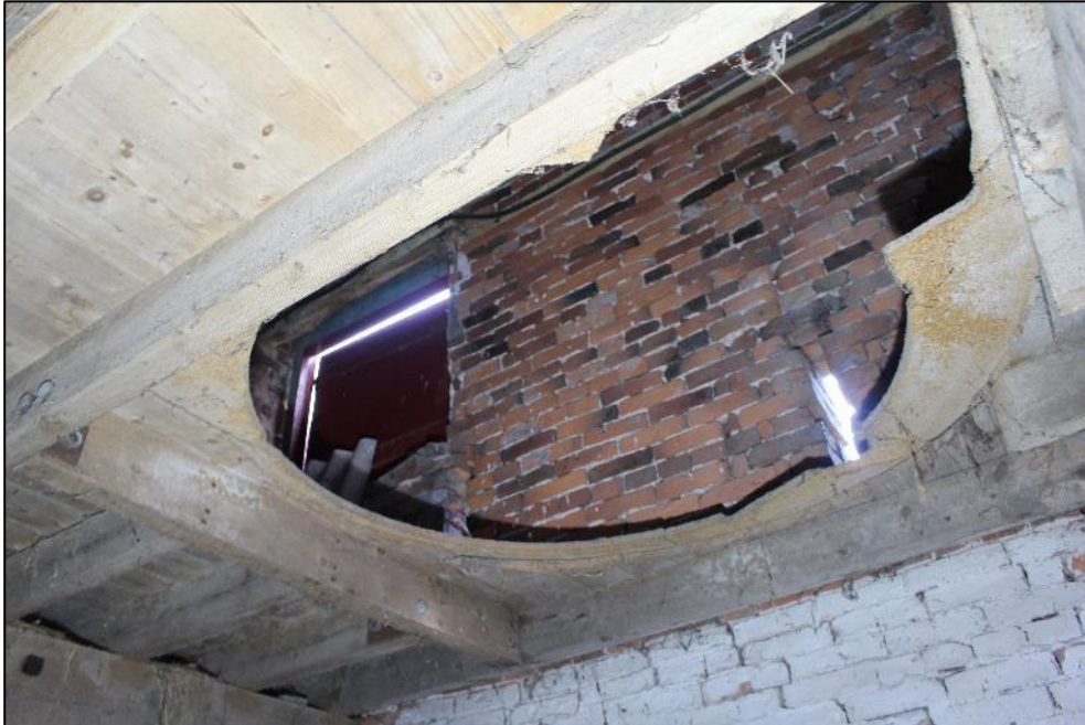
Plate 224: The hole cut in the ceiling of the eastern room of Building 7, providing access to the mezzanine above.
