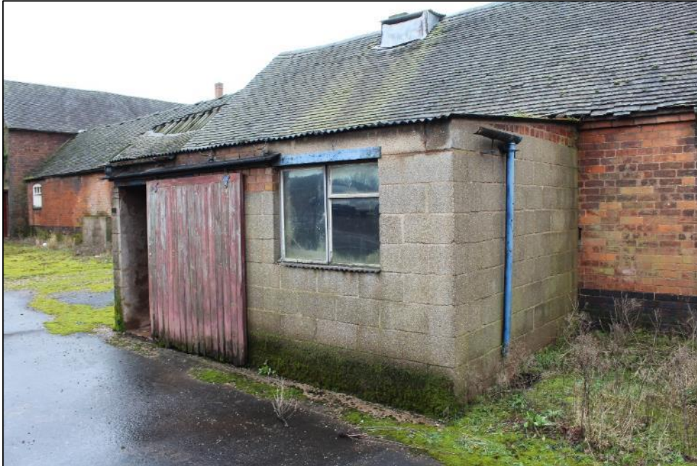
Plate 246: The breezeblock lean-to at the eastern end of the northern elevation of Building 9.
