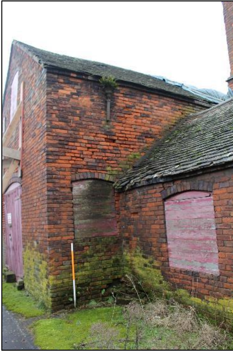
Plate 262: The northern end of the western elevation of Building 10b, and its relationship to Building 10a.
