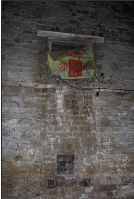
Plate 178: Blocked window/ventilation opening within the eastern wall of Room 1, Building 5.
