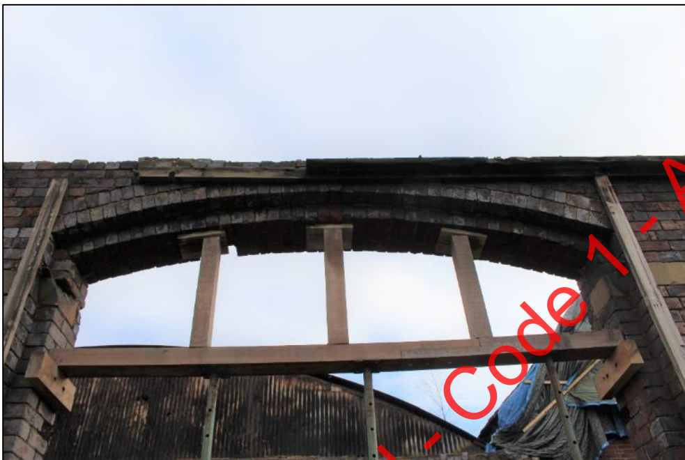
Plate 229: The arch above the central doorway in the western elevation of Building 8.
