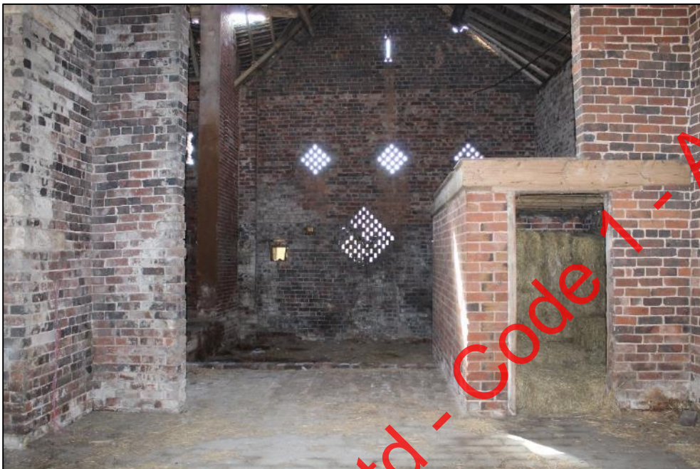
Plate 237: The interior of Building 8 prior to demolition, facing south. Photograph taken by DJV.
