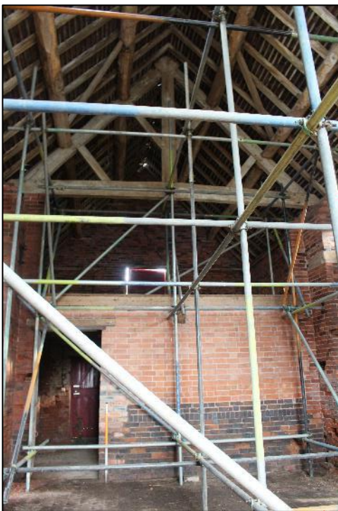
Plate 215: View looking east within Building 7, showing the brick dividing wall, the mezzanine, and roof structure.
