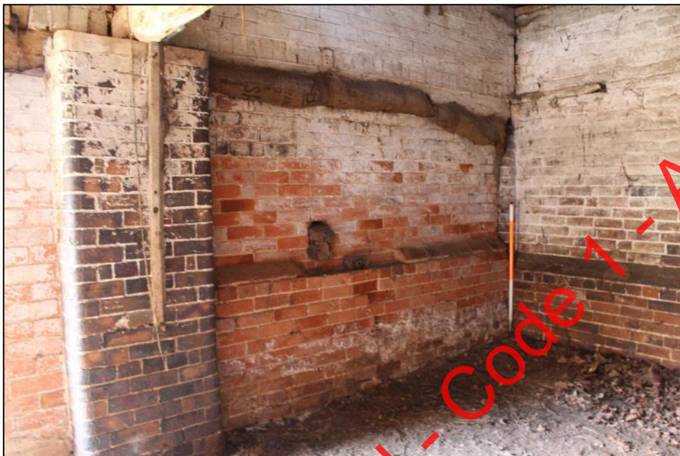
Plate 298: The eastern wall in the southern room of Building 11, this is the division between this space and the western stable room.
