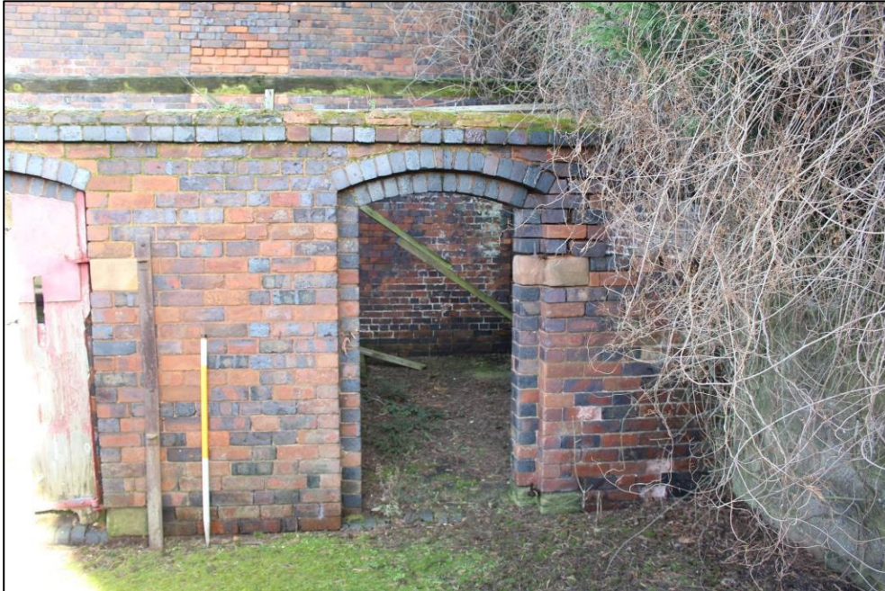
Plate 116: Detail of stable door opening within the southern elevation of the lean-to stable against Building 2.
