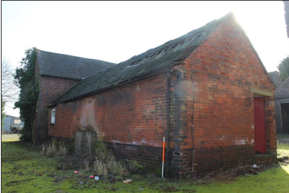
Plate 134: Overview of the northern and western elevations of Building 4 from the north-west.
