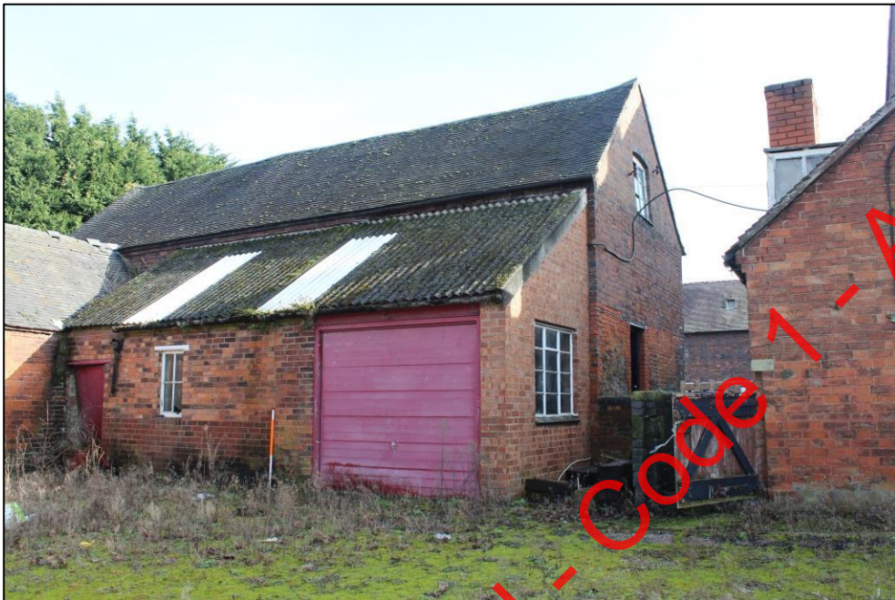
Plate 141: The lean-to against the western elevation of Building 3, viewed from the south-west.
