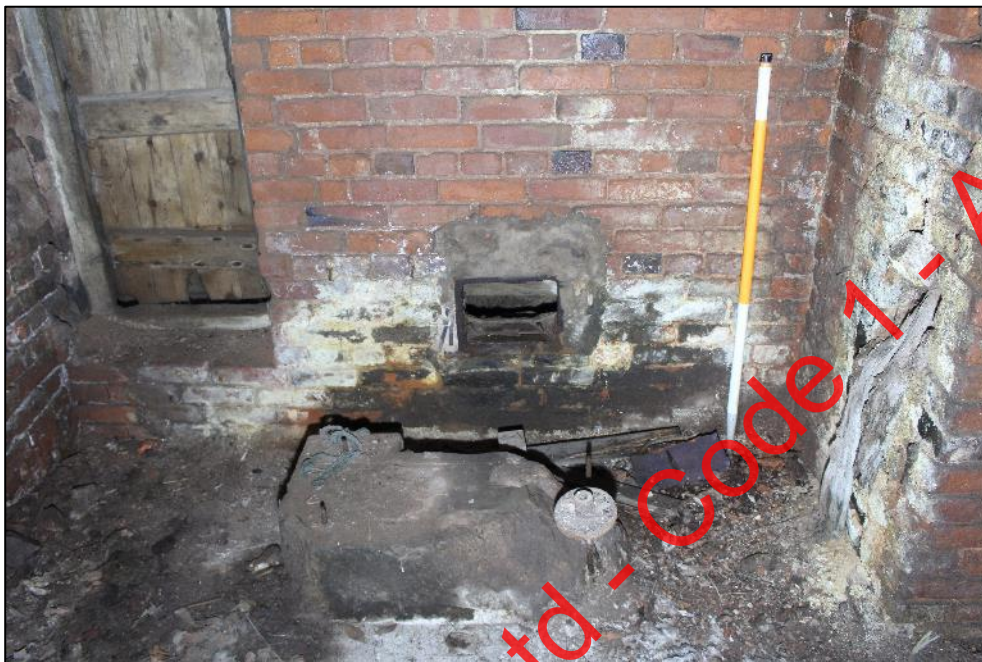
Plate 270: The low vent in the eastern wall of the eastern room of Building 10a.
