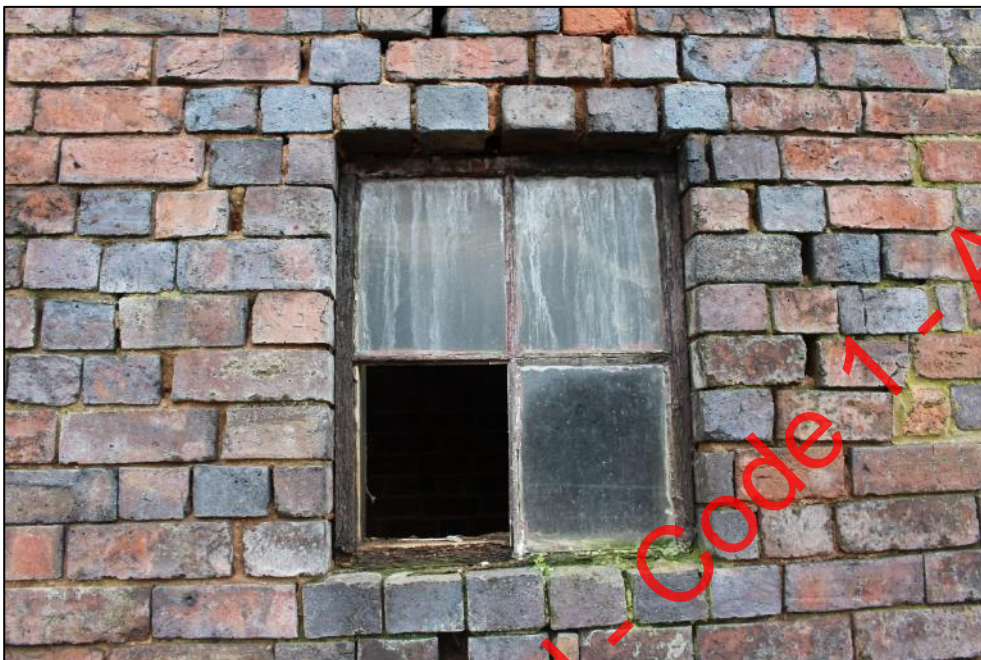
Plate 231: The small timber window in the southern section of the western elevation of Building 8.
