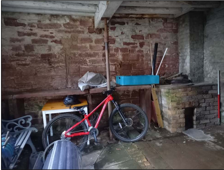
Plate 87: West wall of Wash House showing sandstone shelving and brick wash copper (Scale = 1m)
