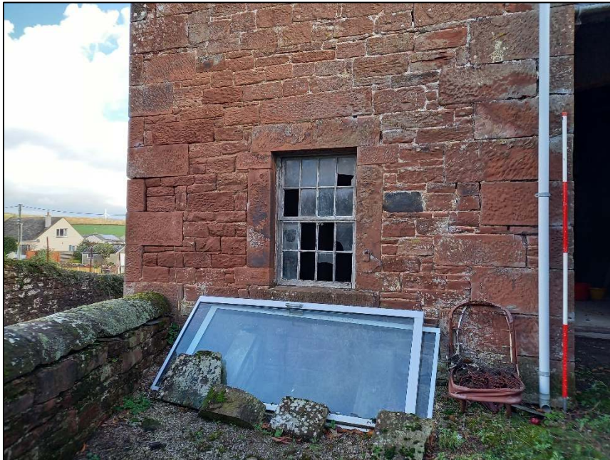
Plate 30: West elevation of northern projection showing window with sloping feeding or loading hatch below
