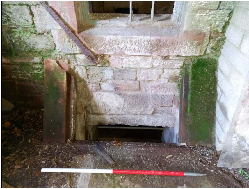
Plate 37: Detail of feeding or loading hatch at the base of the window in the west elevation of the southern projection (Scale = 1m)
