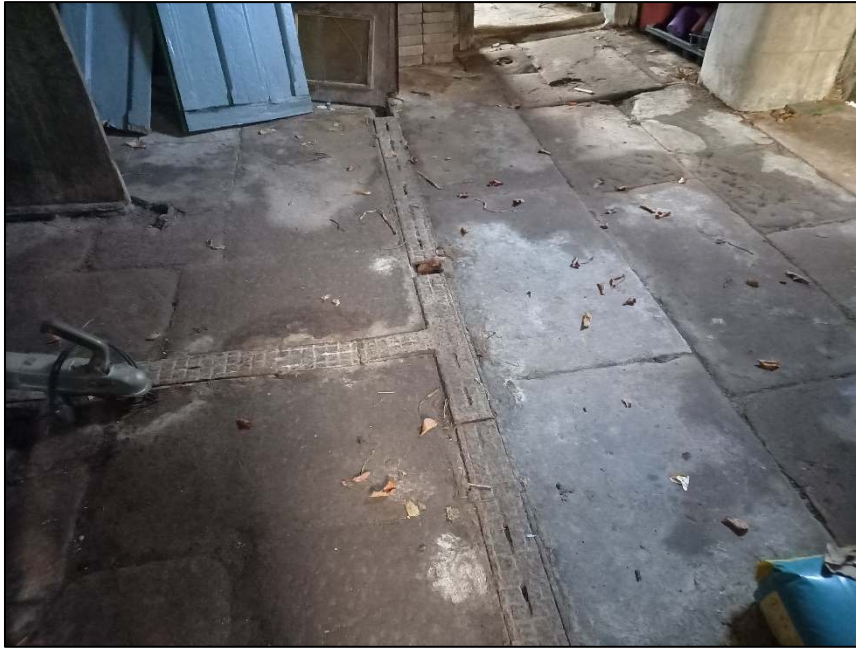
Plate 45: Detail of drainage in floor of stables, ground floor of barn (Room A)
