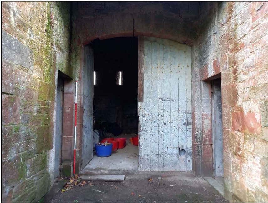
Plate 26: Detail of large doorway in west elevation of the barn (Scale = 2m)
