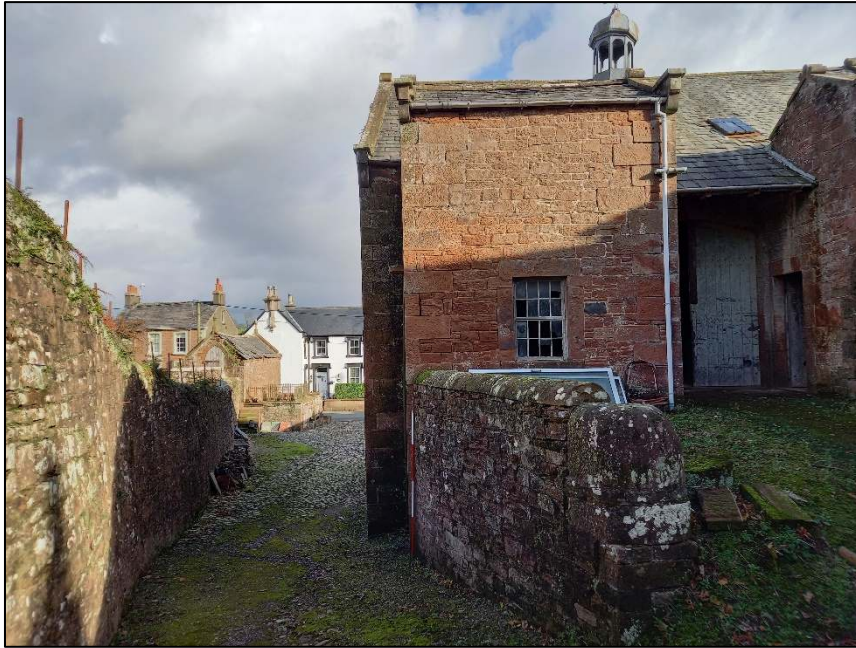
Plate 23: View looking east showing the north end of the west elevation, with the access track which runs along the buildings north side
