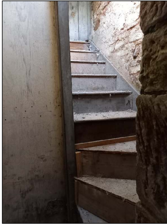
Plate 65: Wooden stairs to pigeon loft, accessed from the upper floor of the southern projection
