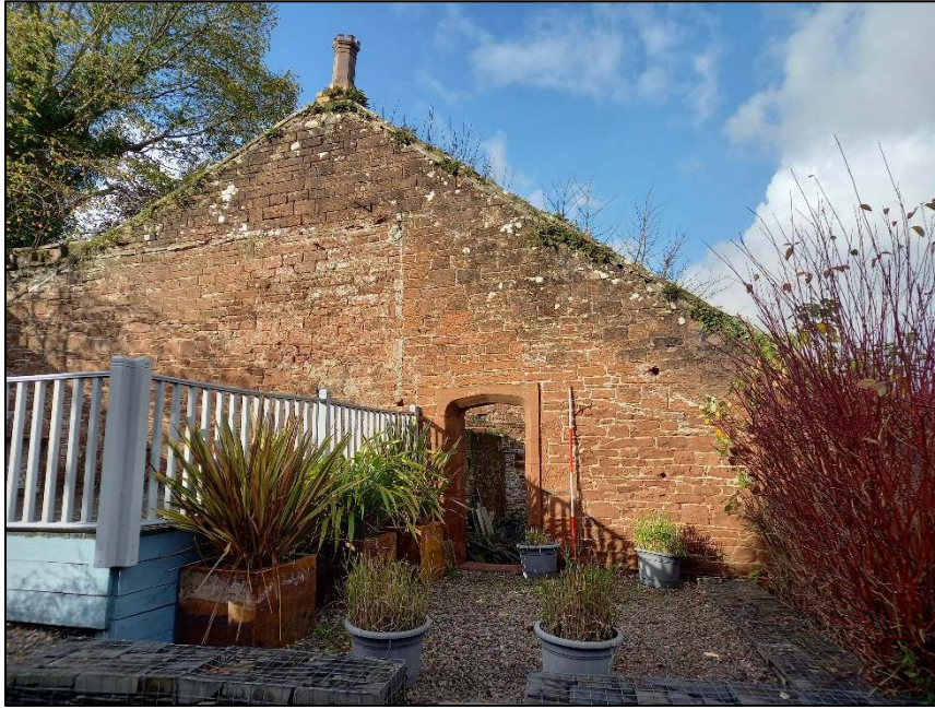
Plate 93: South elevation of part of the ancillary buildings showing the scarring of a former glass house
