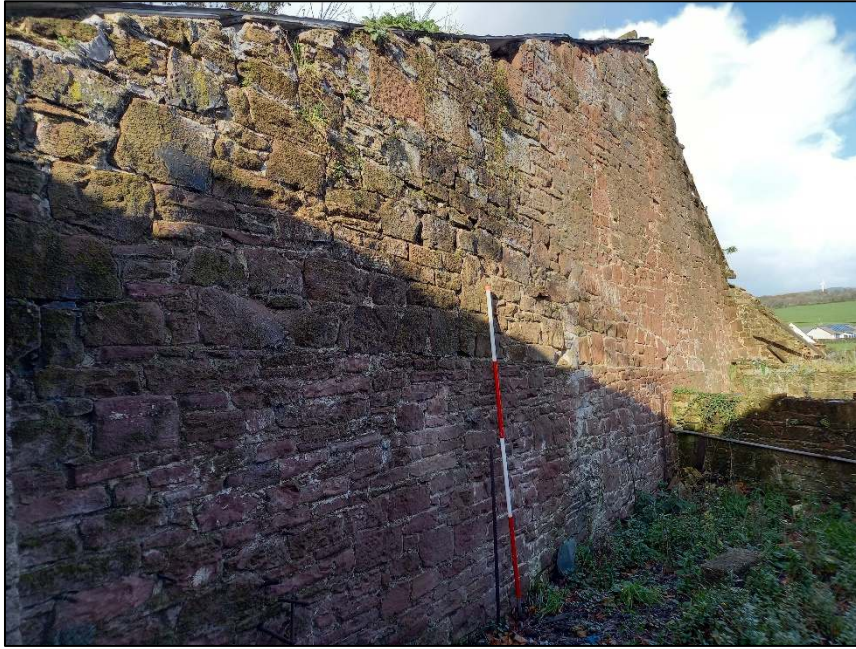
Plate 95: North wall of ancillary buildings, west end, showing evidence for former boundary wall prior to being increased and gabled
