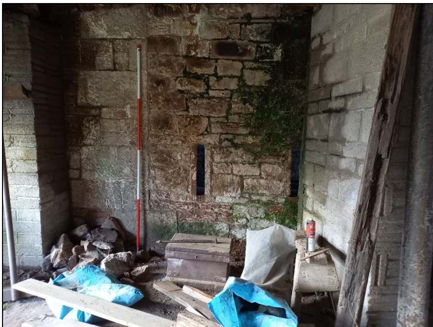
Plate 38: View looking east showing the construction break between the west wall of the southern projection and the ancillary structures (Scale = 2m)
