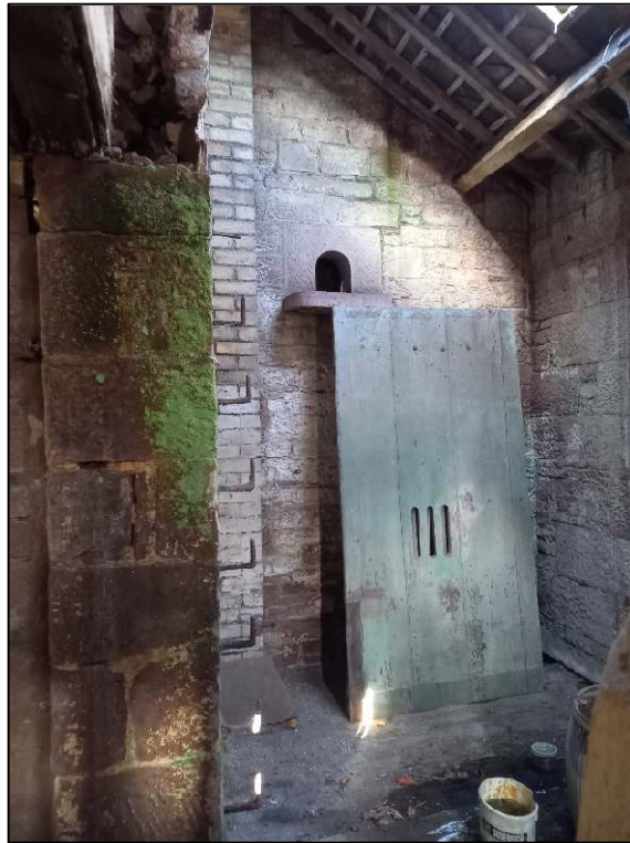
Plate 39: South elevation of the southern projection, now partly obscured by the later ancillary buildings, showing bird ledge and brick flue for a wash copper located in the wash house
