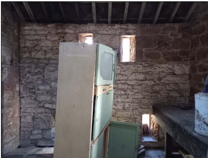
Plate 88: East wall of the addition (south side of Room G) showing ventilation slits
