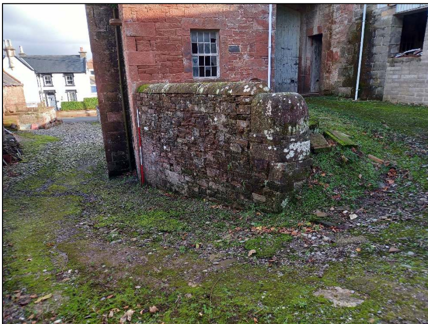
Plate 24: Detail of stone revetment wall which defines the north side of the ramp into the main entrance of the bank barn
