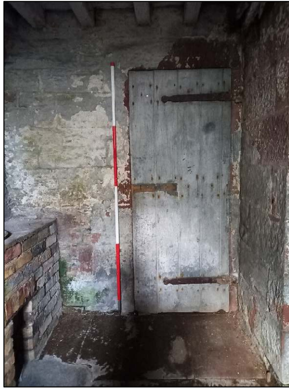
Plate 85: Doorway in north wall of Wash House, provides access to Room G (Scale = 2m)
