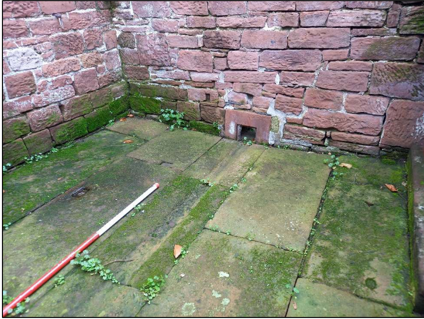
Plate 103: Detail of flagged floor of one of the pig sties in the Hennery-Piggery
