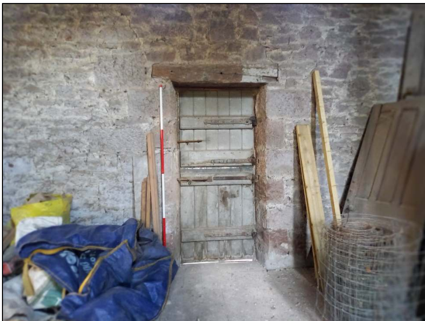
Plate 74: Detail of door in east elevation, first floor of barn (Scale = 2m)
