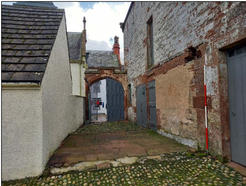
Plate 10: View looking south showing the location of a former building against the east elevation of the barn. The archway provides access to the rear of the house
