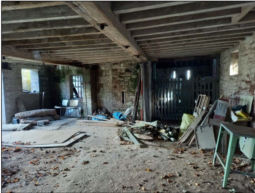
Plate 80: View looking east showing the ancillary building closest to the barn, showing the long beams
