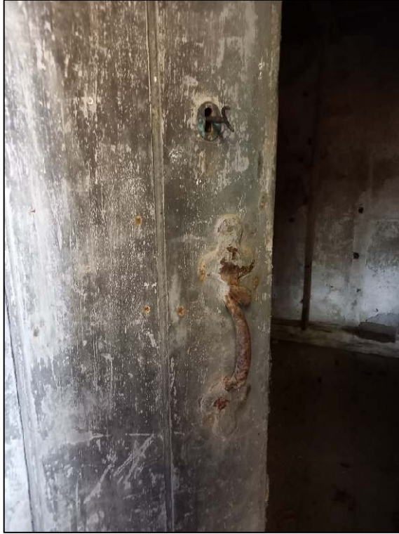
Plate 61: Detail of handle and lock, with remains of key, door into Room G, southern projection
