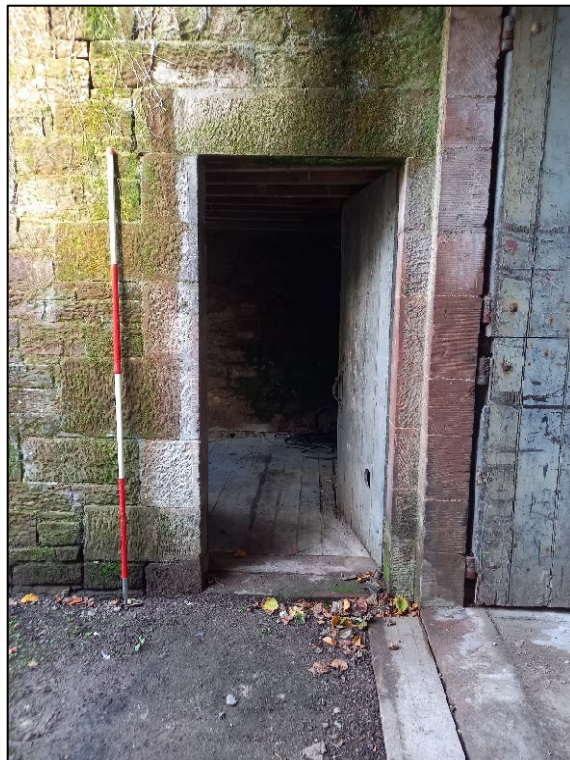
Plate 32: South elevation of the northern projection, detail of doorway to first floor room (Scale = 2m)
