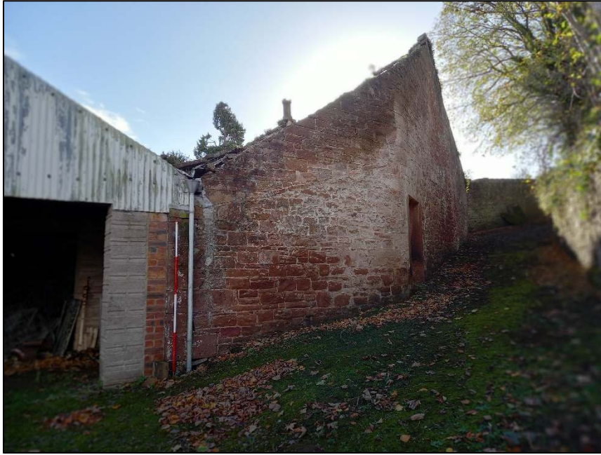
Plate 89: View looking west showing the roofless ancillary building, with evidence for three phases of construction visible in the stonework
