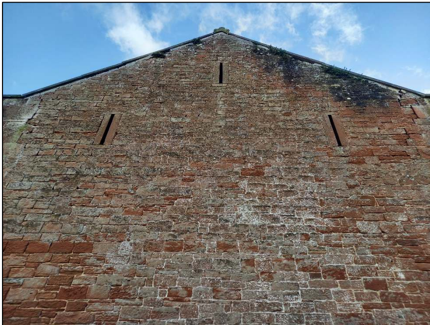
Plate 18: Detail of the three ventilation slits in the north elevation of the barn
