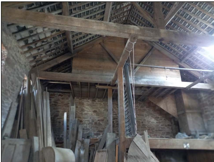
Plate 72: View looking south showing the first floor of the barn. The pigeon loft is located between the furthest roof truss and the south gable wall
