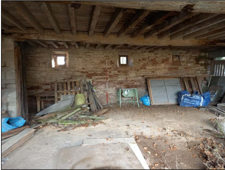
Plate 81: View looking south showing the interior of the ancillary building, possible horse engine house
