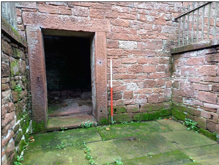
Plate 104: Detail of low doorway into one of the sties, Hennery-Piggery (Scale = 1m)
