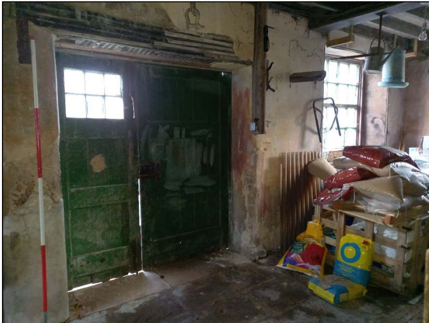
Plate 46: East wall of the stables showing plastered walls and projecting wooden support for horse tack/saddles (Room A)
