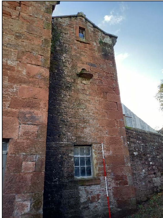
Plate 28: North elevation of the northern projection, or “turret”, against the west elevation of the barn
