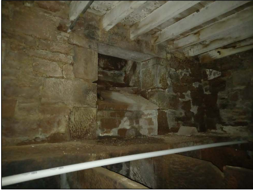
Plate 55: Hatch in the west wall of Room E, ground floor of southern projection
