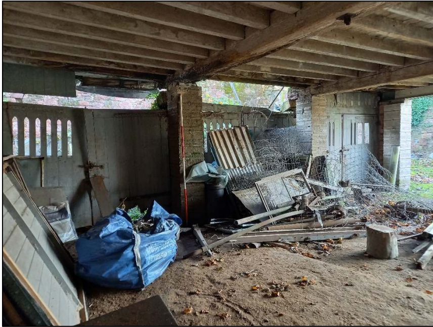
Plate 83: West wall of the ancillary building showing the three double doorways (Scale = 2m)
