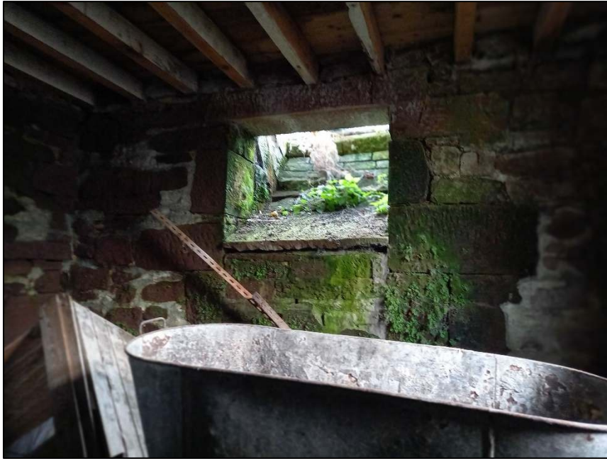
Plate 53: View looking west showing the hatch in the west wall of Room D, ground floor of the northern projection
