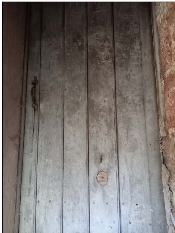
Plate 66: Detail of door to pigeon loft, as seen from the wooden stairs from the southern projection
