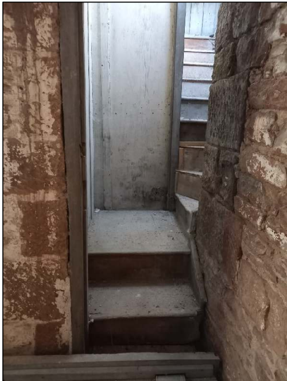
Plate 64: Upper floor of southern projection showings wooden stairs to the pigeon loft
