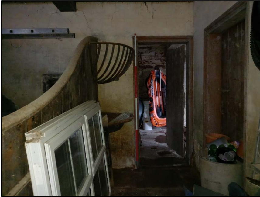
Plate 47: View looking west showing the doorway in the west wall of the stables, ground floor of barn (Room A)
