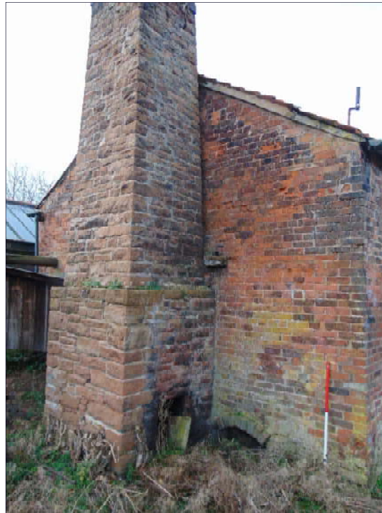
Plate 33: Detail of southeast elevation of Building D, showing arched opening at base of wall, looking west
