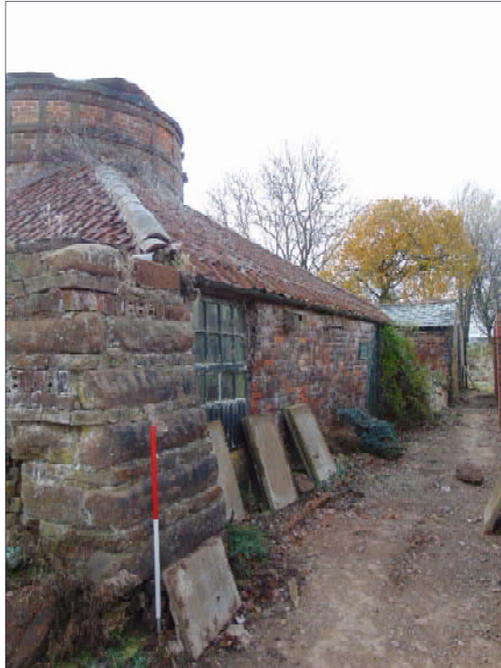
Plate 13: Northwest elevation of Building B, showing remnant stone wall of former kiln, looking southwest [2]
