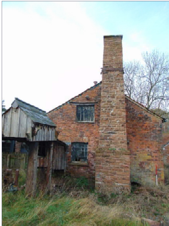
Plate 32: Southeast elevation of Building D, showing chimney stack for boiler house, looking northwest [14]
