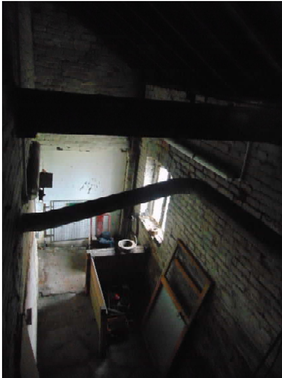
Plate 62: Boiler room in Building D, looking northeast
