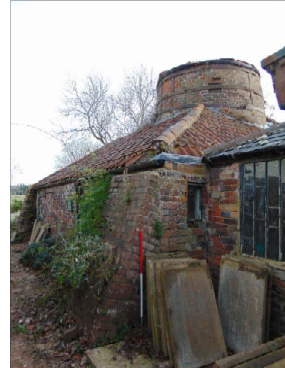
Plate 15: Northwest elevation of Building B, showing modern brick butress at corner, looking northeast [3]
