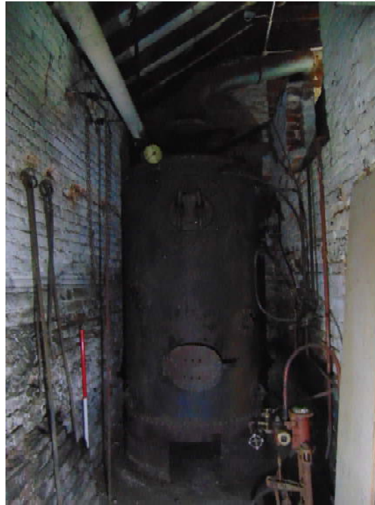
Plate 63: The cross tube upright boiler, looking east
