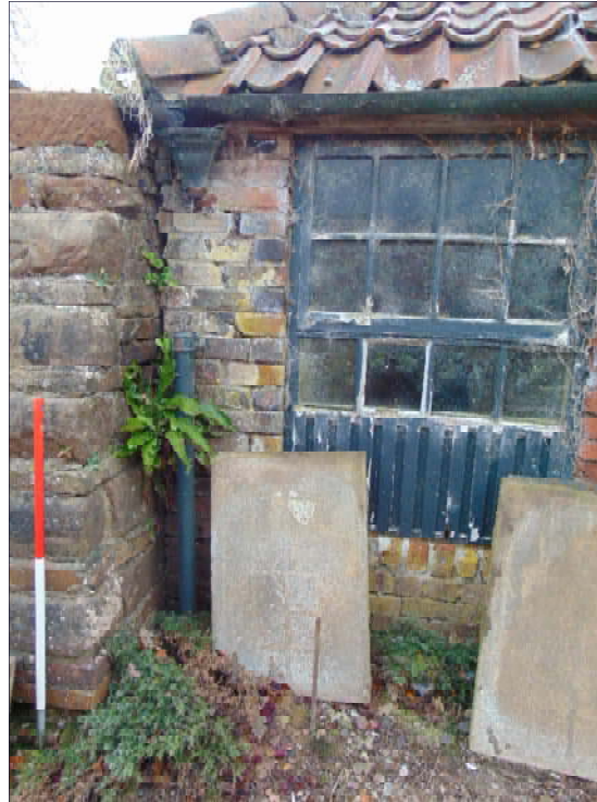
Plate 14: Detail of northwest elevation of Building B, showing later brick wall abutting remnant sandstone wall
