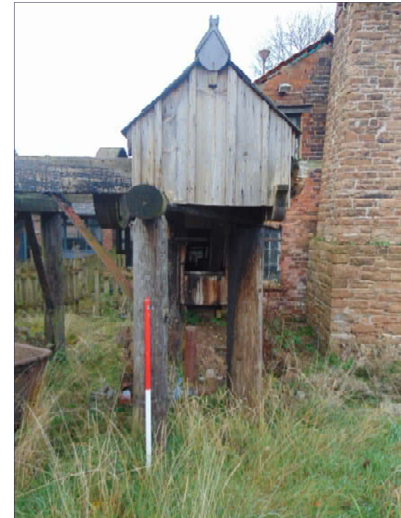
Plate 34: Detail of power transmission belt emerging from southeast elevation of Building D, engine house
