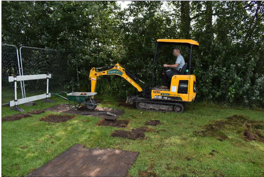
Plate 1: Excavation underway in Area A on the northwest side of the site, looking east
