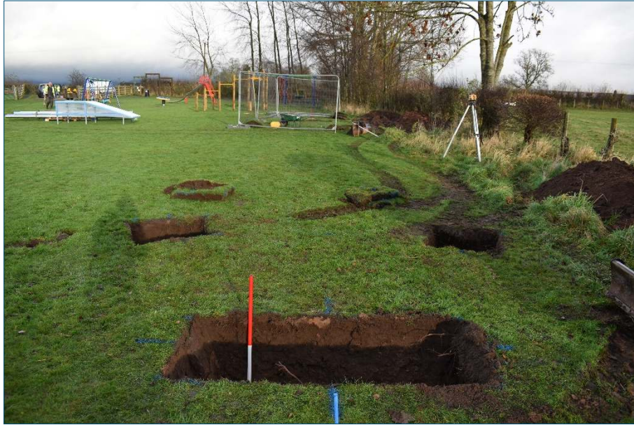
Plate 5: Excavations for the zip wire on the south side of the site, looking northeast (1m scale)
