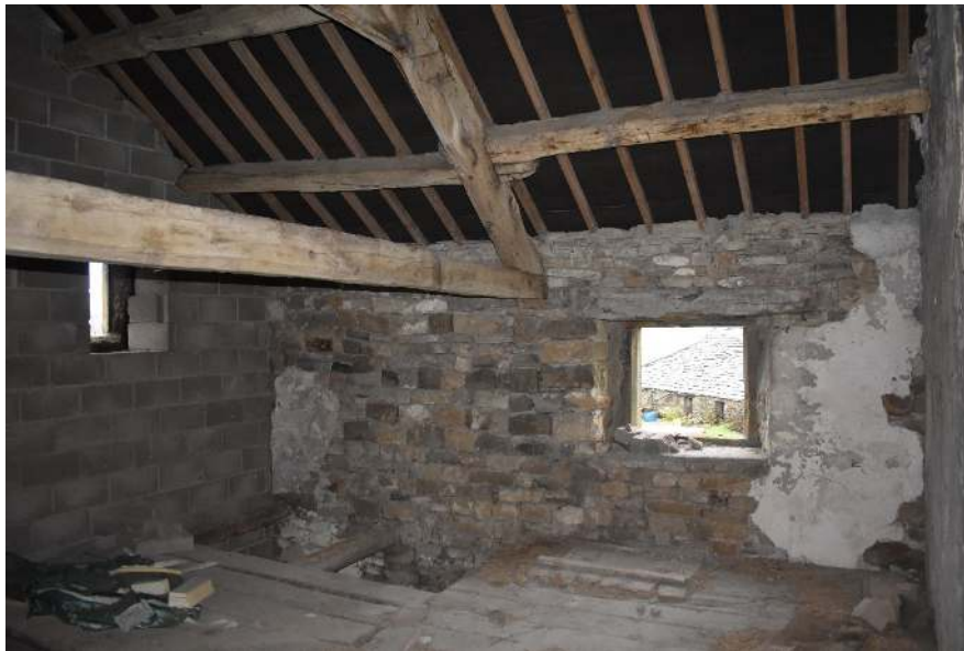
Plate 26: Former mullion window in the northern room on the first floor, looking northeast.
