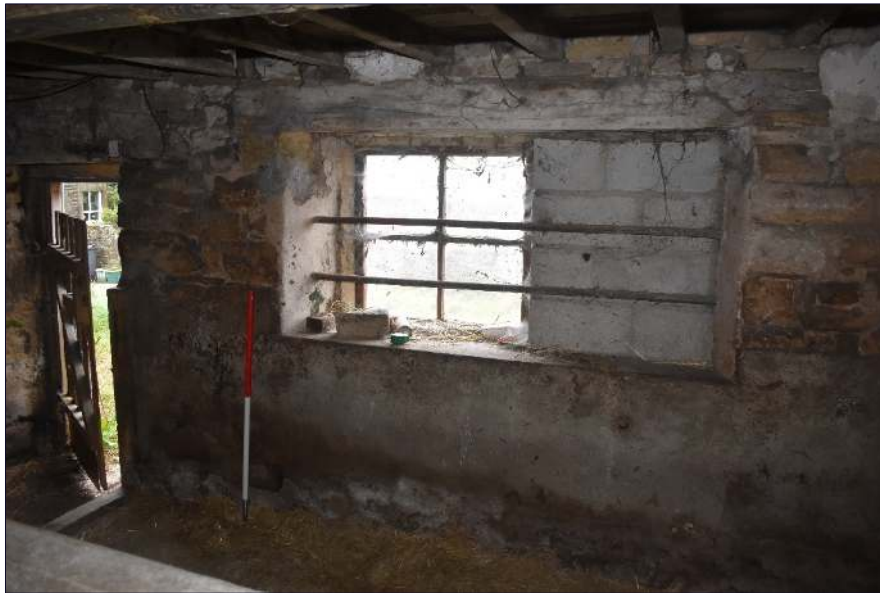
Plate 20: Modified mullion window in the east wall of the central room, looking northeast.
