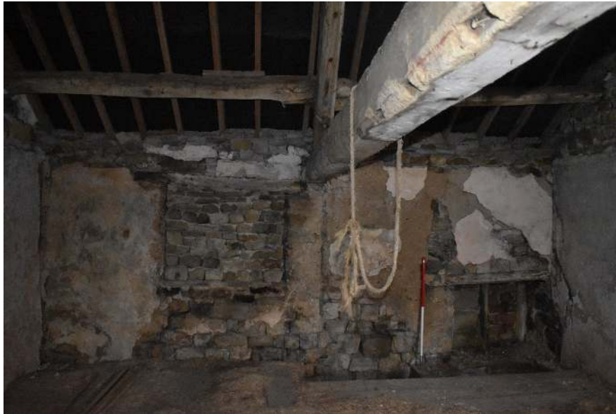
Plate 28: Blocked mullion windows in the central room on the first floor, looking west.
