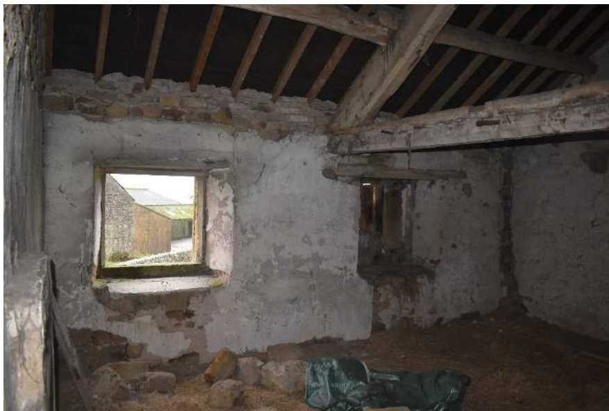
Plate 27: Mullion windows in the central room on the first floor, looking southeast.
