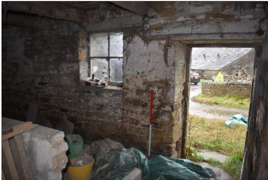
Plate 16: East wall of the northern room showing blocked opening and inserted window, looking northeast.
