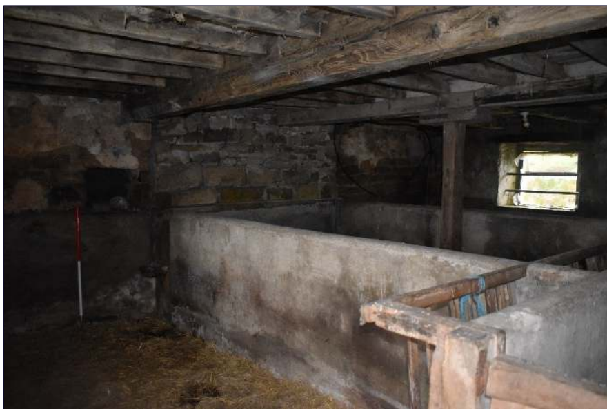
Plate 18: The central room showing concrete partitions and blocked fireplace with niche, looking southwest.
