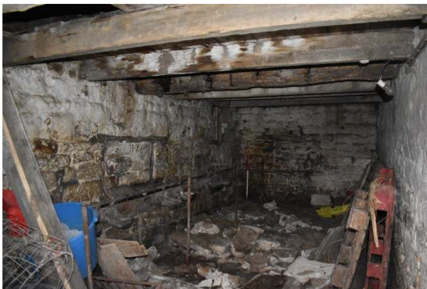
Plate 23: Blocked windows in the southern room on the ground floor, looking southwest.
