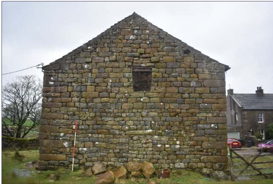
Plate 12: Blocked window with open window above in the south-facing elevation, looking northwest.
