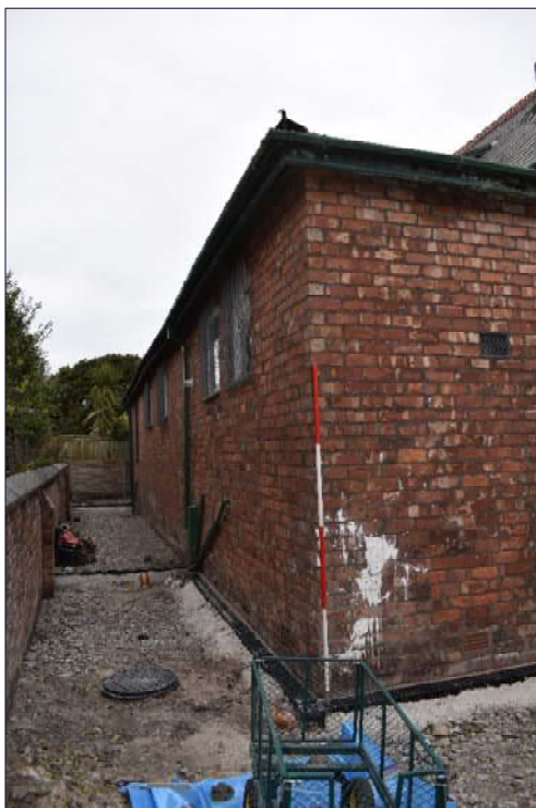
Plate 17: West elevation of the Sunday School building, looking north (1 x 2m scale)
