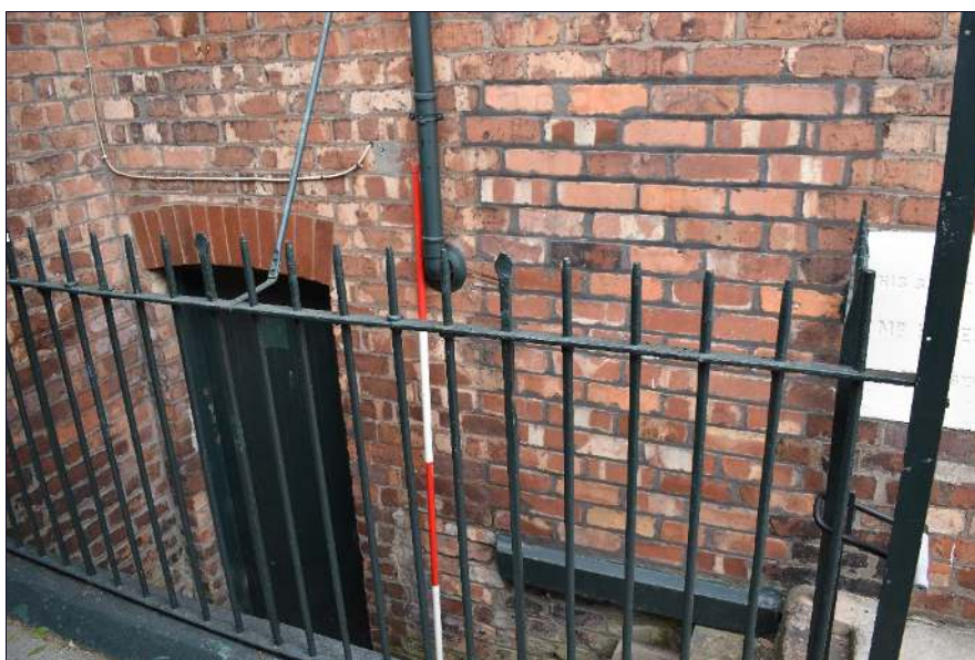
Plate 14: Blocked window and door to basement in south elevation, looking northwest (1 x 2m scale)
