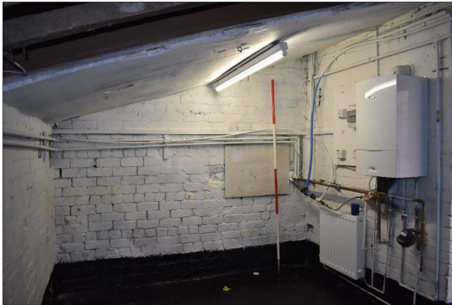
Plate 43: Basement with heating system, looking east (1 x 2m scale)
