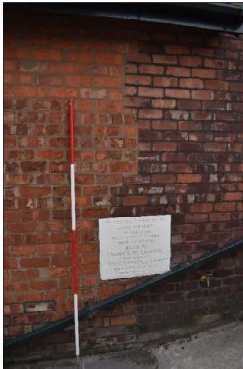
Plate 15: Construction break in the north elevation with commemoration stone, looking south (1 x 2m scale)
