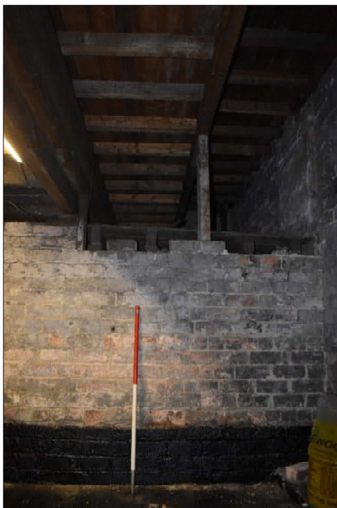
Plate 45: Timber frame supporting the tiered floor in the room above, looking south (1 x 1m scale)
