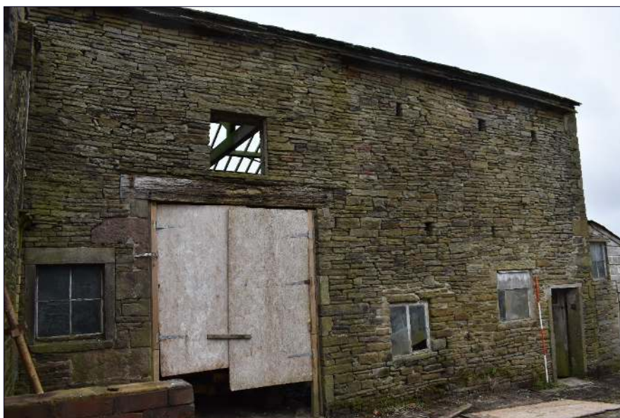
Plate 18: North elevation of the barn (Building B), looking southwest (1 x 2m scale)
