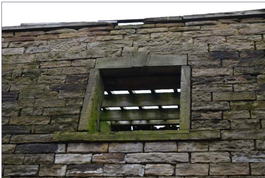
Plate 17: Detail of upper window in the south elevation of the barn (Building B), looking north
