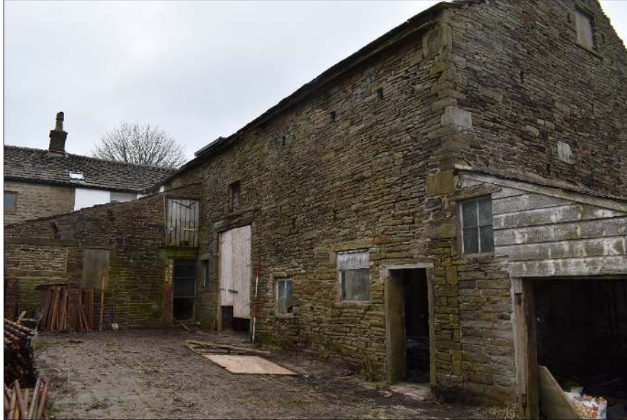
Plate 19: North elevation of the barn (Building B) showing northern extension, looking southeast (1 x 2m scale)
