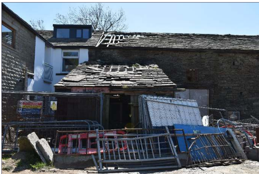
Plate 34: North elevation of the extension (Building D), looking south (taken 24th April 2020)
