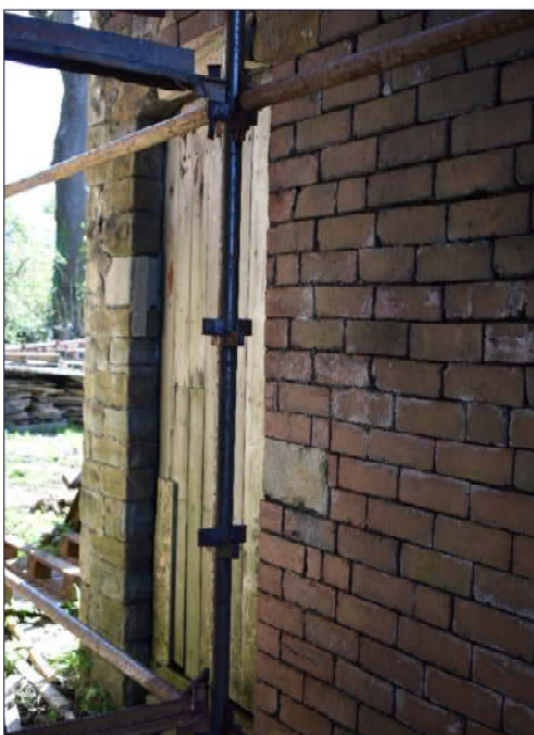
Plate 10: Door in the north elevation of the stable (Building A), looking south (taken 24th April 2020)
