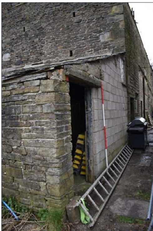
Plate 31: South elevation of the lean-to (Building C), looking east (1 x 2m scale)
