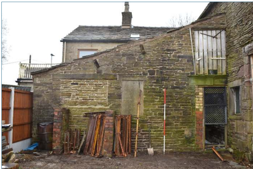
Plate 35: West elevation of the extension (Building D), looking east (1 x 2m scale)
