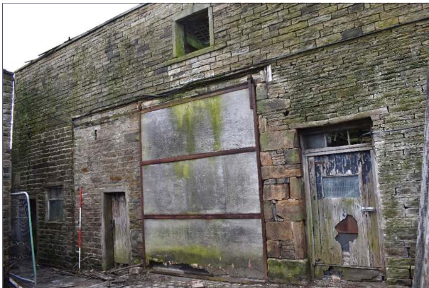
Plate 15: South elevation of the barn (Building B), looking northwest (1 x 2m scale)
