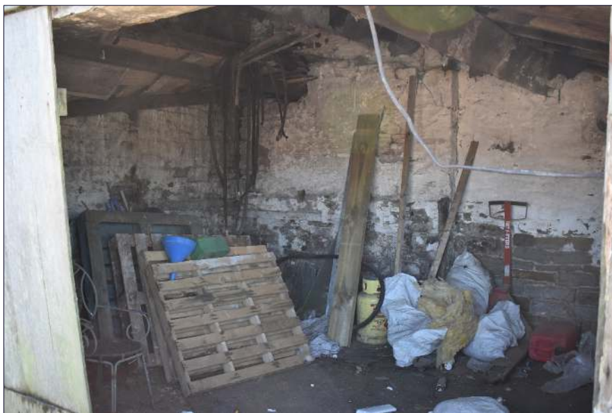
Plate 32: Interior of the north side of the lean-to (Building C), looking south (taken 24th April 2020)
