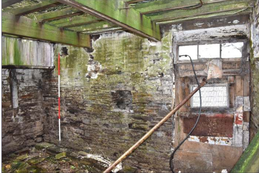
Plate 25: Southeast end of the barn (Building B) showing niche, looking south (1 x 2m scale)
