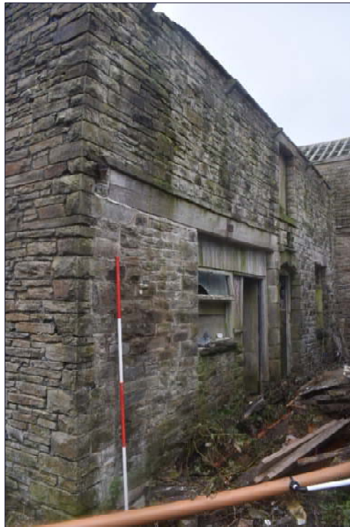
Plate 5: East elevation of the stable (Building A), looking north (1 x 2m scale)
