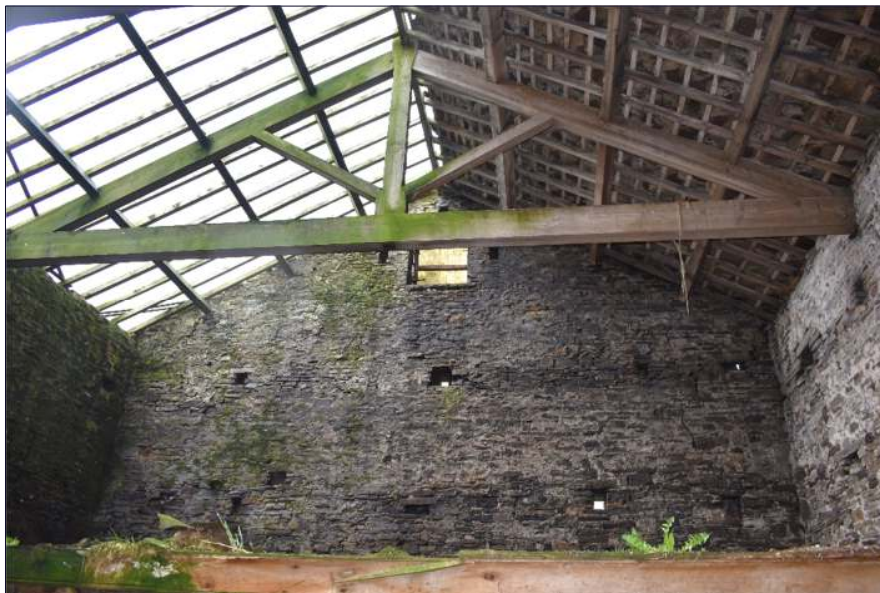
Plate 26: Loft space at the west end of the barn (Building B), looking west
