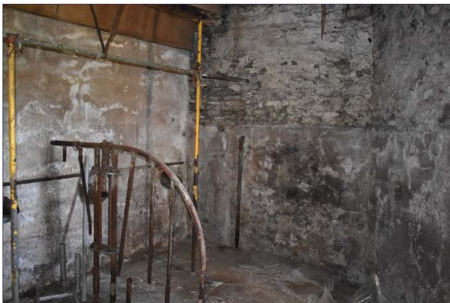
Plate 12: Southwest space in the stable (Building A) showing angled wall, looking south (taken 24th April 2020)
