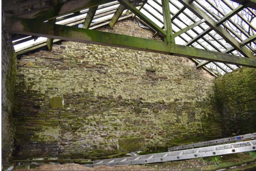
Plate 27: Loft space at the east end of the barn (Building B), looking east
