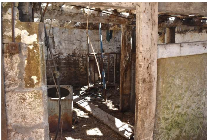
Plate 24: Cattle stalls in the northeast end of the barn (Building B), looking west (taken 24th April 2020)
