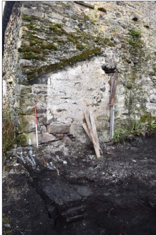
Plate 3: Foundations of the former extension (105) showing building scar and former roofline on the eastern gable of the existing dwelling, looking northeast
