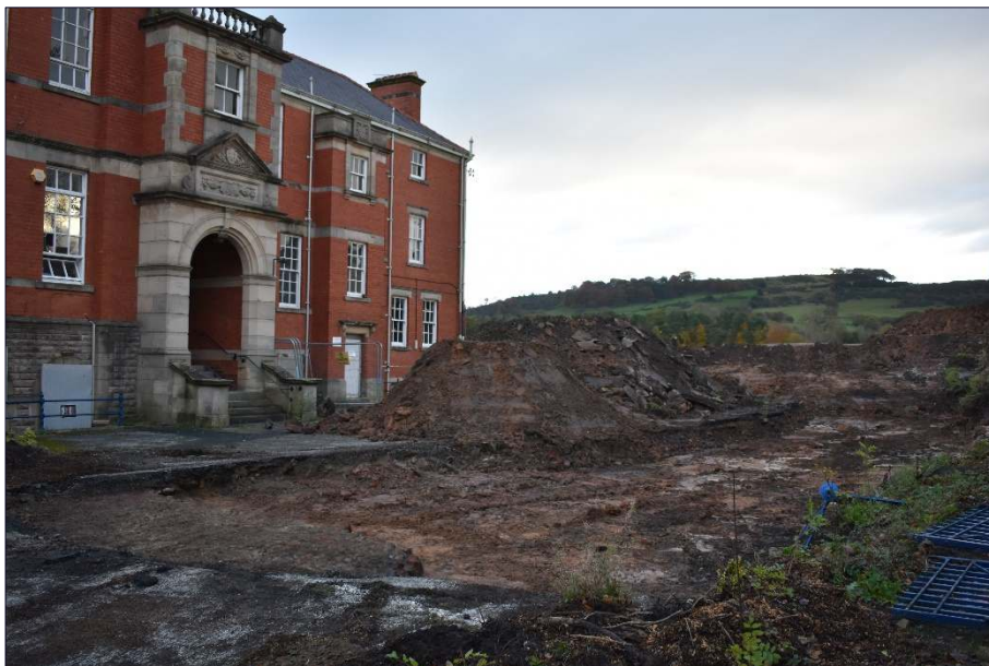
Plate 2: Area excavated for the access road to the south of the main building, looking northeast
