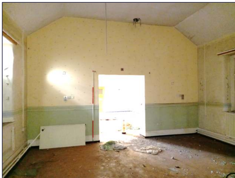
Plate 35: View looking north-west showing the first floor of Block A as seen from the original cottage looking into the brick infill section
