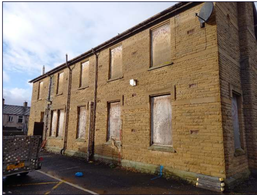
Plate 15: South-east elevation of Cottage 1, Block A, showing the decorative lintels of the windows
