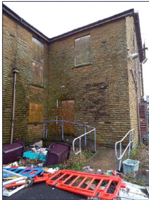
Plate 13: Inserted doorway, north-west facing elevation of Cottage 1, Block A, also showing a blocked window
