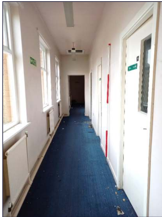
Plate 36: View looking south-west showing the first floor of the brick infill section in Block C, the doors to the right provide access to modern offices
