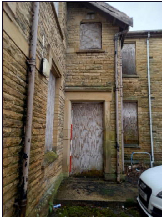
Plate 9: Doorway to Cottage 4, Block C, showing lack of projecting canopy over the door (Scale = 2m)
