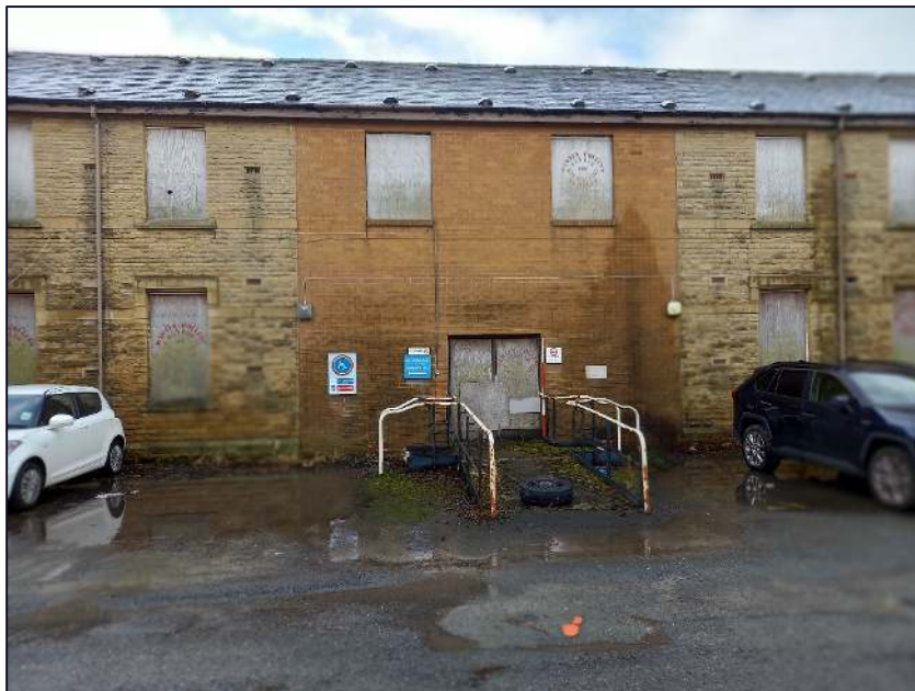
Plate 24: North-east elevation of Block A showing inserted brick infill between Cottages 1 and 2
