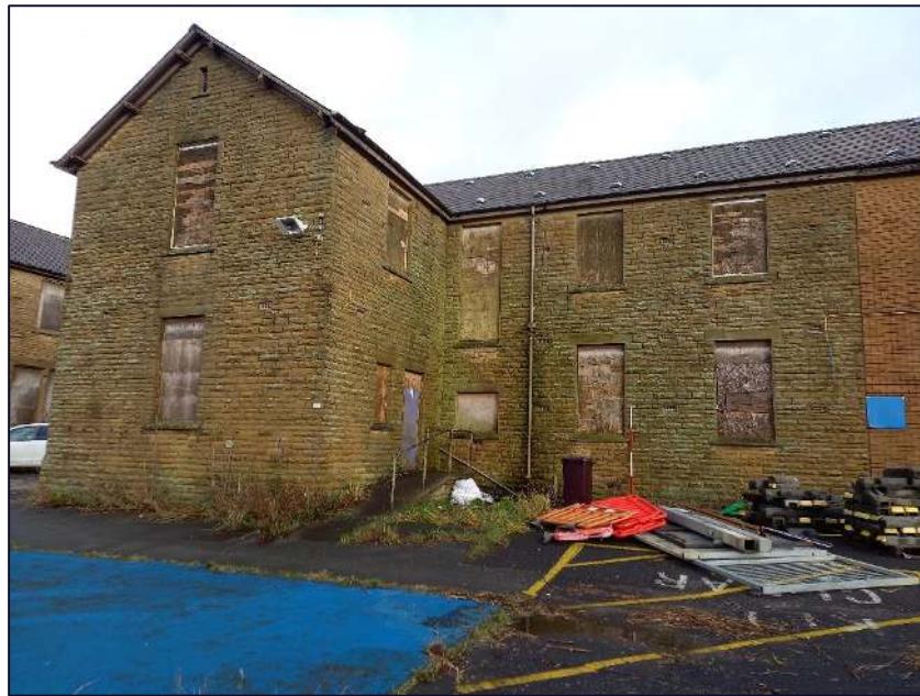
Plate 19: South-west elevations of Cottage 2, Block A, showing the tall first floor window that lit the stairwell
