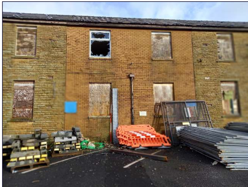
Plate 25: South-west elevation of Block A showing inserted brick infill between Cottages 1 and 2
