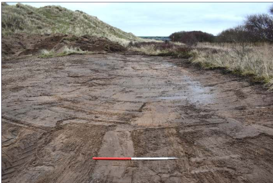
Plate 9: Area excavated for a pond in Area 3 at North Walney, looking east (1m scale)
