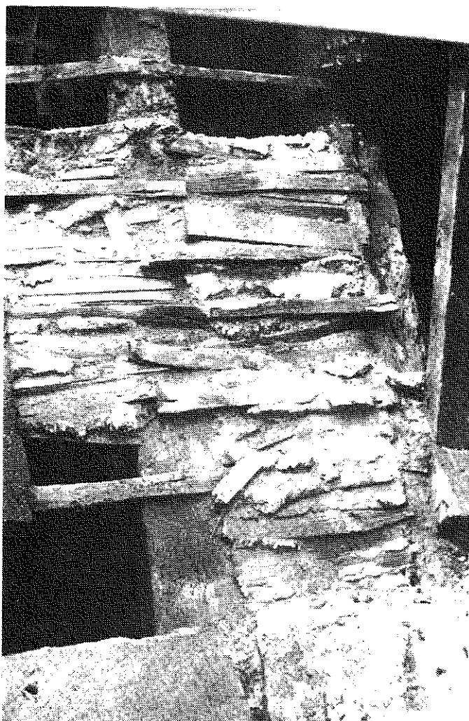
Fig. 1. Original laths, plaster roof and stone slates (removed) revealed during repairs to the roof of the late medieval Charlston Hall (West Yorkshire) in 1987. The absence of another set of lath nail holes shows that the surviving laths are the original ones. The exposed lower backs of the stone tiles were covered with plaster from the plastering between the rafters, forming a kind of ceiling. Similar evidence has been noted on ceramic tiles (photo: S. Moorhouse)
