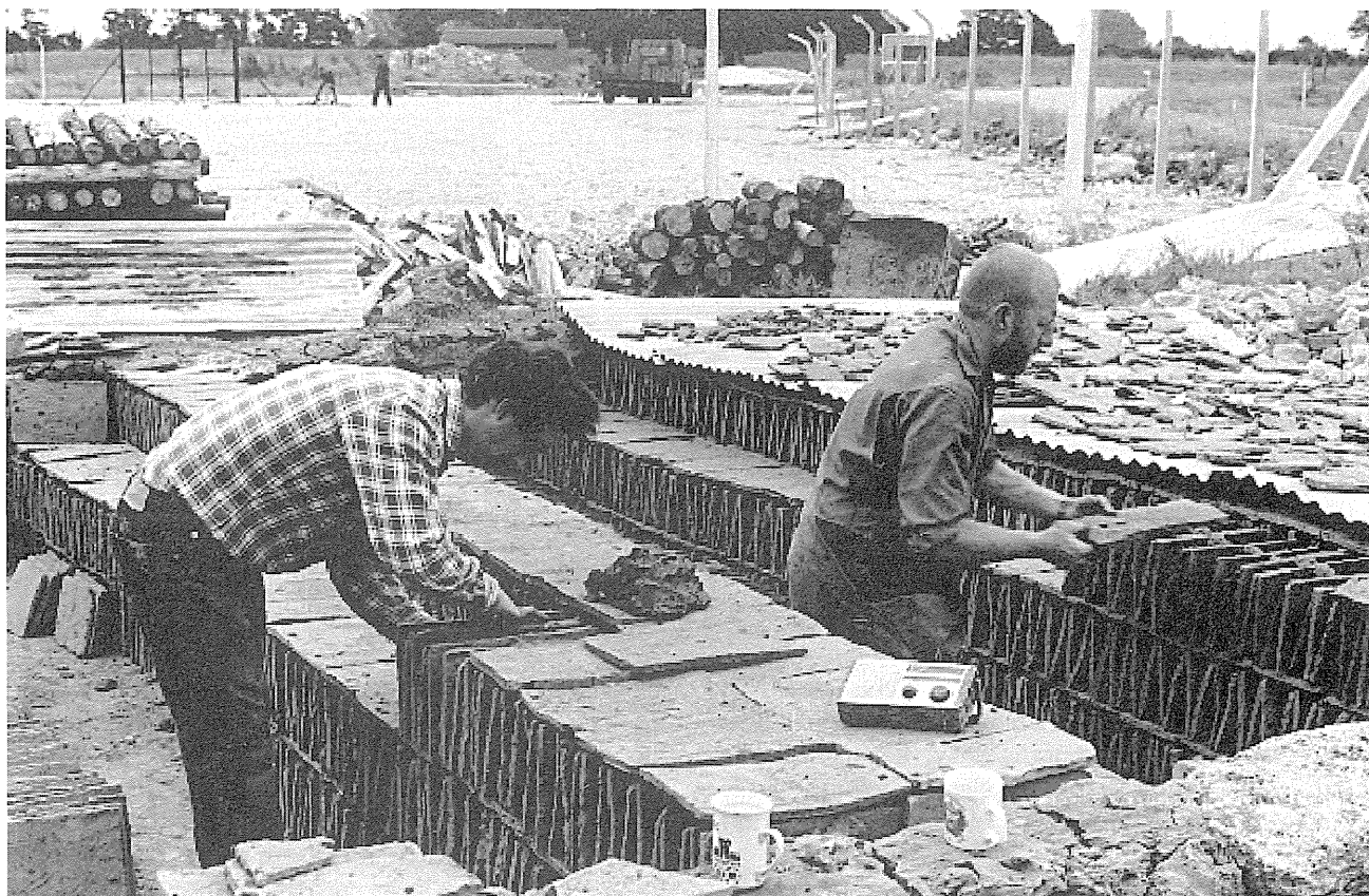
Fig. 8. Phil Dunwell and author packing both the placing areas simultaneously, showing the method of stacking. Photo courtesy of Michael Andrews.
