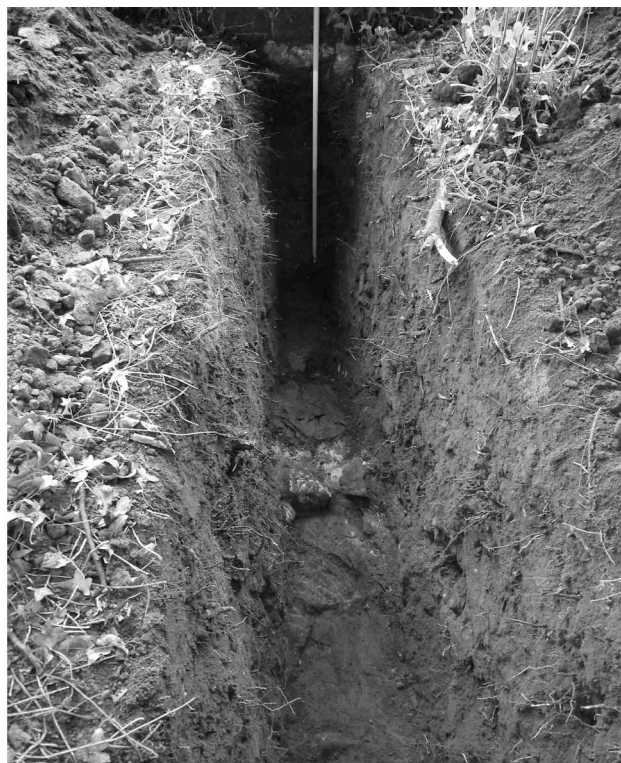
Figure 5 General view of Trench A showing paving 009, wall foundation 008 and paving 007, looking northwest.
