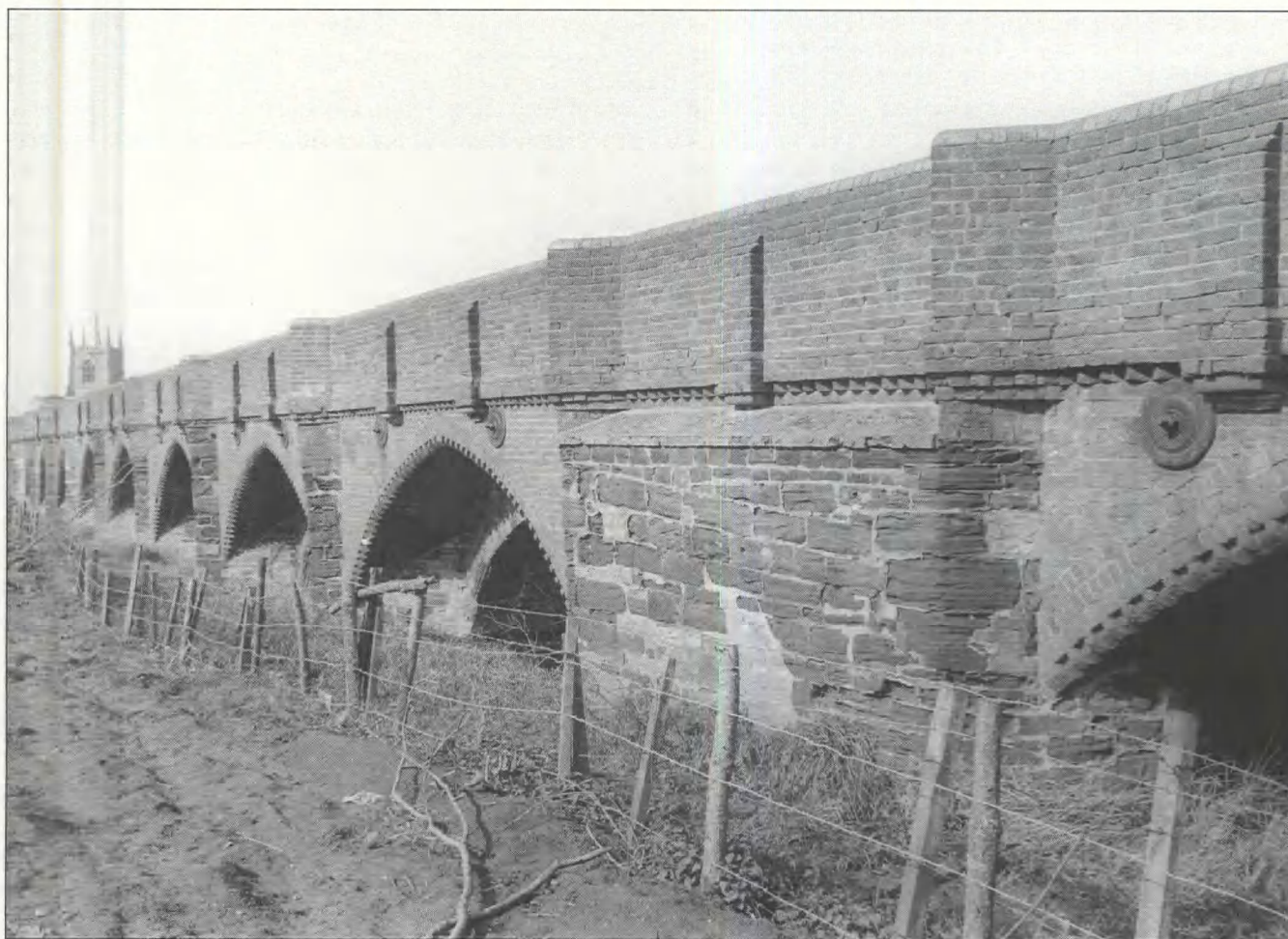
Fig 23 Barford bridge: west face, showing the brick widening of 1873. The sloping courses in the sandstone pier (foreground) mark the south end of phase 2 of the bridge (Beds Photographic Services)
