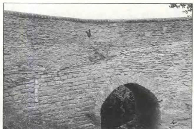
Fig 63 Harrold bridge: east face of river arch 10, showing line of original access ramp on to river bridge (before repair)
