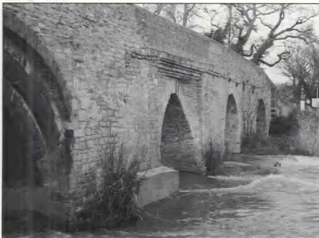
Fig 132 Harrold bridge: east face of arch 12, showing distortion of arch ring
