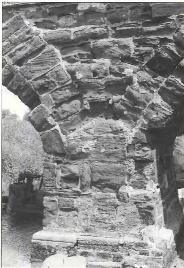
Fig 137 Sutton bridge: fine joints in stonework, with later pointing (before repair in 1986)
