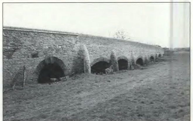
Fig 69 Harrold bridge: west face of flood arches, showing 1857 widening (arch 7 in the foreground was rebuilt in 1893)
