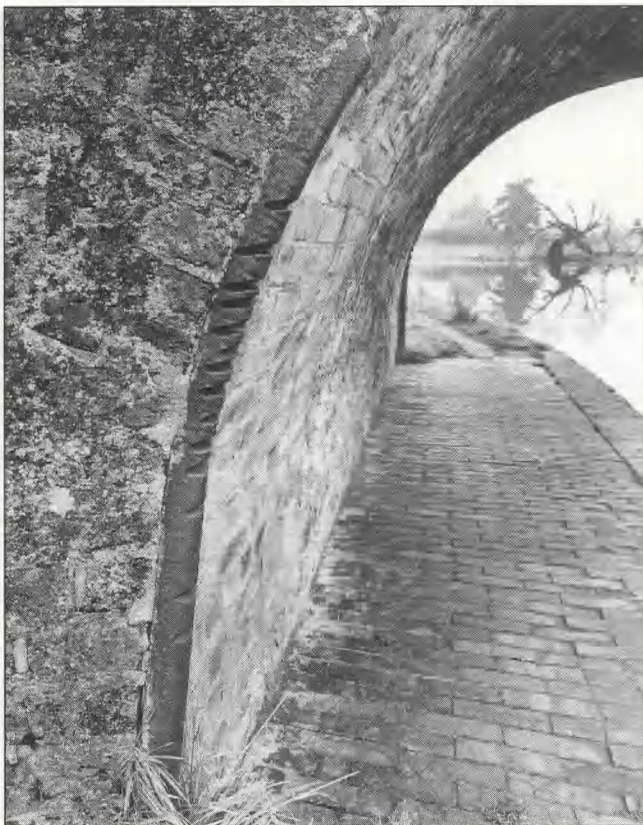
Fig 125 Sandhole canal bridge: iron guard at north-east quoin, grooves worn by tow ropes (Beds Photographic Services)
