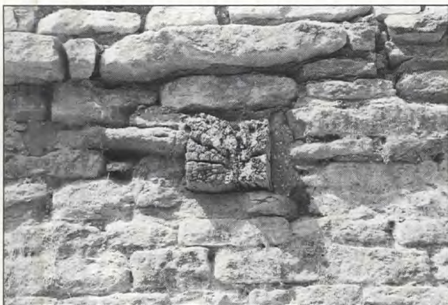
Fig 70 Harrold bridge: remains of timber joist from railing, east face of bridge
