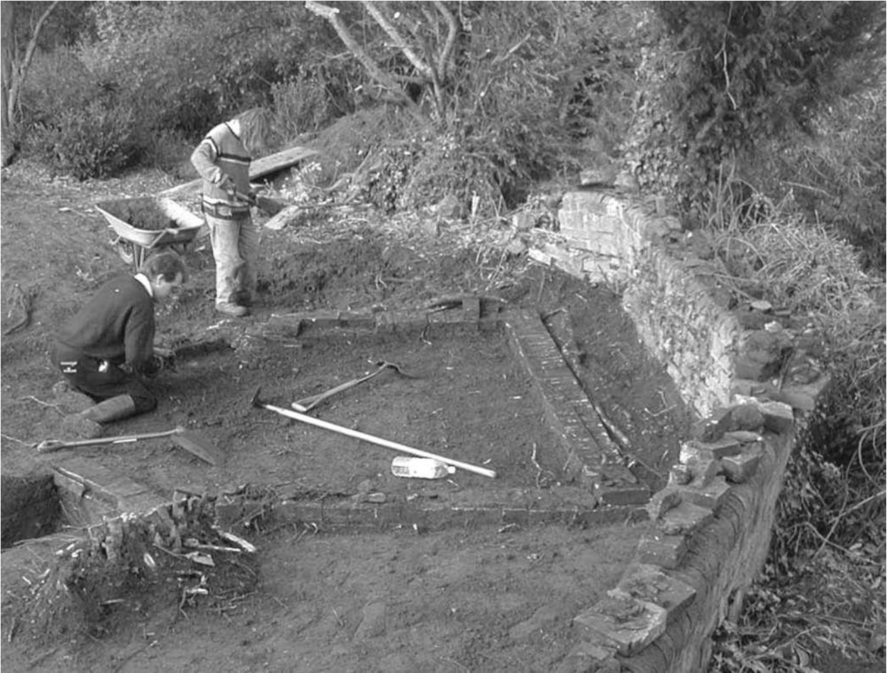
Fig. 6.3 Discovery of an internal wooden building within the early 19 th century aviary at Swiss Garden, Old Warden (© Albion Archaeology).
