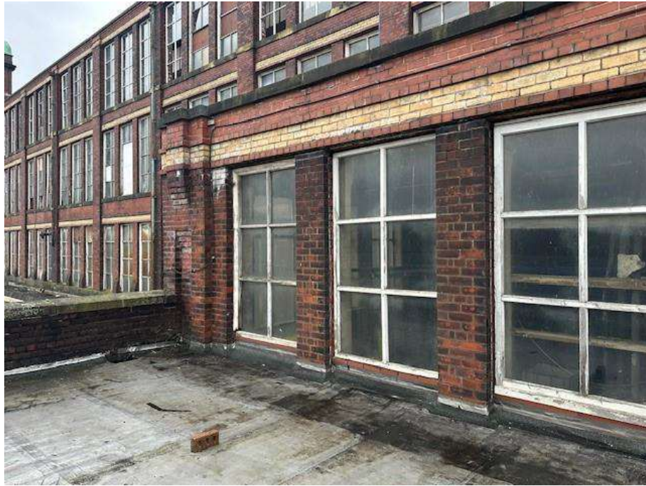
Plate 26: East end of northwest elevation of Building 5a. View looking east from roof of Building 5b
