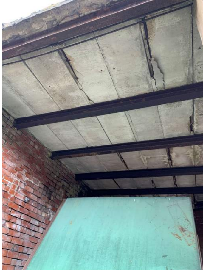
Plate 14: Ceiling and unattached door in Building 2. View looking northeast from exterior
