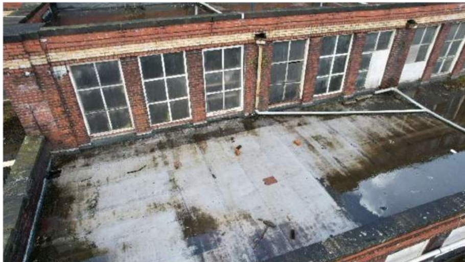
Plate 27: Roof deck of Building 5b with northwest elevation of Building 5a. View looking southeast from roof of adjacent extension
