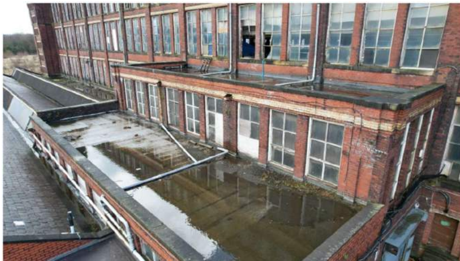
Plate 25: Deck of Building 5b and northwest elevation of Building 5a. View looking southeast from roof of adjacent extension
