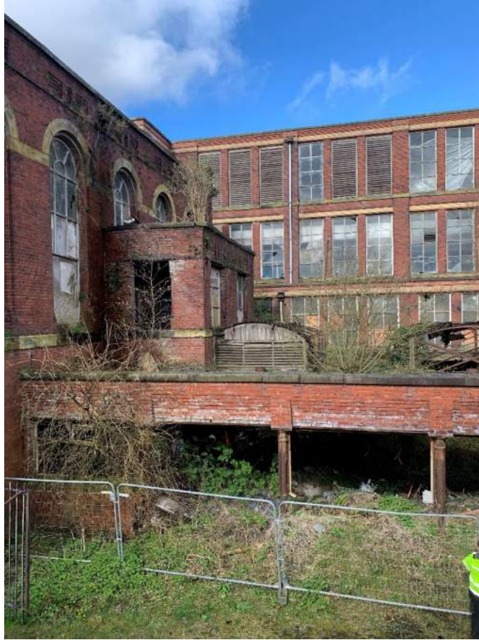
Plate 23: Southeast and northeast elevation of Building 4 which sits atop of Building 3. View looking west
