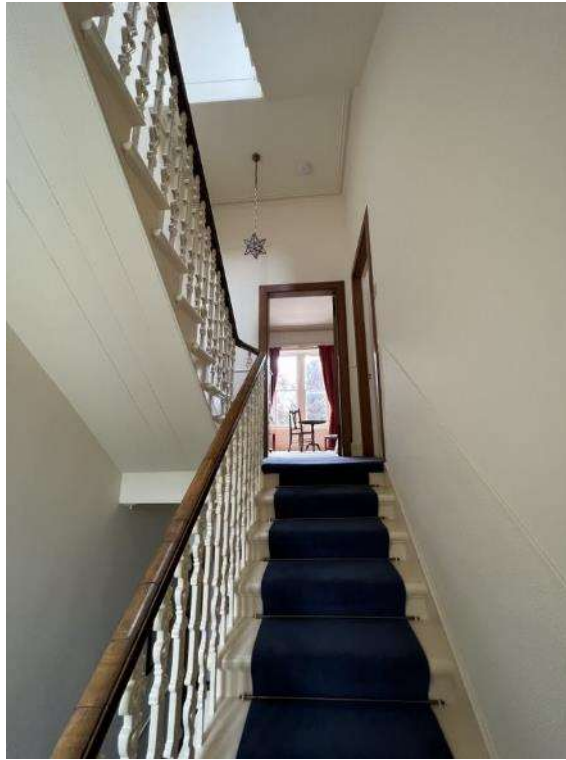
Plate 10: Victorian balustrade. Looking west from landing between ground and first floors (RKA Architectural Design)
