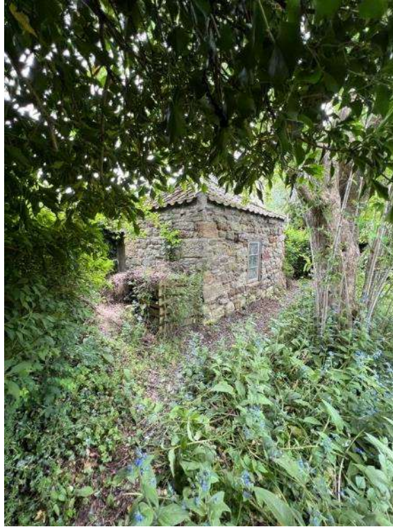
Plate 16: North and east elevations of the potting shed, looking southwest (RKA Architectural Design)
