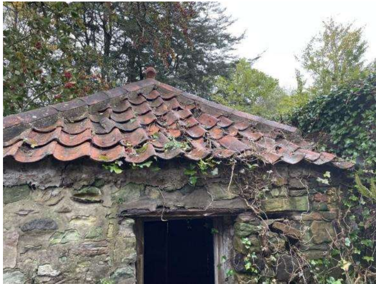
Plate 17: West side of roof of potting shed, looking east from garden (RKA Architectural Design)
