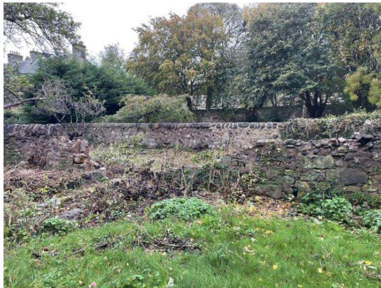
Plate 14: Central rigg wall with eastern rigg wall behind, looking east from garden (RKA Architectural Design)
