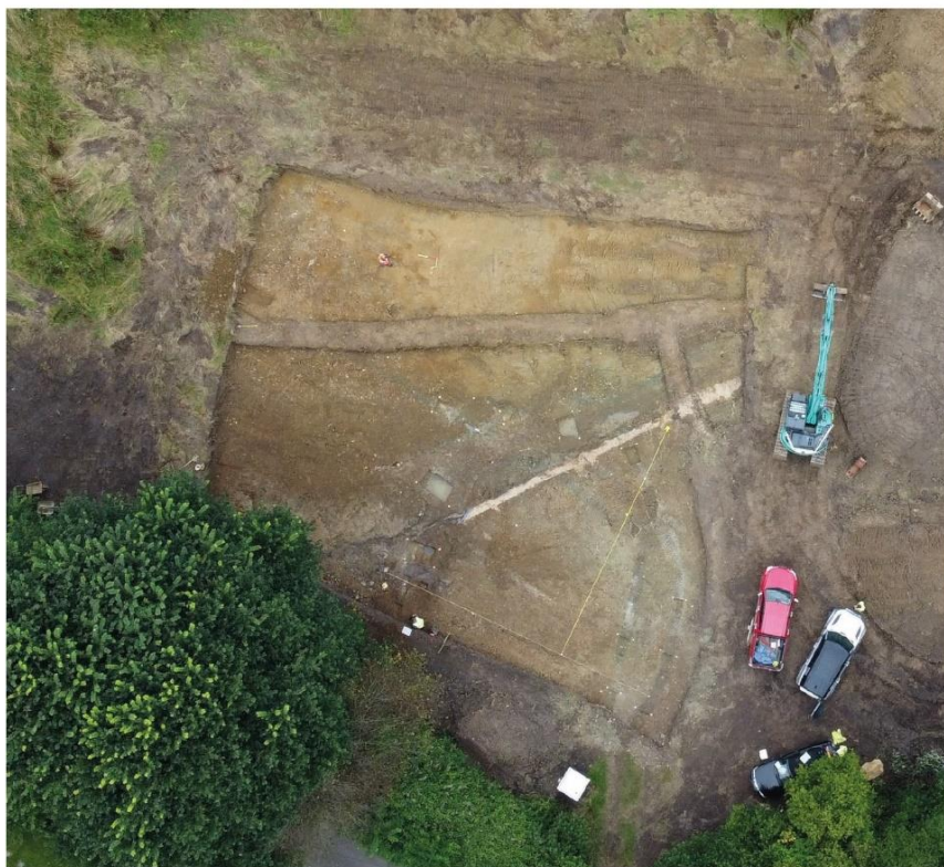
Aerial view of Excavation Area. View to the northwest. (Photograph courtesy of Churchwood Construction)
