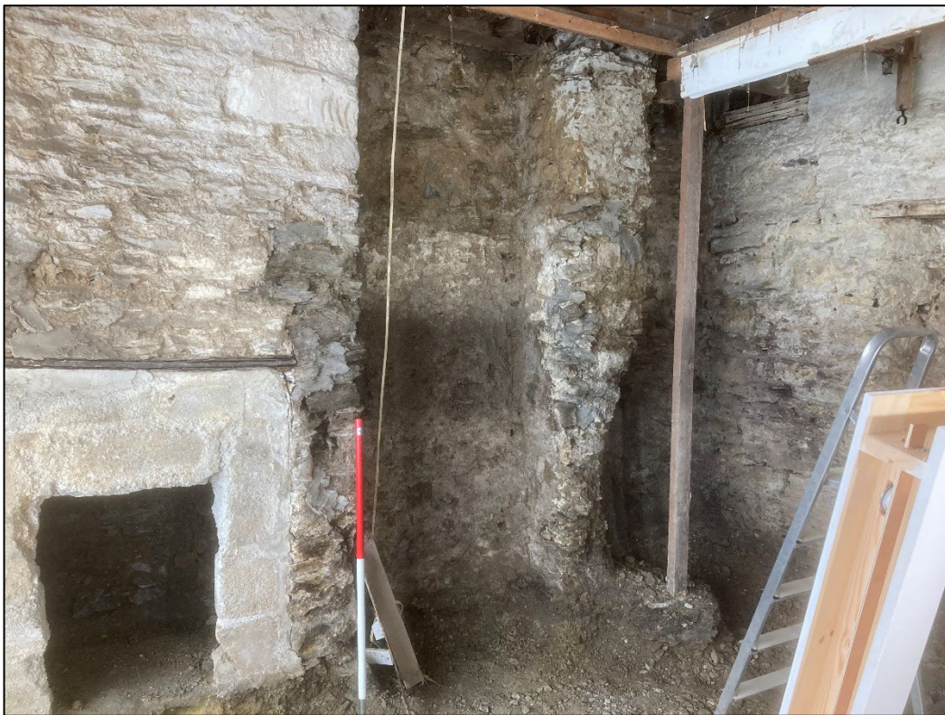
Figure 15: Truncated wall on the northern part of the western wall indicating the location of a historic subdivision. View to the northwest
