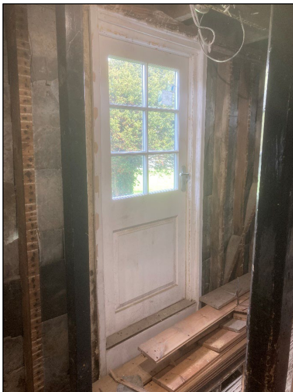
Figure 18: Door on the northern wall eastern side which once served a timber balcony overlooking the churchyard. View to the northeast
