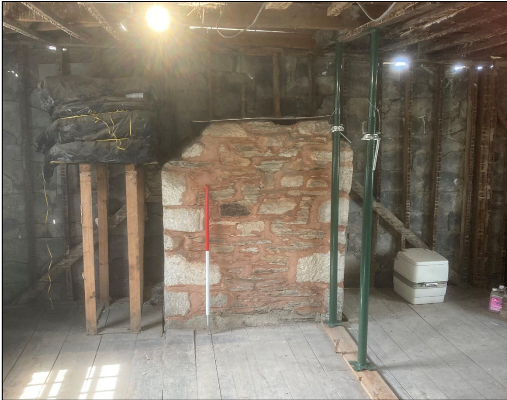
Figure 21: Continuation of the western flue stack. Slate cladding is visible on the buildings western wall. View to the west
