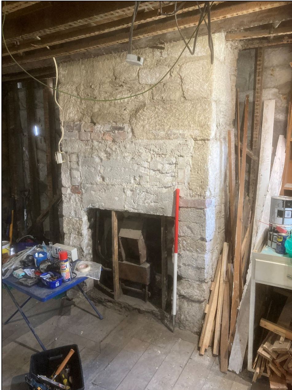
Figure 19: The continuation of the ground floor fireplace stack on the western wall. The stack appears to have been rebuilt from the first floor upwards. View to the southwest
