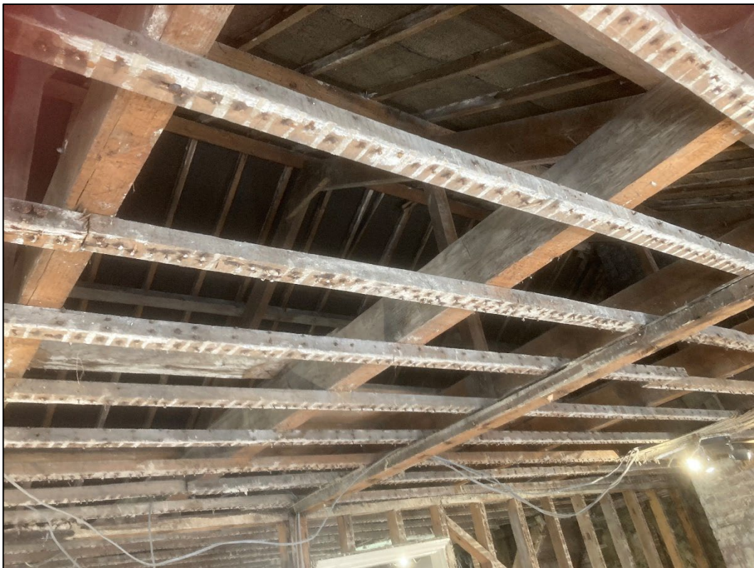
Figure 20: The roof space constructed of queen post trusses with lapped collars. View to the northeast
