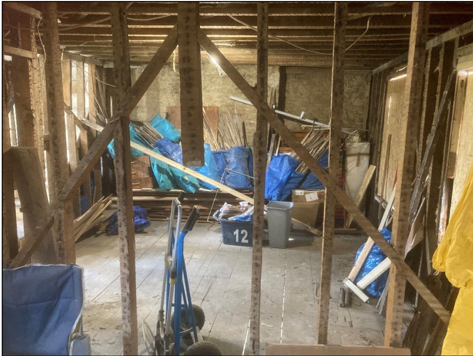
Figure 17: Internal subdivisions on the first floor are of timber stud. Their fibreglass boards have been removed. View to the east
