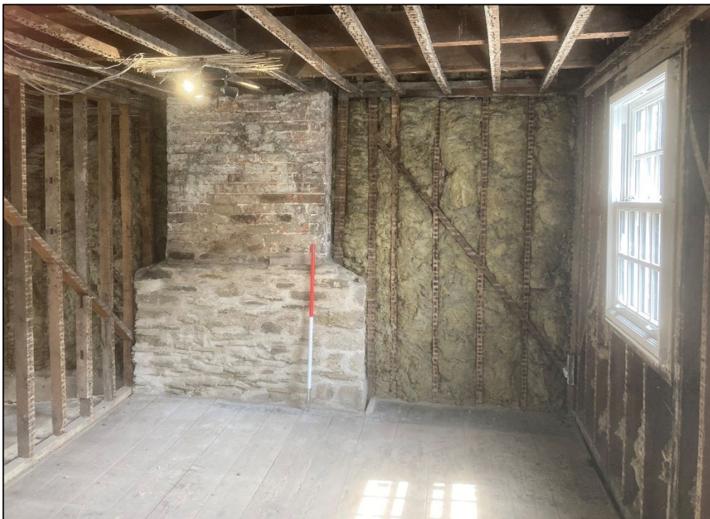
Figure 22: Continuation of the eastern flue stack along the eastern wall. View to the east
