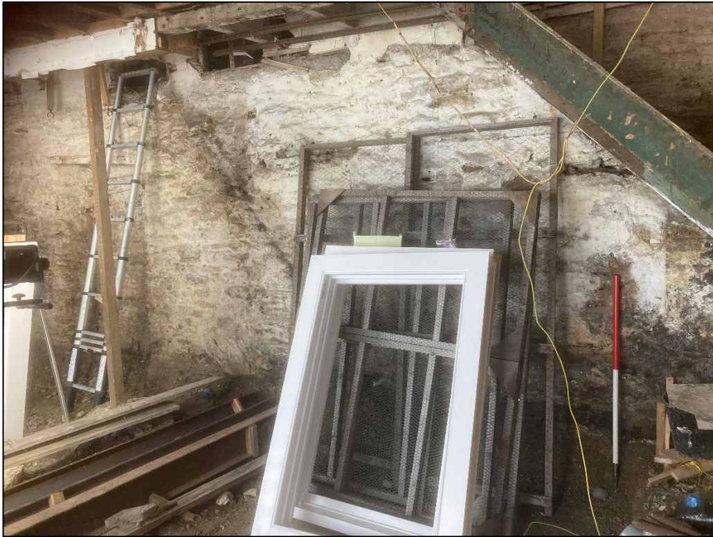
Figure 10: Internal photograph of the northern elevation. The wall is constructed of local killas stone and largely retains a limewashed face. View to the north
