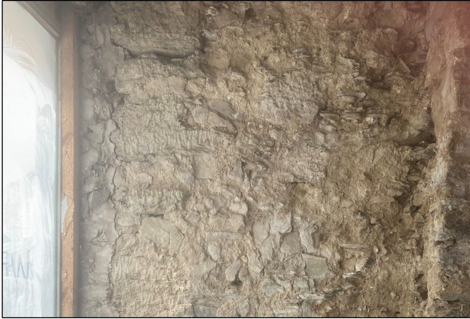
Figure 6: Photograph demonstrating the truncation of the historic western elevation. The truncation occurs where the wall meets the modern shop front. View to the west
