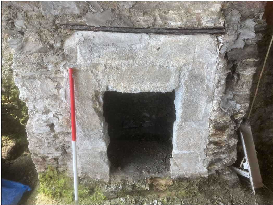
Figure 11: The fireplace stack and flue on the building's western wall. View to the west
