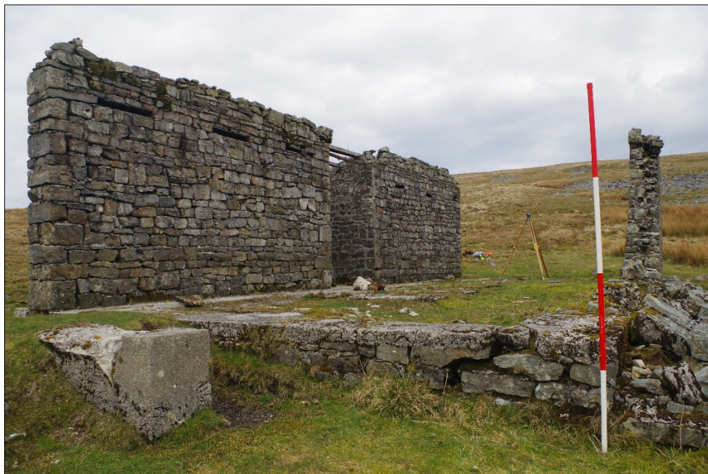
Plate 16: the Brake House, facing north; the collapsed wall is on the right of the picture, and the wall appears to abut the floor slab at this point. One of the external mounting blocks is visible to the left.
