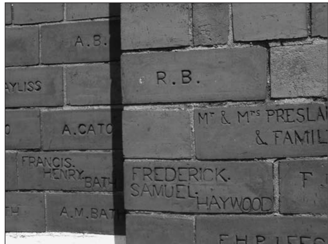
Some of the many names to be seen in the brickwork on the front of the Wesleyan Reform Church, New Swannington.
