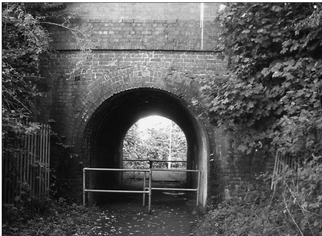
Remains of Ogilvy's route from Prior Park, Ashby, under the Leicester-Burton railway.
