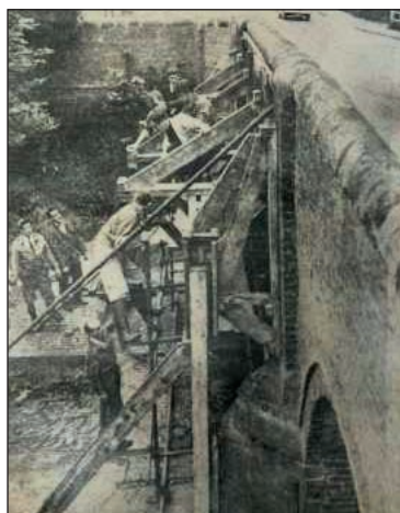
Bridge work, Rugby Road, Lutterworth. (Reproduced by permission of the Record Office for Leicestershire, Leicester and Rutland.)
