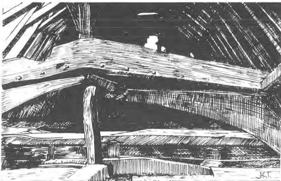
Fig. 3 The roof of Wooburn D'Eyncourt manor house, after a photograph by A. S. Kerry.
